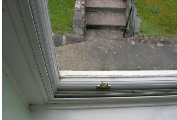
Fig. 4: Secondary glazing added to the interior side of the existing window in the stairwell
