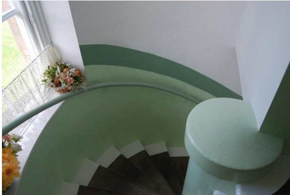
Fig. 3: The stairwell post intervention - aerogel blanket with lime plaster and clay paint finish. The secondary glazing is also visible on the window.
