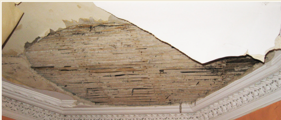
Fig. 12 Collapse can be caused by loss of bond between coats, structural movement and the effects of long term penetrating dampness.
