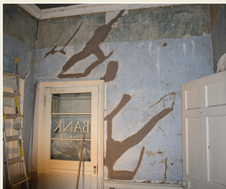
Fig. 14 First coat of coarse plaster for patch repair. (photo credit: Darren McLean)
