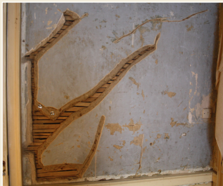
Fig. 13 Loose plaster removed from cracked section of plasterwork. (photo credit: Darren McLean)
