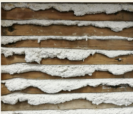
Fig. 9 Plaster nibs or rivets formed on the back side of the lath.
