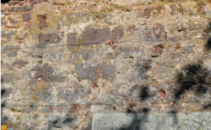
Fig. 1 Flush lime pointing on a wall in southern Scotland dating from approximately 1790.
