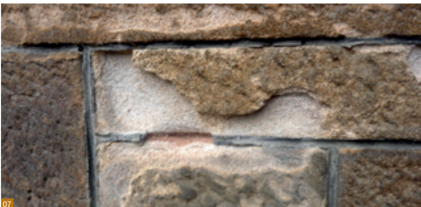
Fig. 7 Cement mortar causing accelerated deterioration of sandstone.
