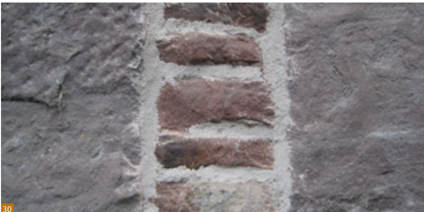
Fig. 30 Poorly replicated ladder pinning.
