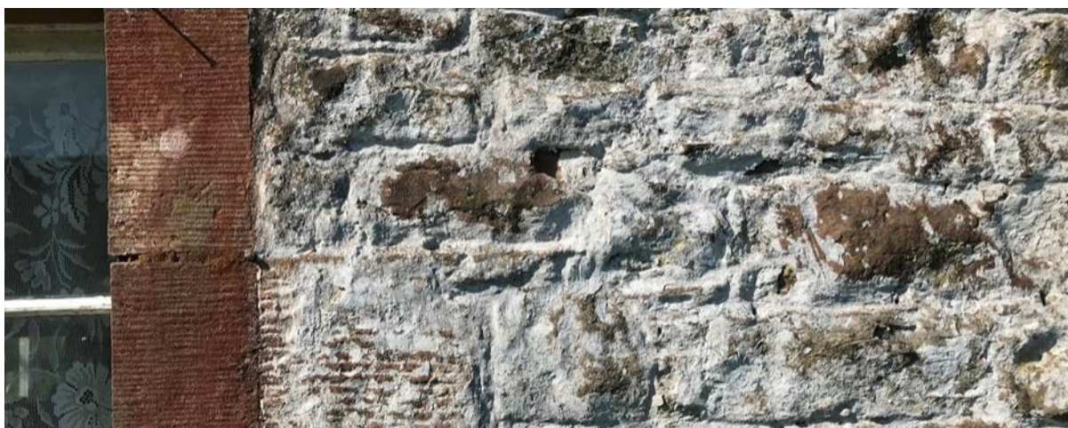
Figure 089.2. Detail of the pointing and limewash at Grange Cottage. The limewash appears to be a single coat.
