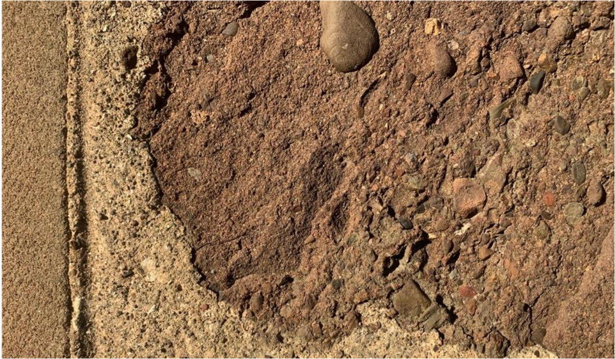
Figure 020.2. Agglomerate stone. Note the vertical lining at the junction with the jamb.
