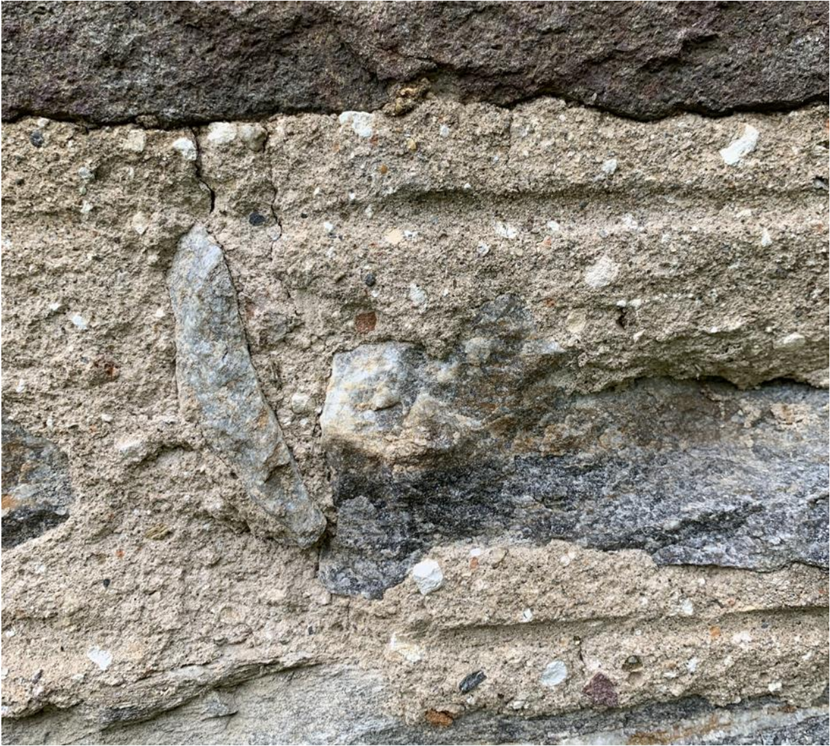
Figure 118.2. A close-up view of the flush point pointing, showing the horizontal ruling out.
