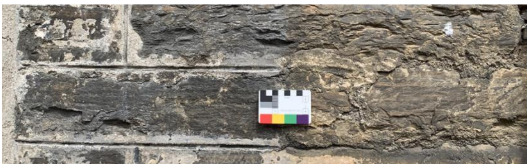
Figure 014.2. A close up of the elevation at the junction of the two buildings, showing the rougher finish to the right, and the more formal work, lined out and whitened, to the left.
