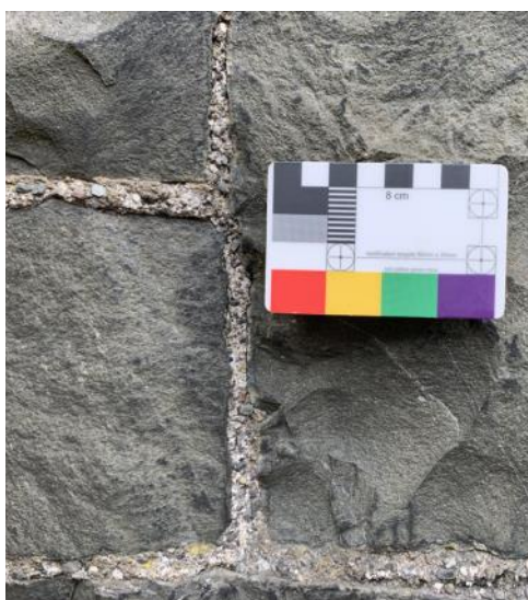
Figure 096.2. Mortar with coarse aggregate and some hints of lining out.
