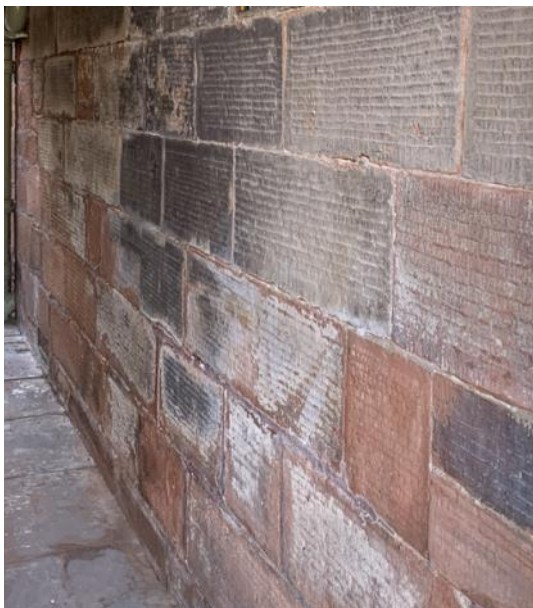
Figure 094.3. The close to the left of the hotel, showing signs of original masonry finishes.
