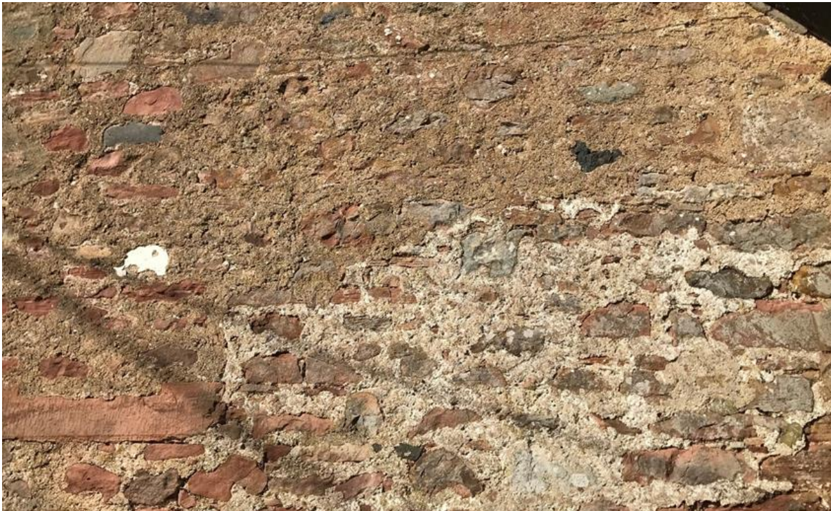
Figure 007.2. Wall finish from the 18th century showing as a whiter flush point, with a similar mortar finish from the 1906 work.
