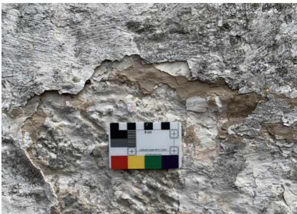
Figure 032.2. Multiple layers of limewash.
