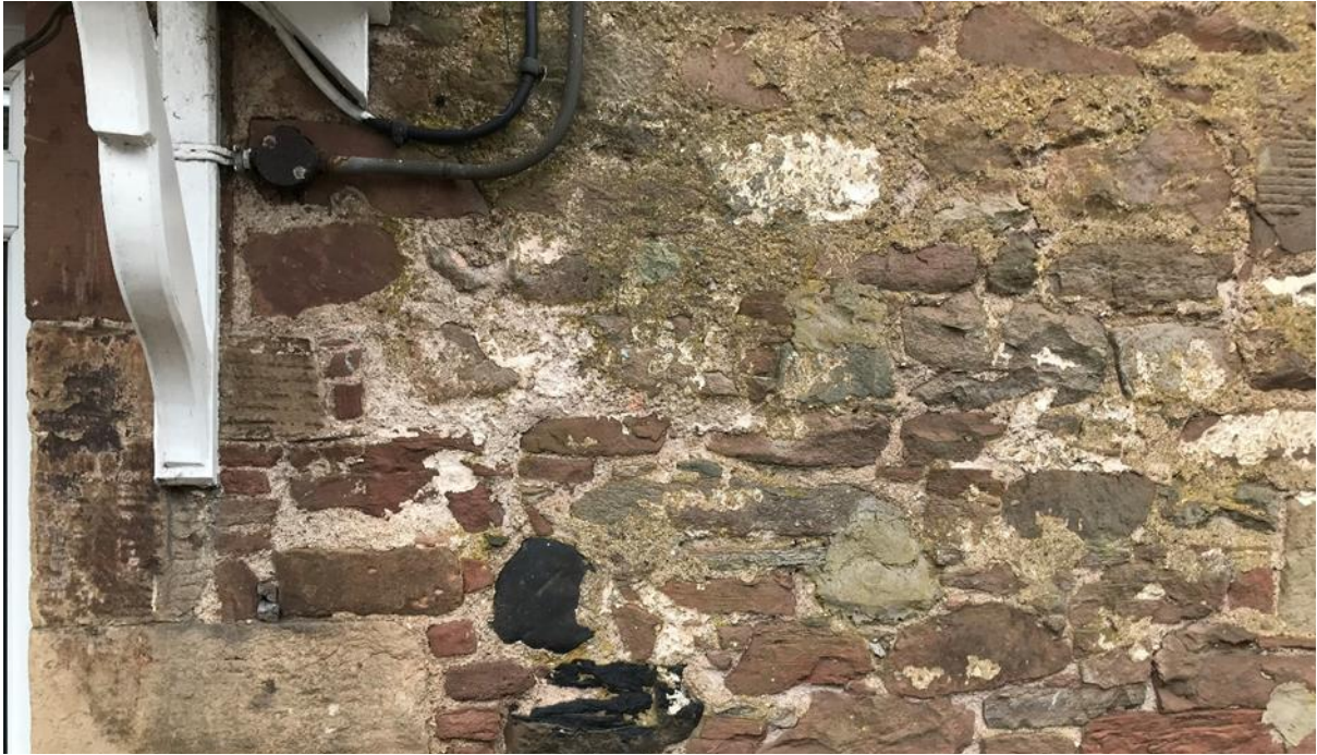
Figure 036.2. A close up of the original cottage wall at ground floor level, showing flush pointing and layers of limewash.
