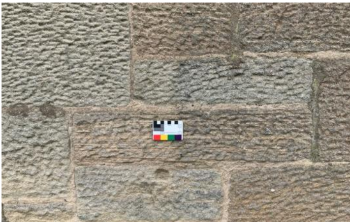
Figure 123.2. The stugged block on the main elevation showing an unmarked flush point.
