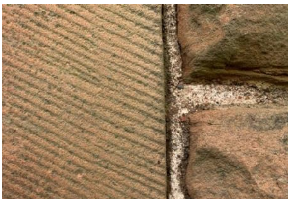
Figure 127.2. The worn back lime mortar as seen on most of the building.
