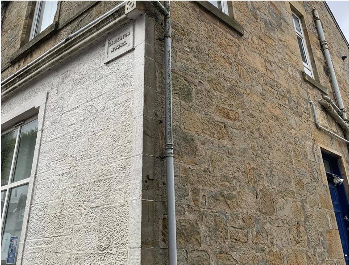
Figure 103.1. Corner of what is now the Semple Centre in Fairlie, showing broad ruled flush pointing to the gable.
