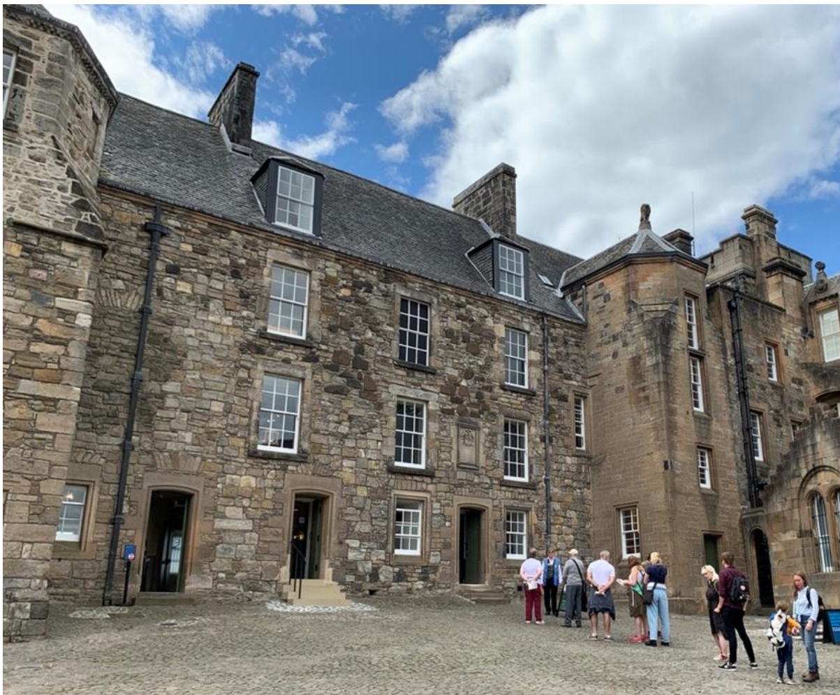
Figure 001.1. The Kings Old Building, Stirling Castle. To the right is the 19th century repair work.
