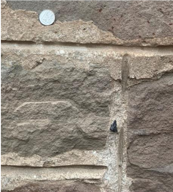
Figure 044.2. Flush pointed with half round informal ruling out. Possible integrated mortar and lime inclusion visible.
