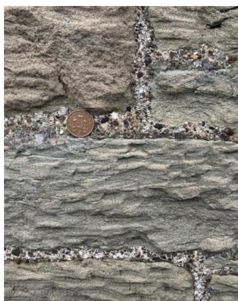
Figure 088.3. Very coarse mortar with large, rounded aggregate.
