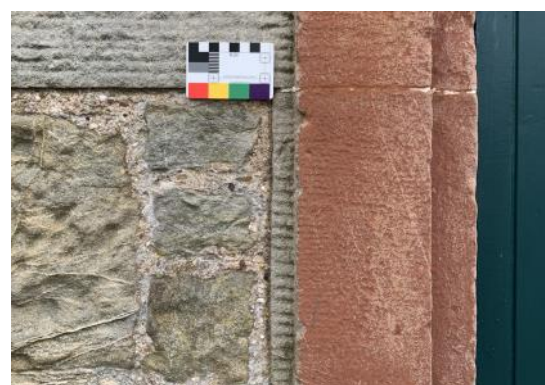
Figure 124.3. Detail of red wash with the sandstone and pointing, also showing the aggregate, coal and lime inclusions.
