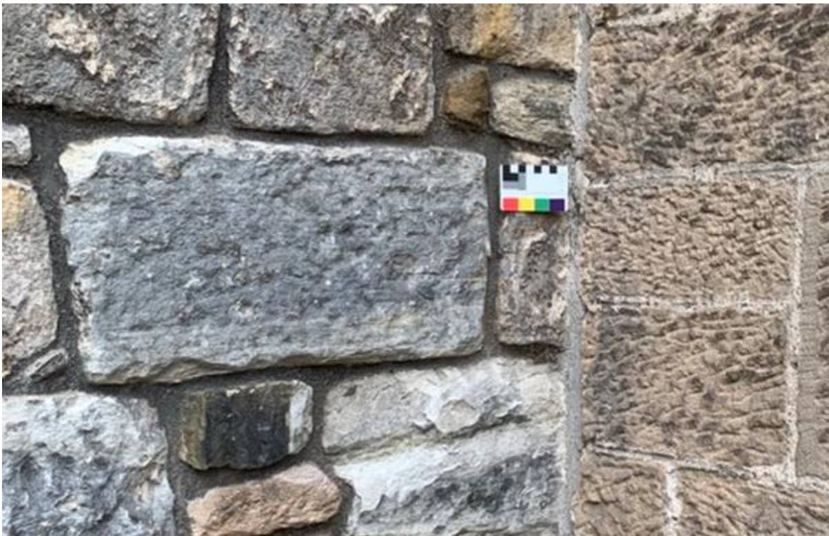
Figure 001.3. 20th century recessed pointing on the 15th century masonry of the Kings Old Building. To the right is 19th century masonry and lined out pointing; work done following the fire.
