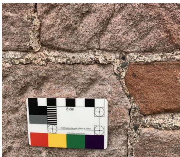
Figure 095.2. The lime rich mortar with large aggregate showing. The angle of the pointing, called 'weather struck', can be seen.
