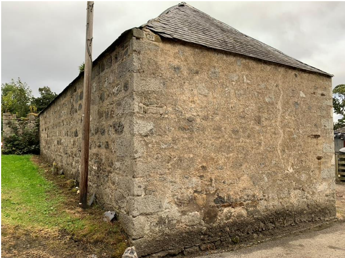
Figure 024.3. The front and rear of the building pointed while the gables are harled.
