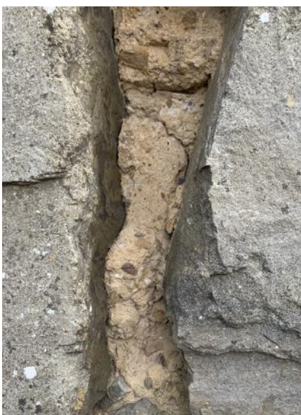
Figure 015.2. Historic earth/lime bedding mortar, showing the coarse aggregate.
