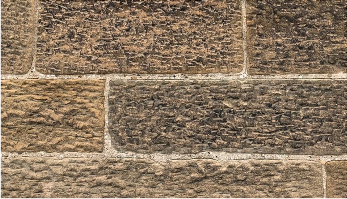
Figure 079.2. Fine lined out joints with gritty mortar.
