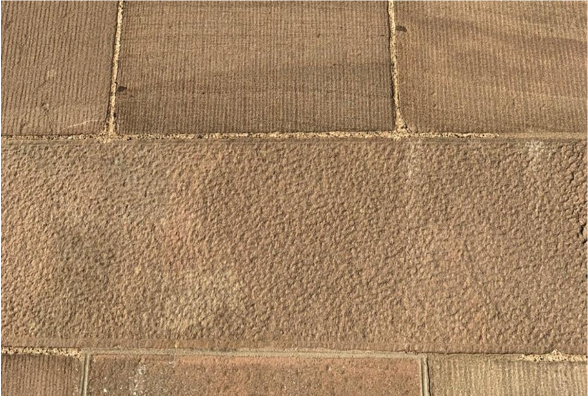
Figure 114.2. The ashlar work with traces of a lined out joint.
