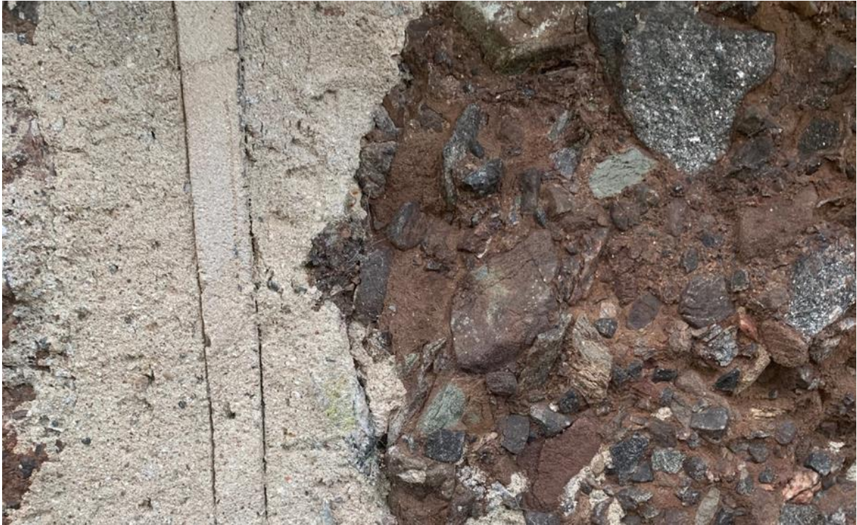
Figure 042.2. Poor quality local agglomerate stone with traces of irregular vertical and horizontal ribbon pointing. Traces of what maybe c.1816 harl in the deeper recesses of the agglomerate stone with overlaying ribbon pointing from the 1879 work.
