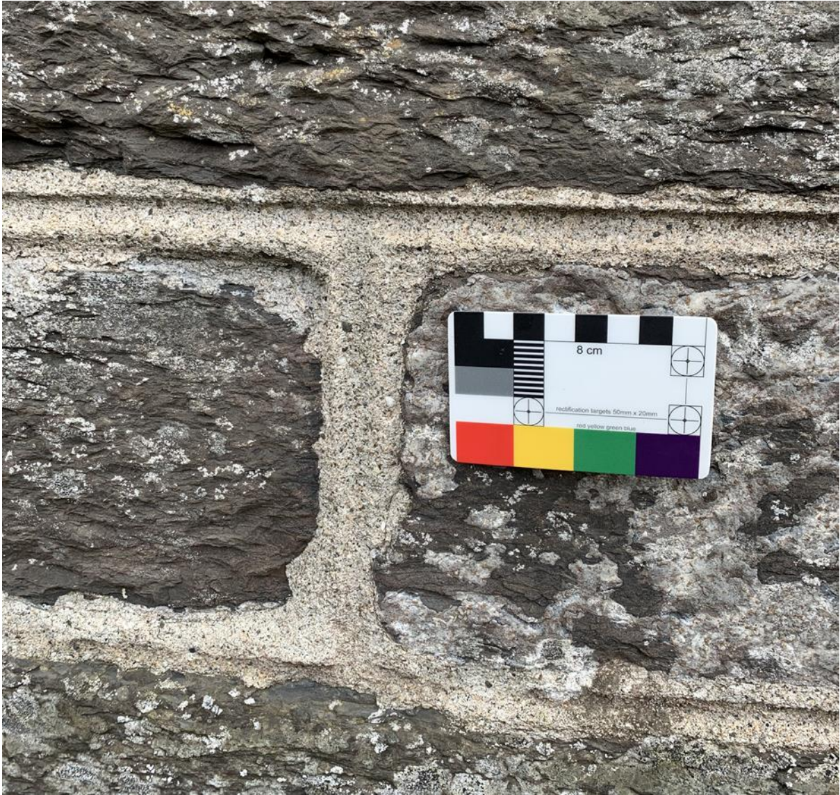
Figure 017.2. Detail of the flush point with horizontal and vertical lining out. The tool used has given a slightly wider line than is normal.
