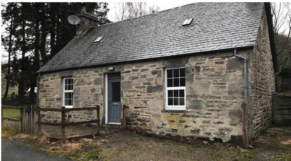
Figure 066.1. Single bay stone cottage with flush pointing and a crude attempt at ruling out.
