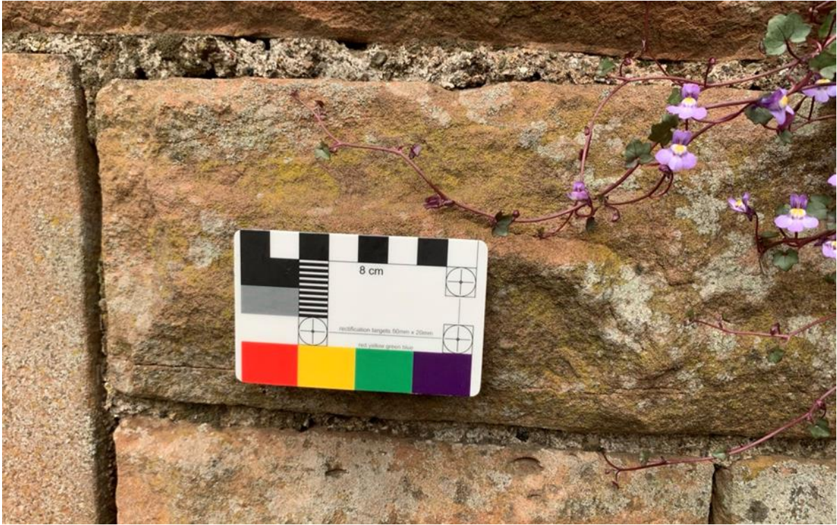
Figure 128.2. Weathered and eroded joins in the original mortar.
