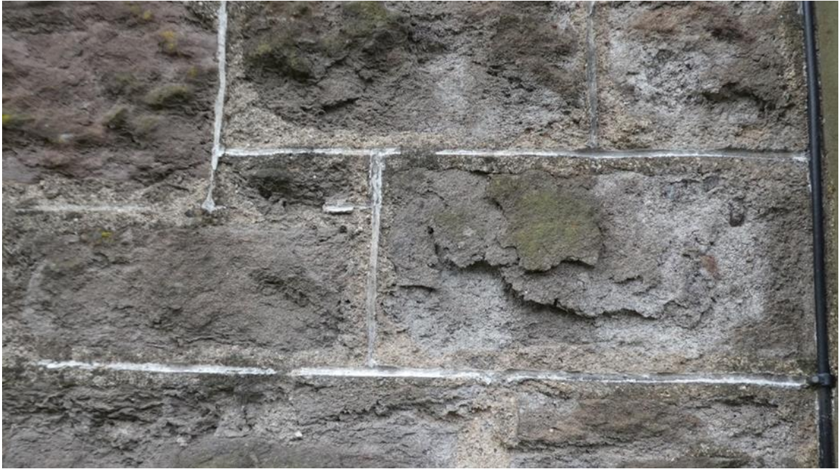
Figure 119.2. Ruling out and white lining. Stone decay evident.
