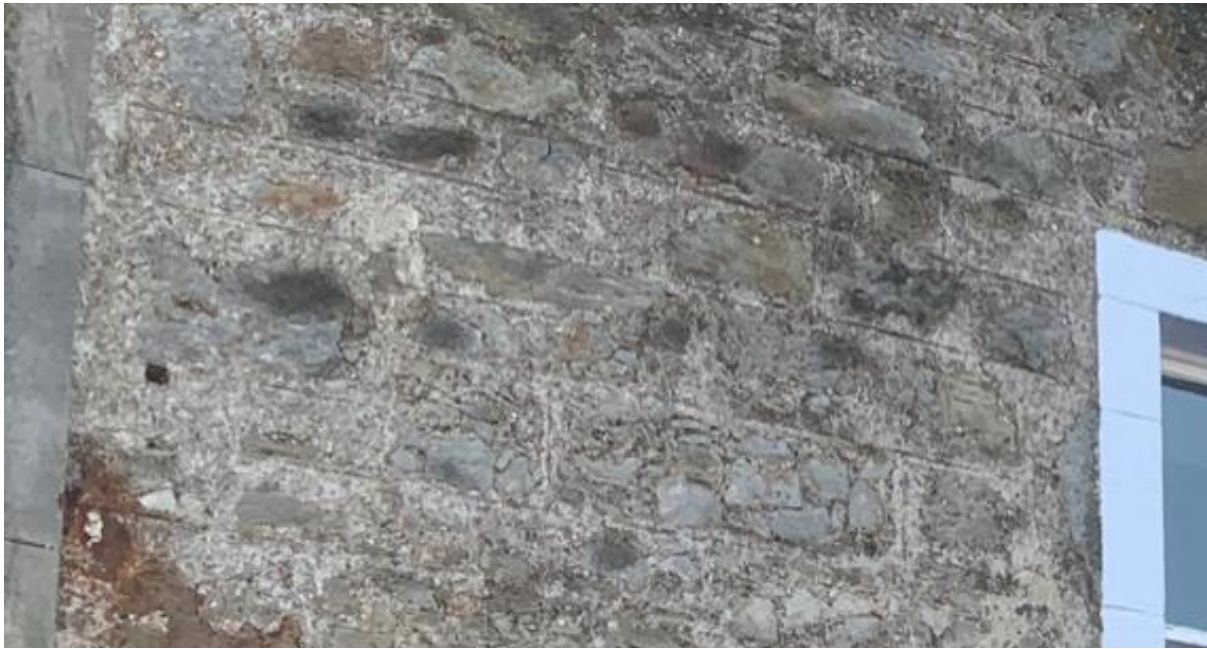
Figure 010.2. Change in masonry above close entrance.
