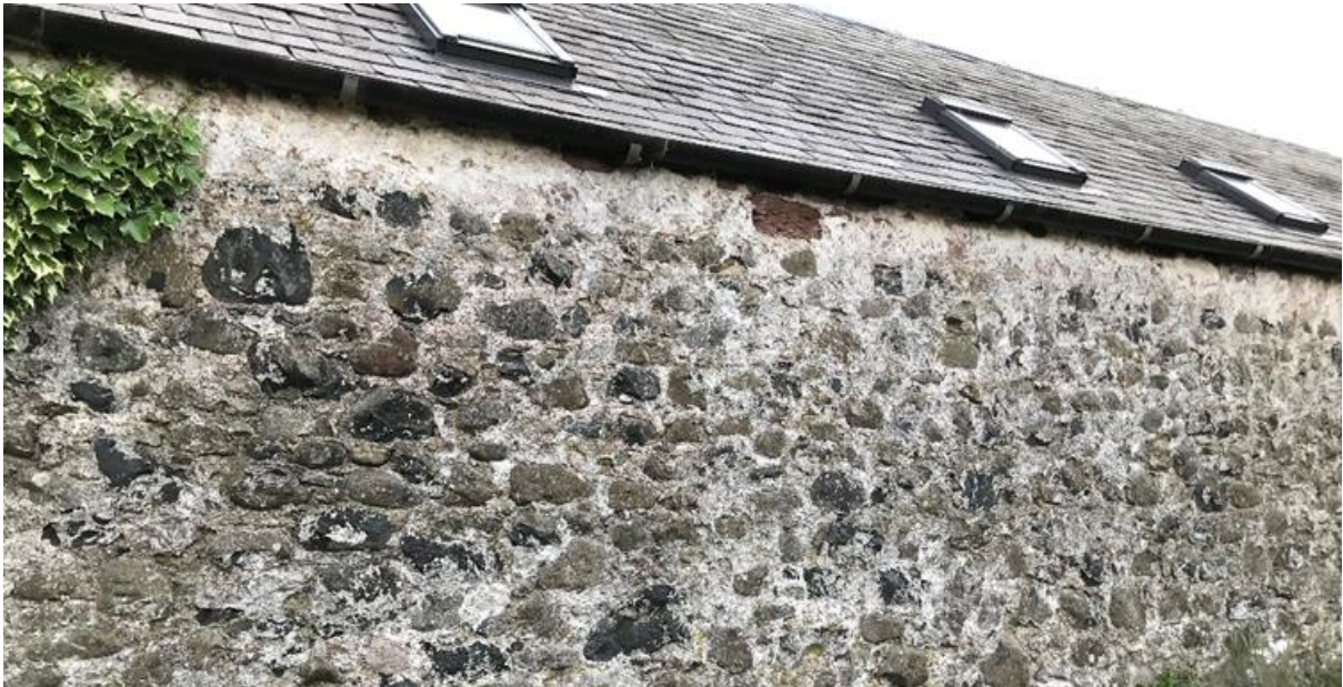
Figure O85.2. The roadside elevation of the steading with what appears to be original finishes. Note the better survival of limewash and pointing under the rhone.
