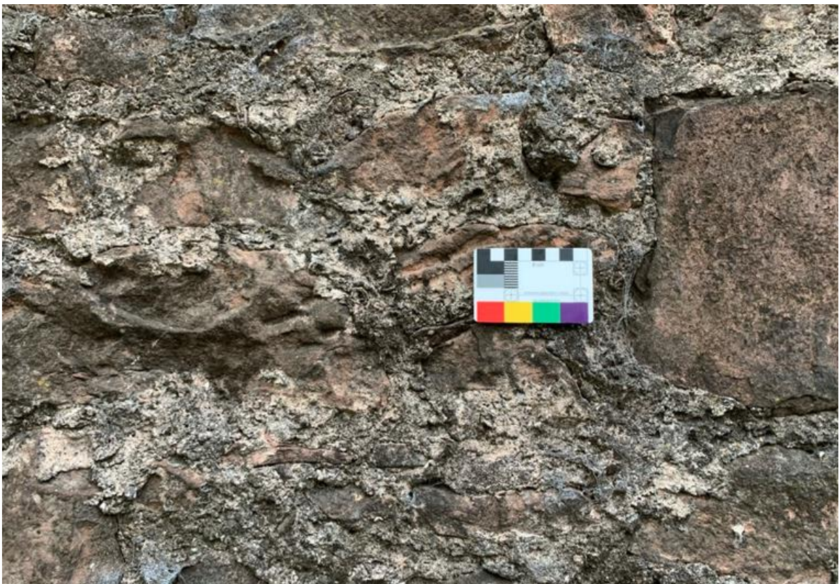
Figure 040.3. Remains of a coarser sneck harl or flush finish on a rear building in the complex.
