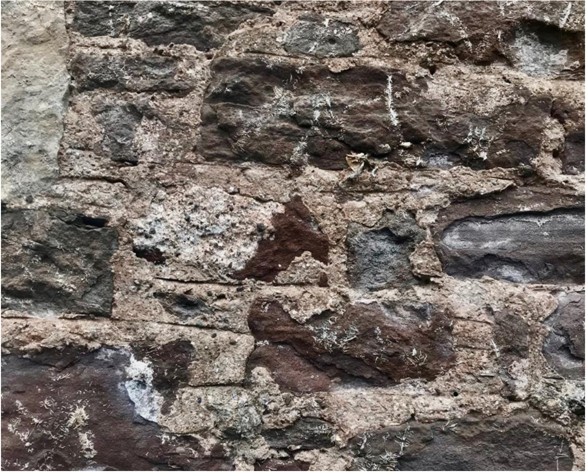
Figure O31.2. Informally ruled, flush lime pointing of modest quality. The lighter patch of harl on some of the stones indicates that the building may once have been fully harled.
