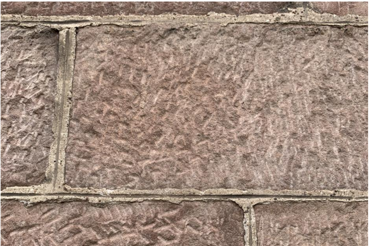
Figure 050.3. Multi directional tooling of the masonry blocks on the principal elevation. Crisp lined out flush pointing still in good condition.
