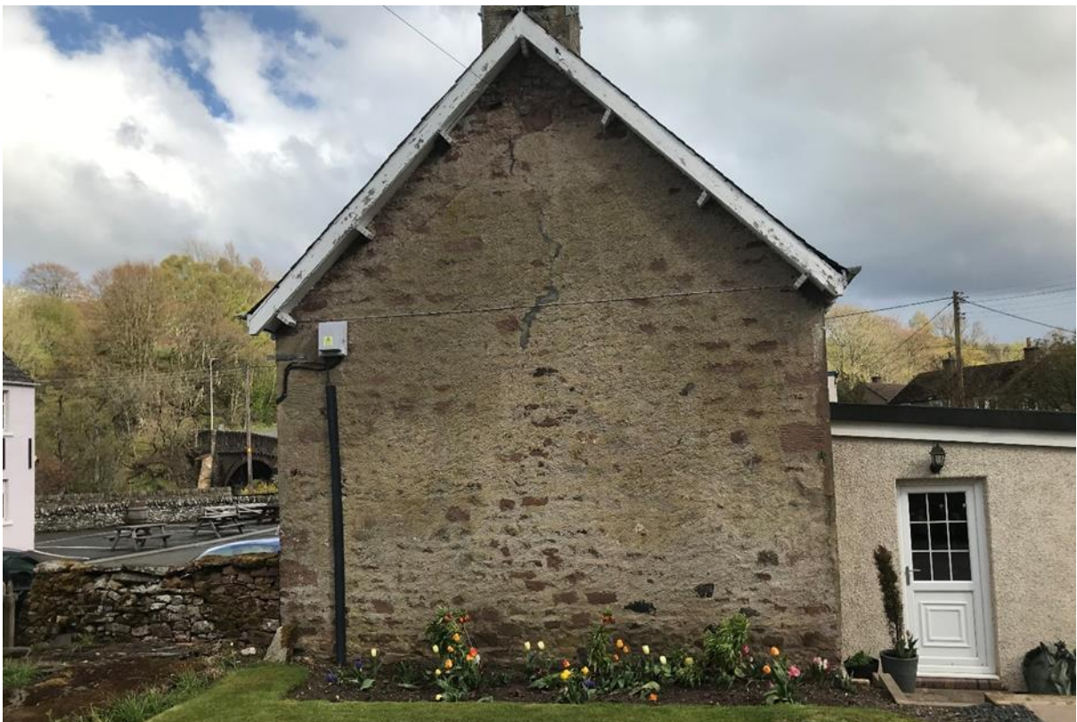
Figure 036.3. The East Gable, showing the later sneck harl using cement, but applied in a traditional fashion.
