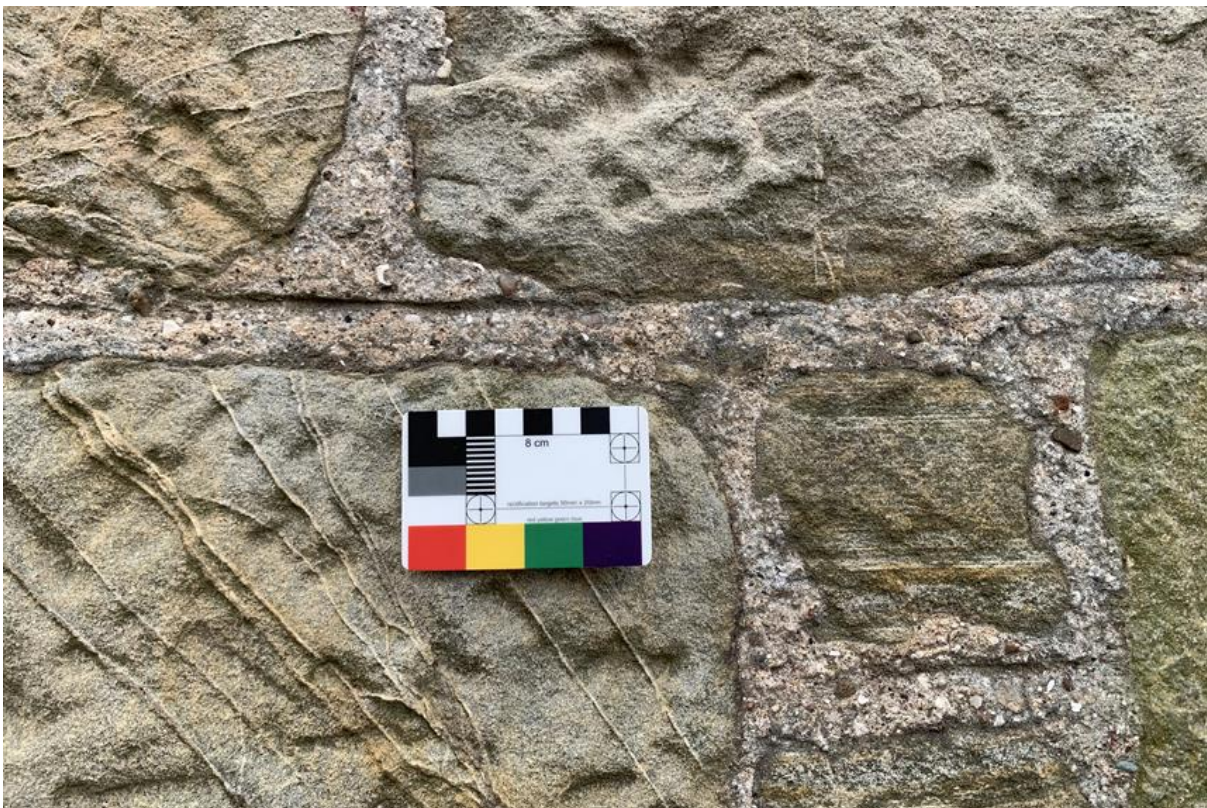
Figure 125.3. Masonry on the side elevation with rougher cut masonry blocks and a flush finish, with horizontally ruling.
