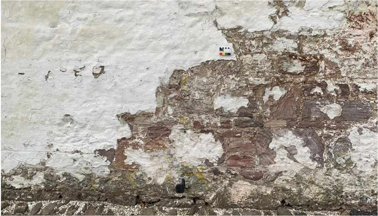
Figure 038.2. The flush pointed elevation with multiple layers of limewash.
