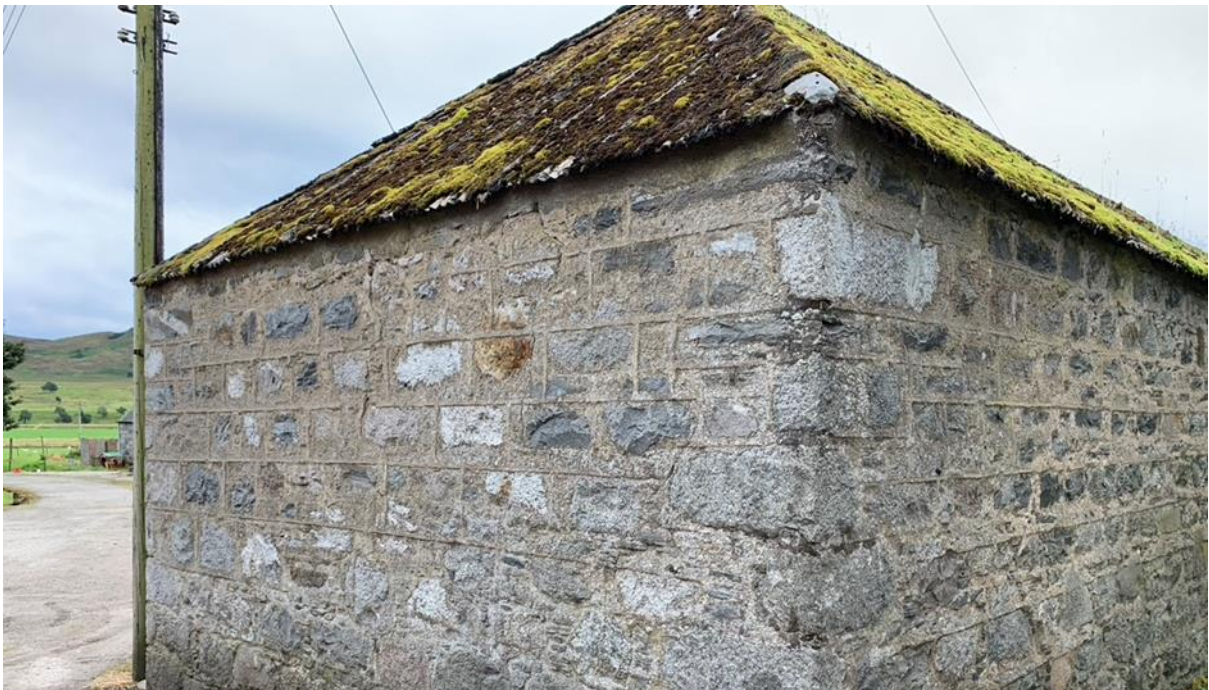
Figure 024.6. Continuous sneck and ribbon pointing applied to all elevations. Note how the quoin stones interrupt the ribbons but do not interfere with the band continuity.
