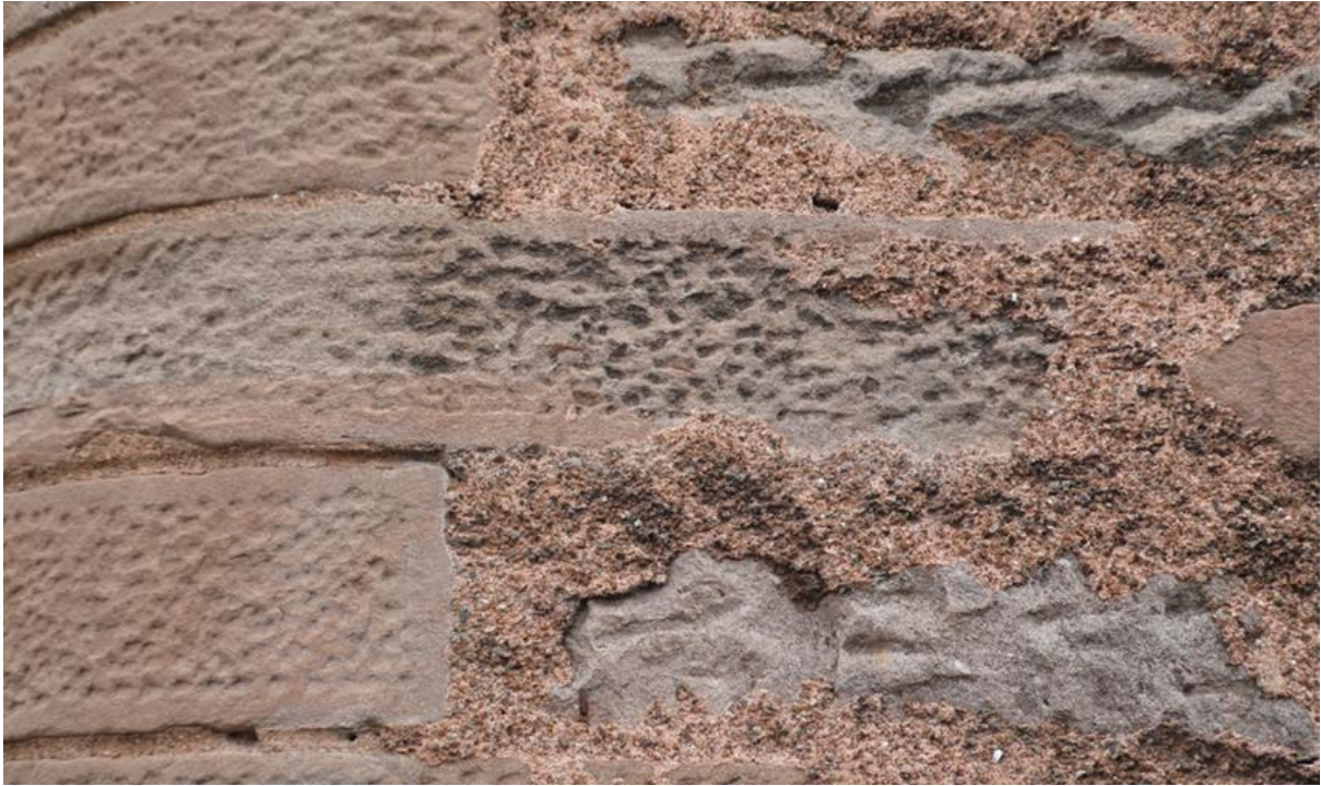
Figure 107.2. Coarse pink mortar used for both the ashlar work and the sneck harl.
