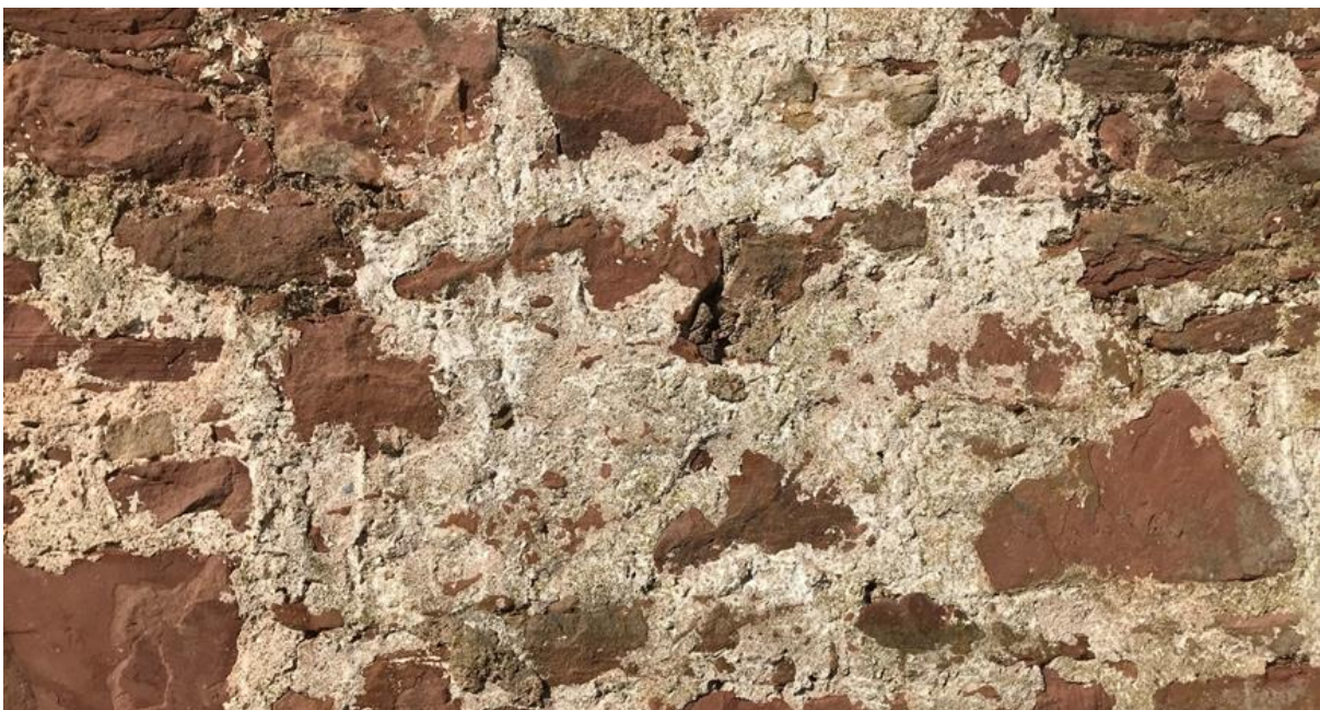
Figure 007.3. Flush pointing and limewash traces on the lower part of the gable dating from the 18th century.
