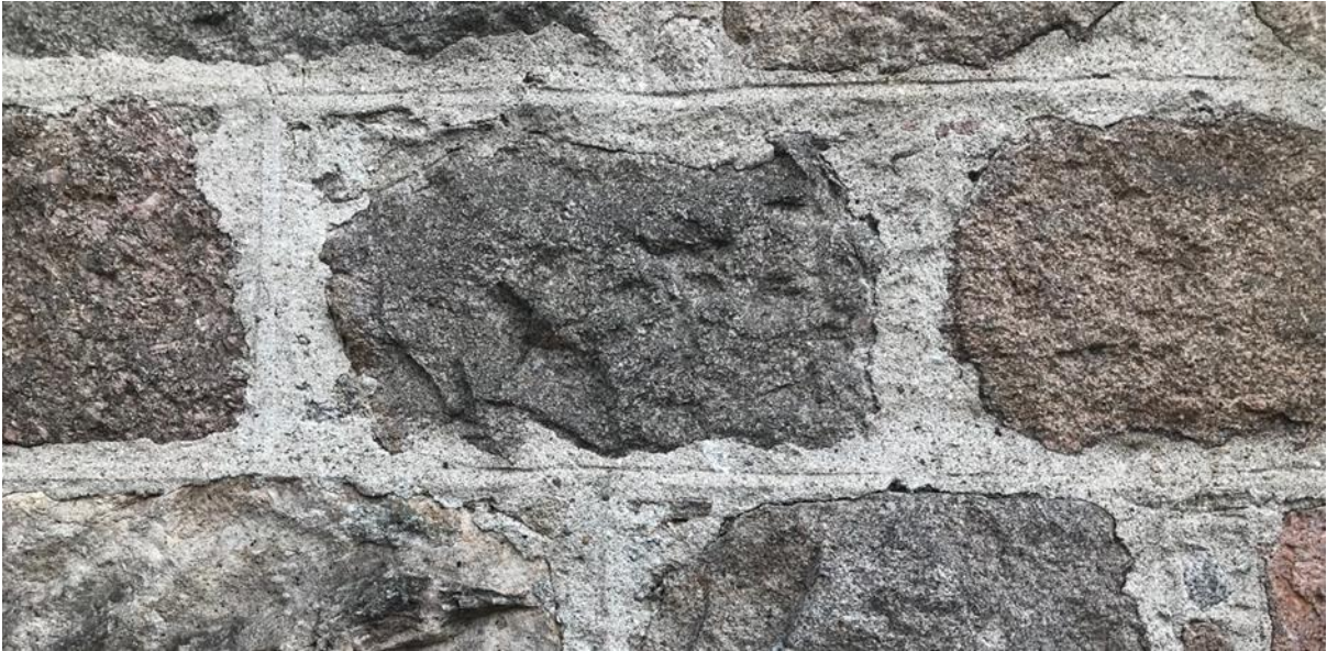
Figure 009.2. Worn raised band pointing.
