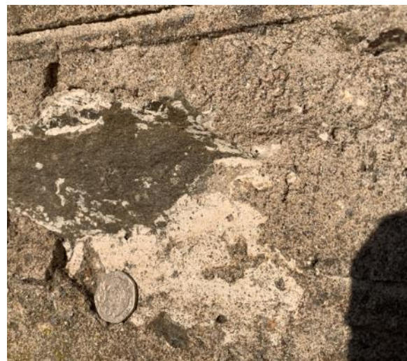
Figure 027.3. Traces of limewash.
