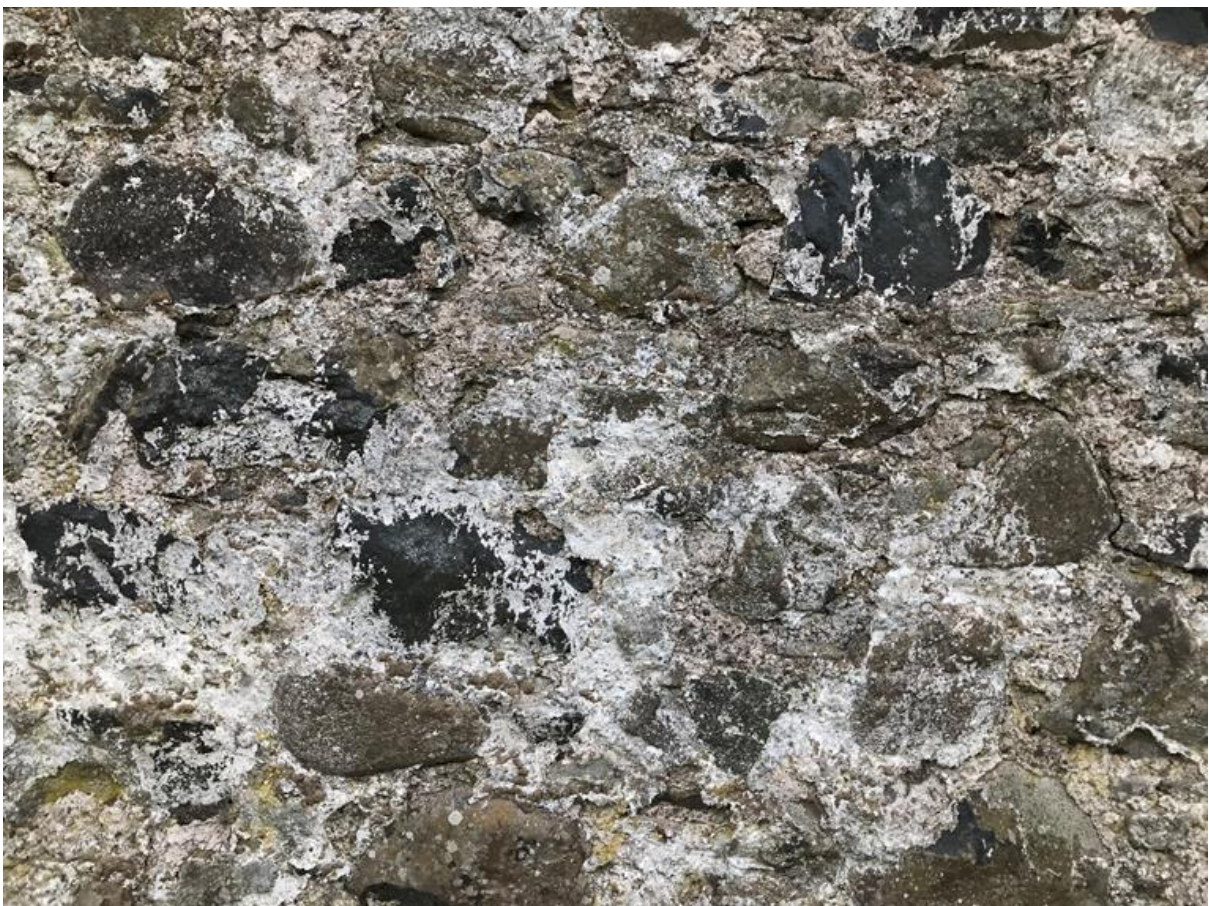
Figure O85.3. Detail of the masonry finish at Ladyrigg, showing the flush or sneck point and the surviving limewash.
