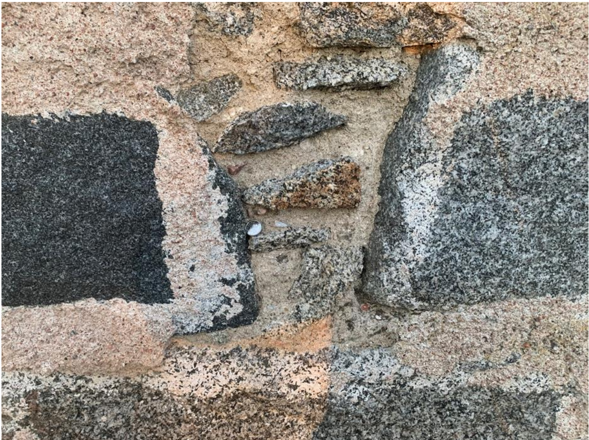
Figure 113.3. An area of pointing loss, with ghost marks of the mortar in relation to surviving sneck harl.
