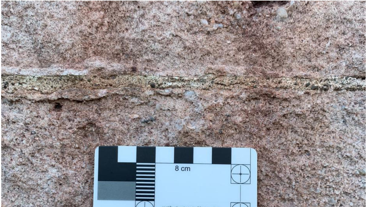
Figure 094.2. Worn, ruled pointing on the main body of the hotel.
