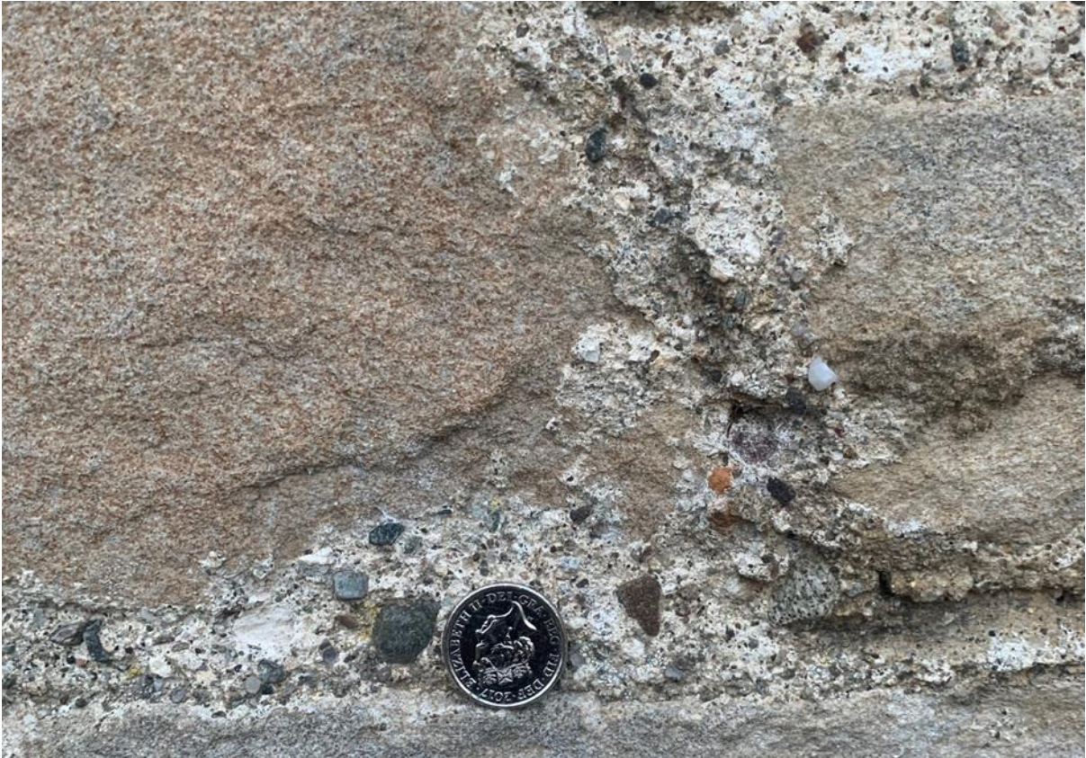
Figure 121.2. Very coarse mortar used for bedding and finishing.
