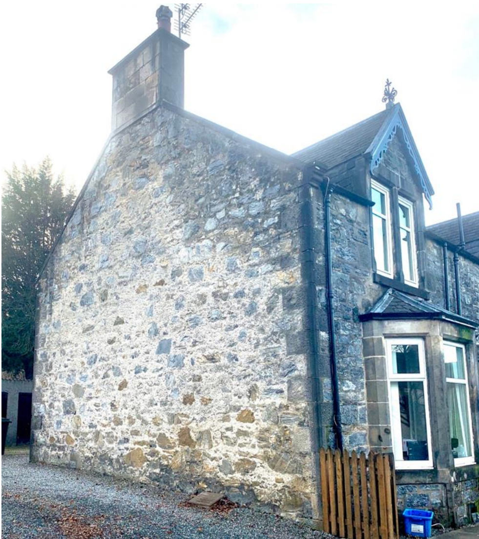
Figure 110.1. Gable elevation showing sac fungus.
