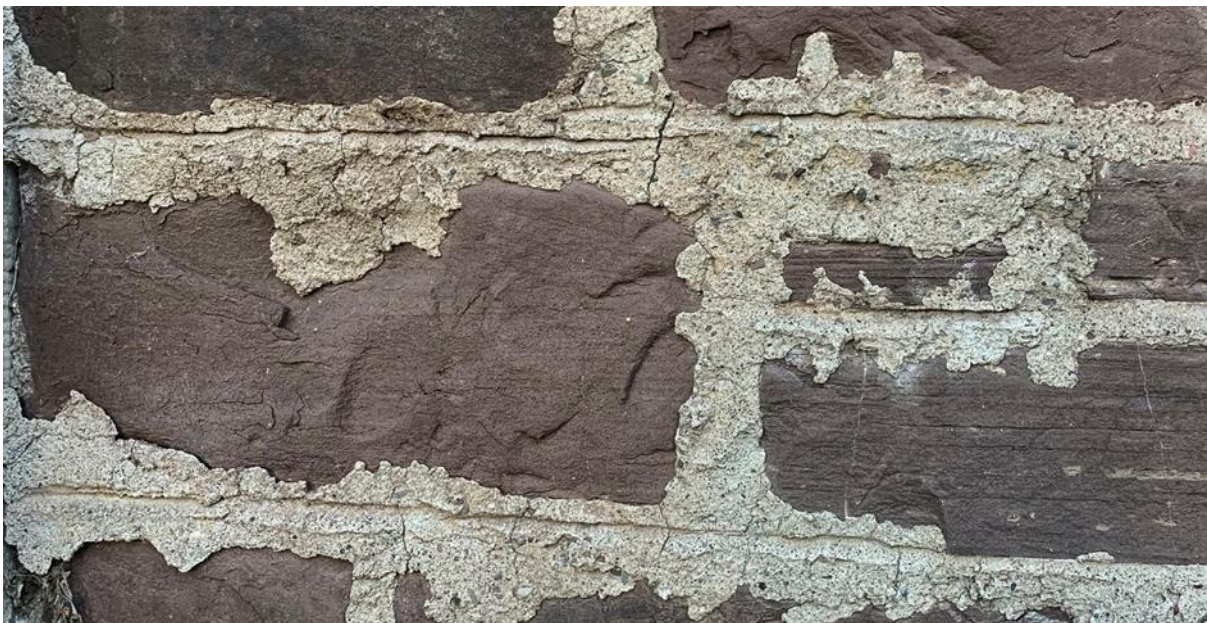
Figure 072.3. Informally ruled out flush pointing on rear elevation.
