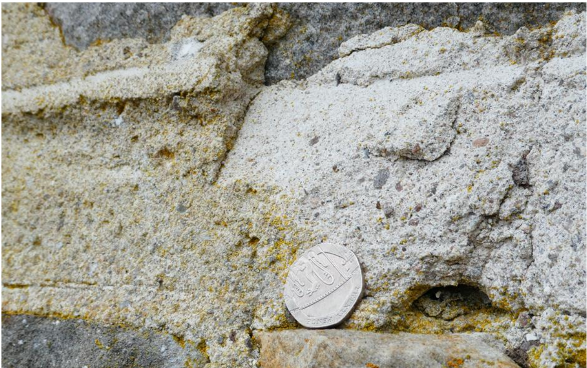
Figure 102.5. The first flush finish was integrated with the construction work. The final coat was applied once the building work was complete.
