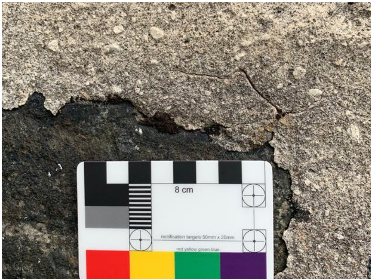
Figure 104.3. Soft lime pointing with multiple lime inclusions. This earlier style covered much more of the whinstone than the later pointing.
