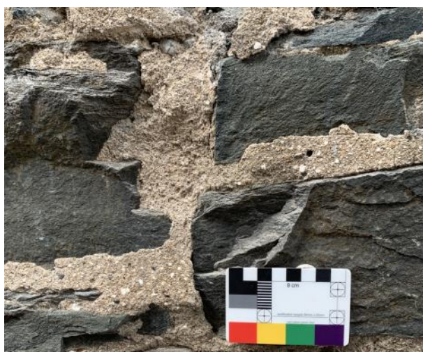
Figure 067.2. The weather struck pointing on the gable end.
