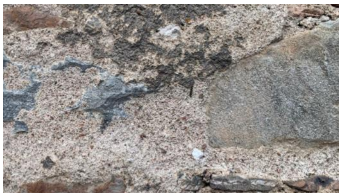
Figure 045.3. Mortar with lime inclusions.
