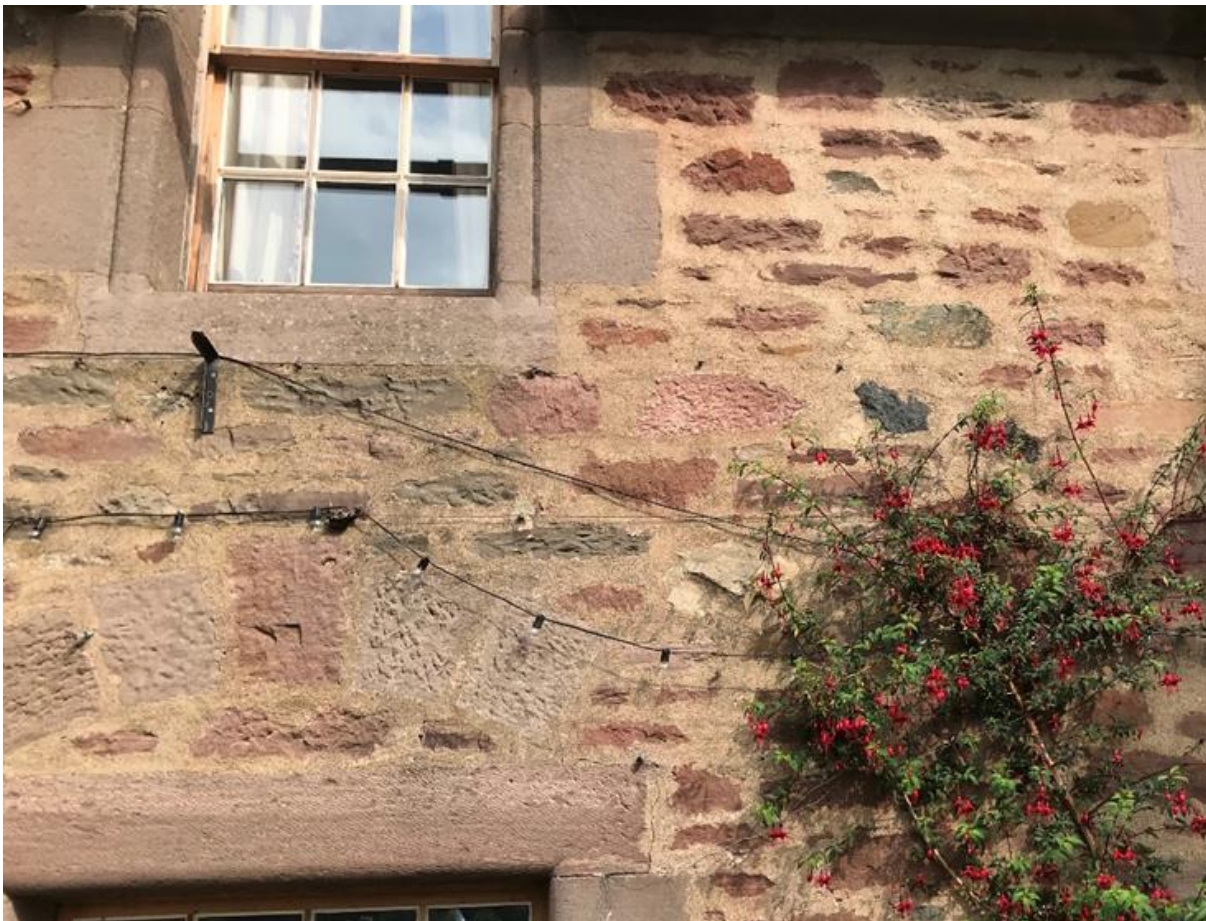
Figure 130.3. Pointing work from the 1920's on the south wall of a 17th century range. This work is flush to the masonry.
