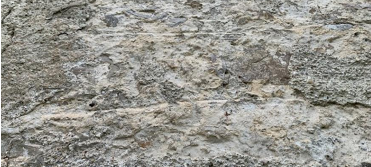
Figure 018.2. The lined out flush pointing from Phase one of the building, probably around 1830.
