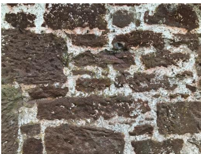
Figure 028.2. Close up of the pointing on the north east elevation. Limewash shows on the joints and in the broaching of the rubble.
