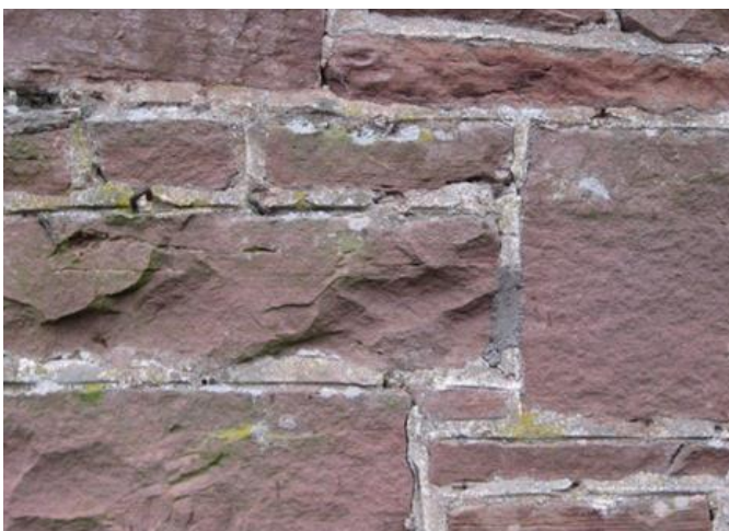
Figure 090.2. The pointing on the front elevation showing the weatherstruck finish, it appears to be original.
