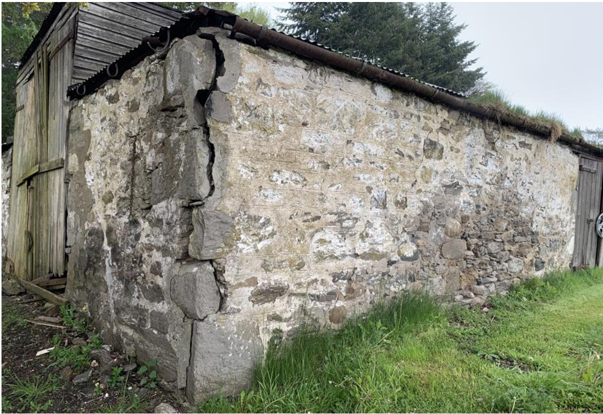
Figure 026.1. The steading building showing the flush pointed ruled out masonry and limewash.
