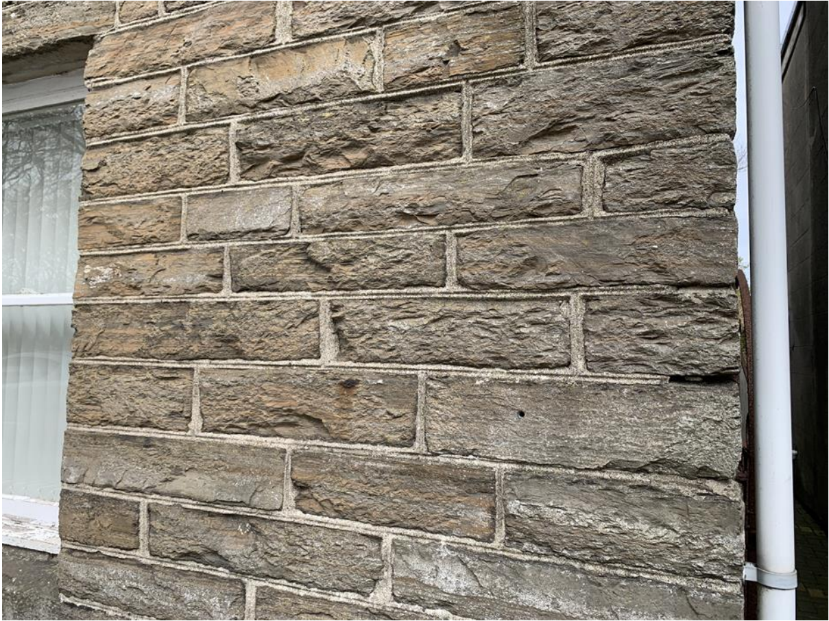
Figure 011.2. Coursed masonry with horizontal and vertical lining out on the pointing. The mortar appears to be original.
