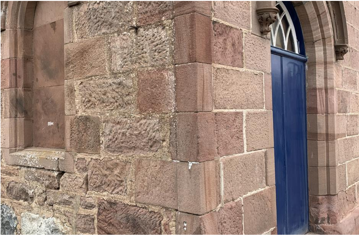
Figure 050.2. The corner of the building showing the hierarchy of finishes - smoother cut blocks with lined out pointing on the principal elevation, with the coarser finishes for rear elevations showing on the left.
