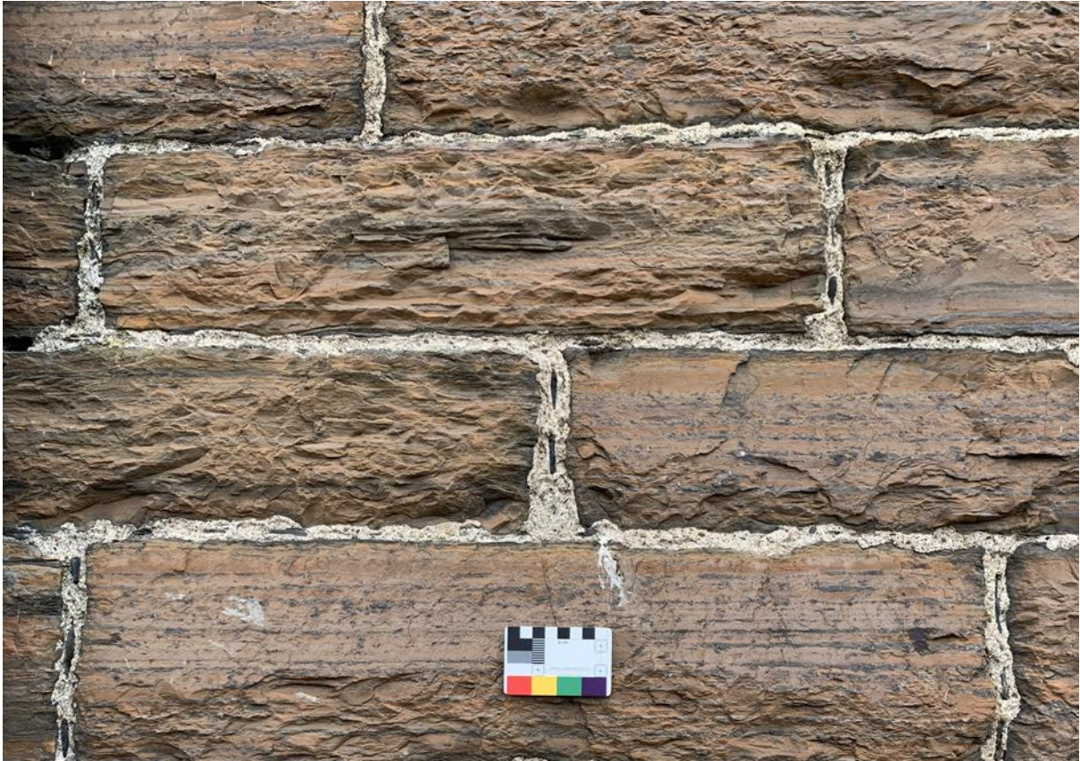
Figure 016.2. Cherry cocking of the joint with slate pieces, a feature done in lieu of the more common lining out seen in many other buildings in this study.
