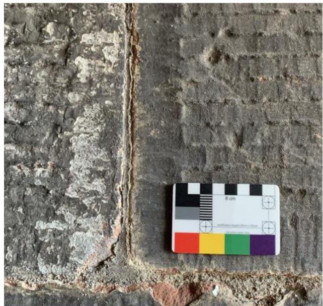
Figure 094.4. Masonry finishes in the adjacent close, showing fine pointing and discoloured layers of remaining limewash.
