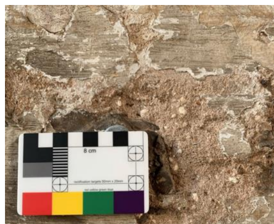
Figure 081.3. The mortar showing through where the limewash has come away.
