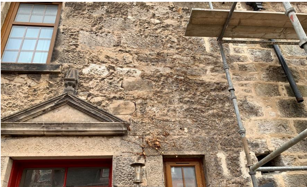
Figure 098.3. West elevation with extant harling to the left and new pointing work to the right, in a modern style.
