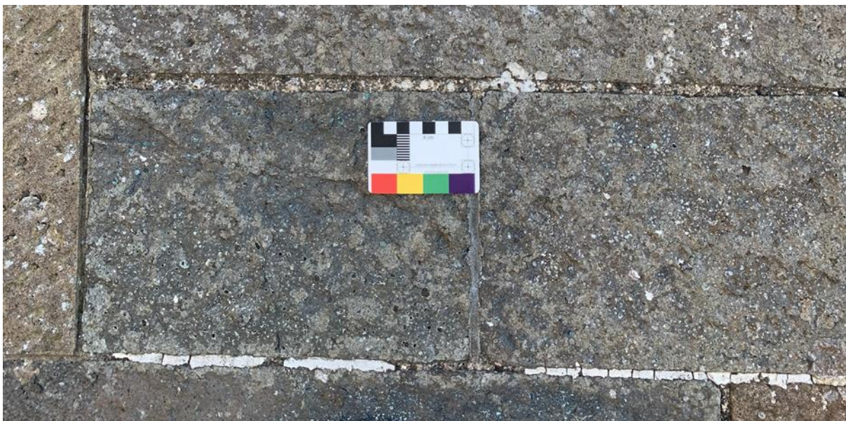
Figure 093.3. East elevation of the porch with the remains of white putty pointing.
