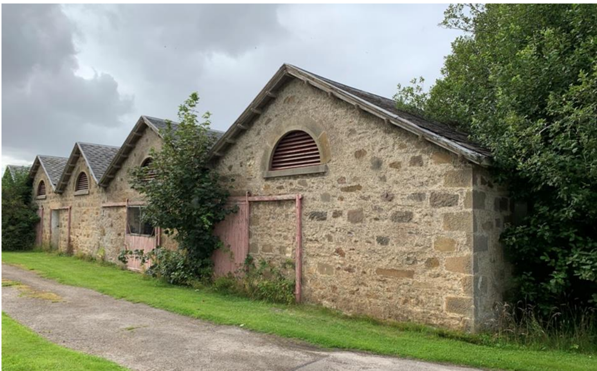
Figure 100.3. The rear, harled elevation of the steading, material wearing away with the best preserved remaining under the eaves.
