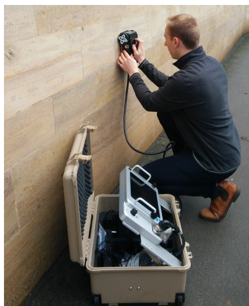
Figure 26 - A high-resolution radar being used. The antenna is placed on the surface of the wall, while the control unit (in the case) records the signals reflected by the wall surface and from components of the sub-surface.
