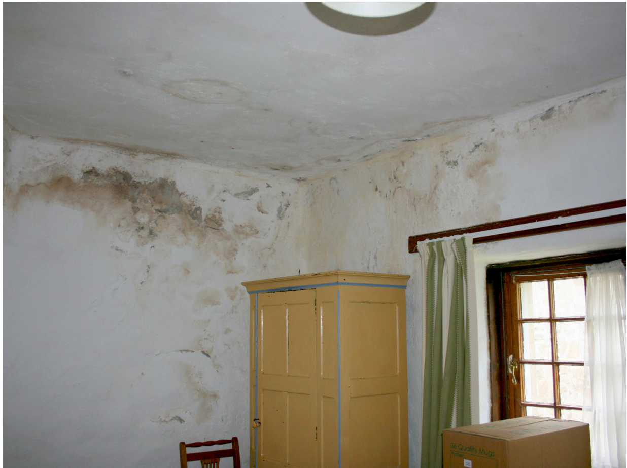
Figure 3 - Moulds and other microorganisms will colonise damp internal walls.
