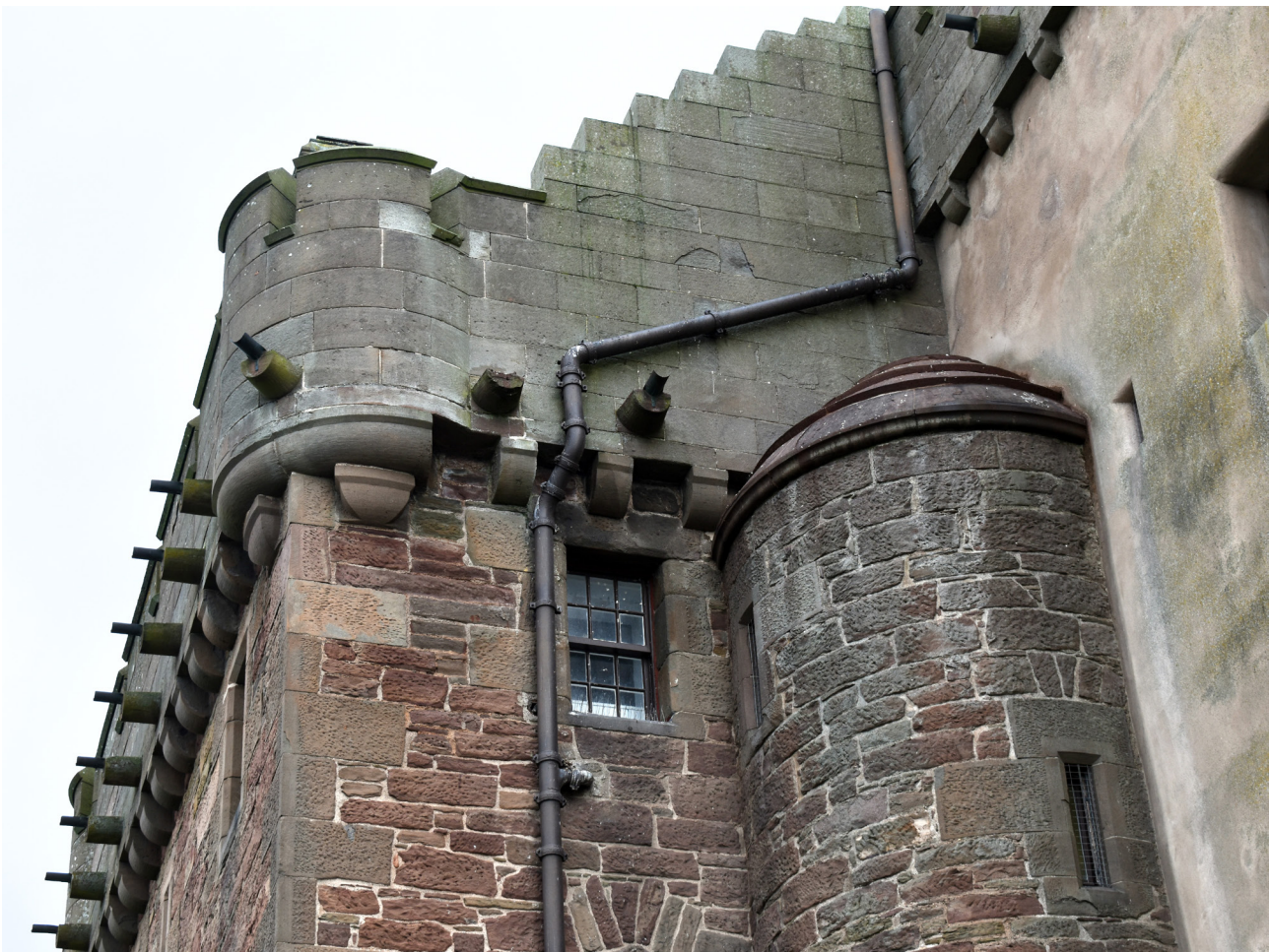
Figure 1 - Buildings in the historic environment may contain complex combinations of materials, methods of construction and past repair interventions, making the interpretation of moisture data complex.
