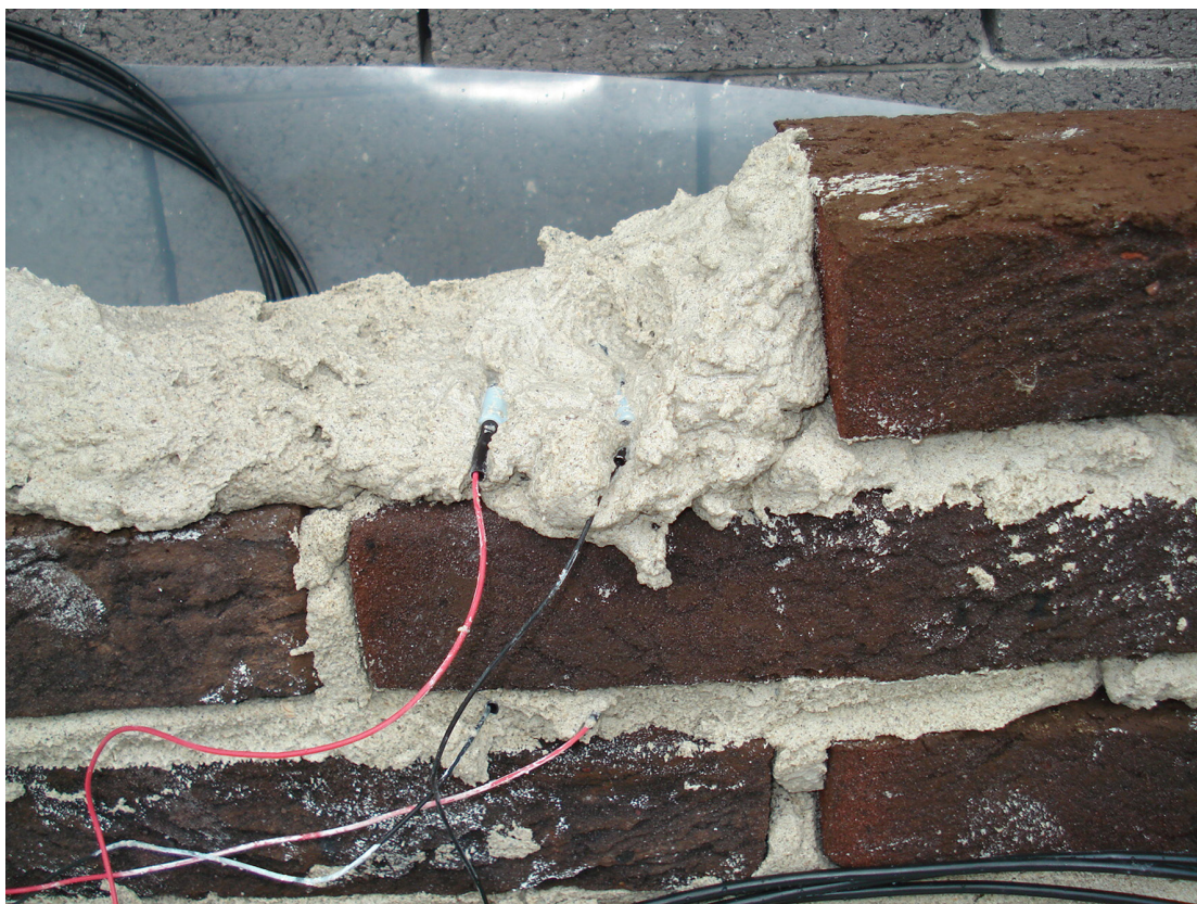
Figure 8 - Invasive electrical probes being built into the bedding mortar of a purpose-built test wall. Probes can also be installed by drilling holes into the masonry units and mortar joints of an existing construction. © Dr Evy Vereecken
