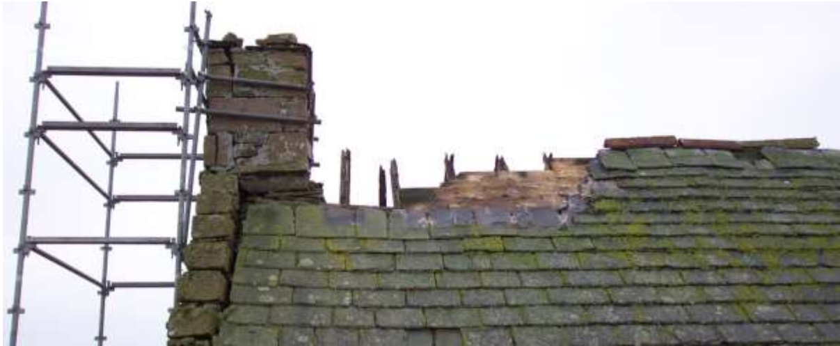
Figure 17: North gable chimney stack showing the gable separation from the roof structure
