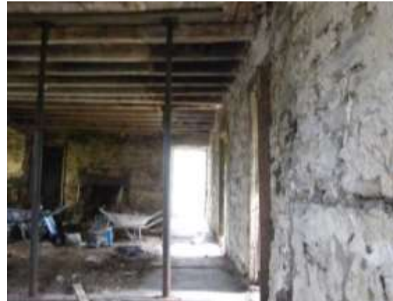
Figure 19: Existing ground floor condition with temporary props supporting the floors and the masonry partition above
