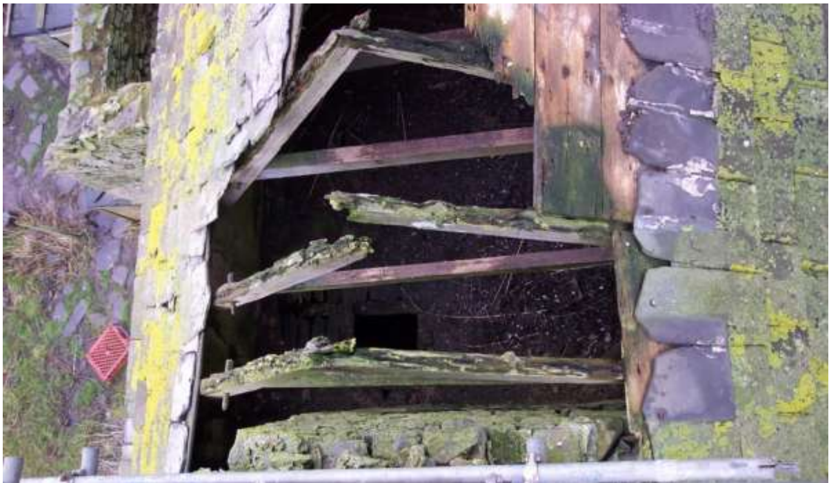
Figure 15: The roof before works, showing rotten timbers at the apex
