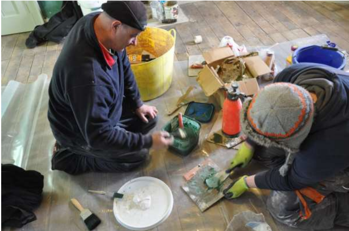
Figure 25: Local plasterers learning how to mix the lime plasters and paint from the lime consultant
