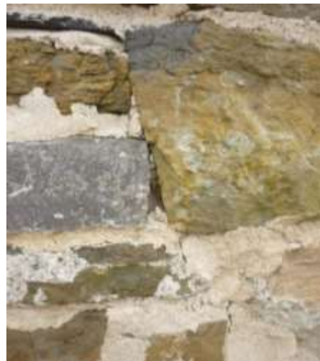
Figure 28: Section of the external wall showing existing lime mortar at the top and new lime mortar
