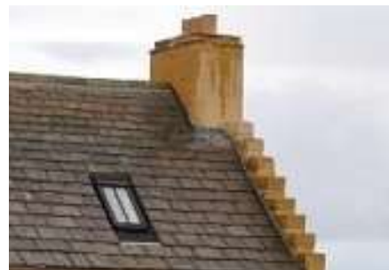
Figure 29: Lead soaker ragged into the base of the chimney
