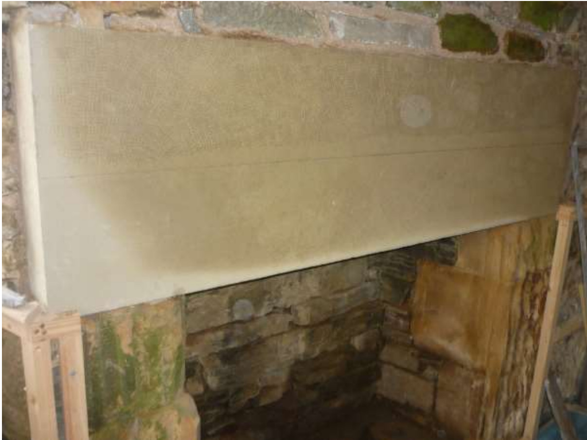
Figure 41: New stone lintel in situ above the ground floor fireplace in the west gable
