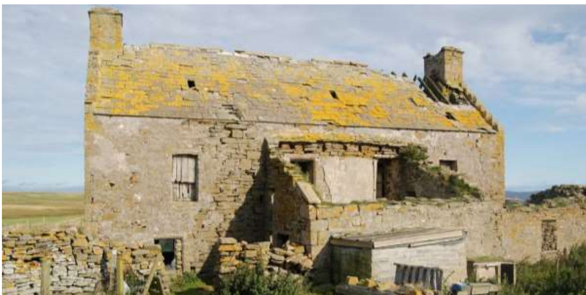
Figure 18: South elevation with vertical crack to the east. The pockets in the masonry of the wall in the entrance wing where the rafters would have been bedded are visible
