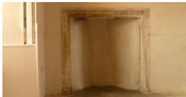
Figure 13: First floor, west gable hearth during repair, with a simply detailed moulded wooden surround
