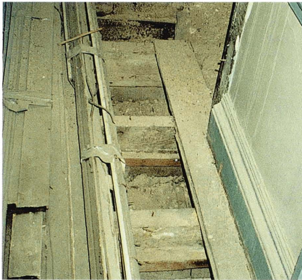
Illustration 32. Floors opened up to increase ventilation. Opening up floors will improve ventilation, promote drying and prevent further decay by the dry rot fungus.
