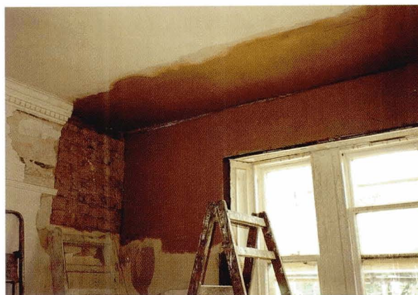
Illustration 8. Conventional dry rot treatment Conventional dry rot treatments may be very destructive and are not appropriate for the types of repair required in historic buildings or buildings with historic interiors. In this illustration the loss of original fabric is well seen. Note also the 'cutting back' of plaster by at least 1 metre on the party wall and loss of the decorative cornice .
