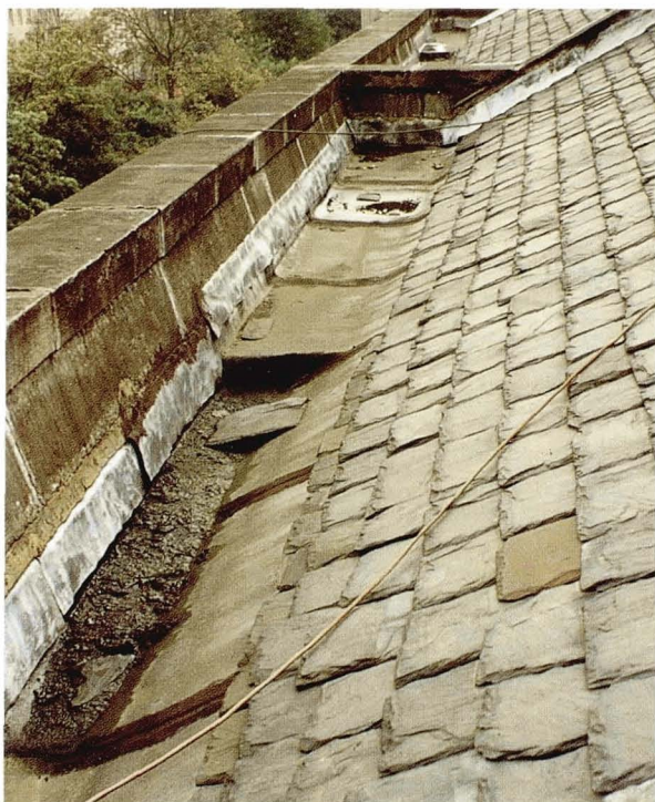
Illustration 12. Poorly maintained parapet gutter responsible for dry rot attack. Poor maintenance, substandard materials, missing and slipped slates, inadequate falls and a choked outlet led inevitably to an associated dry rot attack in this property.
