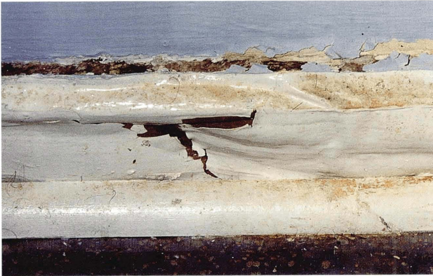
Illustration 4. Surface coatings may mask the destruction of wood. Trying to discover dry rot attacks by looking for decayed wood is an inappropriate strategy as the attack will often not appear on the visible surface of wood. In the case shown severe decay has developed under what was, until recently, an intact paint surface. The cracking across the grain is well illustrated.
