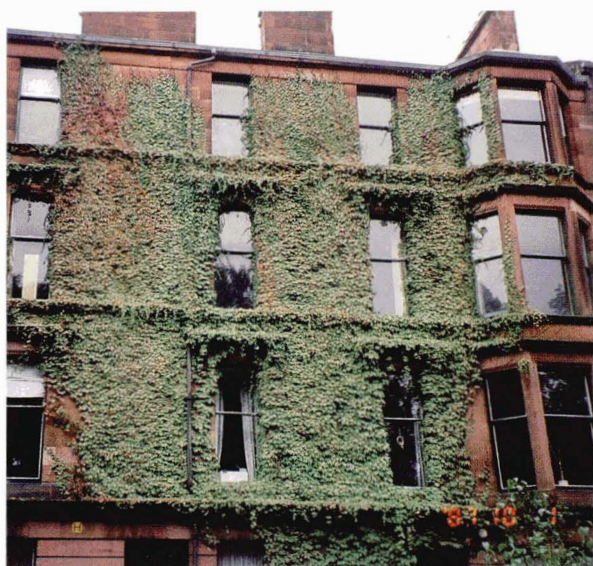
Illustration 26. Plant growth on a building façade This tenement in Glasgow boasts a luxuriant growth of ivy on its façade. Such growths may encourage retention of moisture in a wall and certainly should not be allowed to block rain-water discharge systems. However, uncontrolled removal of ivy can cause damage to stonework. The ivy should be cut at ground level (a section of stem removed) and the plant allowed to die before careful removal by hand from vulnerable stonework or brick wall.
