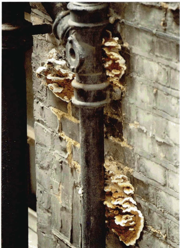
Illustration 27. Faulty rainwater pipe saturating a brick facade resulting in an internal outbreak of dry rot and an external fruiting body. © Hutton+Rostron
