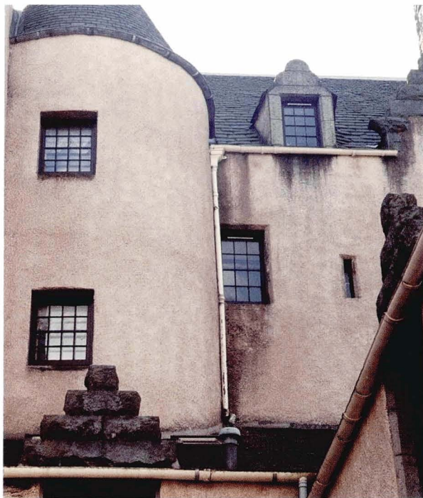
Illustration 19. Complex roof systems present serious challenges to the property manager. A series of roofs at different levels drain to a single small outlet. The wall area around the outlet can get very wet when the outlet overflows and this is inevitable unless maintenance levels are high.
