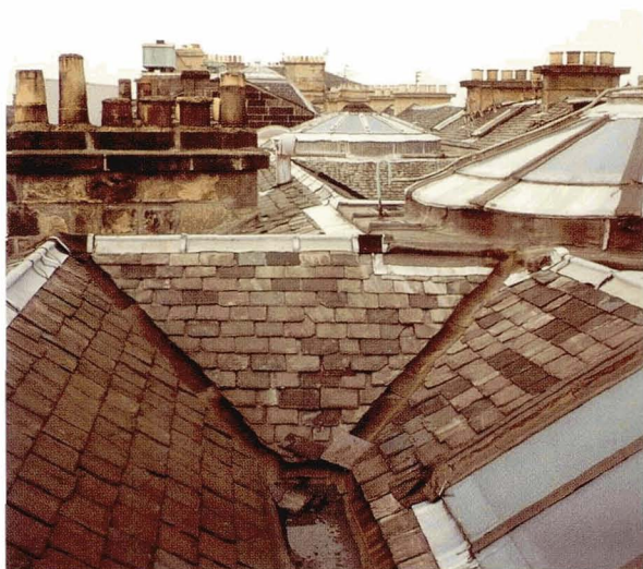
Illustration 16. A complex roof arrangement. Poor quality repairs, lack of maintenance, an internal outlet and inadequate falls have all resulted in water penetration to this property followed by a dry rot outbreak. It is likely that evidence of the water penetration was available long before the development of dry rot.
