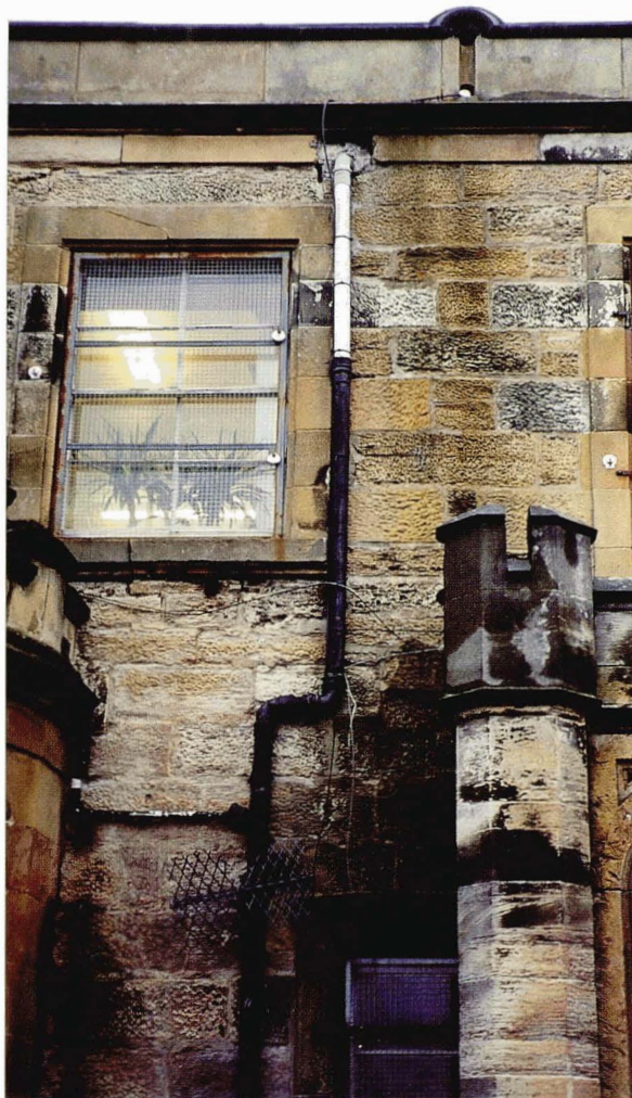
Illustration 28. Stained walls The black staining on the walls indicates a problem with the rain water discharge from the roof of this Tudor-style villa of c. 1828 on the outskirts of Glasgow.
