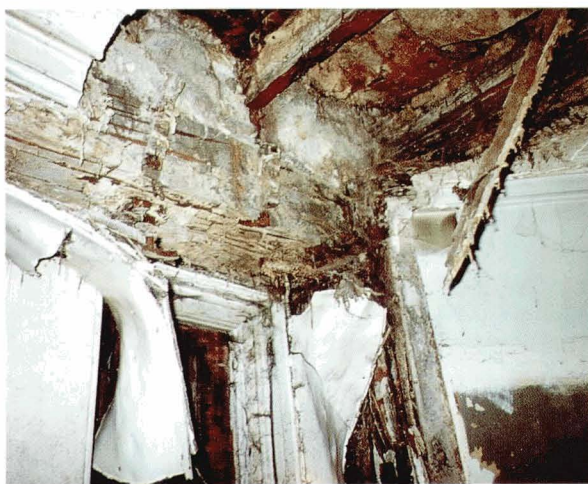
Illustration 22. A severe dry rot outbreak. Dry rot outbreak at intermediate floor level resulting from external wall defects. Note the infected safe lintols and the badly degraded floor joists
