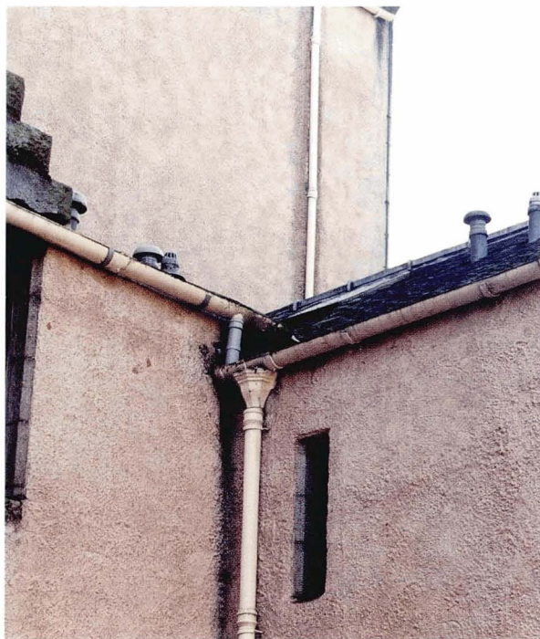
Illustration 20. A detail from Illustration 19. The concentration of downpipes in the corner can lead to wetting of the area. Water causing soaking of masonry at internal corners does not evaporate easily.
