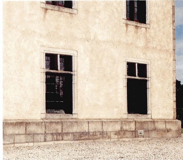
Illustration 39. Careful attention was paid to external ground levels and new air vents fitted where appropriate
