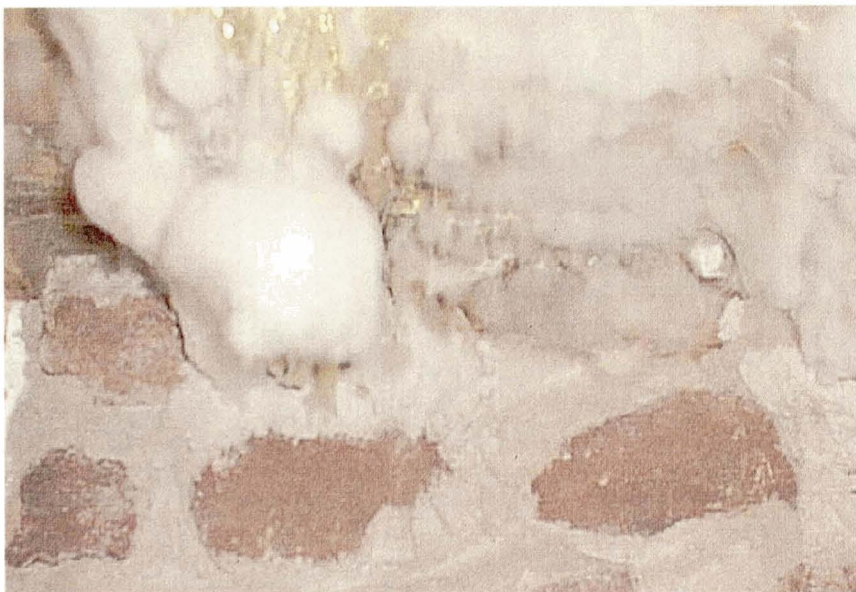
Illustration 2. Lush growth at a wood/ masonry interface Unlike most other wood decay fungi found in buildings the dry rot fungus has an absolute requirement for both nutrients from the wood and metal ions extracted from masonry (see Appendix F – Bibliography). Because of this the organism grows in a particularly luxuriant way around wood/ masonry interfaces. This is particularly well seen at the rear of lath and plaster or walls and ceilings.
