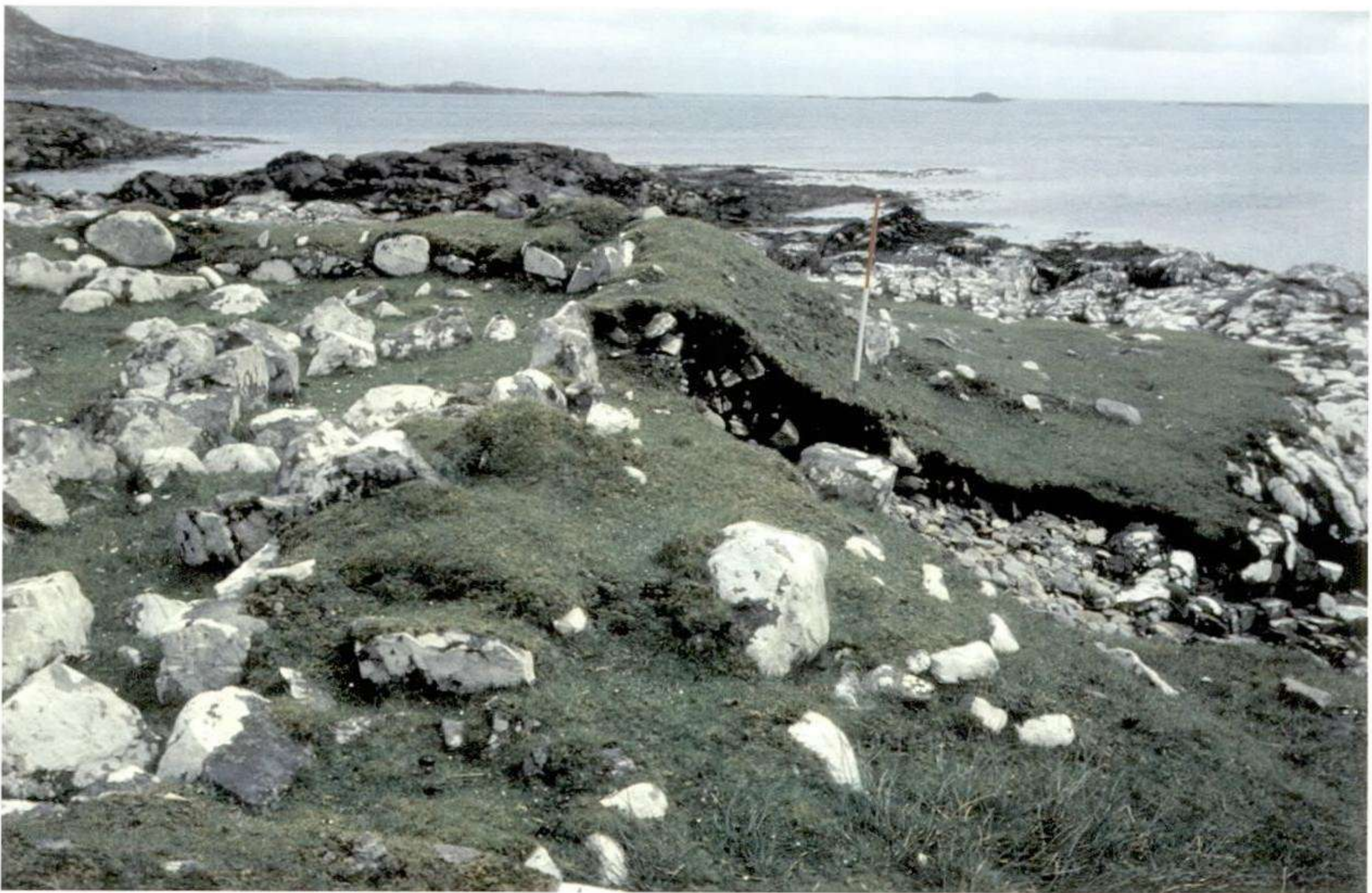
Figure 8.11. Site L7, a blackhouse on the east coast of Barra. The southern wall has been breached by the scouring effect of the tide.
