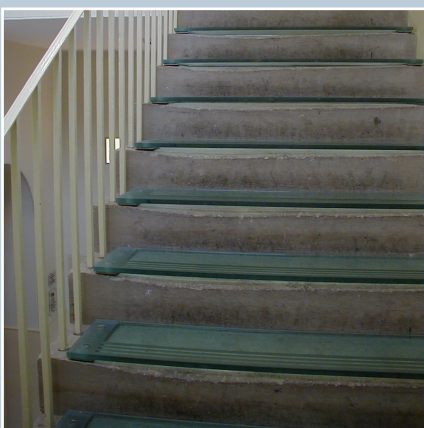
Glass treads with a textured finish are laid over the worn stone stairs in the Old School building at New Lanark. The wear on the treads is part of the significance of the school because it records many years of use by the children.
