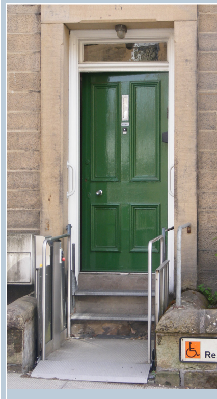
A small platform lift providing disabled access at a property in Hawick.
