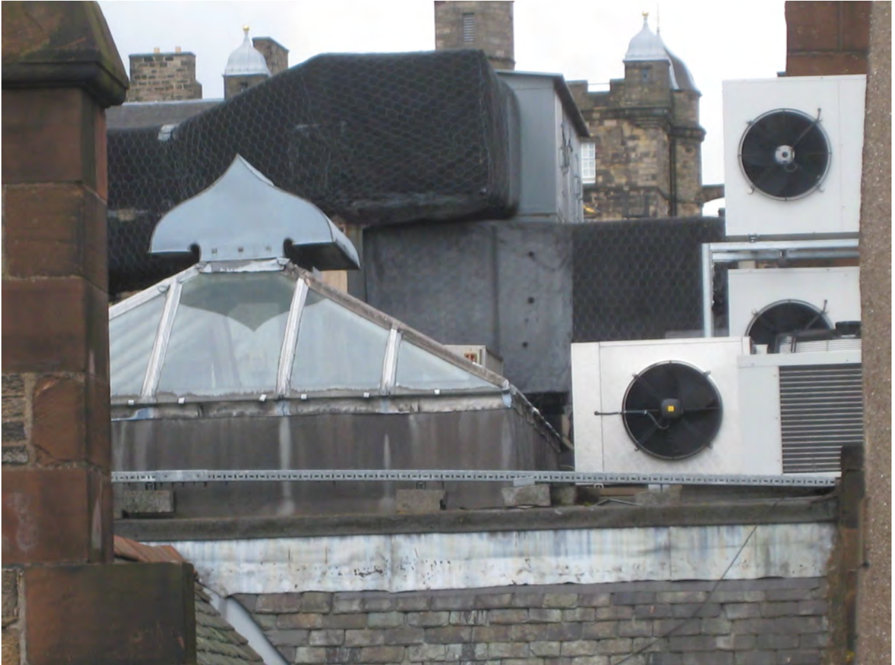
Figure 6 - A passive ventilation cowl can be seen at the top of a stairwell in Edinburgh and to the right a modern mechanical installation.
