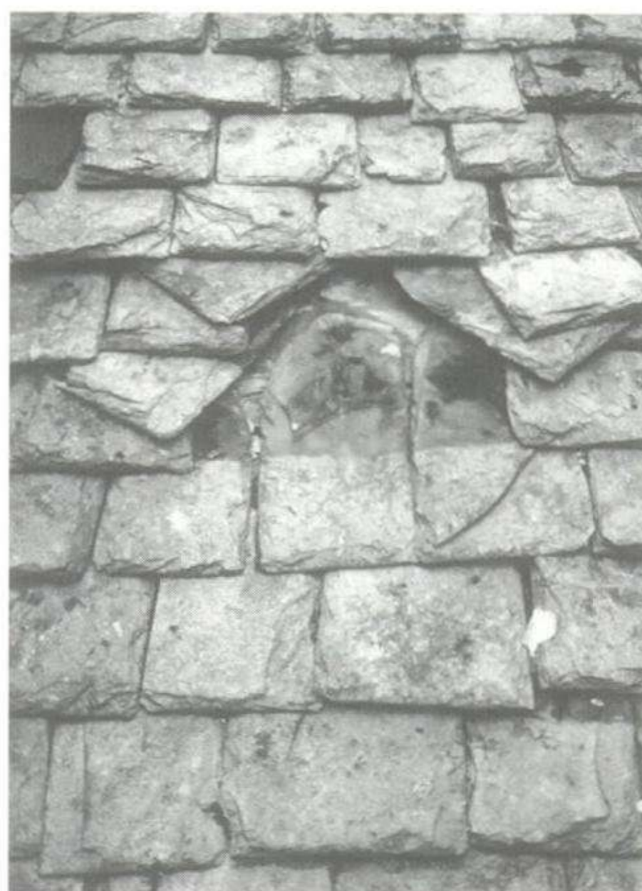
PRACTICE: The traditional practice of random slating to diminishing courses, the slates are shouldered, single nailed at the head and laid on sarking.
