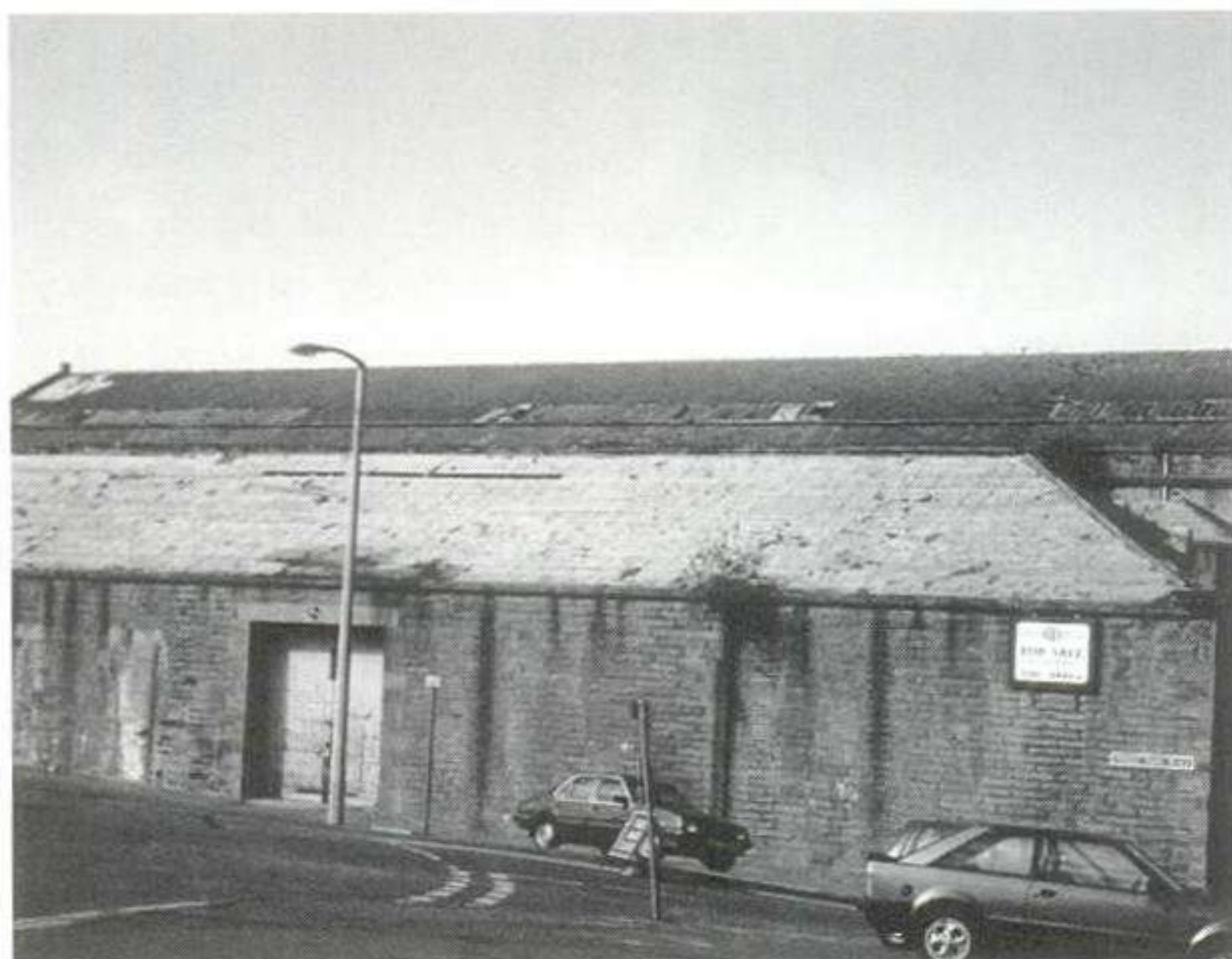
LOSS: Scottish slates lost and probably recycled for another building. An unsuitable source.
