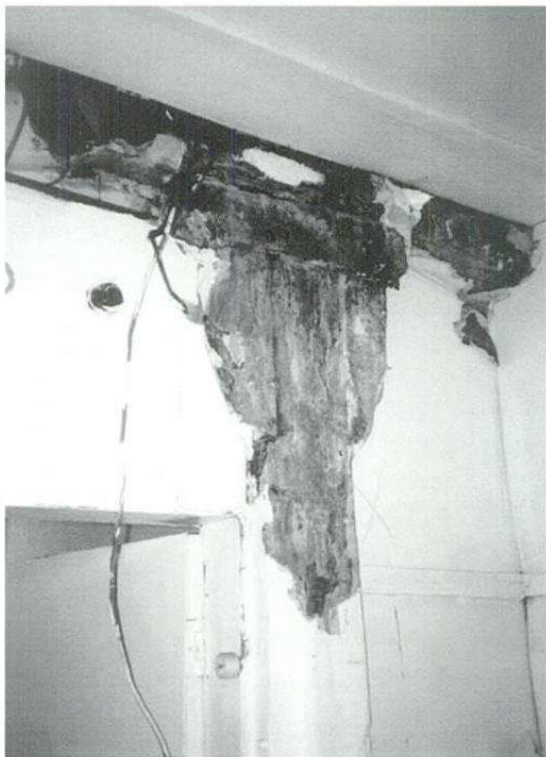
Figure 4: Vertical timber support, Gardyne's Land, High Street, Dundee
