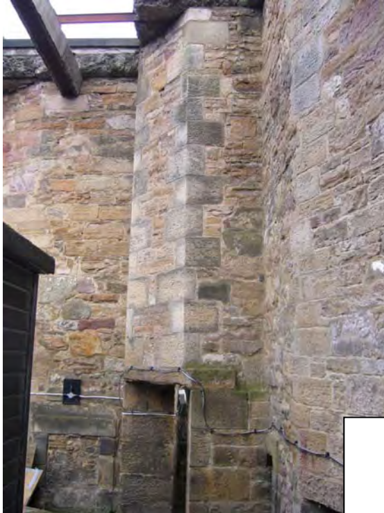
Sentry box(?) at SE corner of Shot Yard/Water Tower 1. Note blocked mural fireplace to left.
