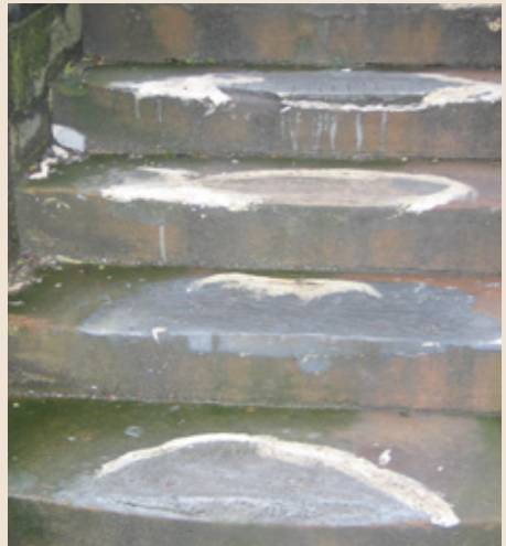
Fig. 8 A poor quality repair using cement.
