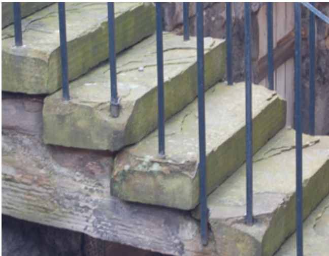
Fig. 10 A lack of maintenance can lead to rusting ironwork and masonry decay.
