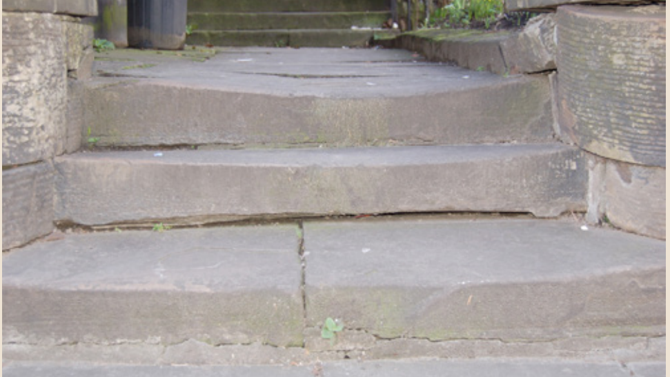
Fig. 6 Open joints can allow water to penetrate leading to masonry decay.
