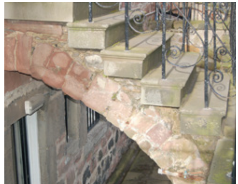
Fig. 2 Rectangular steps built with a supporting arch over a basement, a typical urban detail.
