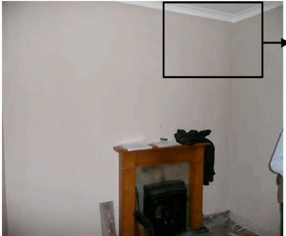
Fig. 14 Photograph of the east wall pre-intervention, showing the junction between the east wall and ceiling
