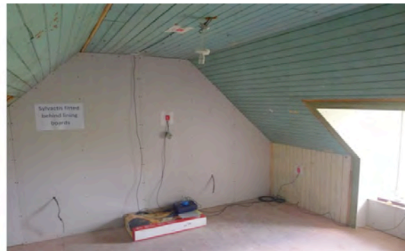
Fig. 36 Heat-flow mats on the first floor for post-intervention monitoring
