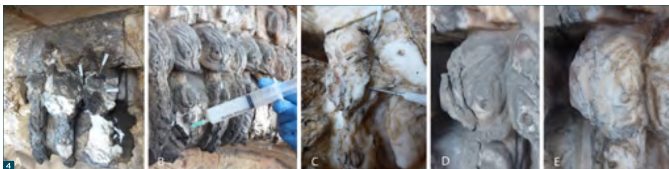
Figure 4: Stones during pre-consolidation with nano-lime (A and B), filleting repairs and grout injection to detaching scale (C), detail image of fractured and degraded stone prior to conservation (D) and same detail following completion including spot-fixing with acrylic resin, grouting and mortar repairs.
