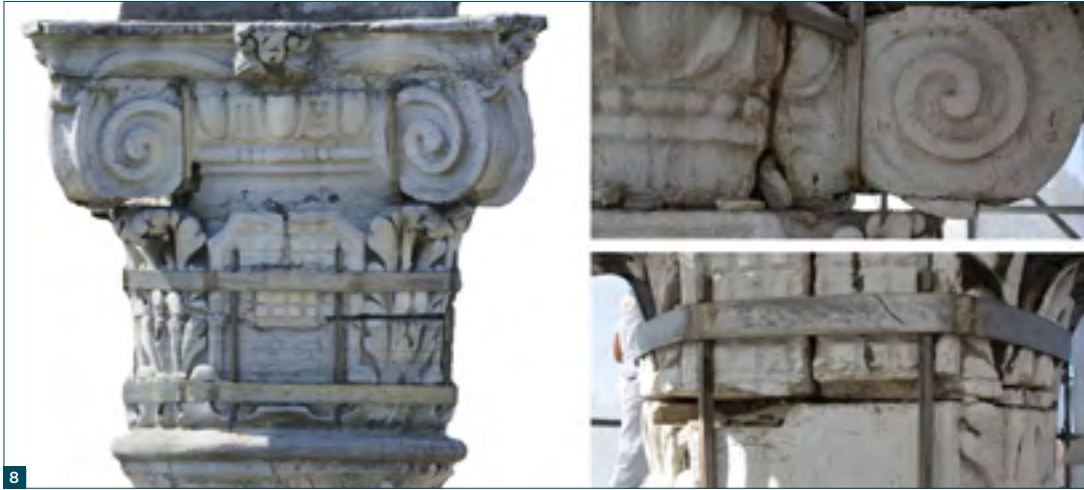
Figure 8: Capital of the column before the restoration works and the dismantling of each stone element.
