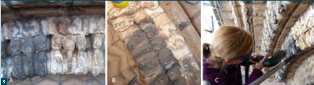
Figure 3: Laser cleaning, stone to the left before and to the right after (A), upper section of stone cleaned (B), cleaning in progress (C).
