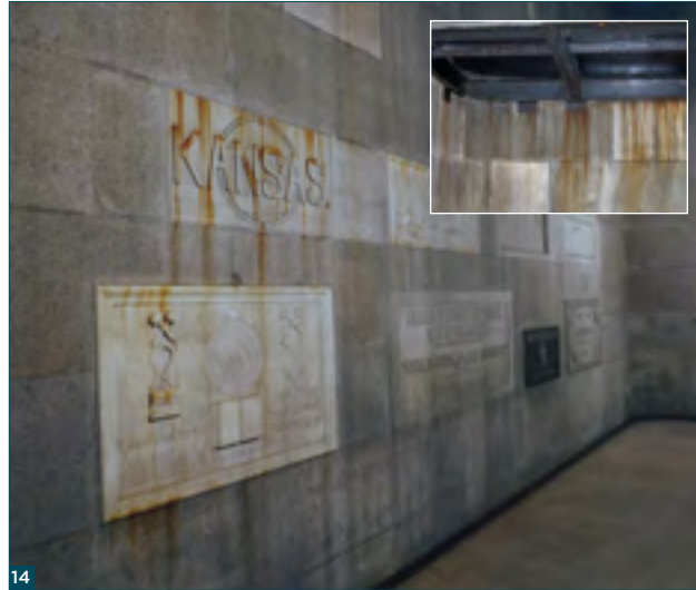
Figure 13: 220ft level following a period of drying; salts from cement grout behind stones, 2009.
