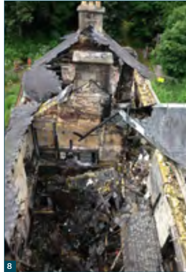
Figure 7: Inspecting the damage from the 'man-basket'.
