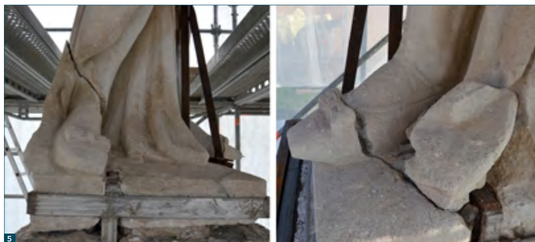
Figure 5: Statue of Ariosto disconnected at the base.
