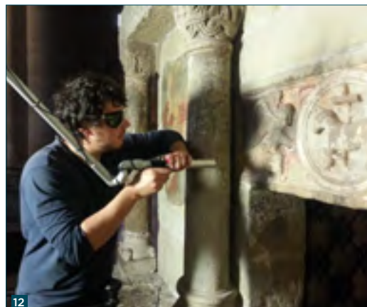
Figure 11 and 12: Resultant colour after removing dust was dark white.
