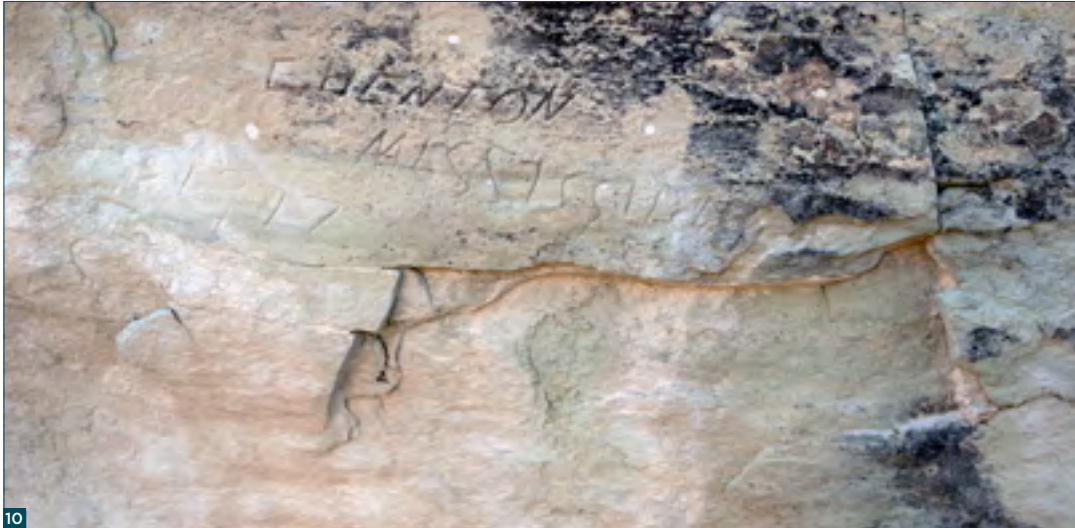
Figure 10: Example of previous treatment: pinning and edging, panel WW5. Pins are concealed with a natural hydraulic lime fill, which can be seen as white circles. Photo: UNM.
