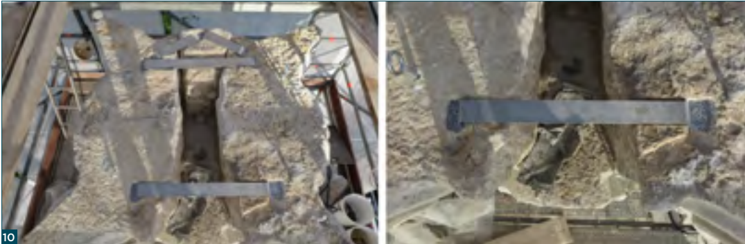
Figure 10: New cramps in duplex stainless steel connecting the various elements of the capital.
