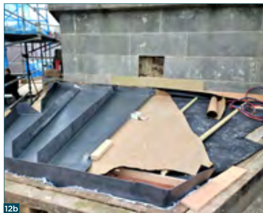
Figure 12: a) Monument conservation works in-progress, 2018. b) Replacement lead flat roof coverings in-progress, 2019.
