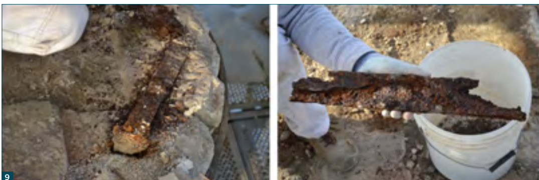
Figure 9: Oxidation of the internal fixtures between the parts which define the individual stone elements of the capital.
