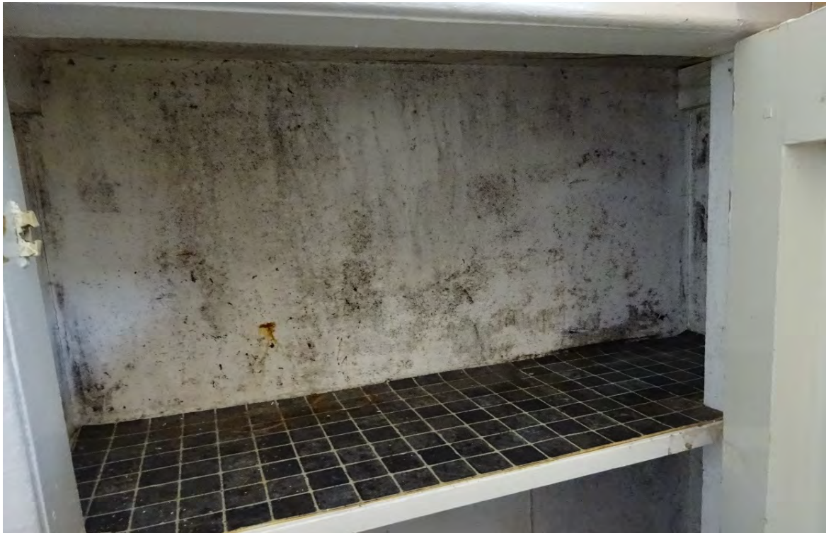
Figure 4. Mould growth in a press cupboard built into the masonry wall. As the wall is thinner at this point and therefore colder, it is a vulnerable point for condensation and associated mould growth.
