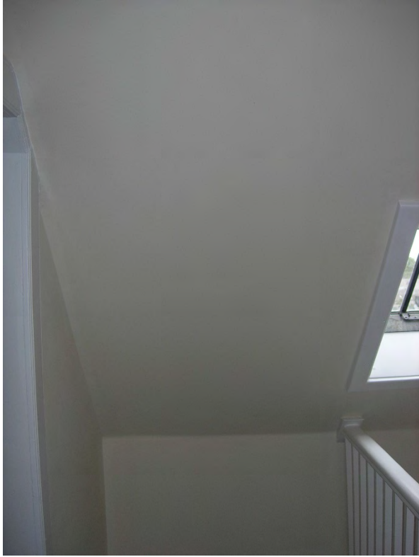
Figure 6. The new insulation was finished with plasterboard. This is the same area of stairwell shown in Figure 2, but following the works.
