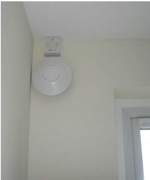
Figure 9. The new humidity controlled extractor ventilation system in the downstairs bathroom.
