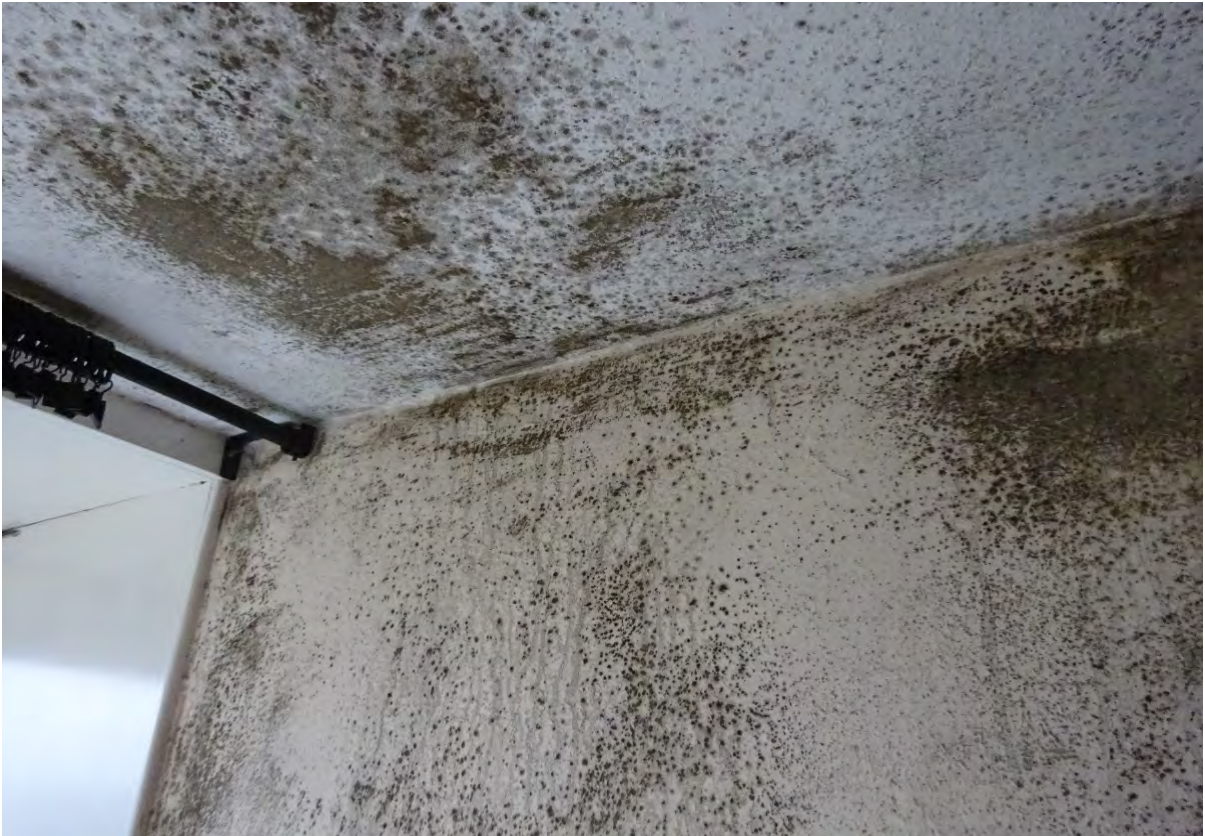
Figure 2. Previous insulation and ventilation schemes had failed, leading to substantial mould growth throughout the building.
