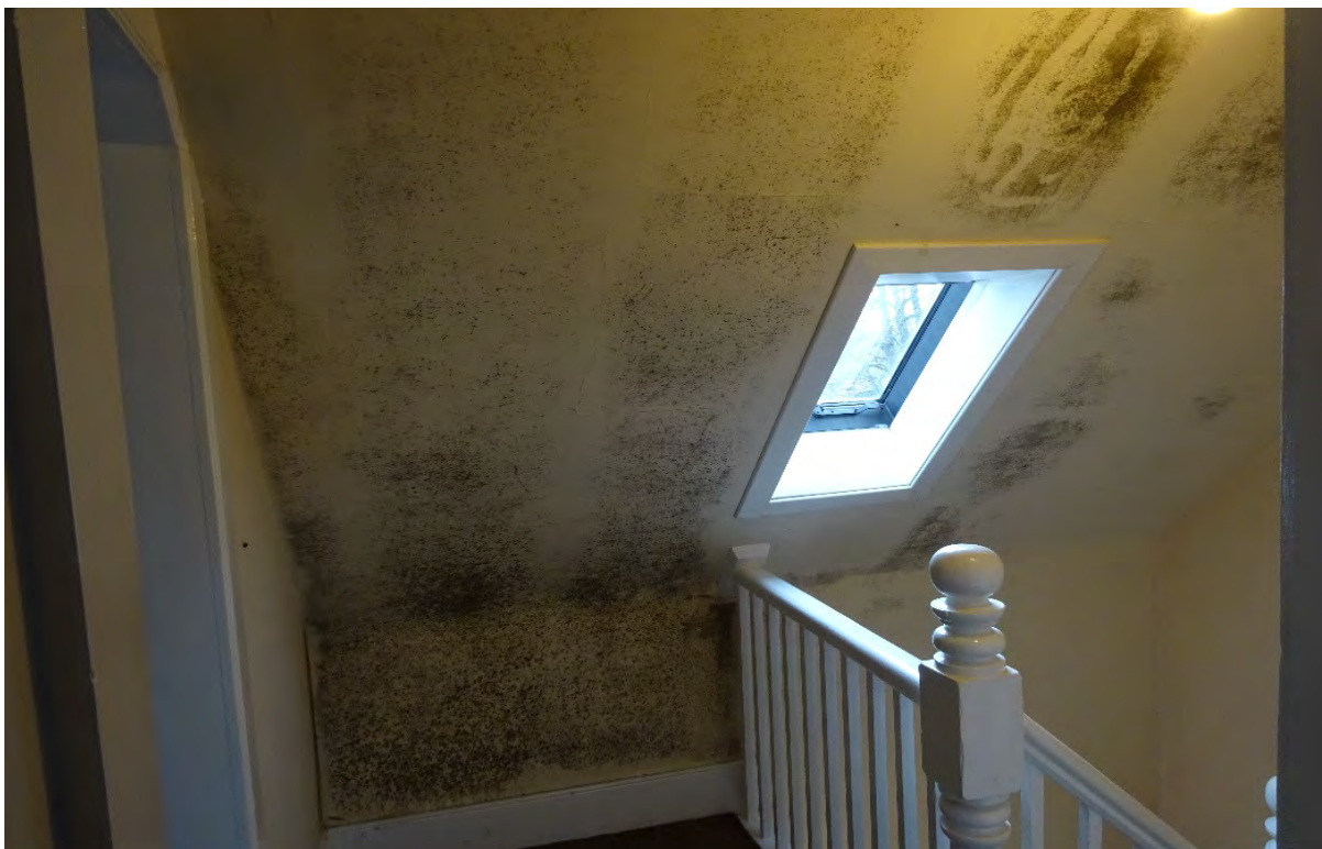
Figure 3. Substantial mould growth on the surface of the uninsulated stairwell roof space.
