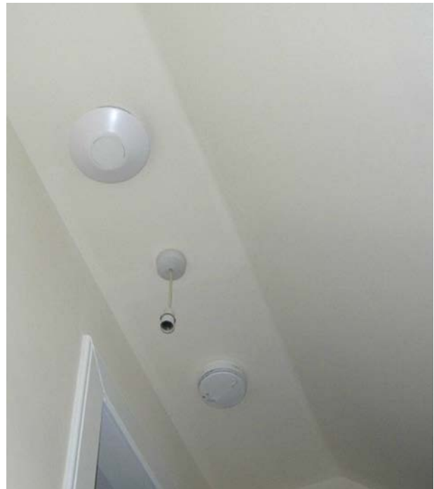
Figure 10. Humidity controlled extractor ventilation system in the stairwell which had previously suffered significant condensation and mould growth.
