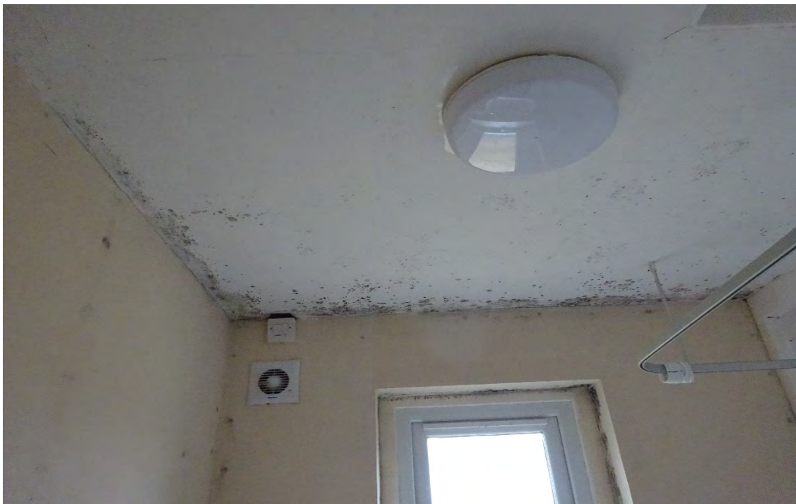
Figure 5. Mould growth in the bathroom, note the inadequate extractor ventilation system in the top left of the wall.
