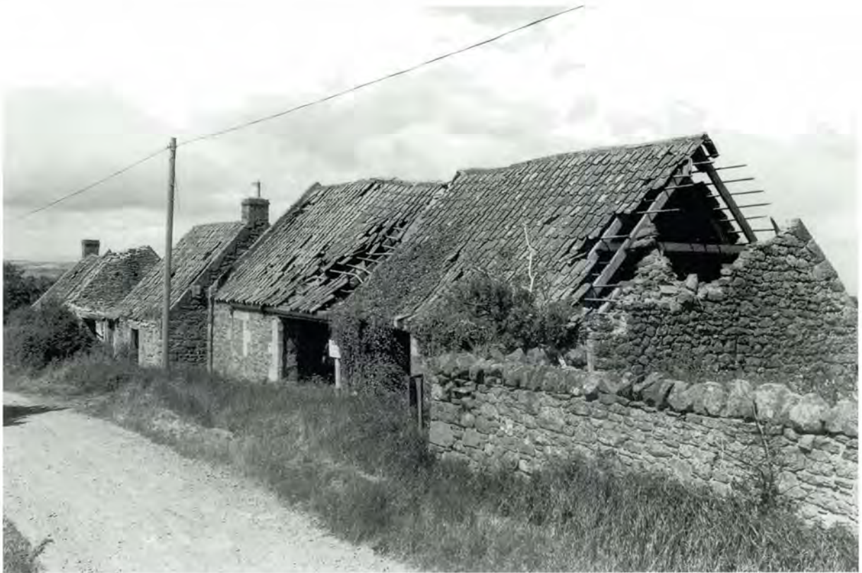
4 Derelict cottages at Loanhead, East Lothian.
