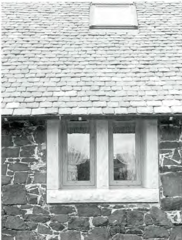
238 New side-hung casement windows in new openings (Gowanbank, West Lothian). The wood was still to be painted at the time of the photograph. Note also the diminishing courses in the slating and the low-profile roofline.
