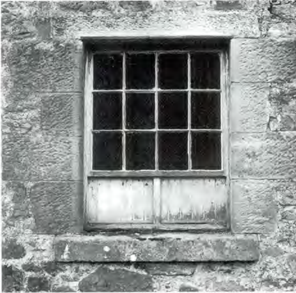
224 Fixed glazed upper light with double, inward-opening shutters below (Broadwoodside, East Lothian). This form of window was widely used in farm buildings and mills in the eighteenth and nineteenth century. The proportion of glazing to shutter varied.
