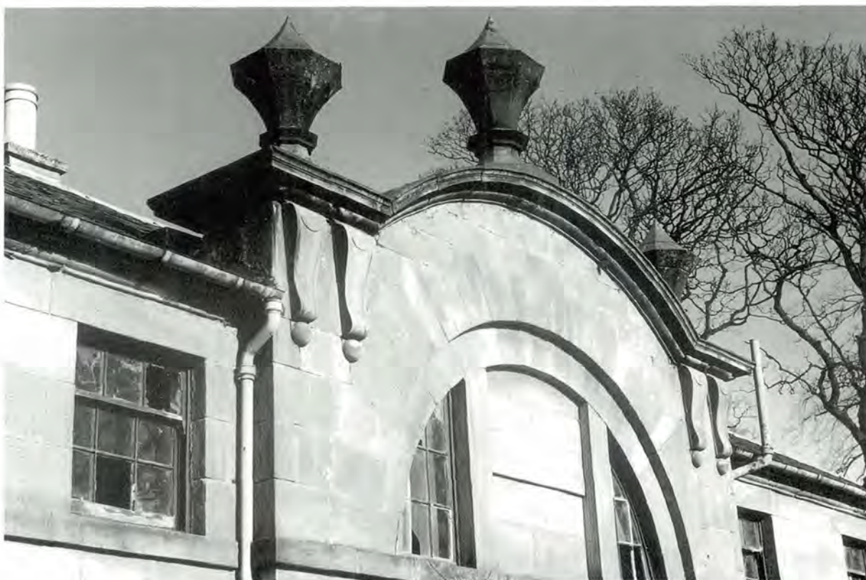
90 Dressed stonework at Binny House steading, West Lothian. Polished ashlar sandstone with very fine joints.
