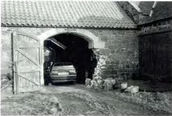
414 Redside steading during conversion; arched opening with double doors, and sliding door to engine house at right.
