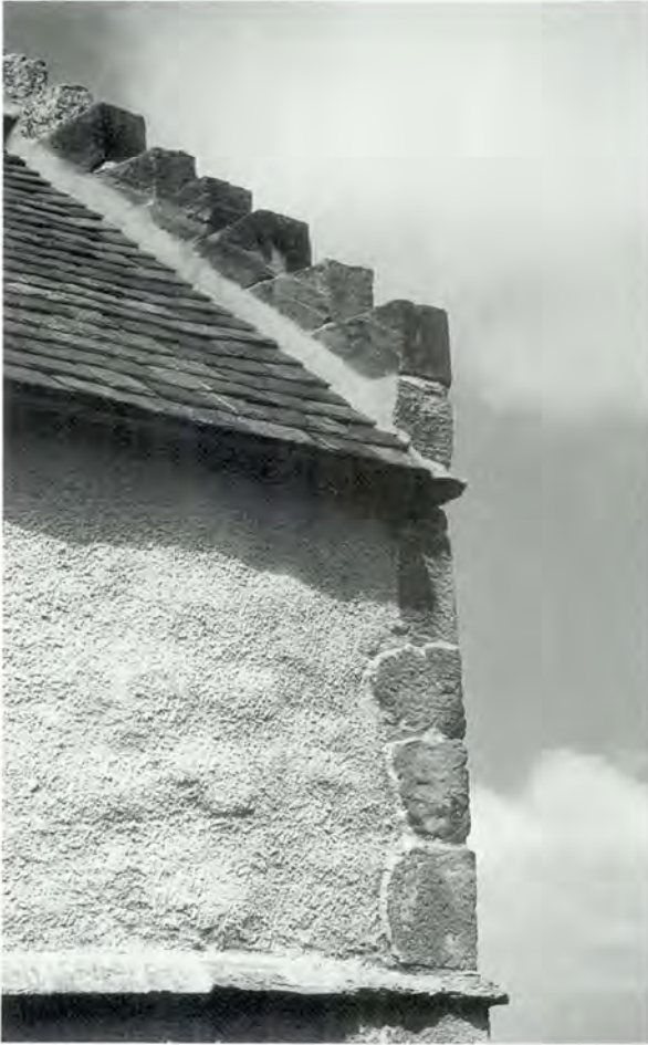
443 Skew detail between slating and crowstepped skew copes. There is a newly introduced lead underflashing to give additional protection against water ingress, but it is hidden beneath a mortar fillet, so that the detail does not appear to have changed.
