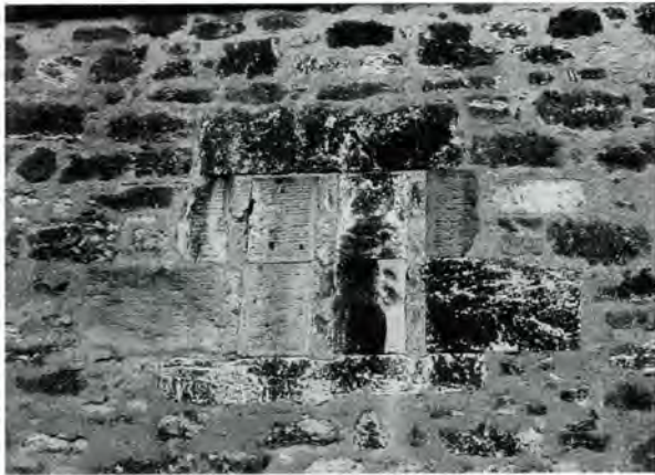
137 Harl pointing probably in hydraulic lime mortar, Brunstane, Edinburgh, causing damage to the face of the stone in places.
