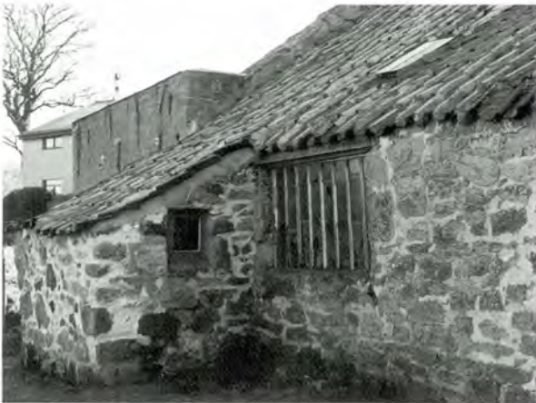
220 Fixed-light window (Cousland Smiddy, Midlothian). The vertical panes are held in place by metal window bars, probably zinc. Such metal-framed fixed windows are a distinctive feature of eighteenth and nineteenth century smiddies and workshops.
