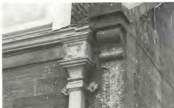
206 Cast-iron rainwater goods at Millbank Cottage, Midlothian. Ogee gutter, rectangular downpipe and classical detailing to the hopper.
