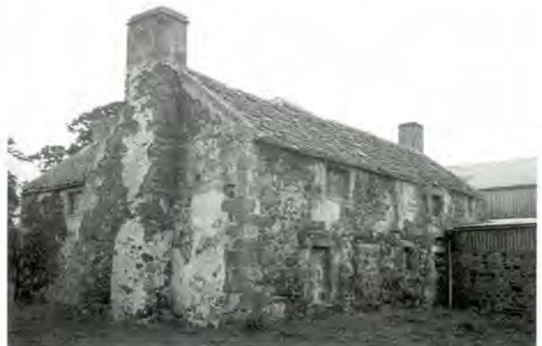
129 This lime harl to seventeenth-century Sydserf in East Lothian, was sparse at the time of the photograph and has since almost completely disappeared.
