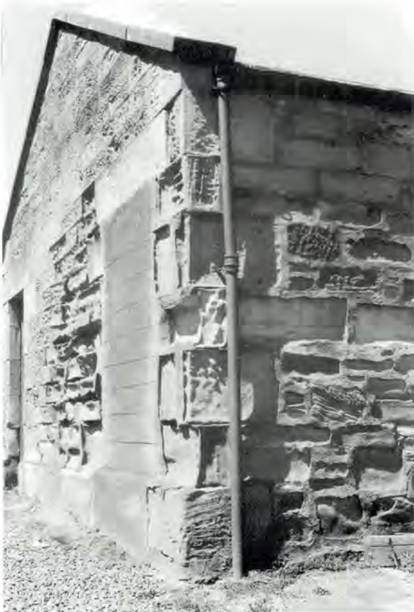
127 Hard cement pointing and render is contributing to accelerated decay in the softer adjoining stones (tooled ashlar sandstone masonry) at Thurston Home Farm, East Lothian.
