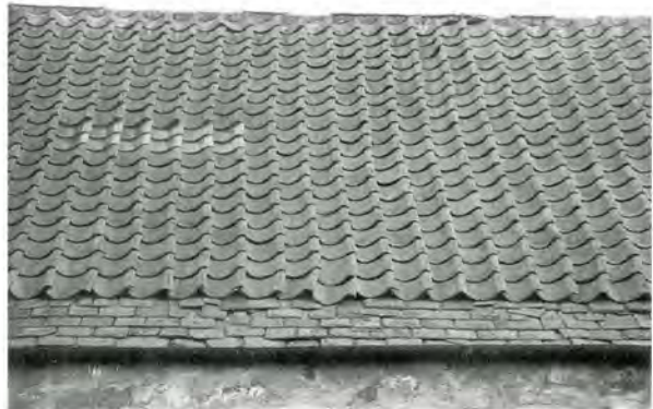
159 Slate easing courses and glass pantiles on a roof at Almondhill Steading, Edinburgh.
