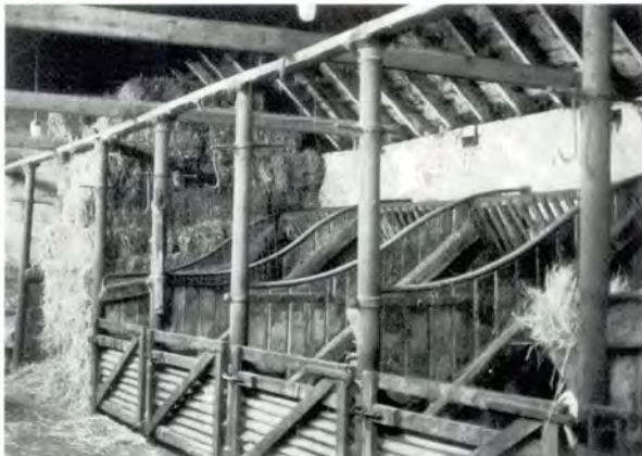
312 Stable interior (Kippielaw or Southside, Midlothian), showing trevises linked to the ties of the exposed timber roof structure, and hay racks.
