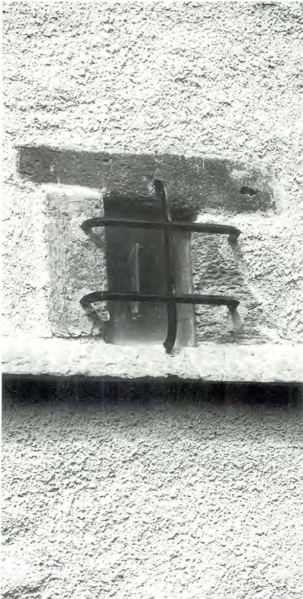
445 A wrought-iron grille has been provided at the window, reusing the original fixing points into the masonry, and glazing has been introduced behind it, set into the existing rebate.
