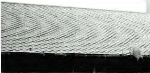
171 Half slating over a cattle byre and shelter shed at Hallhill, East Lothian.
