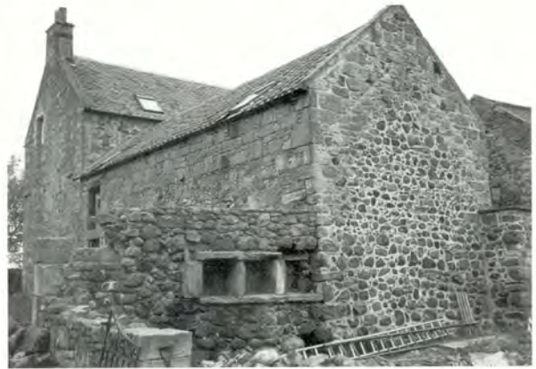
109 Evidence of three stages of masonry in this rubble gable at Hiltly, West Lothian. It has been recently repointed in lime mortar. Note the beeboles in the wall to the left.
