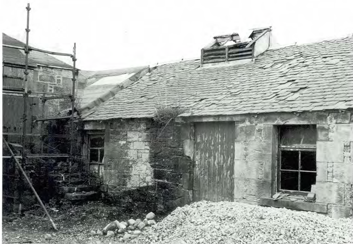
423 East end of the south courtyard front, adjoining the cartshed and granary (which is in different ownership), during conversion. The ridge vents have not been renewed.
