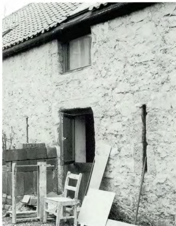
253 Stable door renewed to provide a window by double-glazing the upper half in a residential conversion (Easter Carriber, West Lothian). The ideal would have been to retain a boarded upper part, but this is a better compromise than many. Note the ventilation slits, unobtrusively glazed.
