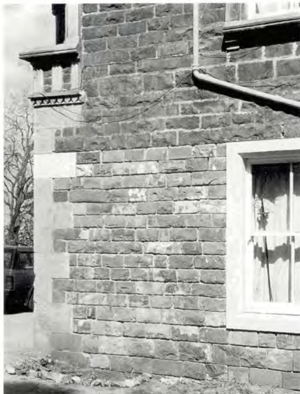
111 Reinstated infill to a garage door at Gowanbank farmhouse, West Lothian, reconstructing the original wall. The coursed, squared whin stones were recovered from the surrounding ground, where they had been lying half buried for many years. The joints have not yet been pointed up, hence the different appearance of the new masonry.
