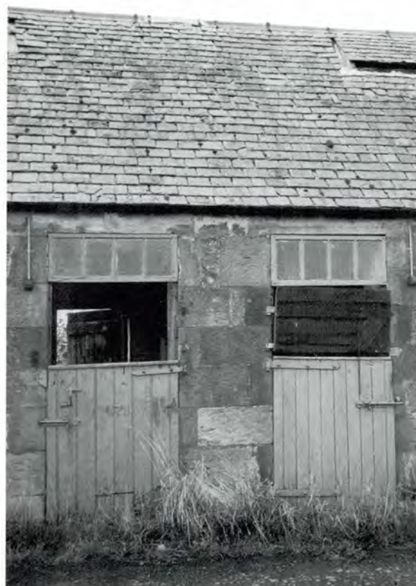
250 Stable doors (Almondhill, Edinburgh) with fanlights above, and missing/ replaced top sections of door. These doors open outward.
