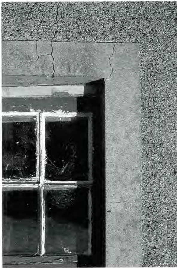
138 Cement render added in the twentieth century to an earlier building at Bridgend, West Lothian.
