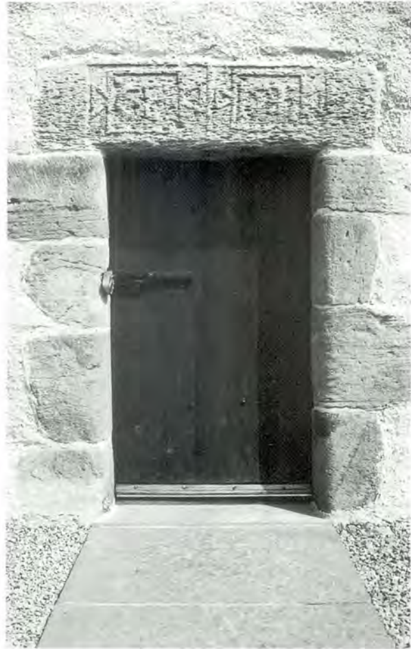
444 The boarded replacement door is similar to the previous one. There are Caithness slabs set into the gravel path at the entrance.
