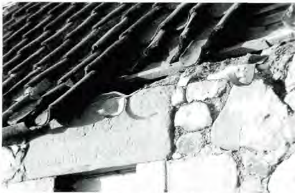
162 Eaves detail at Pottishaw, West Lothian; the provision of a rhone is not traditional, and it may have been added later. Sarking straps are used, but as there is no sarking, the fixings appear to be to the masonry or wallplate. Note the profile of the tile with a shorter upper roll than modern pantiles have.
