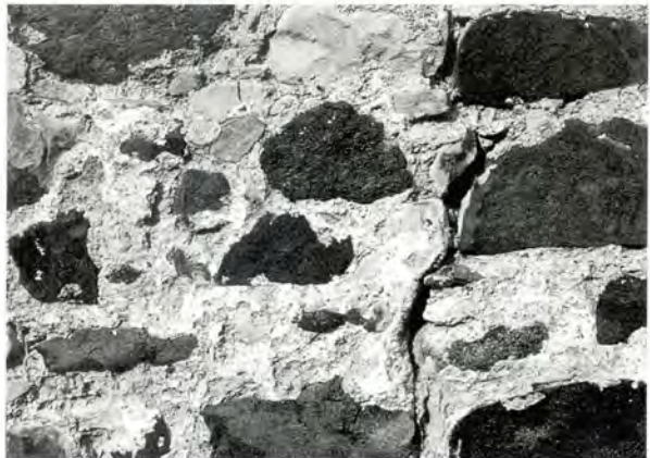
136 Detail of traditional harl pointing in lime mortar at Cauldhame, West Lothian.
