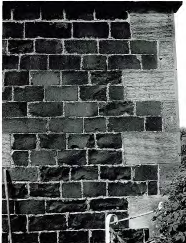
93 Coursed and squared whin at Ochiltree Mill, West Lothian, with droved ashlar sandstone quoins and window surrounds.
