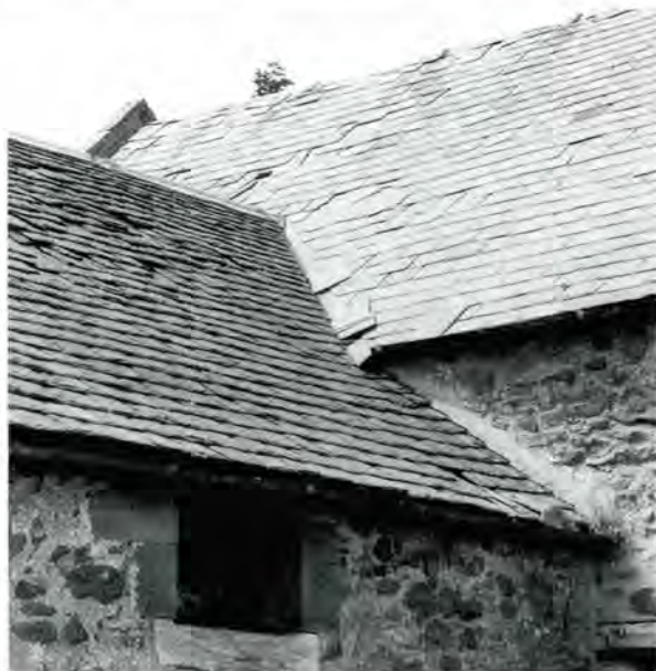
169 Slated roofs at Brunt, East Lothian. The slates on the left are Scottish slates, probably West Highland, while those on the right are probably Welsh. They are smoother, thinner, purpley-blue and more uniformly sized. Both roofs appear to be nailsick, the right being in a worse state.
