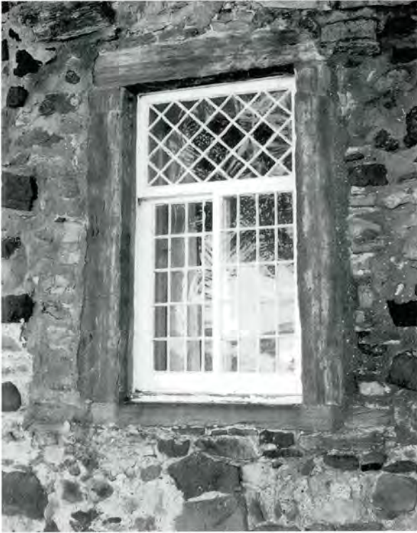
216 Rare horizontally-sliding sash and case windows at the Gardener's Cottage, Luffness, East Lothian, perhaps eighteenth century. The astragals may be zinc.
