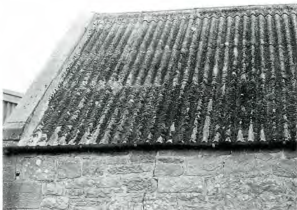
179 Corrugated asbestos roof, West Lothian. This material is particularly susceptible to the growth of lichens and mosses.
