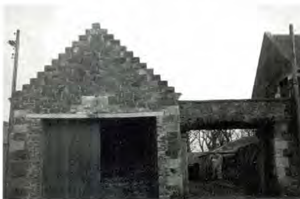
121 A DIY alteration, where an opening has been widened, using brick sides (bonded, but probably not tied into the stonework) and a too-slender lintel. The structure should have been more robust, and the detailing less mean in scale.
