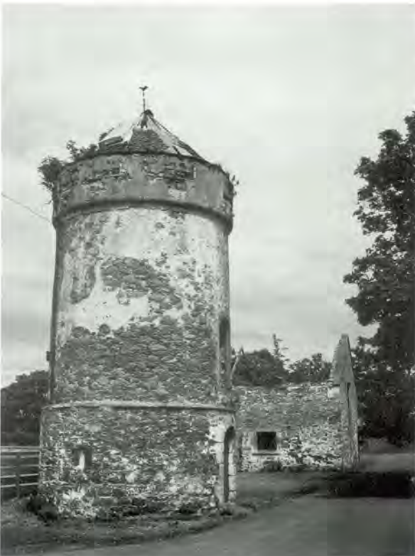
128 A thin traditional lime harl, in a very worn condition at the eighteenth century Rockville Doocot, East Lothian (possibly originally a windmill).
