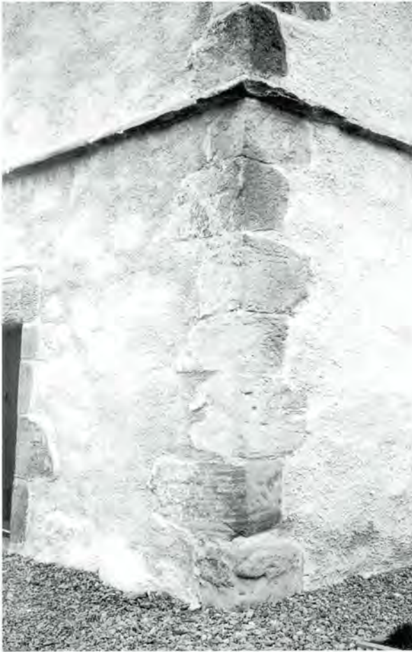
142 Recent lime harling at Athelstaneford Doocot (see case study 11.7) allows the form of the stonework behind to show through.
