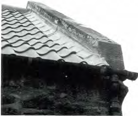
161 New skew detail at gable, using a lead cover flashing, of good quality but non-traditional. The traditional detail is a mortar fillet, and sometimes an undercut cope stone to shelter the junction.
