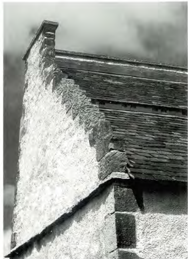
442 West gable showing new crowsteps, dressed stone unharled, and flight entry holes in the roof.
