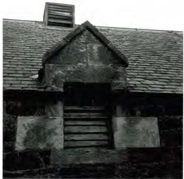
227 Fixed glazing (in three panes) with horizontal louvres below (East Fortune, East Lothian). This may be a later modification rather than being original.
