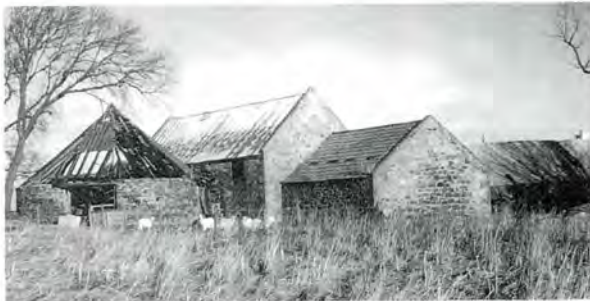
184 The horsemill at West Broadlaw, West Lothian, where deterioration of the roof has exposed the timber structure. (See illus 60 for a photograph of the building with the roof intact. Note also the loss of pantiles on the cottage, and their replacement with a sheet material).
