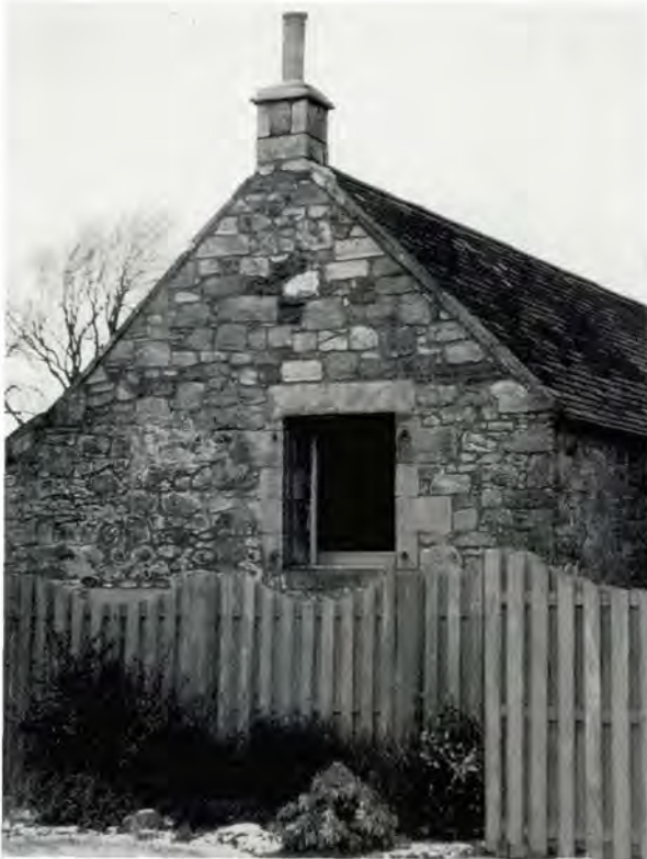
122 A partially reconstructed gable at East Whitburn Mains, West Lothian. The new build above the eaves line is evident. Although many of the stones have been reused, the build is different, with fewer small field stones and the masonry never brought to a level course. Compare this with the partially re-built gable at illus 386.
