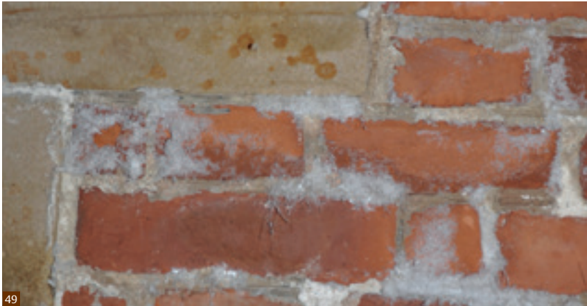
Fig. 49 Formation of salts on brick masonry due to migration of contaminated groundwater through a retaining wall.
