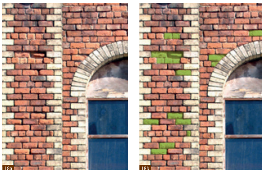
Fig. 18 Although the wall shown in image (a) needs fairly extensive re-pointing, the number of bricks which need to be replaced is small as highlighted in green in image (b).
