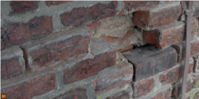
Fig. 30 Three bricks which had suffered severe decay have been removed, and the pocket which is left has been cleaned free of dust and debris. The brick which can be seen in the lower of the three courses is one of the three replacement bricks which will be inserted.
