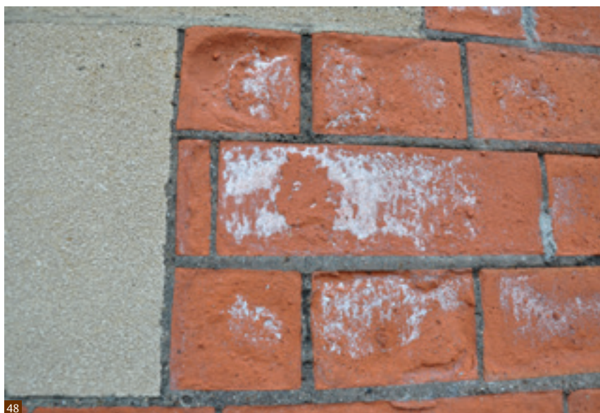
Fig. 48 Subflorescence showing as a white build up on the surface of brickwork. On this occasion it is likely to have been caused by the inappropriate use of cement re-pointing.
