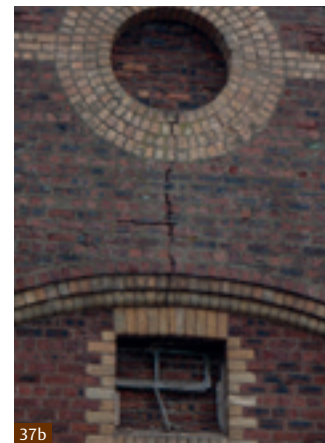
Fig. 37 With severe cracks such as this it will be necessary to cut out the fractured bricks and replace them. The addition of stainless steel reinforcement will almost certainly be advisable.
