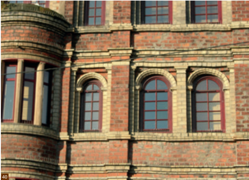
Fig. 40 Structural movement leading to distortion of walling, Glasgow. In situations such as this a structural engineer with experience in traditional masonry should be consulted.
