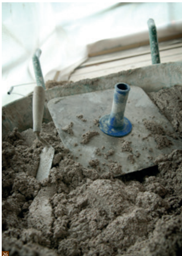
Fig. 26 Lime mortar with the consistency of modelling clay, with hawk and trowel ready to begin re-pointing work. If this mortar was being used for bedding bricks slightly more water would be used to give a less stiff mix.
