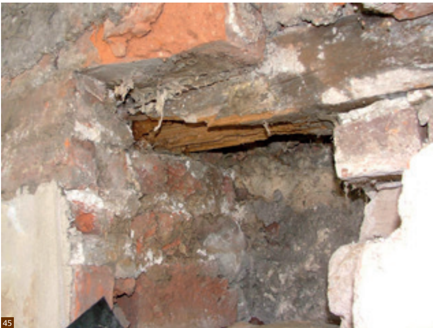
Fig. 45 Timber built into brickwork and showing advanced decay.
