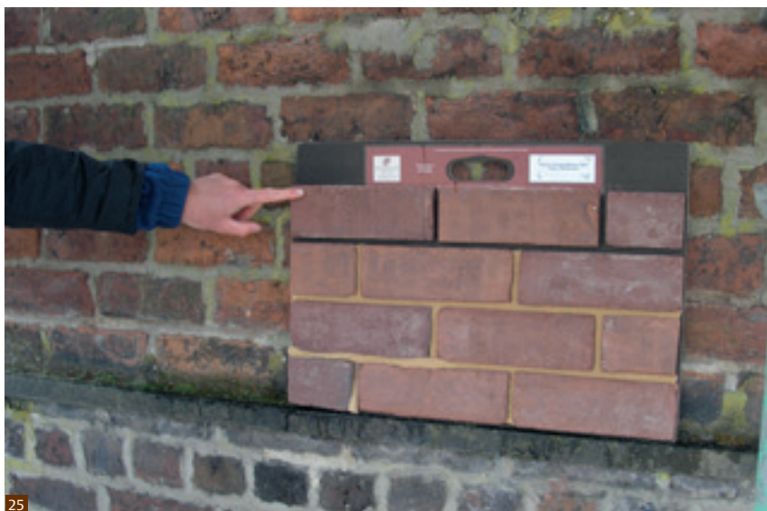
Fig. 25 Where new bricks are being manufactured for a repairs project these should be carefully assessed to ensure they match the characteristics of the originals.
