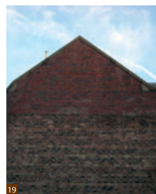
Fig. 19 An example of facing bricks on an exposed elevation with common brick on the lower parts which would have originally been protected by a now demolished adjoining building, Stirling.
