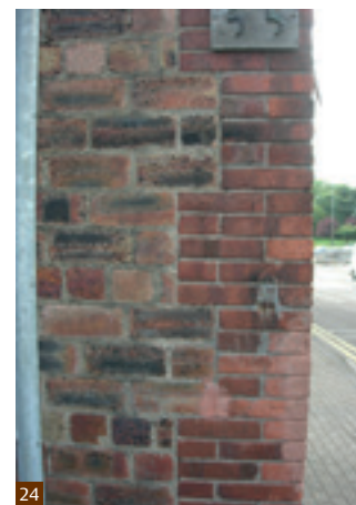
Fig. 24 Example of block bonding on an area where facing bricks meet common bricks.
