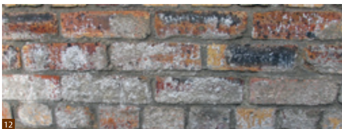
Fig. 12 Efflorescence on the surface of bricks caused by salt leaching from inappropriate cement re-pointing.
