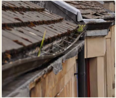
Fig. 6: Tenement gutters need to be resilient as they are subject to high winds and need to deal with a lot of rainfall from large roofs and increasingly wet winters. Plastic gutters and downpipes are not really up to the job.
