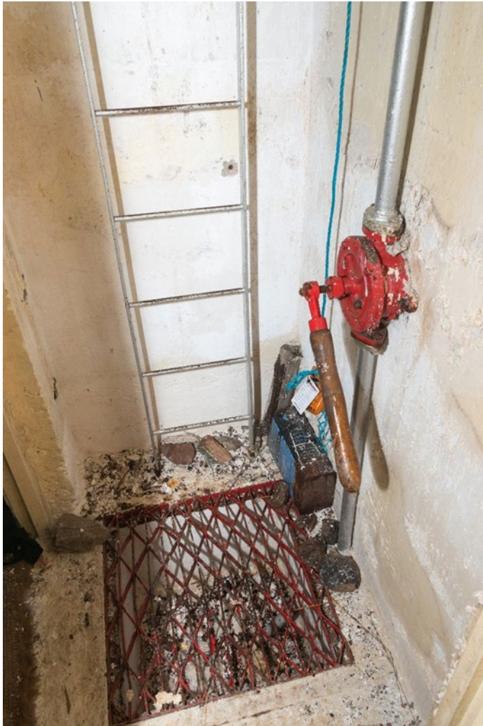
Figure 4: Image of entrance area to ROC post showing the 'shower tray' and hand-pump. © Crown Copyright HES.
