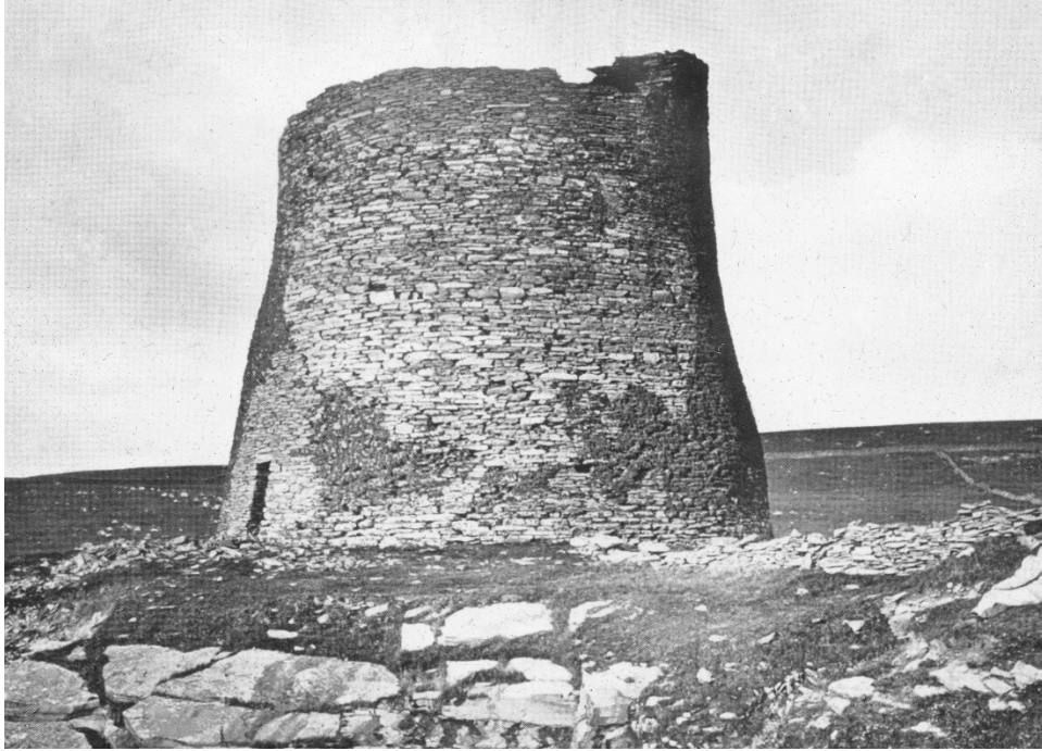
Paterson's 1919 photograph, clearly showing rebuilding above the entrance but still with a considerable amount of consolidation to be done on the walls, and the wall-head work apparently not yet done. HES collection – SC 1330617
