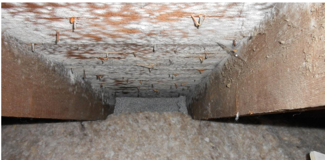
Fig. 10. White mould on the roof slope, caused by insufficient ventilation
