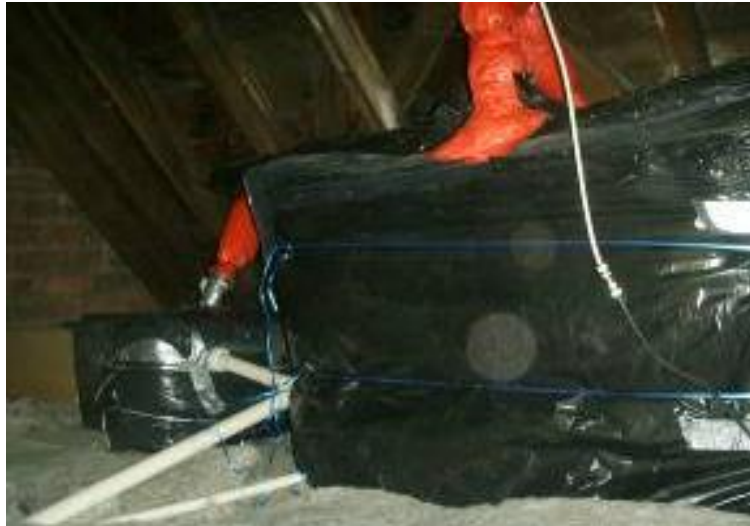
Fig. 9. The water tank and pipes were insulated top prevent freezing.
