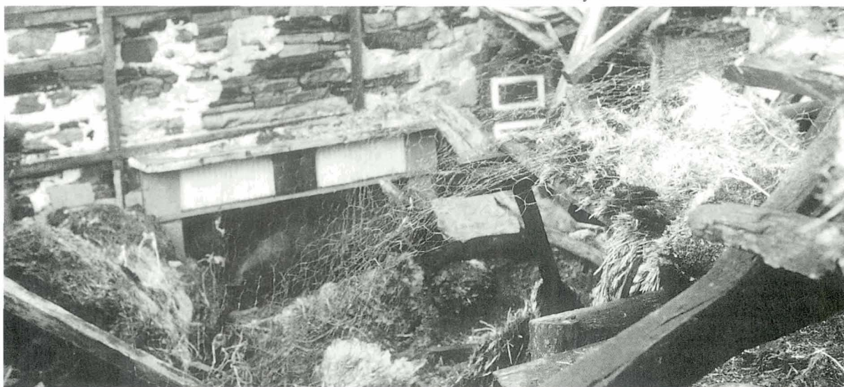
Up to 1m of organic material can accumulate after the collapse of the roof. (Gimps, Orkney 1996 see section 6.4)
