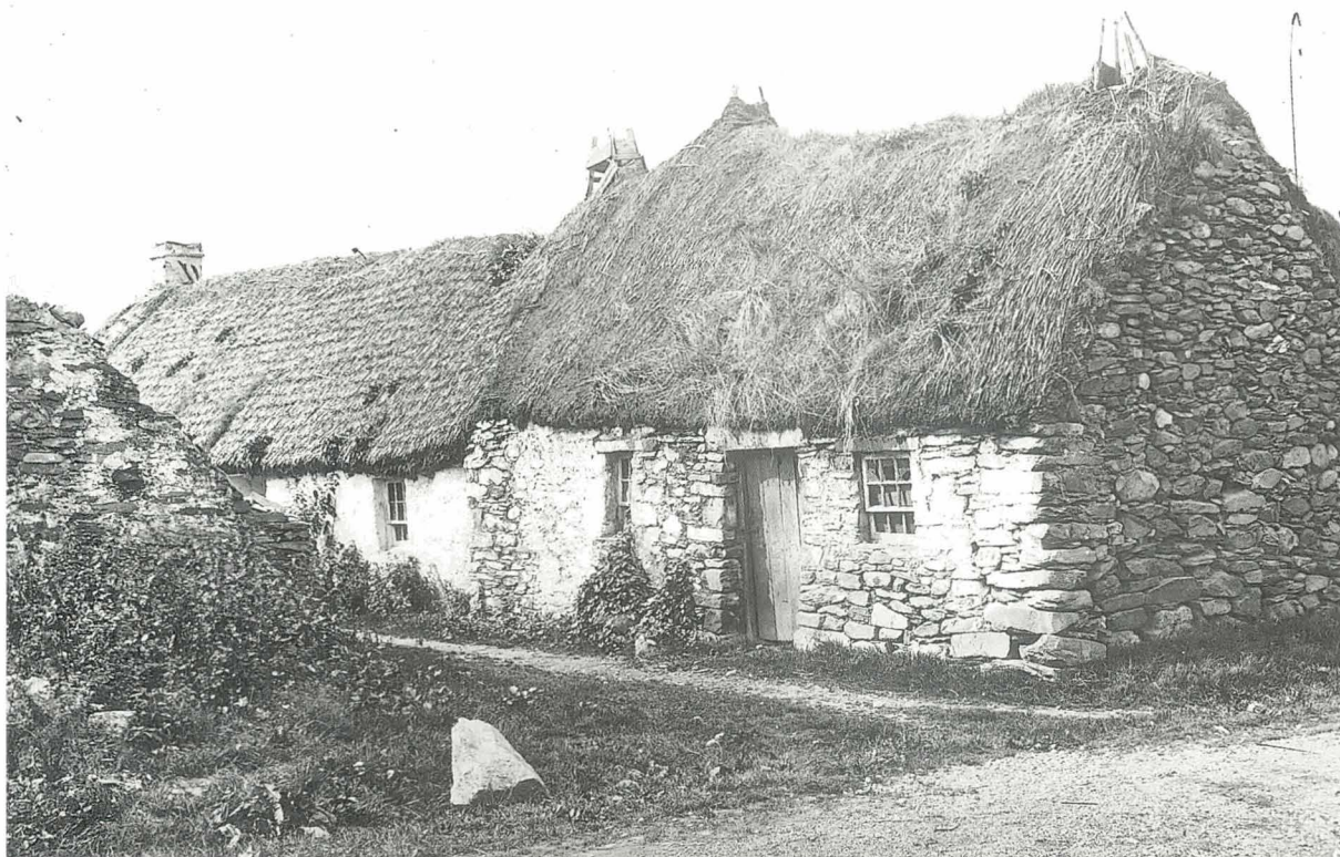
Two Highland cottages, at Luss, Loch Lomond. Different thatching techniques are shown on adjacent buildings. The house on the left is probably a bracken thatch, the horizontal lines being formed by the blackened basal parts of the stipe exposed on the surface. Close to the apex wand and scob have been used as a fixing. The house on the right is in a much poorer condition and appears to have a coarse material such as bracken close to the skewers but other parts of the roof look more like cereal straw. (G.W.W. Aberdeen University Library F4310)
