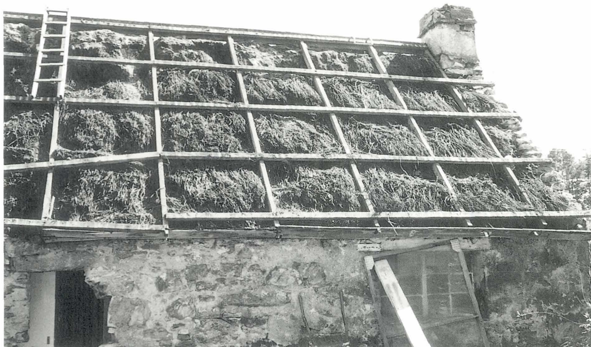
Johan Cottage, view of the north face of the roof. (S. Whymant)
