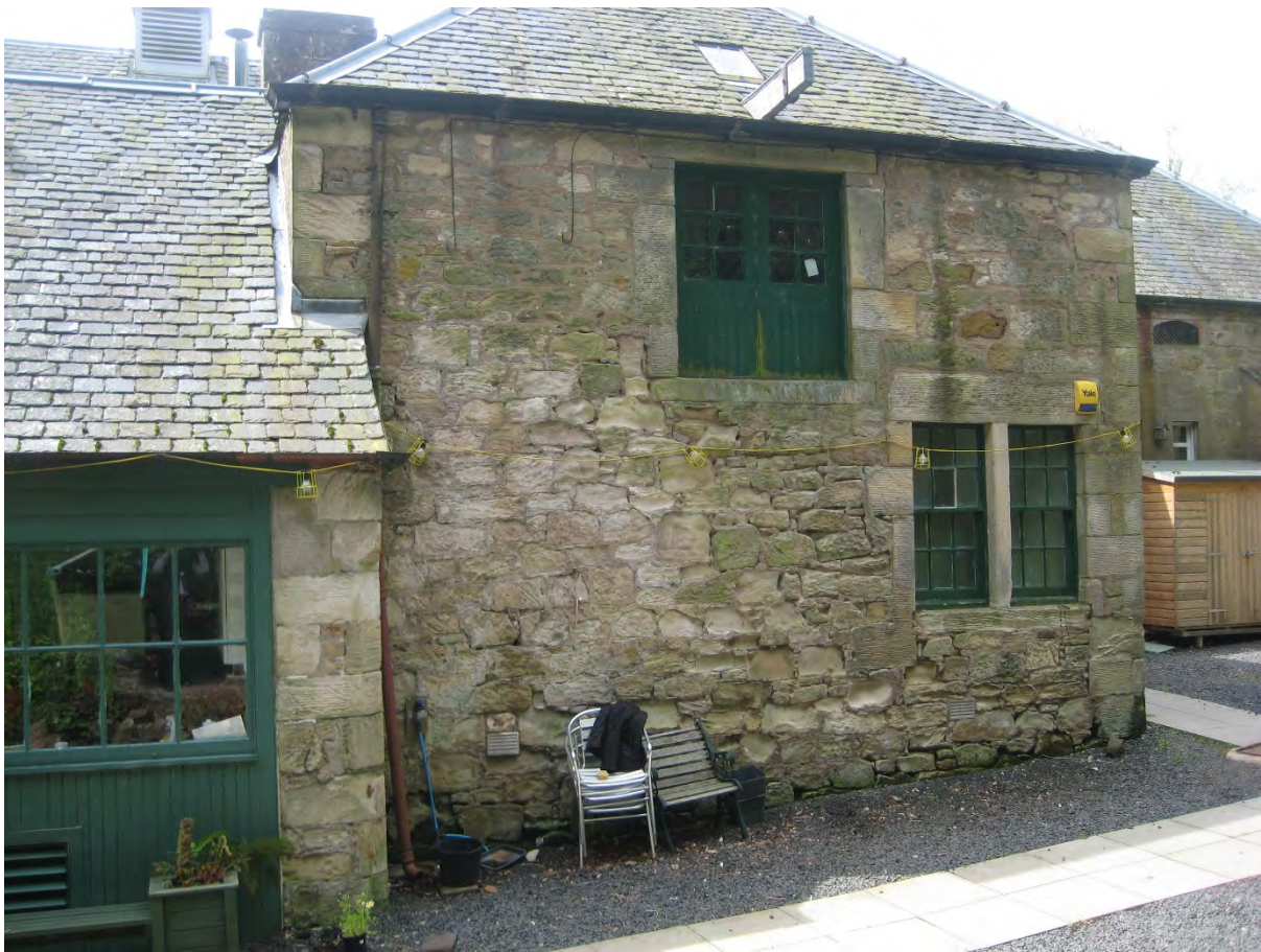
Figure 1. View of the north elevation of the stable block where the works took place. Note the poor condition of the stonework at lower levels.
