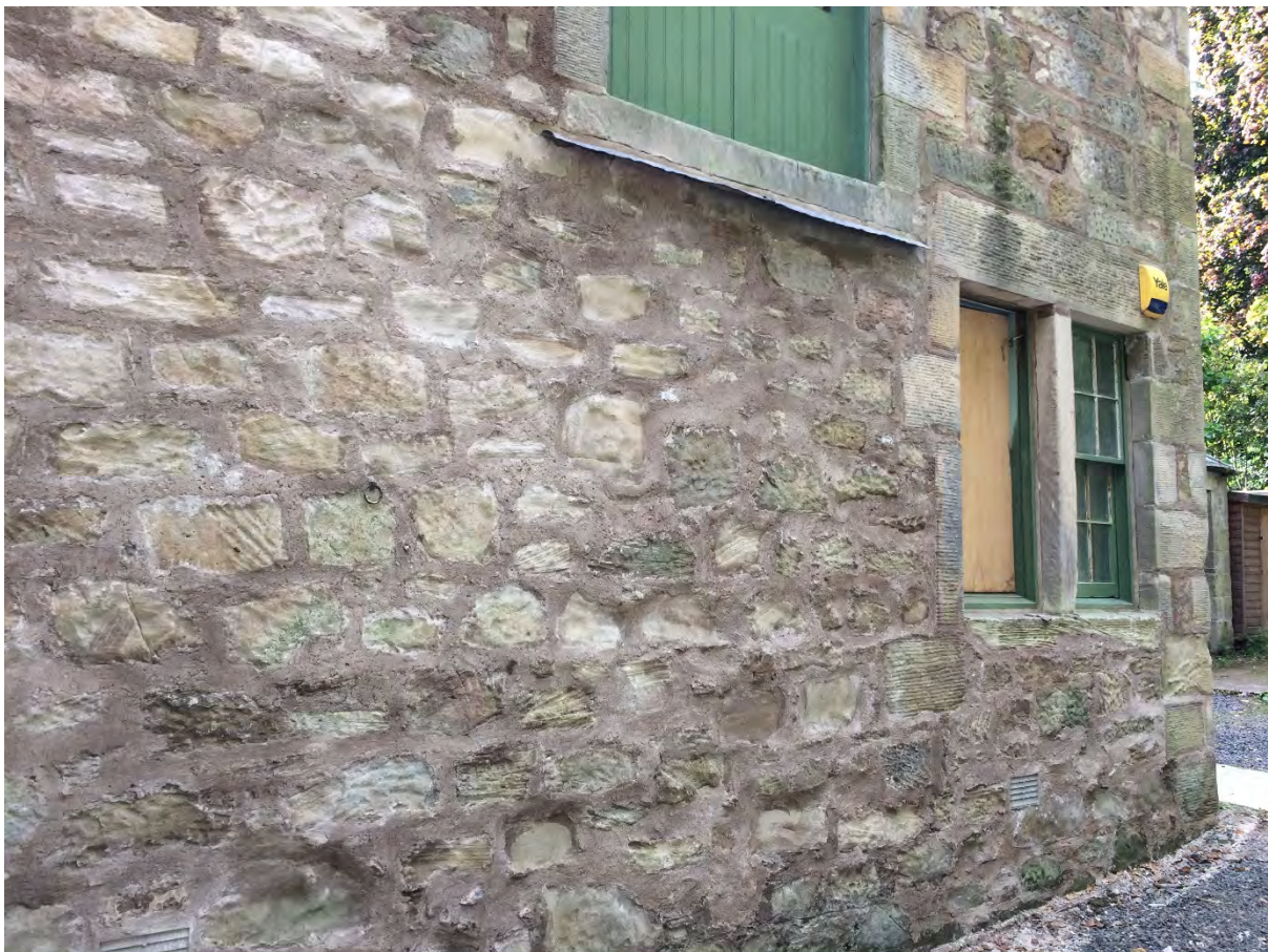
Figure 7. The replaced stones and the finished lime mortar surface following the final scrape back of the mortar.
