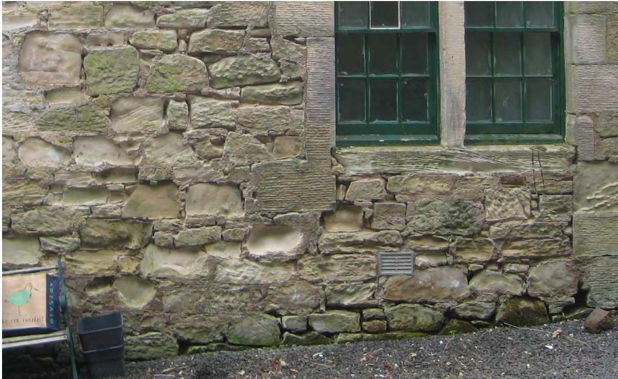
Figure 3. Extensive stone decay at the lower part of the wall. Greening of the masonry due to damp at the base of the wall can be seen bottom right.
