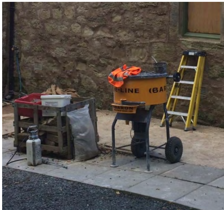
Figure 5. The small forced action mixer used for the preparing the hot-mixed lime mortar.
