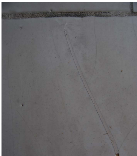
Fig. 8: Missing pointing should be replaced to avoid water ingress and further deterioration
