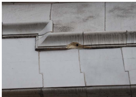
Fig. 4: In this faience clad structure spalling of the material has revealed deterioration of the anchoring system
