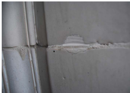
Fig. 3 Small areas of material spalling can be repaired using a fill of hydraulic lime mortar
