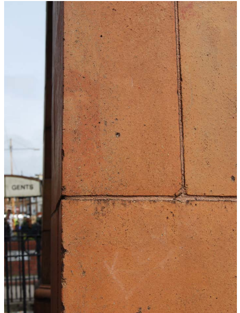
Fig. 6: Re-pointing work should be undertaken using lime based mortars and can be coloured to blend in with the architectural ceramic.
