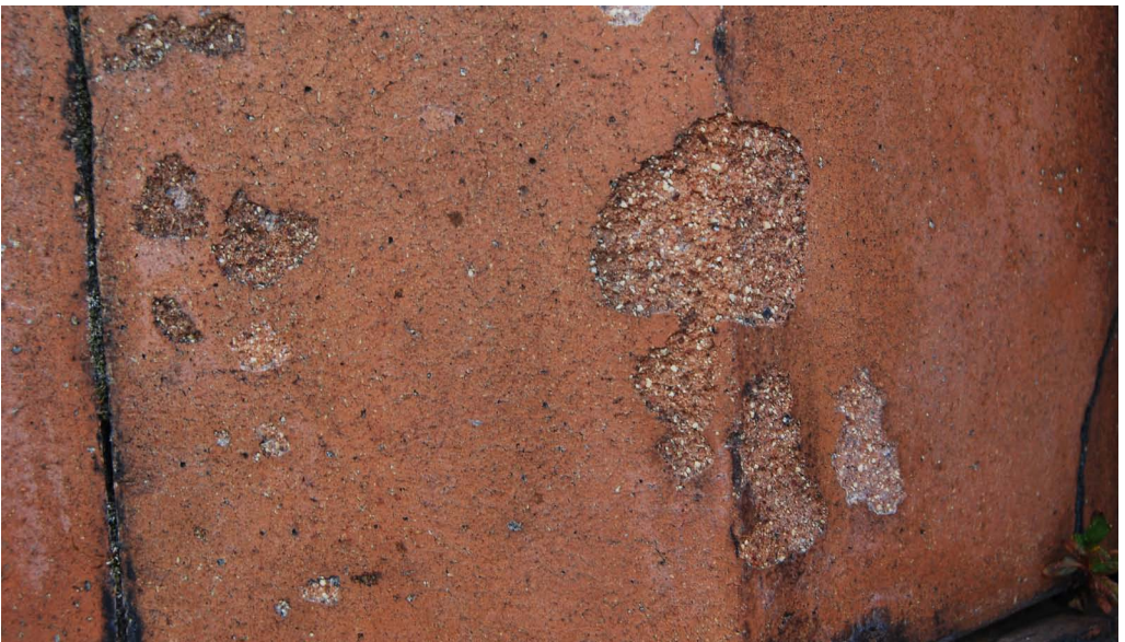
Fig. 2: Spalling has led to the loss of the terracotta fireskin leaving the material vulnerable to further decay
