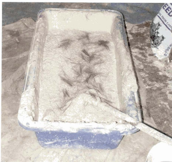
Illus 24. Coarse stuff; lime plaster mix with animal hair ready to be mixed in. © William McVey
