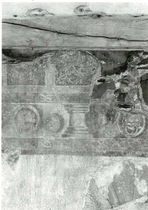
Illus 46. Amisfield Tower, Dumfries and Galloway; late C16 painted decoration on flat plaster showing lion heads and other medallions, framing with columns, floral enrichment etc, motifs which recurred in moulded plasterwork. © Crown copyright RCAHMS
