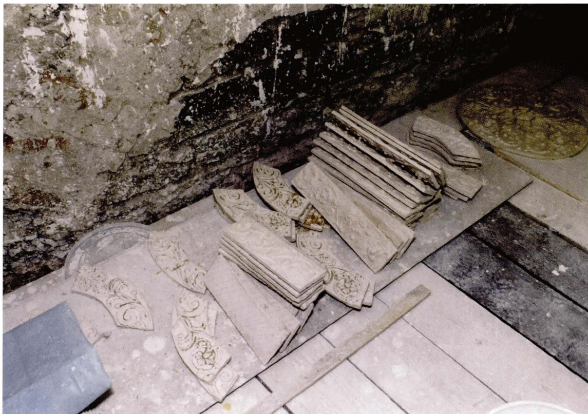
Illus 41. Cast rib enrichments ready for application to the soffit of ribs. © Crown copyright Historic Scotland
