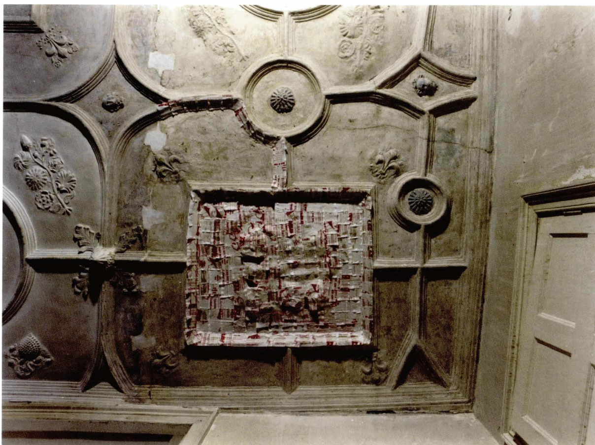
Illus 17. Croft-an-Righ, Edinburgh; damaged plasterwork temporarily supported by water-based adhesive paper. © Crown copyright Historic Scotland
