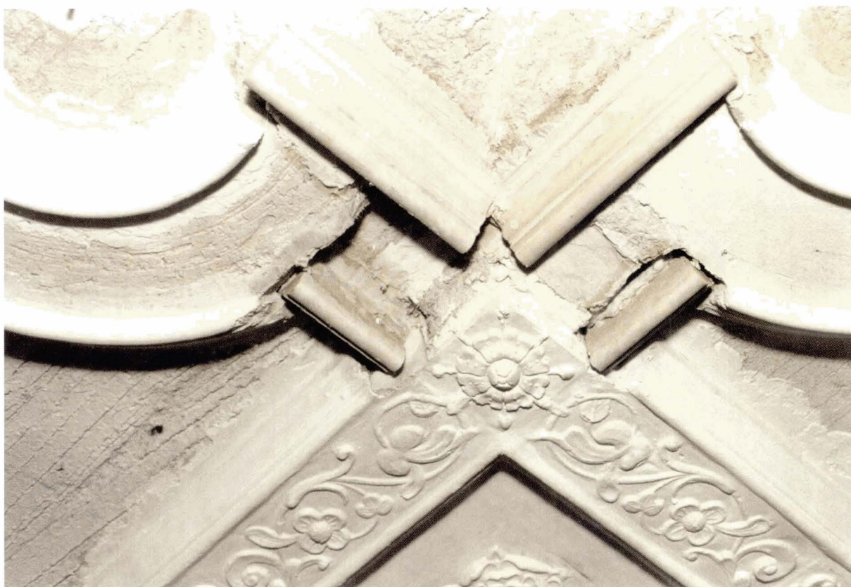
Illus 36. Pre-cast sections of rib have been inserted to link in-situ run ribs. The junctions will be finished by hand. © Crown copyright Historic Scotland
