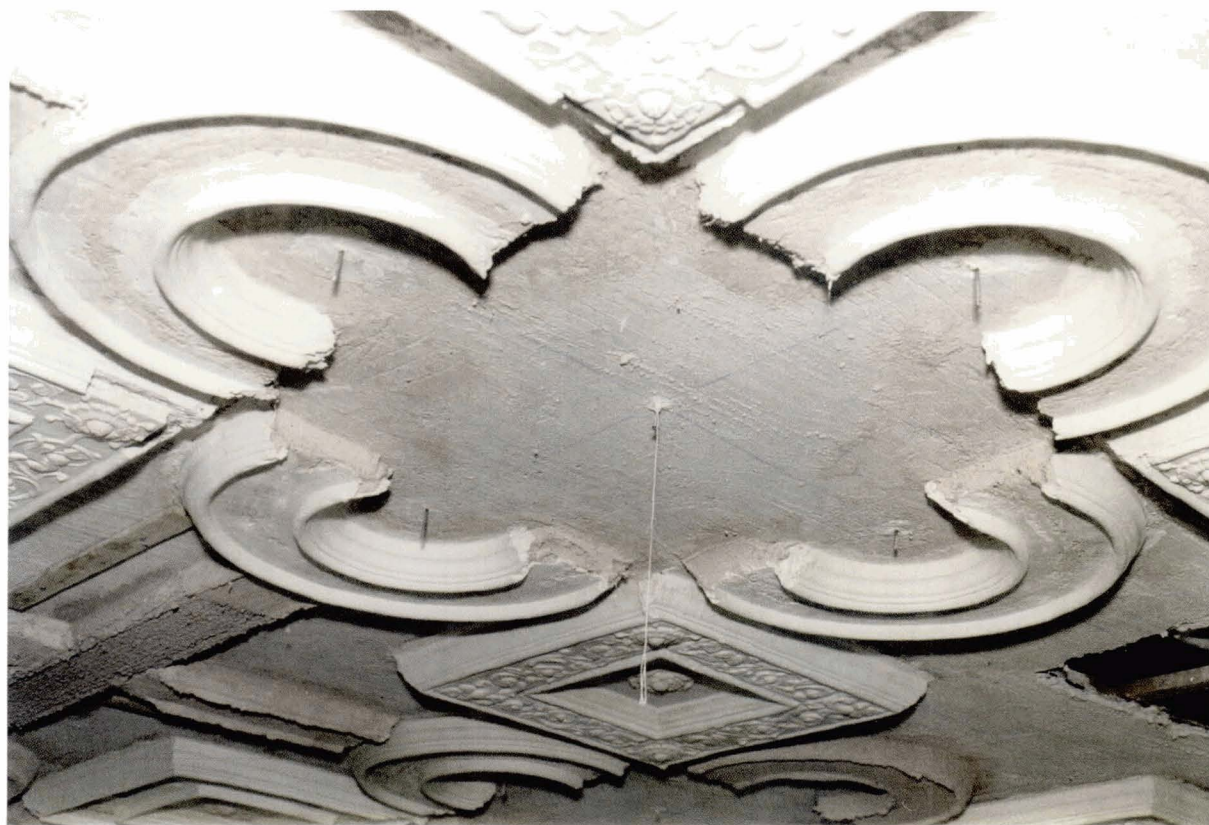
Illus 35. The finishing coat has been added and run in-situ to semi-circular mouldings. Nails and string at centre points provide guidance. © Crown copyright Historic Scotland
