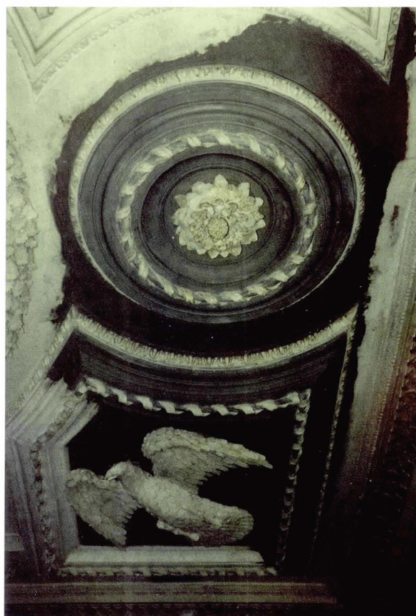
Illus 26. Thirlestane Castle, Scottish Borders; restoration of missing and damaged surface decoration (run mouldings and cast/ modelled applied decorations). The finished ceiling is seen after the repair. © L. Grandison and Son
