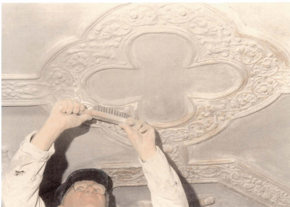
Illus 44. Crawfurdland Castle, East Ayrshire; brushing down the ceiling to remove dust and old limewash in preparation for renewing limewash. © William McVey
