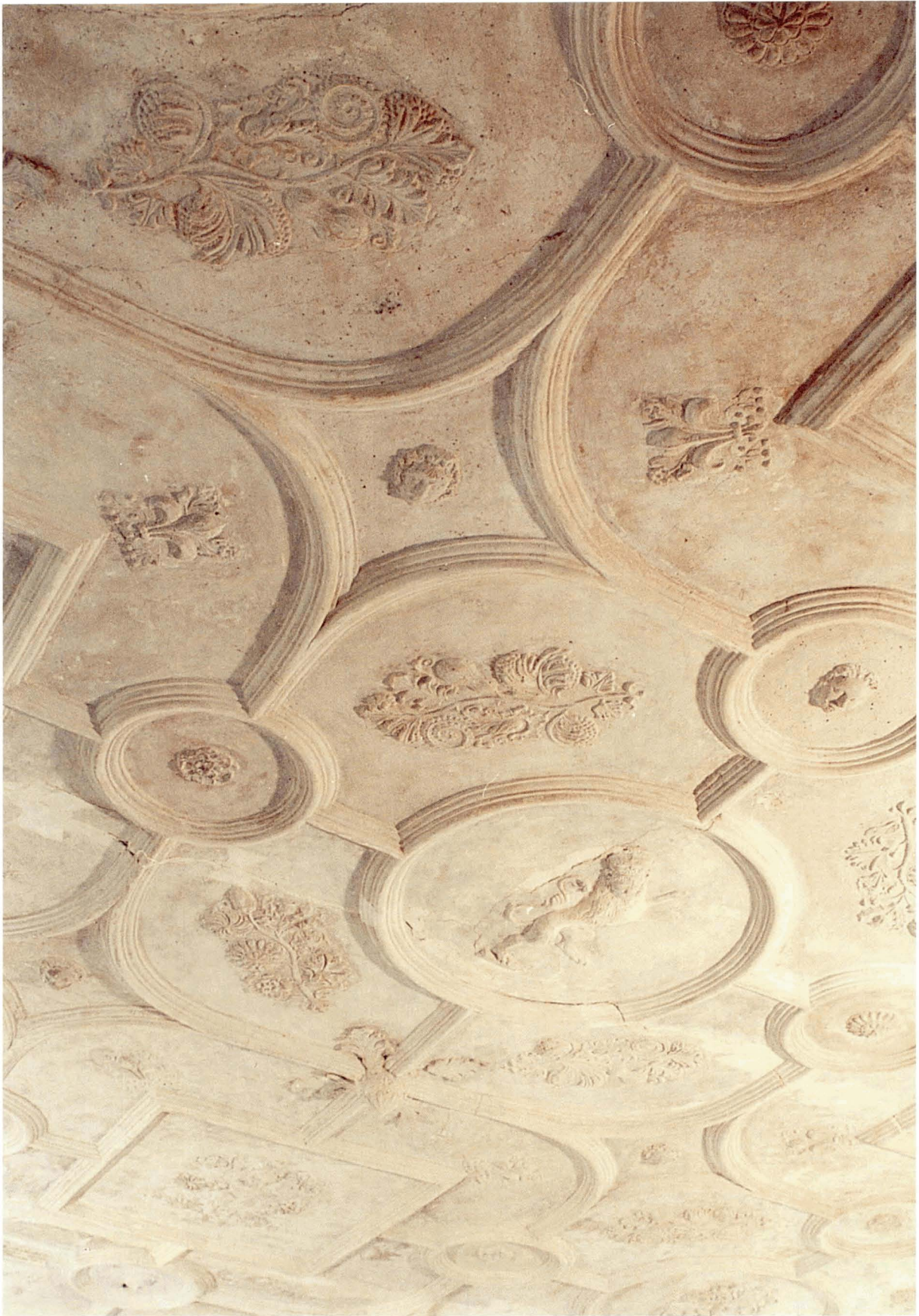
Illus 43. Croft-an-Righ, Edinburgh, moulded plaster ceiling at first floor with reliefs of animals, figures, fruit and flowers. © Crown copyright Historic Scotland
