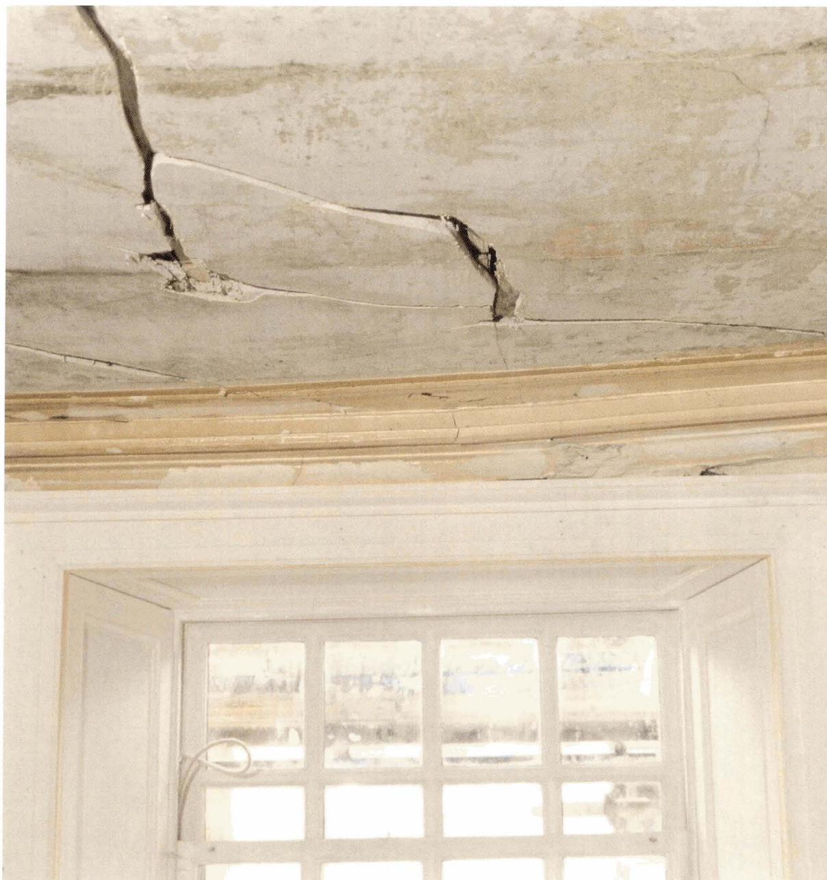
Illus 8. Sandgate, Ayr (later C17 or C18); damaged plaster, with cracks cleaned out ready for refilling. © William McVey
