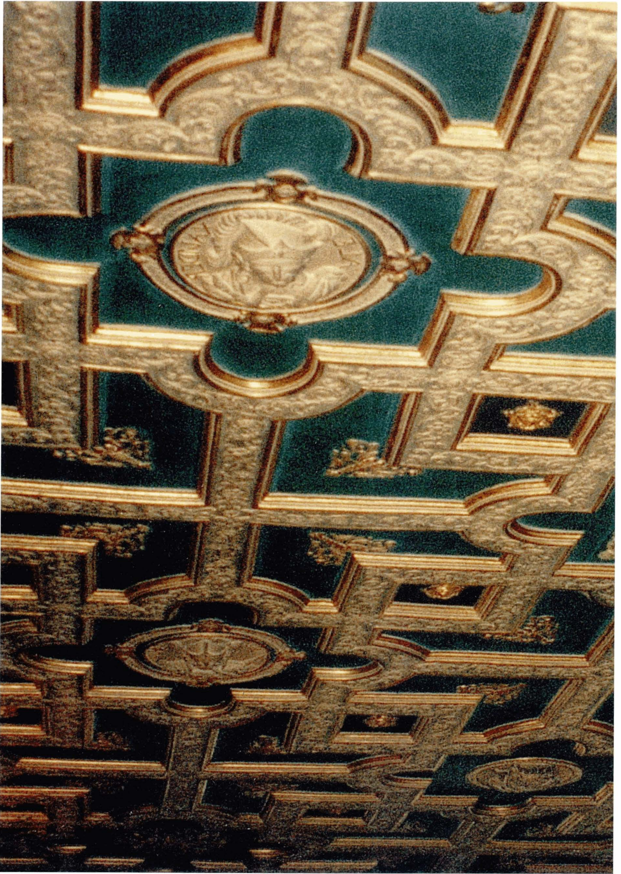
Illus 1. Balcarres House, Fife, first floor hall ceiling, c1630. © Crown copyright Historic Scotland
