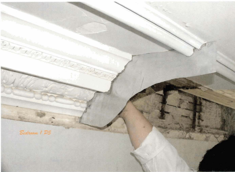
Illus 31. Taking a profile from the original cornice in order to renew part of it (in this example the plasterwork is much later). © William McVey
