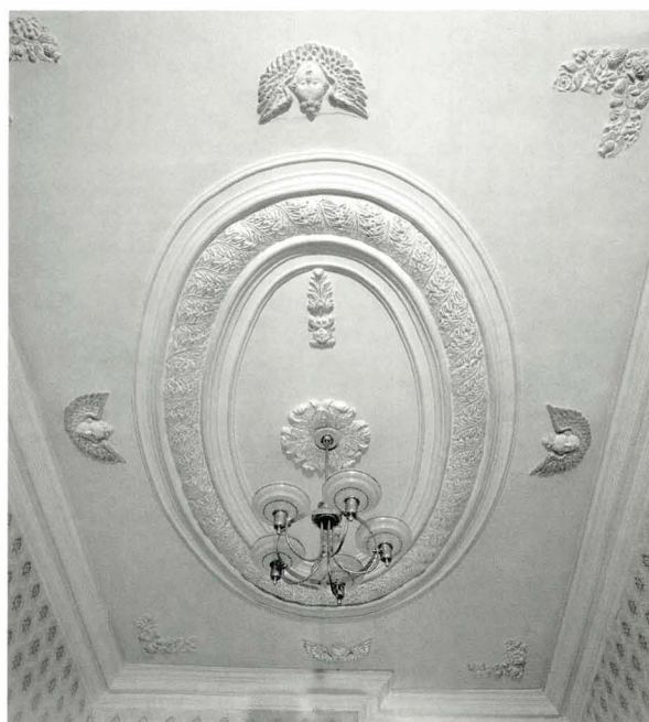
Illus 63. 341 High Street, Kirkcaldy, Fife (c1672); the oval panel was a new fashion, as was the use of a single central panel. © Crown copyright RCAHMS
