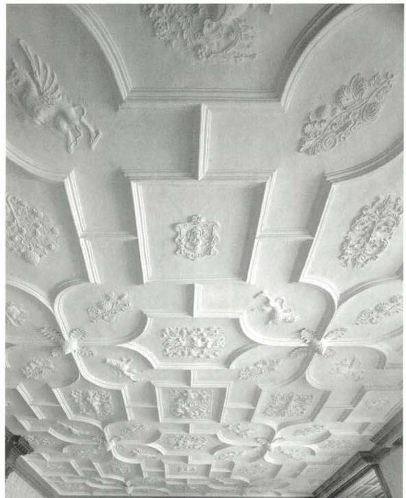
Illus 6. Newbattle Abbey, Midlothian; the library ceiling, probably 1620s or 1630s, with a layout based on a different arrangement of squares and quatrefoils. The run mouldings forming the ribs are narrow and have no additional decoration. © Crown copyright RCAHMS
