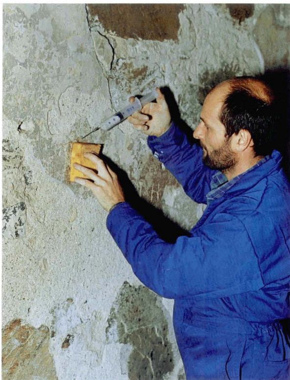
Illus 29. Historic Scotland conservator grouting loose plaster to give a better bond to its backing. © Crown copyright Historic Scotland
