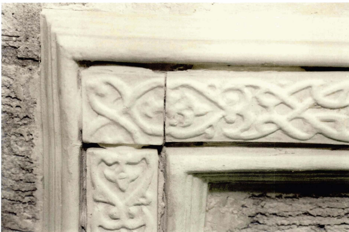
Illus 37. Cast rib enrichment positioned on soffit of in-situ run ribs, using fresh plaster as the adhesive. © Crown copyright Historic Scotland
