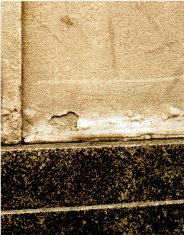
Illus 13. Blistering of this sandstone is caused by moisture trapped against the underlying, impermeable granite.
