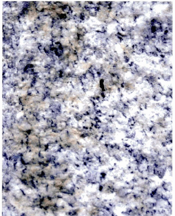
Illus 24. Staining. Iron-staining of this granite has been caused by alkaline cleaning chemicals left in contact with the surface for too long.
