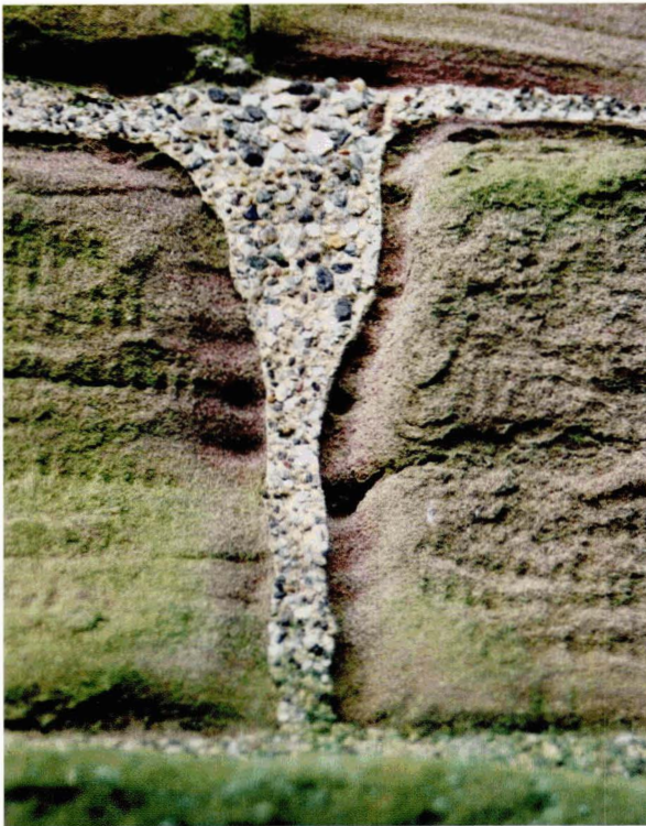
Illus 14. Decay of this sandstone around the joint is caused by the use of a mortar that is too hard and impermeable. Moisture movement is concentrated in the sandstone rather than the mortar.
