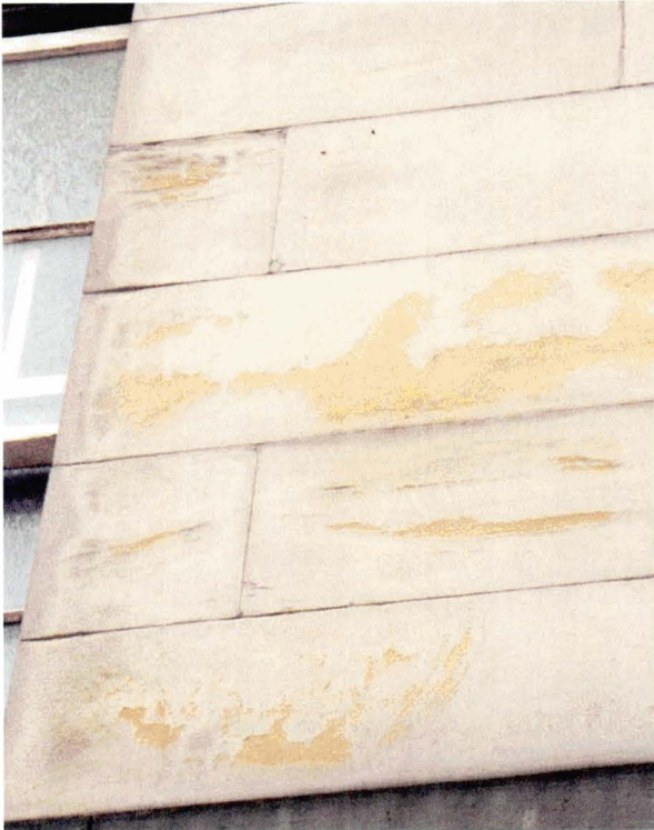
Illus 25. Bleaching. The surface of this sandstone has been bleached by chemical cleaning. Coloured iron-bearing minerals have been dissolved and re-deposited under the surface - now visible due to superficial granulation.
