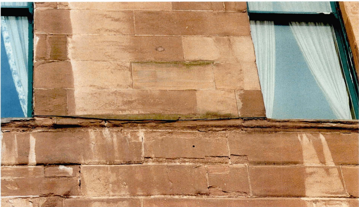
Illus 43. Rapid stone decay on this façade has been caused by a harmful interaction between cleaning and water repellent treatments applied to the stone.
