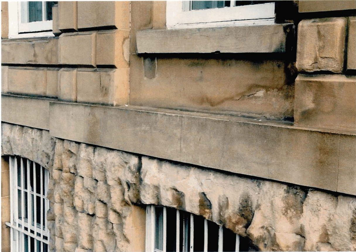
Illus 2. Loss of functional detail post stonecleaning. On this building a decayed string course has caused excessive erosion of the rock-faced sandstone below the string course. An unsatisfactory plastic repair to the string course has subsequently been carried out.
