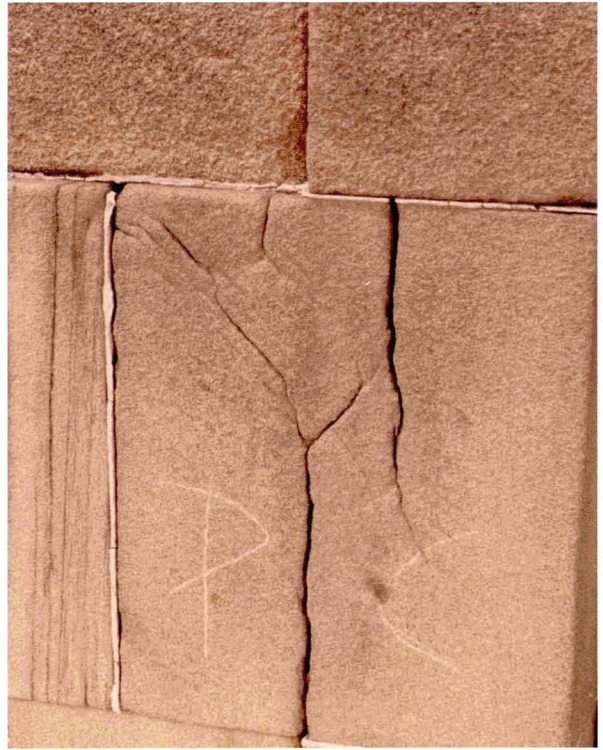
Illus 39. Fissures. Lines of fracture or open cracks. Fissuring of this sandstone occurred because the stone was edge bedded and subject to relatively high stresses adjacent to a window opening.
