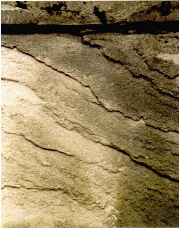
Illus 33. Delamination. Detachment of single or multiple planar sheets parallel to the natural layering or bedding of a stone. This sandstone has been face bedded and layers are now delaminating from the surface.
