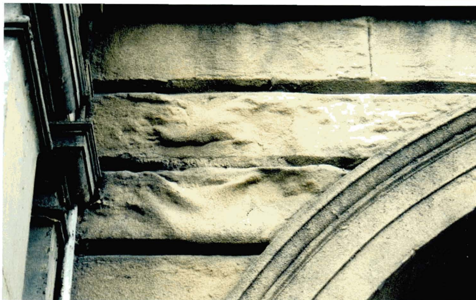
Illus 56. The bond between the thin PVA-based repair coating and the underlying sandstone has failed resulting in slumping and detachment of the repair.
