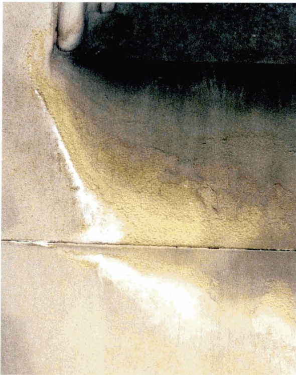
Illus 10. The 'drape' of salt efflorescence below this window is caused by run-off water concentrating salt residues from a large volume of stone within a small zone of evaporation.
