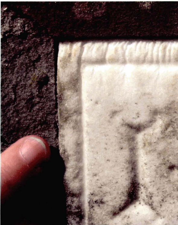
Illus 34. Dissolution. Partial or selective dissolution of mineral grains, especially carbonates. On this marble plaque, set into sandstone, dissolution by rain water running over the upper edge has cut small gullies into the marble.
