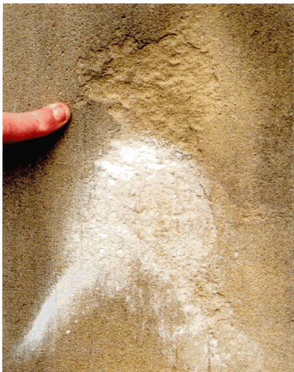
Illus 29. Granular disintegration. Generalised loss of stone surface caused by detachment of individual mineral grains. Granular disintegration of this sandstone surface is caused by sub-surface crystallisation (cryptoflorescence) of salts. Crystallisation on the surface (efflorescence) can be seen below the area of decay.
