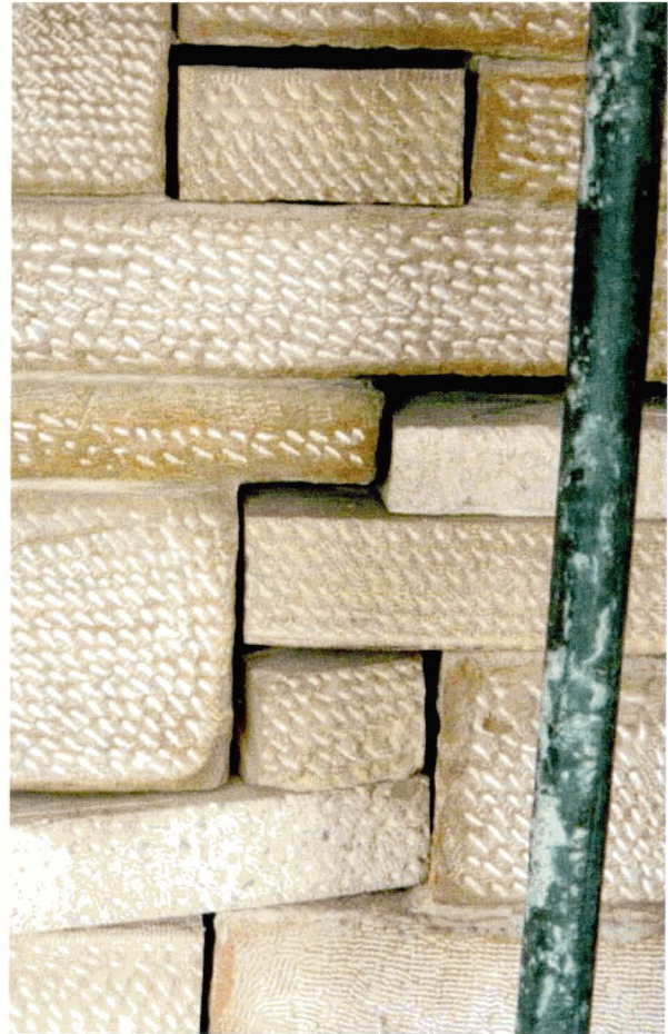
Illus 66. Repair involving partial replacement or indenting of a damaged stone (shown prior to bedding and pointing).
