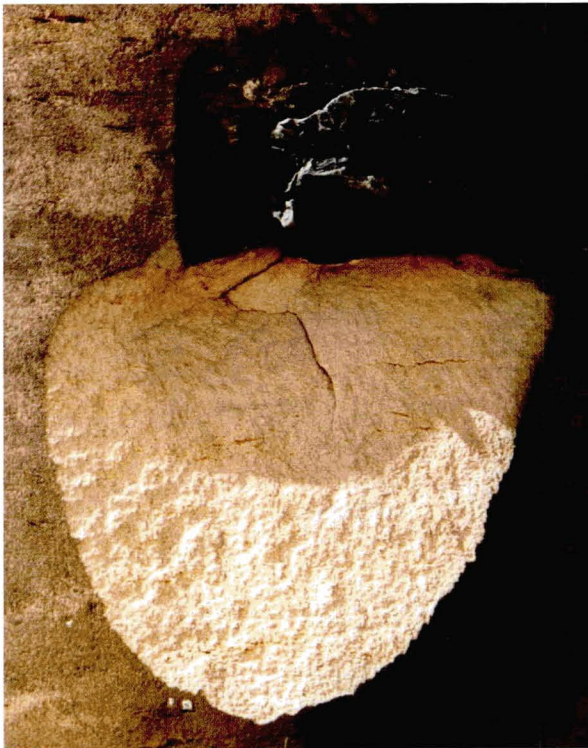
Illus 38. Mechanical damage. Loss of compact stone fragments by fracturing. In this case oxidation and expansion of an iron fixing has caused fracturing and loss of a piece of adjacent sandstone.
