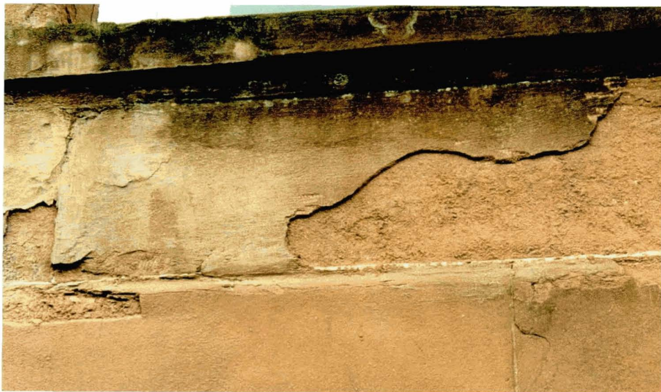
Illus 55. This poorly executed plastic repair on a sandstone facade has failed to bond with the underlying stone.
