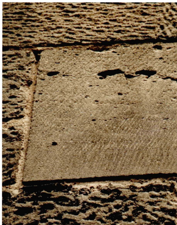
Illus 31. Decay of components. Clearly bounded zones of decay caused by the loss of elements or inclusions, e.g. clay nodules (as seen in this sandstone) or pebbles.
