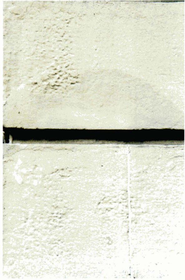
Illus 60. City-centre building, Glasgow. Close-up view of part of the façade in Illus 59 shows the crude nature of the repair after circa fourteen years exposure.
