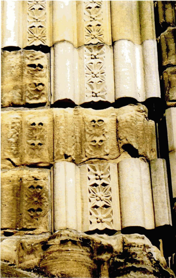
Illus 65. Repair involving replacement of damaged stone. The new stone conforms to the original profile and surface finish of the façade.
