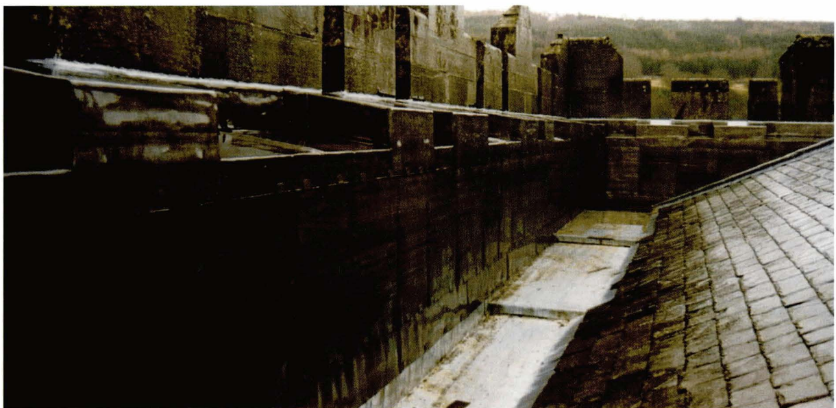
Illus 52. Protective covering. Lead sheeting has been used to prevent water penetration at roof level.
