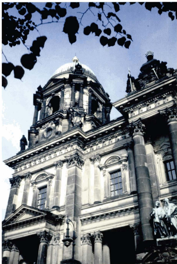
Illus 3. Typical soiling pattern on a sandstone building façade. Soiling is heaviest on areas exposed to rain and run-off.
