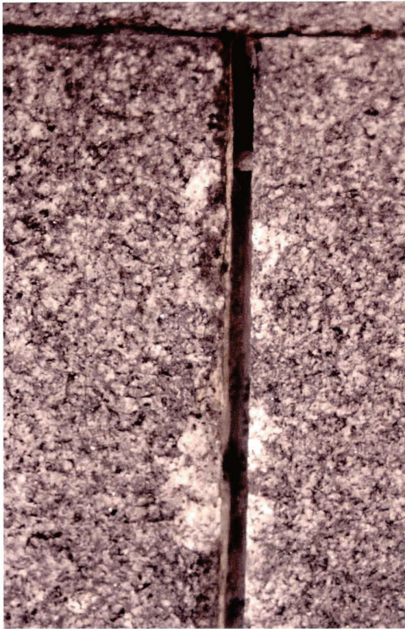
Illus 51. The edges of these granite ashlar blocks have been damaged during raking out of joints prior to repointing.
