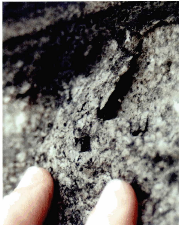
Illus 28. Blistering. Localised blistering of stone caused by expansion of a surface layer. This blistering on granite is caused by growth of gypsum crystals (black crust visible above the blister) which cause expansion and detachment of the surface layer.
