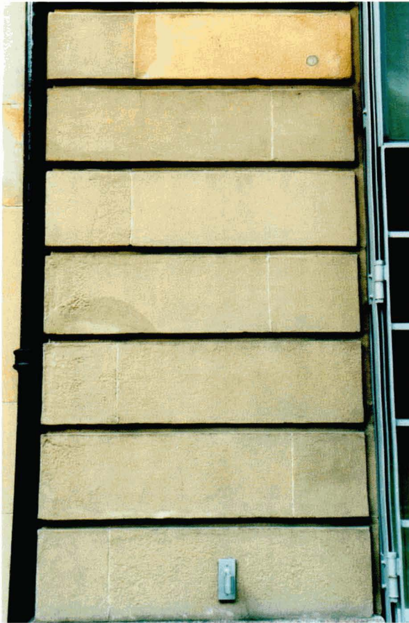
Illus 59. Part of the façade of a city-centre building, Glasgow, showing an extensive area of plastic repair.
