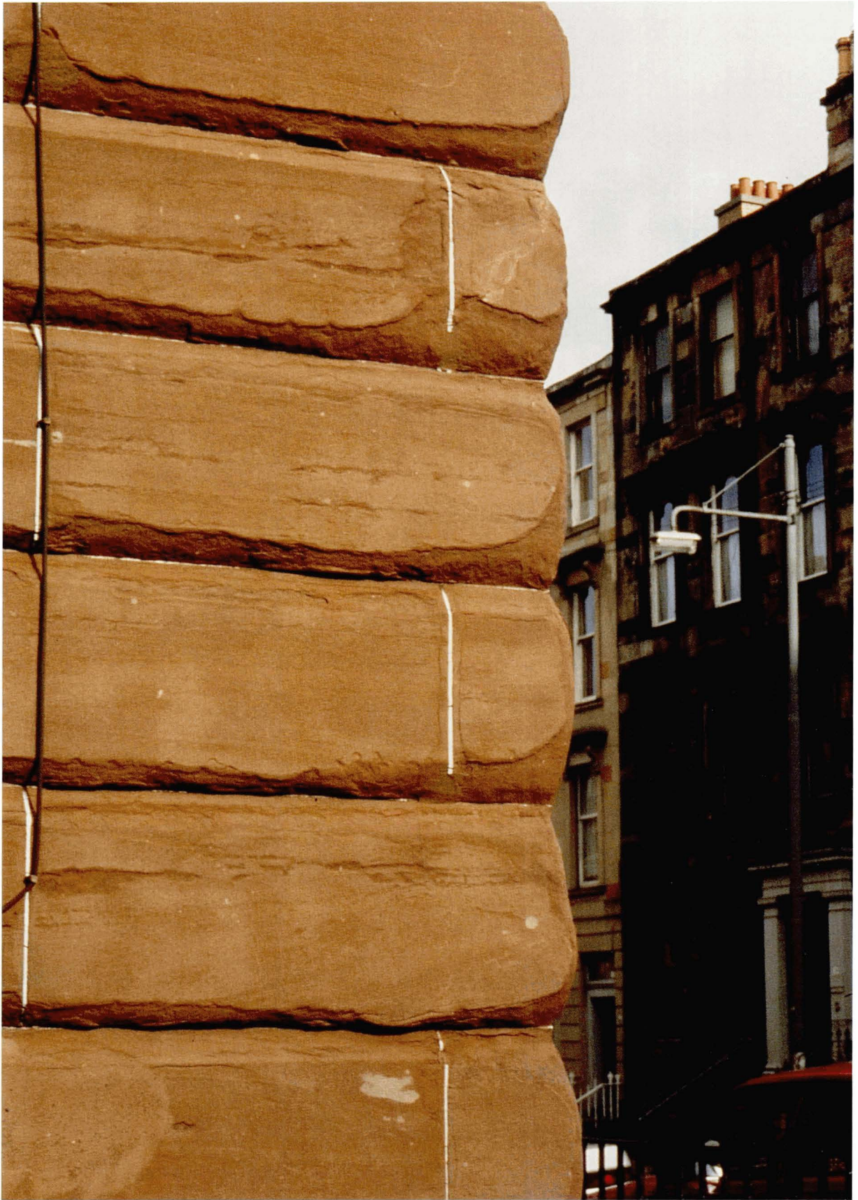
Illus 47. Enhanced widespread decay on this Glasgow tenement resulting from severely abrasive stonecleaning.
