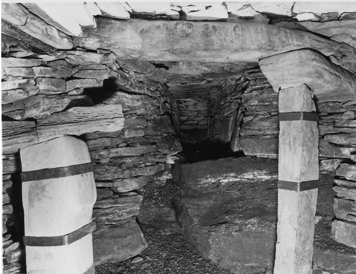
Figure 7: View from within chamber, looking towards passage. After the site was taken into State care, the stonework was consolidated and reinforced in places, to provide safe public access to the interior of the structure. Image 1971 © Crown copyright: HES.
