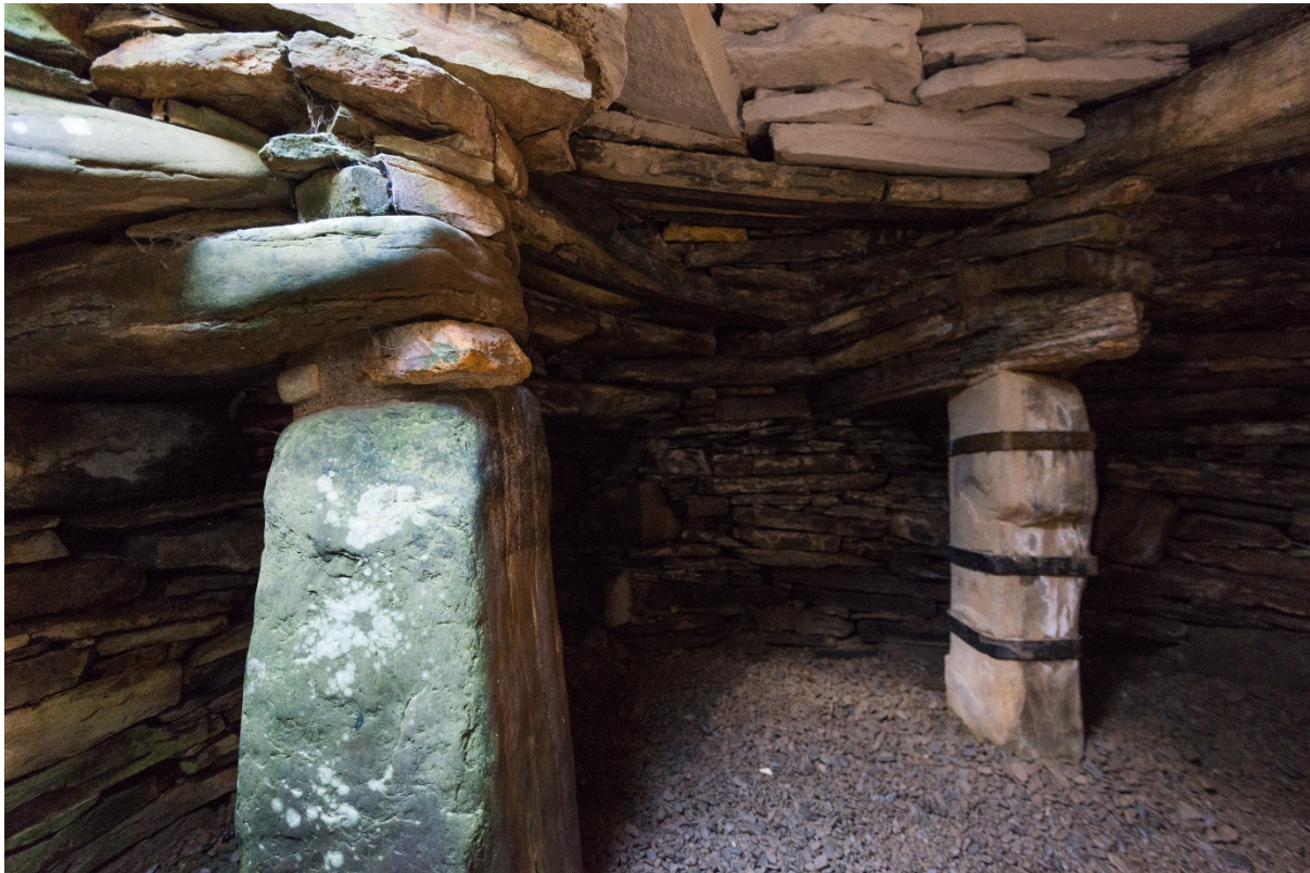
Figure 3: Looking south-west within the subterranean chamber of Rennibister Earth House. Its lintelled ceiling is supported by freestanding orthostats; a feature typical of Orcadian examples. At Rennibister these have been reinforced with modern, metal bars, and the roof has been partially rebuilt following damage by agricultural machinery in 1927. © Crown Copyright HES.
