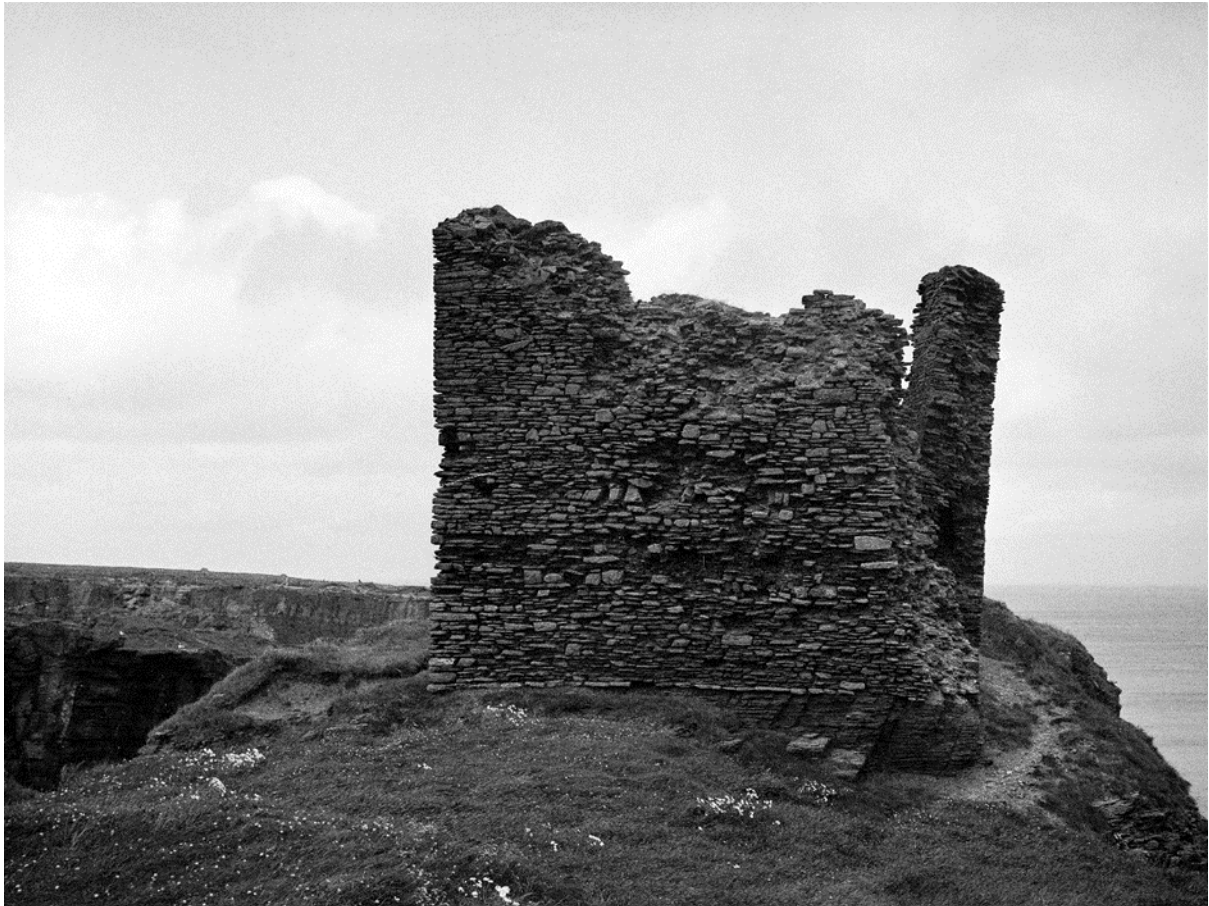
Figure 2: Photograph of masonry tower, 1952. Note the general decay of the tower's masonry (here the south-west external face), much consolidated since. The lower course, southern end of the tower reveals that it is constructed upon bedrock. Plainly the fronting ditch has also since been cleared. © Crown Copyright.
