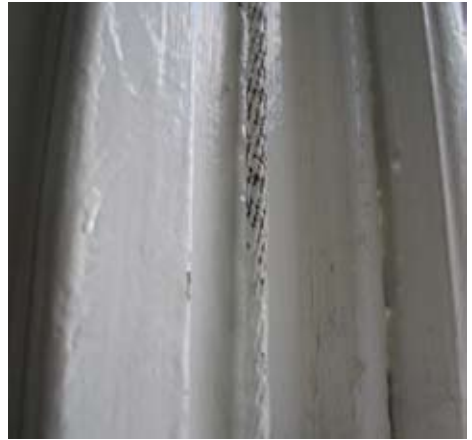
Paint-covered sash cords will make the window more difficult to open and close
