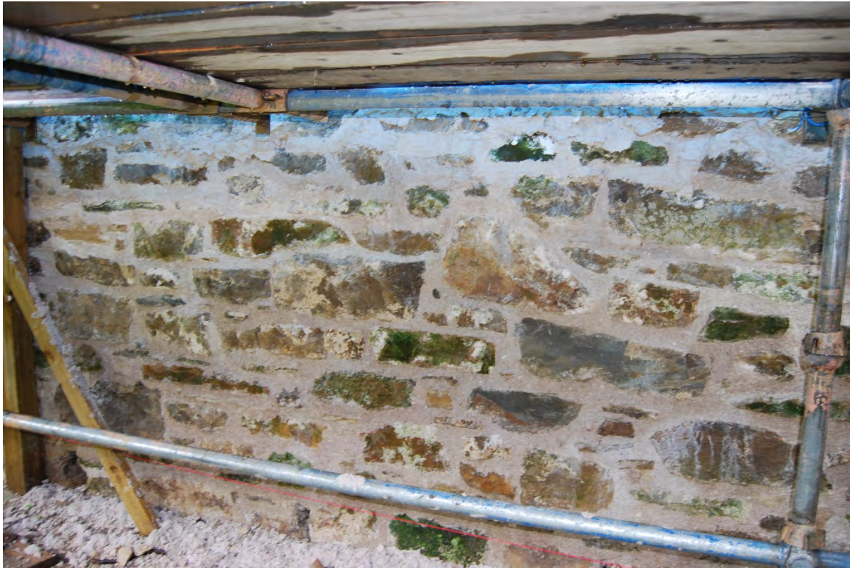
Figure 9. The reused stones in the new wall. Note the original mortar and lime wash still showing on the surface of the re-used stones.
