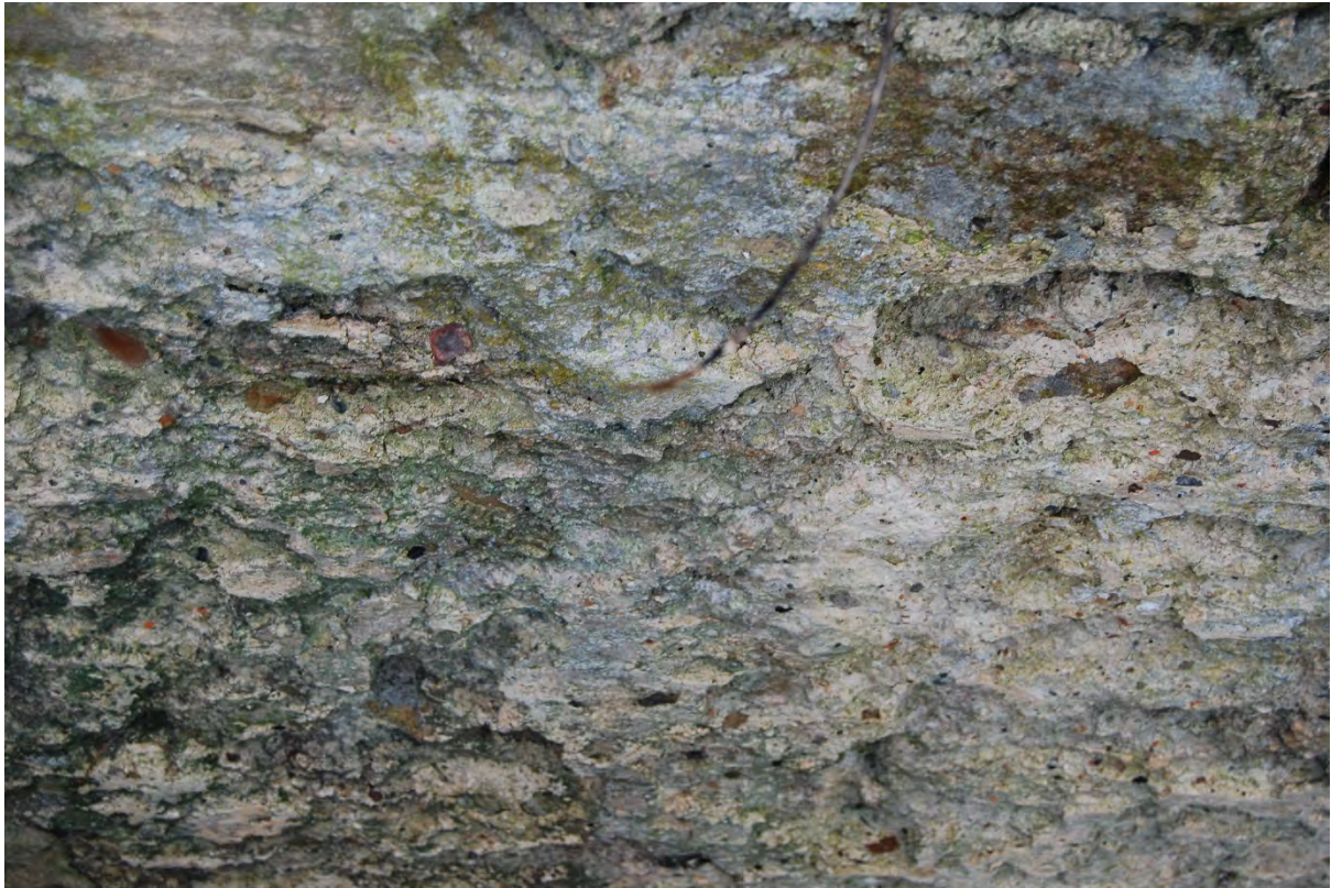
Figure 10. An area of historic masonry finish at the base of the orchard wall prior to the works.
