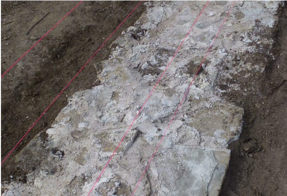
Figure 7. The foundation layer laid with a hydraulic lime mortar. The red lines are the setting out strings for the line of the new wall masonry.
