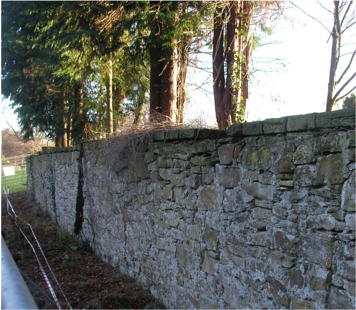
Figure 2. The orchard wall prior to the works. Note the trees very close to the upper side which contributed to its instability.
