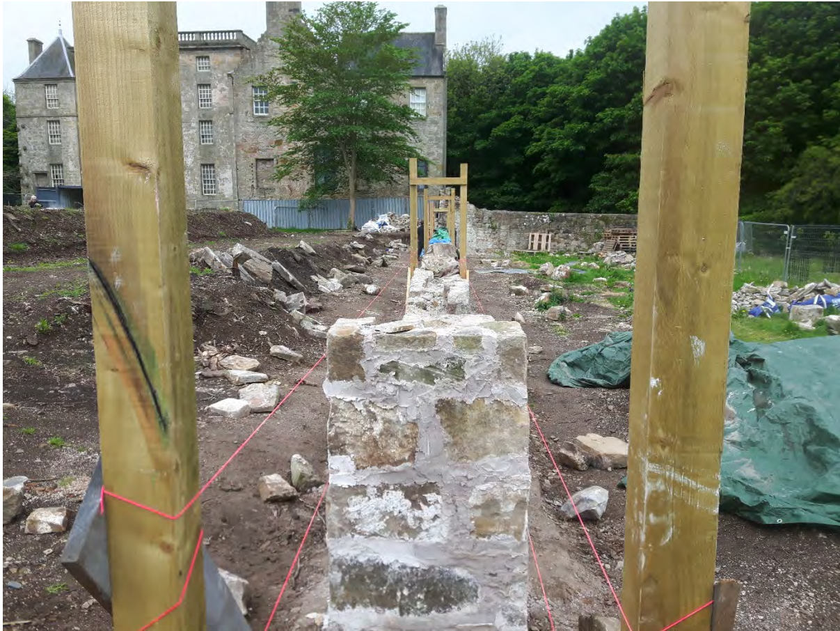
Figure 8. The string lines set up along the length of the new wall.
