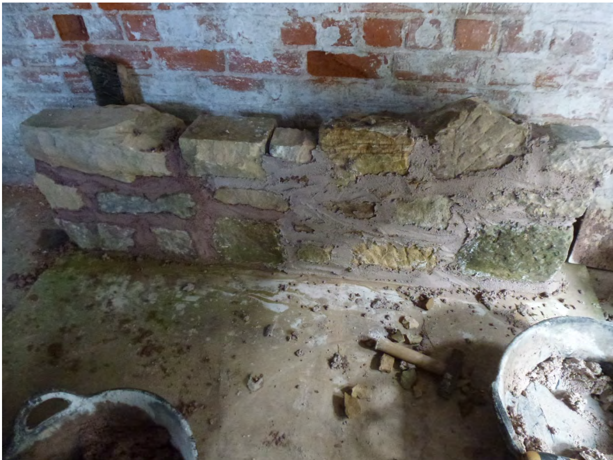
Figure 4. A small area of trial mortar in a new section of rubble wall in the HES yard at Blackness Castle.
