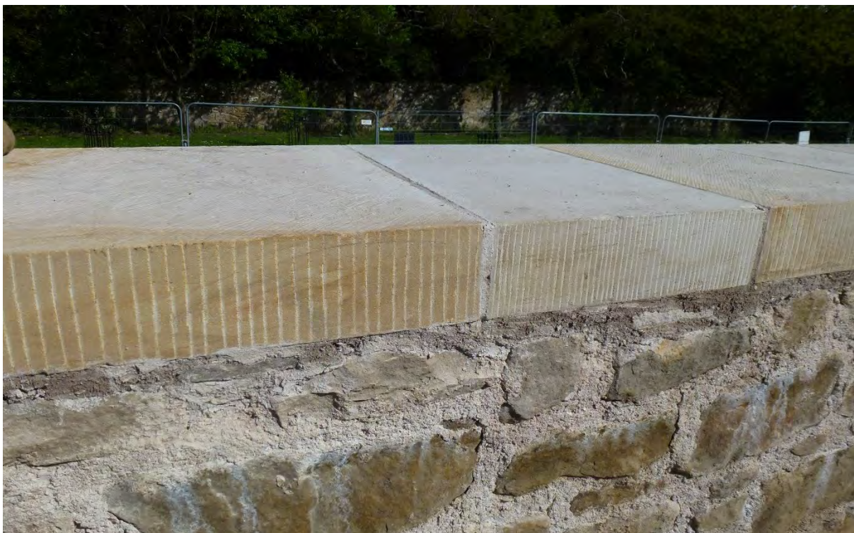
Figure 12. The new sandstone cope with frost damage on the mortar. Note the slight slope, or the 'wash' of the cope.
