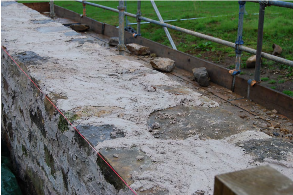
Figure 11. Detail of the completed wall awaiting the cope stones. The pointing on the left-hand side still needs to be scraped back.
