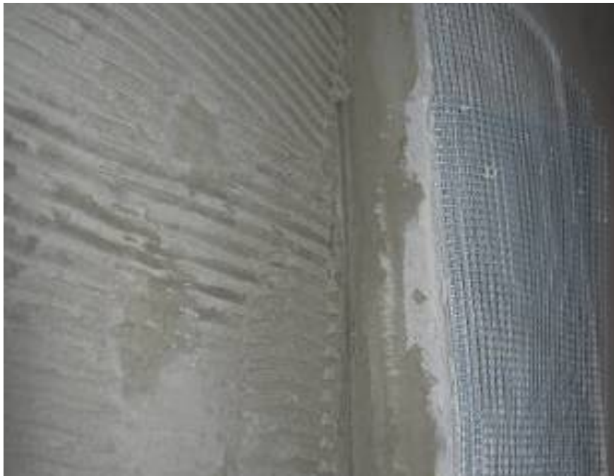
Fig. 3. Solid wall insulation using calcium silicate board, left open to show the layers
