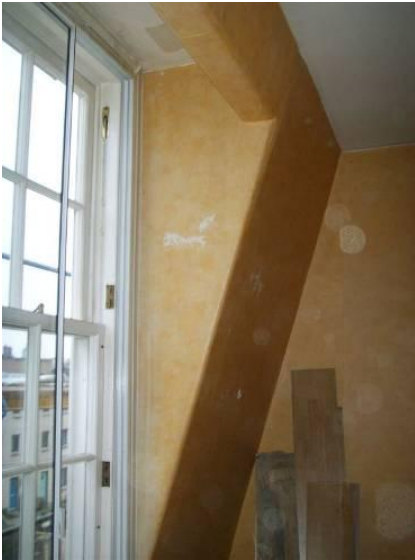
Fig. 7. Dormer cheeks in the living room, showing the existing aluminium-framed secondary glazing
