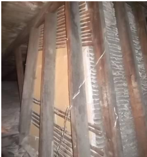
Fig. 2. Un-insulated lightwell within the attic space. Image by Adam Dudley Architects
