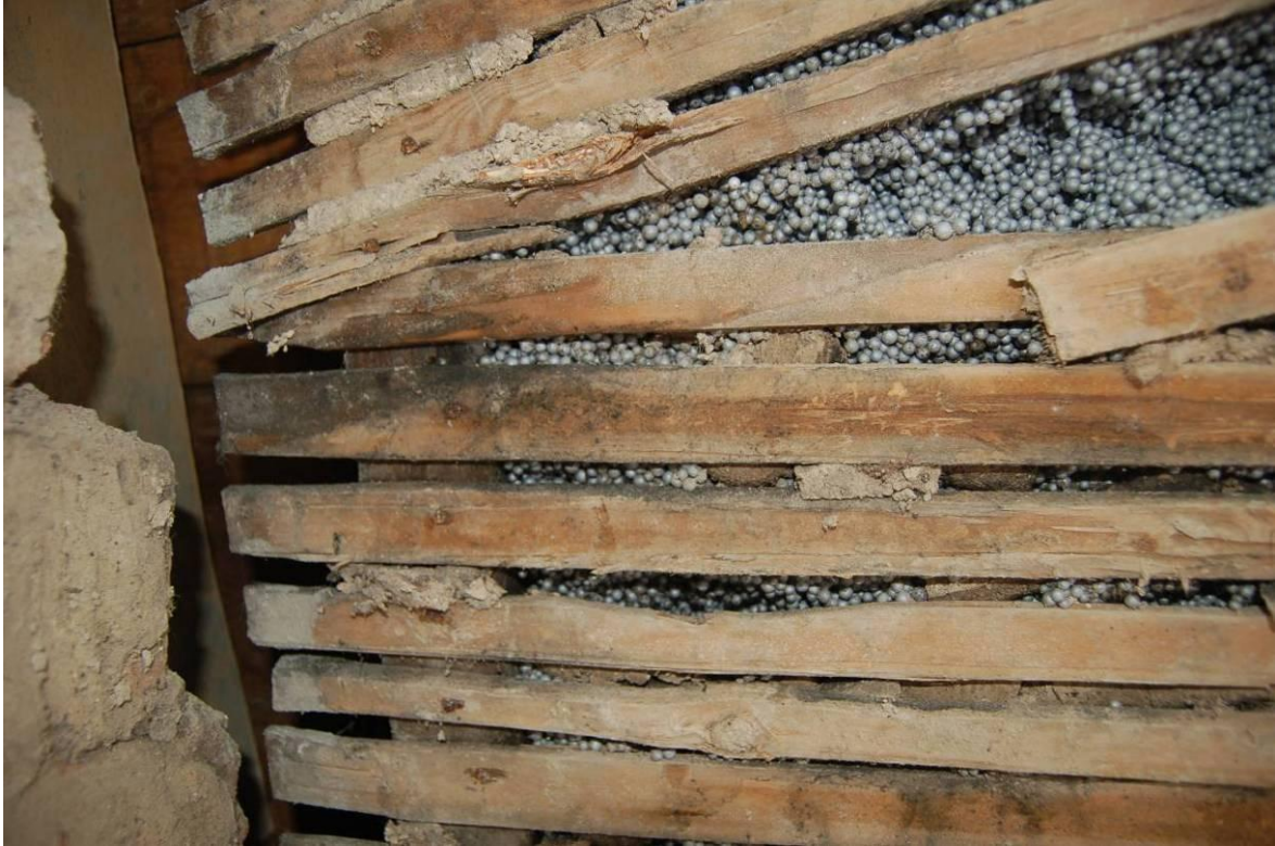
Figure. 23. Bonded bead following the water damage
