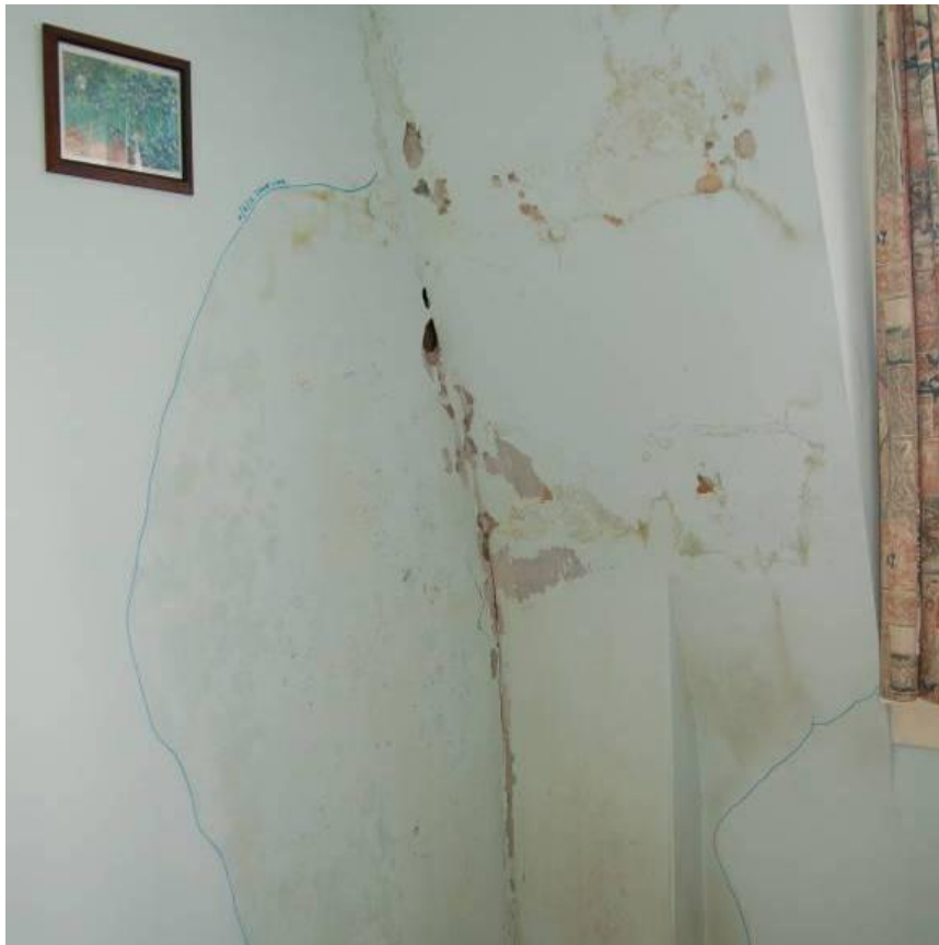
Fig. 22. Water damage to the coom ceiling from damaged pipe in the water tank
