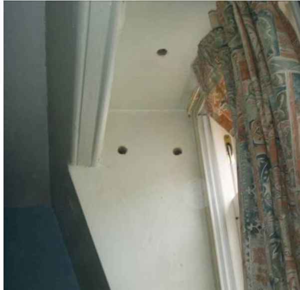
Fig. 20. Dormer cheek, drilled prior to injection of the bead. Image by Adam Dudley Architects
