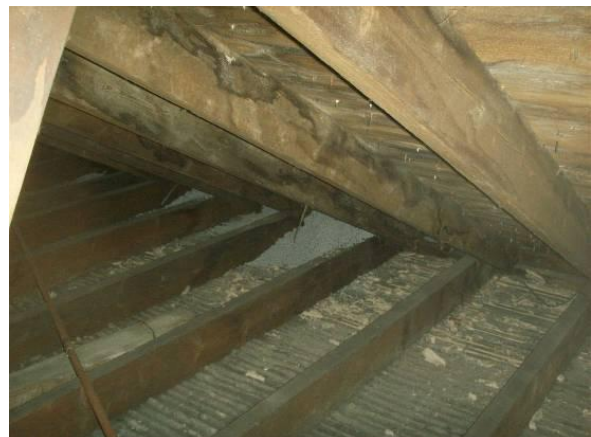
Fig. 13. Blown bead showing at the top of the filled cavity. Image by Adam Dudley Architects
