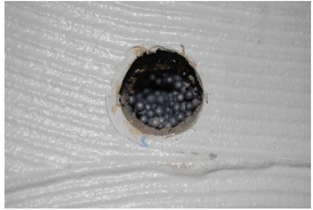
Fig. 17. The polystyrene bead insulation is pumped through holes approximately 30 mm in diameter
