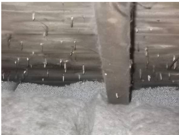
Fig. 14. The blown bead and the sheep's wool overlap to provide a fully insulated roof. Image by Adam Dudley Architects
