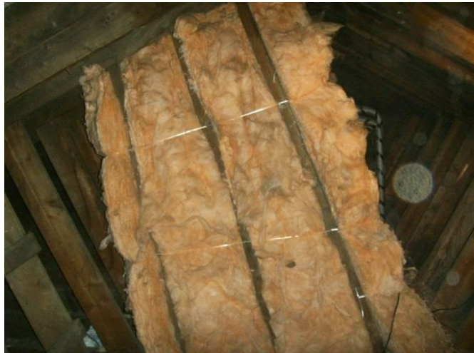
Fig. 3. Old glass fibre insulation to lightwell. Image by Adam Dudley Architects
