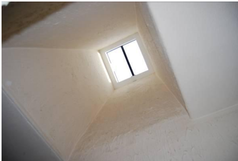
Fig. 10. New double glazed mechanized roof light
