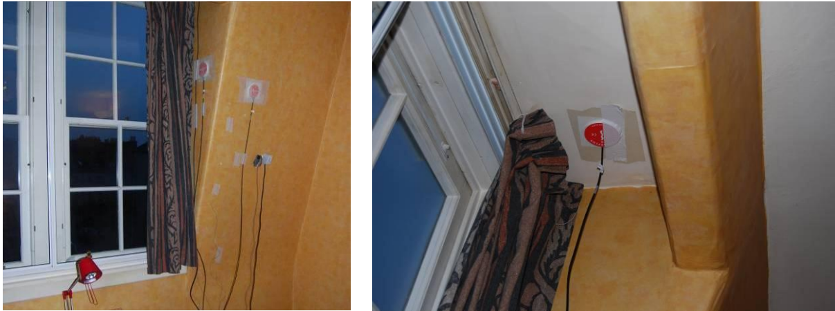
Fig. 9. U-value and humidity monitoring equipment whilst in place on coom ceiling, dormer and dormer roof
