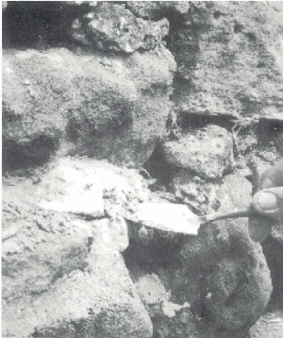
Figure 17 Repointing of a rubble wall. Note the use of pinning stones (to left of trowel).
