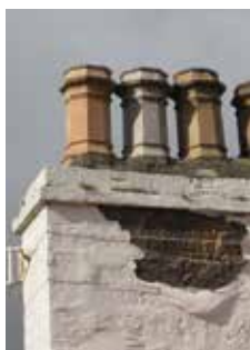
Top: Poor detailing of rainwater goods has led to overflow and saturation of masonry
