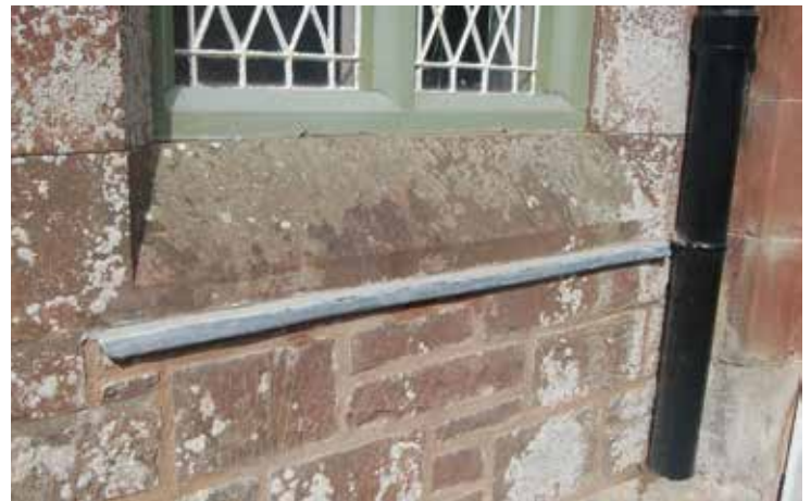
Below: This small addition below a window cill has kept the masonry below dry
