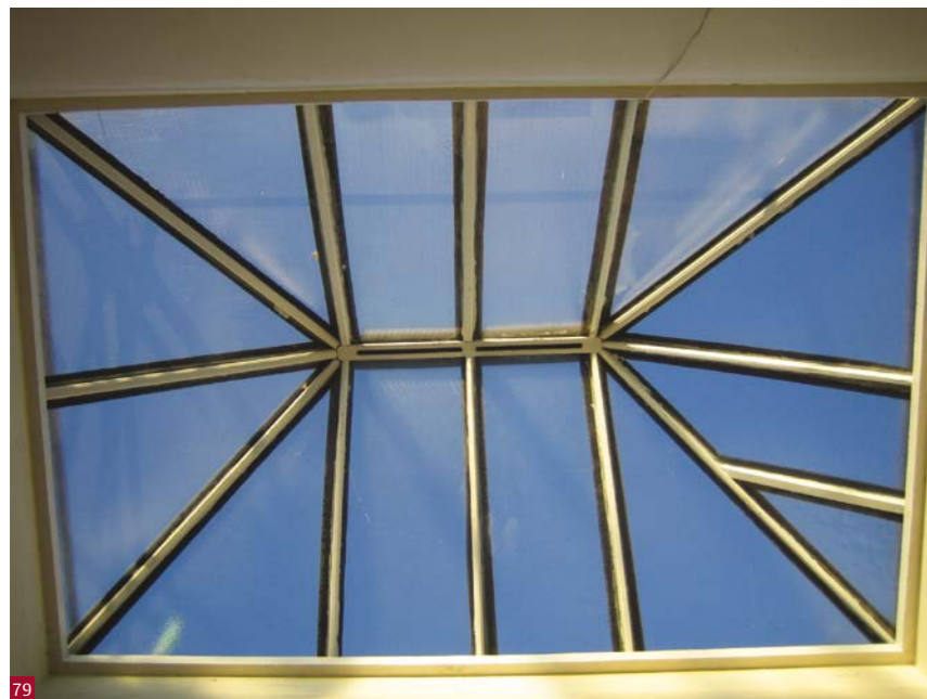
Fig. 79 A discreetly placed vent at the apex of a lightwell in an Edinburgh tenement stair.
