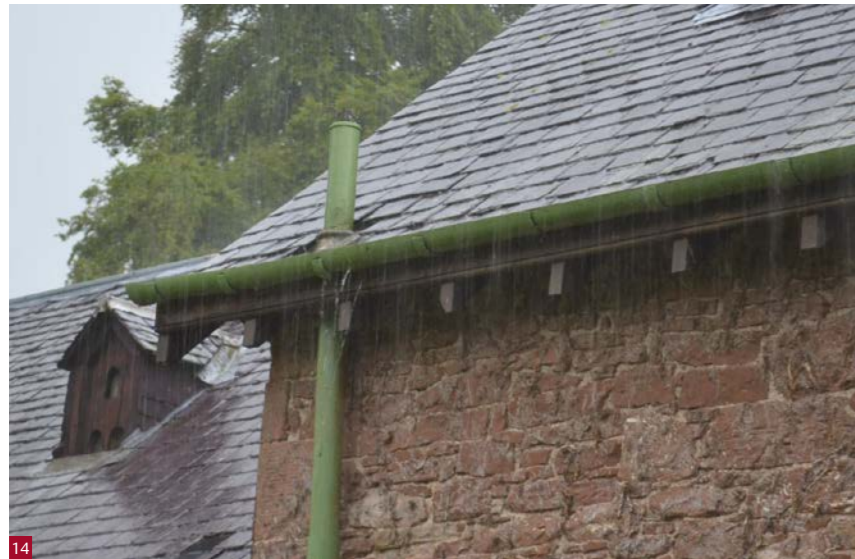
Fig. 14 Heavy and sustained rainfall may overwhelm existing drainage.
