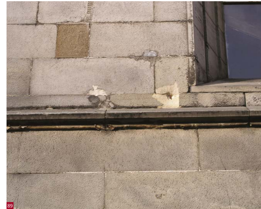
Fig. 89 Open joints in masonry have allowed water to penetrate, leading to corrosion of embedded iron cramps and fracturing of stone.
