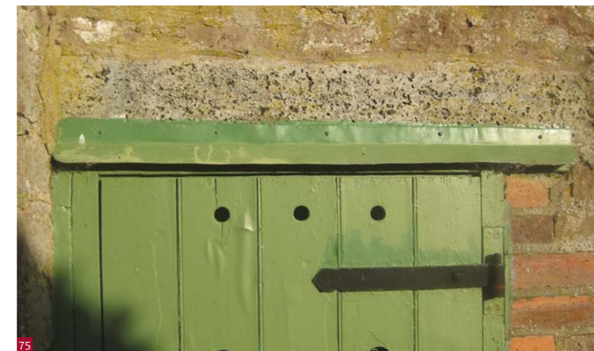
Fig. 75 The addition of a small hood over this flush mounted storeroom door has kept water off the top of the frame and the door.
