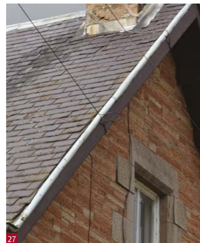
Fig. 26 Edge of slate cut to drive water away from the junction and minimise run off onto the gable.
