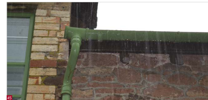
Fig. 45 Overflowing rhones in an area of high water flow.
