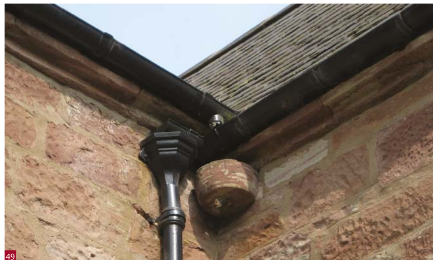
Fig. 49 Works to this building have neglected to reuse the original stone rainwater bracket, resulting in an overly complex arrangement.
