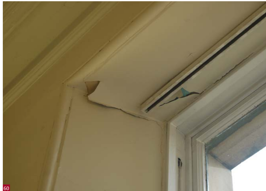
Fig. 60 Internal decorative damage, indicating defects on the external cornice.
