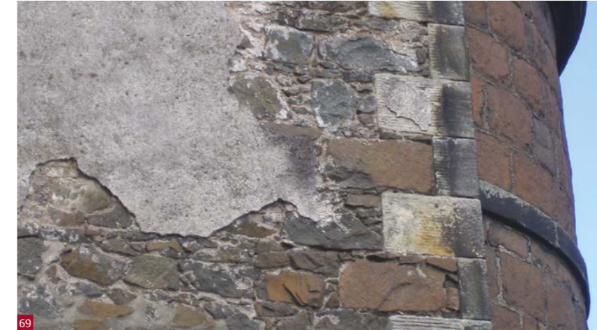
Fig. 69 Traces of original render on the gable end of a late 18th century building in Stirling.
