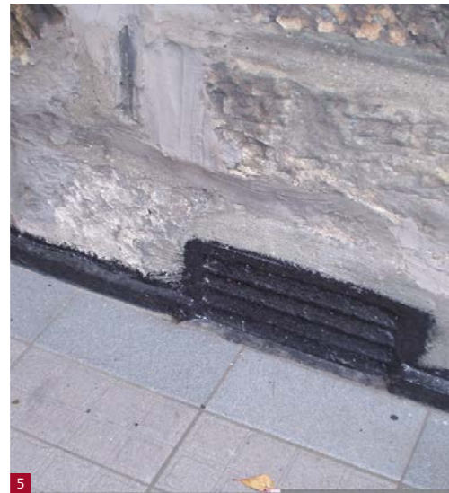
Fig. 4 Water ingress has led to progressive failure of the chimney and masonry below.
