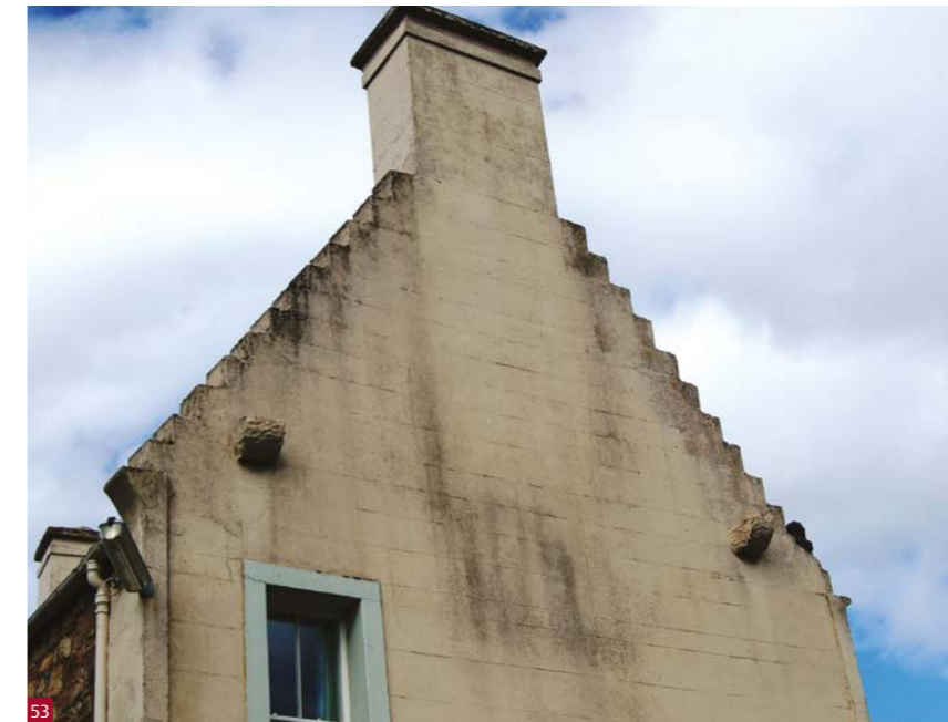
Fig. 53 A lack of protective water shedding detailing has led to staining, and progressive crazing of this cement-rendered gable.
