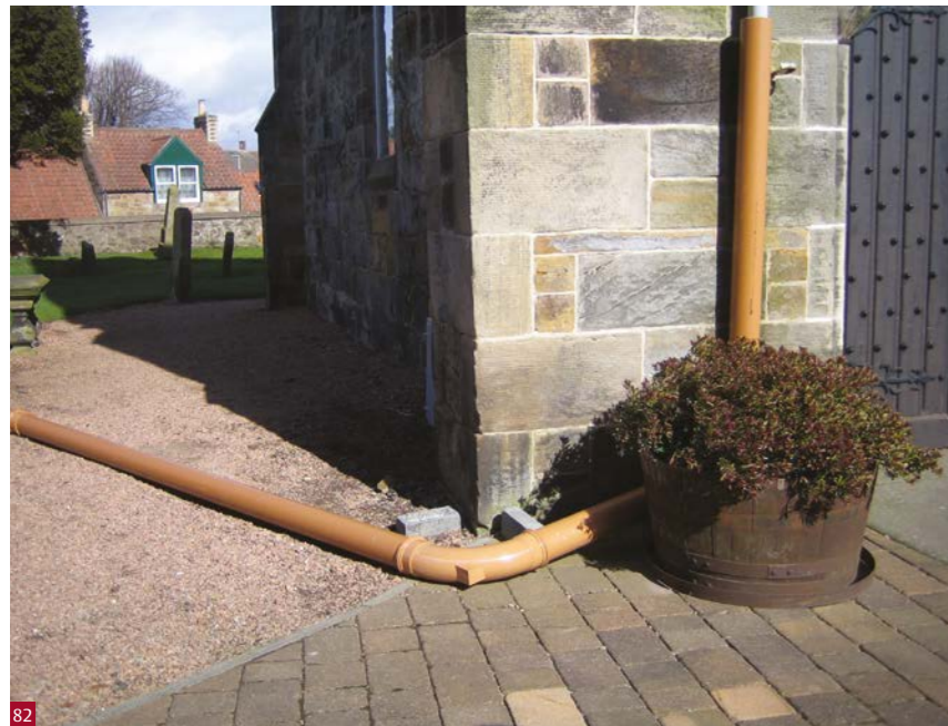
Fig. 82 A temporary but sensible solution to cope with blocked below ground drainage.
