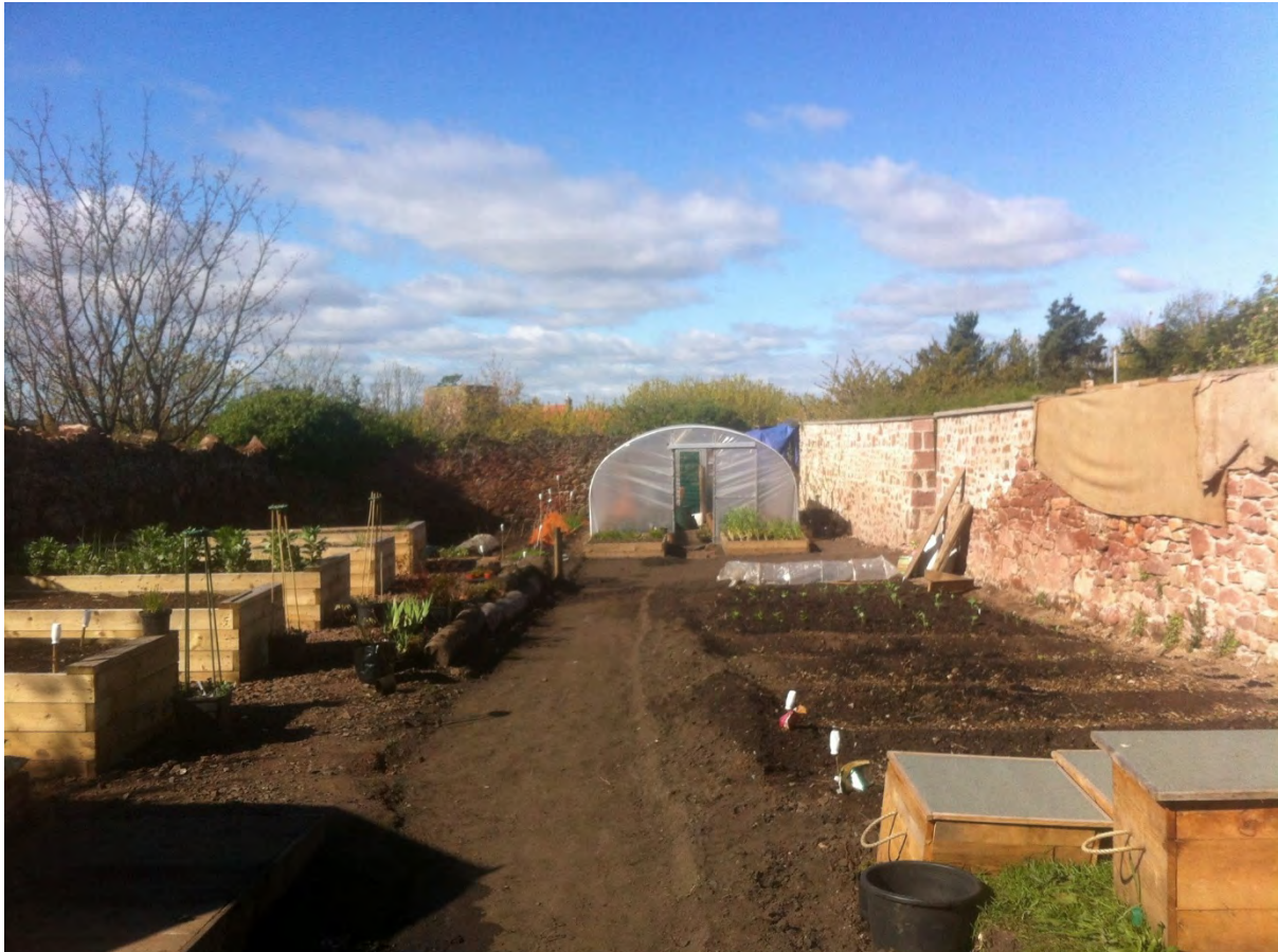
Figure 9. The finished walls from Phases 1 to 3 can be seen middle-right. The hessian protection is still covering the repaired upper masonry and new copes on the right.
