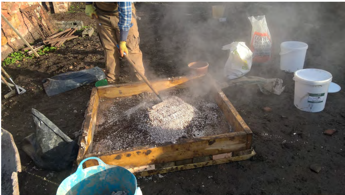
Figure 4. Hand-batching the sand and quicklime. This mortar bath was used to prepare the mortar for the test mortar and the rest of the project.
