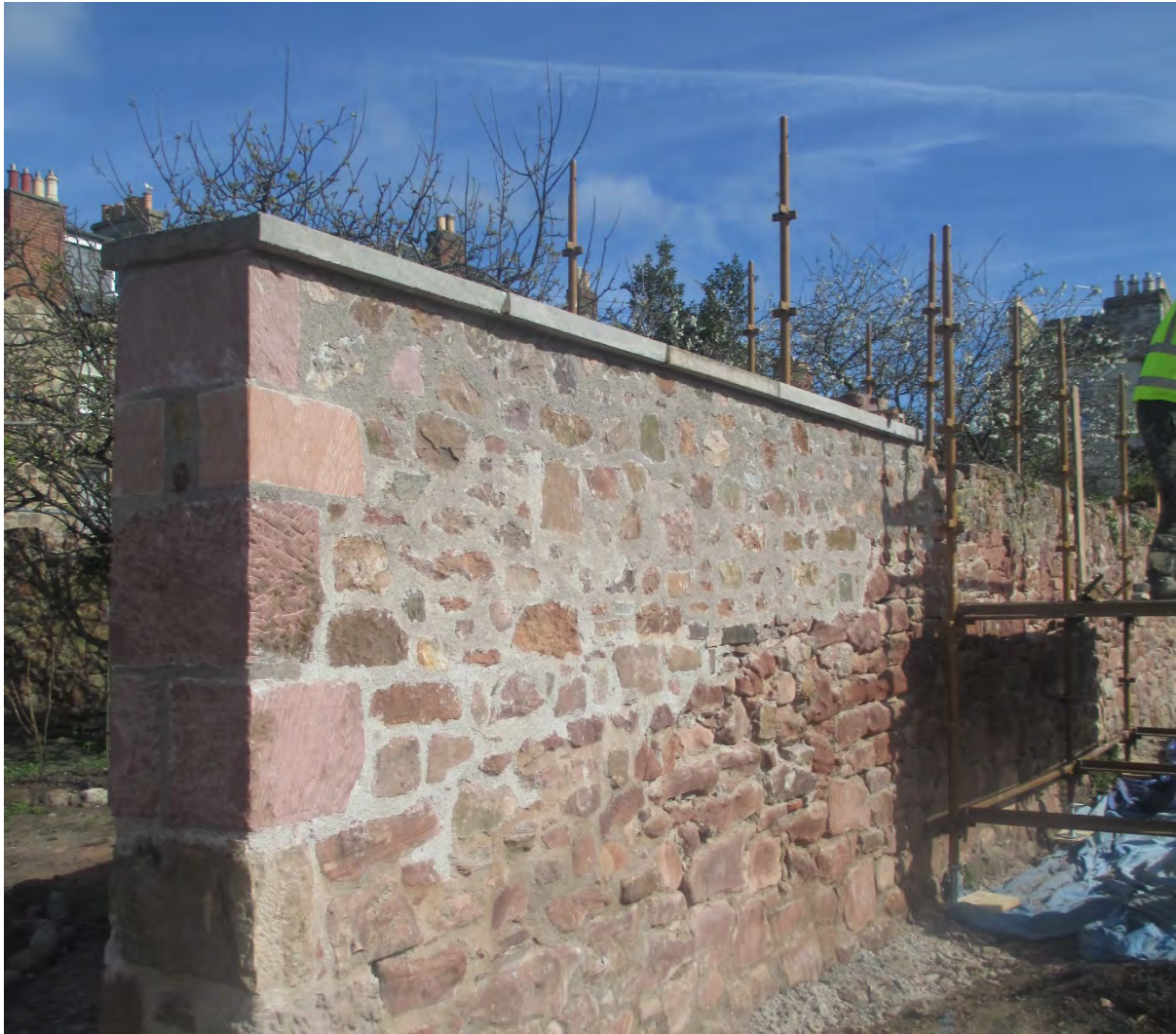
Figure 7. The rebuilt middle section of the boundary wall following scraping back towards the end of Phase 3 in April 2017.
