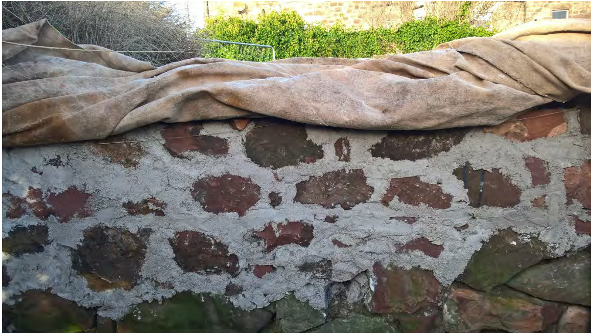
Figure 5. The wall head protection in place at the end of Phase 1 in December 2016. This mortar has yet to take a set and be scraped back.
