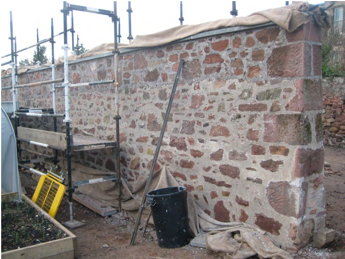
Figure 6. The rebuilt boundary wall at the end of Phase 2 in March 2017, with the flush pointing finish clear. The upper quarter of the wall has yet to take a set and be scraped back.
