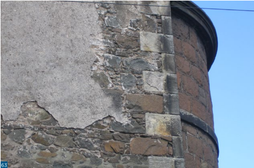
Figure 63: This gable end, which is in need of maintenance and showing the remains of a lime render, is well placed to receive an appropriate form of thin external insulation.
