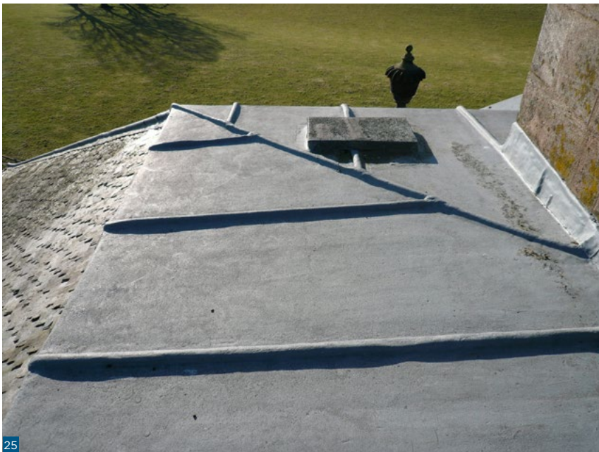
Figure 25: Where a flat roof is covered in lead or other metal, care is required not to cause conditions on the underside that lead to corrosion following retrofit.
