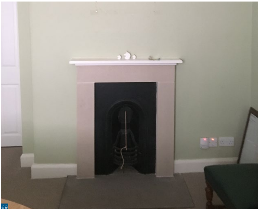
Figure 69: A baffle plate was installed in this fireplace to improve the control of ventilation.
