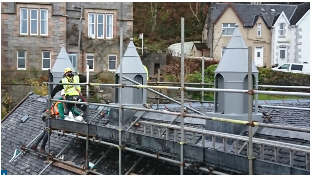
Figure 6: Reinstated ridge level vents at a former school in Oban. Image © Rockfield Centre
