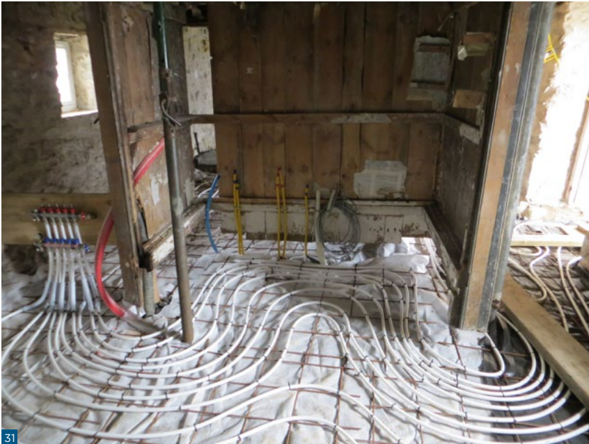
Figure 31: Coils for an underfloor heating system laid on top of a lime concrete floor. The heating is powered by a ground source heat pump. Image © Callum Innes
