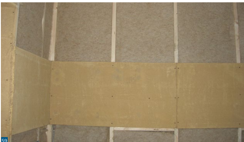
Figure 59: Hemp fibre insulation with clay board.
