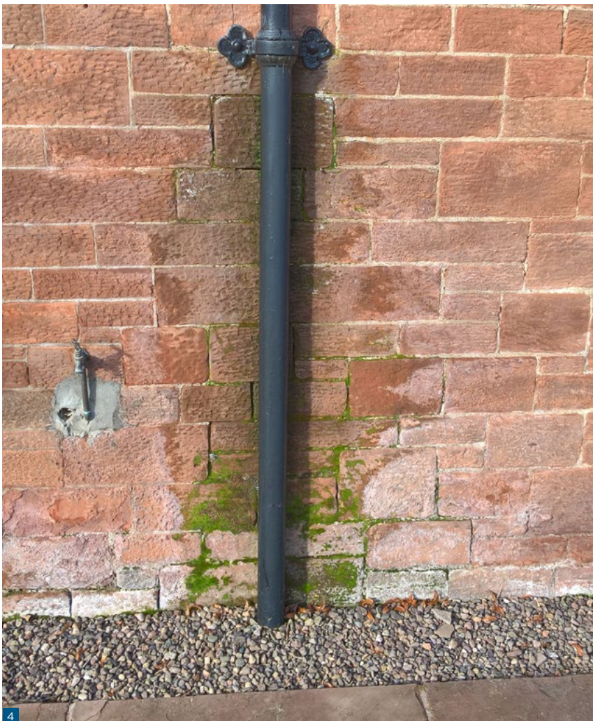
Figure 4: All buildings should be well maintained and any defects should be repaired before retrofit work is undertaken. This downpipe has been blocked for some time and the masonry behind appears to be saturated; the defect should be addressed first, before any insulation work.
