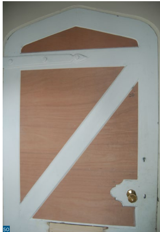
Figure 49: A door in a tenement with the insulation under the new plywood panels prior to painting.
