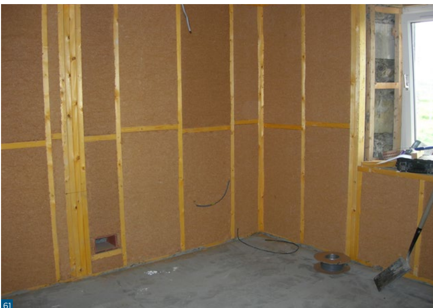
Figure 61: Wood fibreboard insulation applied within framing. A U-value of 0.19 was achieved in this example.
