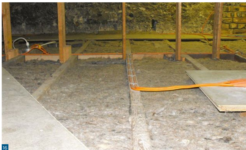
Figure 16: Sheep's wool insulation laid between rafters at Edinburgh Castle. Note the accommodation and fastening of wiring above the insulation.
