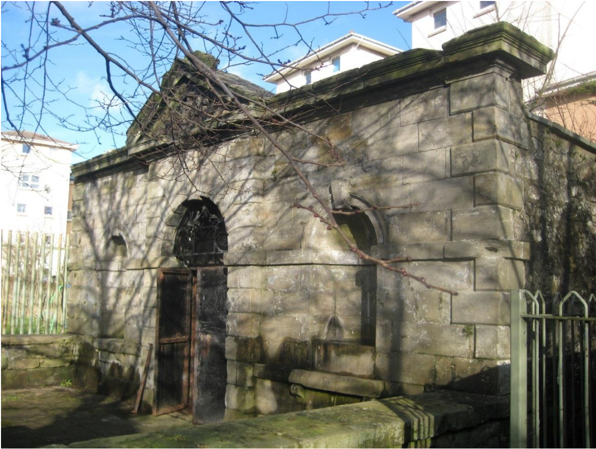
Fig. 1. The main elevation of the Wauchope mausoleum, view from the south west
