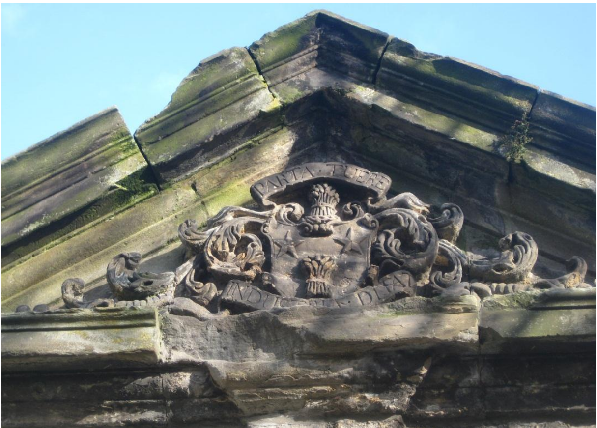
Fig. 5. Staining on the carved stonework from open ashlar joints and damaged cornice
