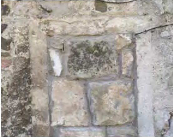
Figure 66.2. Lime applied as a harl running up to a window surround whose raised margin is modelled in mortar.
