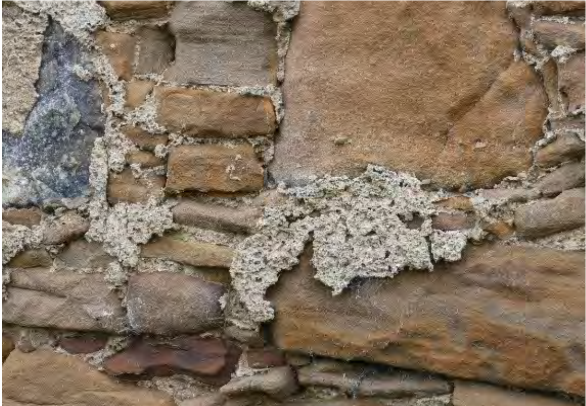
Figure 03.3. Section of masonry with heavily eroded harl.
