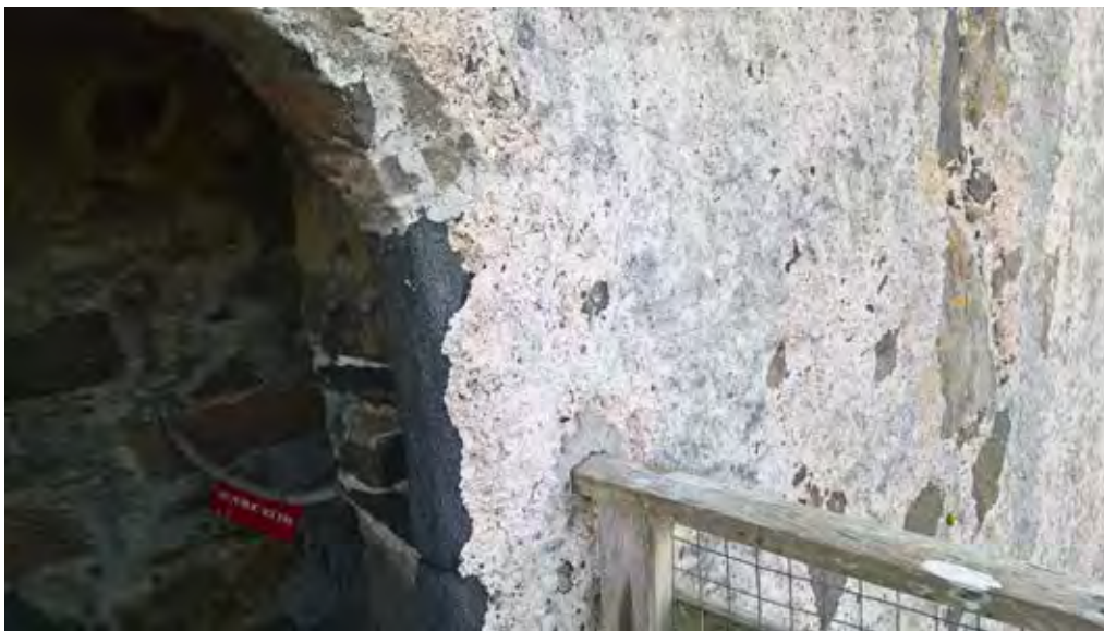
Figure 07.2. The historic harl extending over the dressed stones of the tower doorway. The good condition of the historic harl can also be seen on the rest of the wall.
