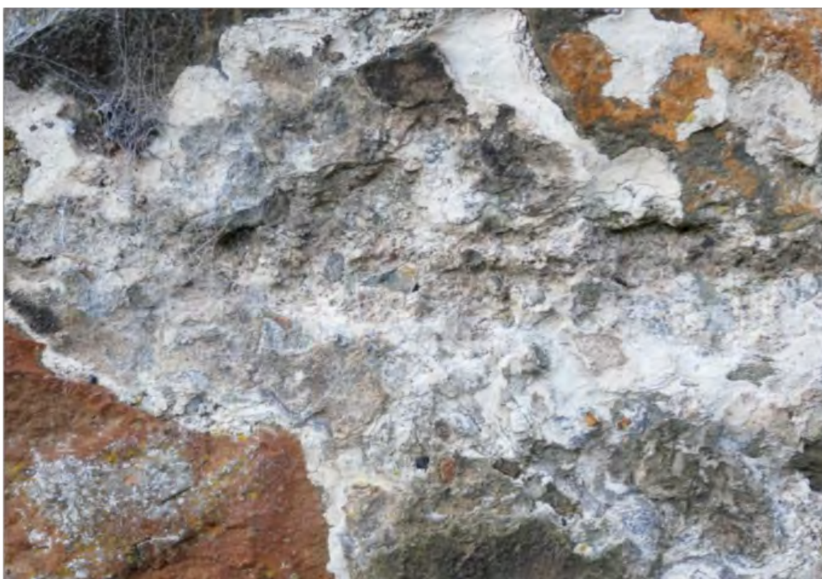
Figure 20. The Kirkcudbright Tollbooth, with harl clinging directly to the stone with many layers of limewash also visible.
