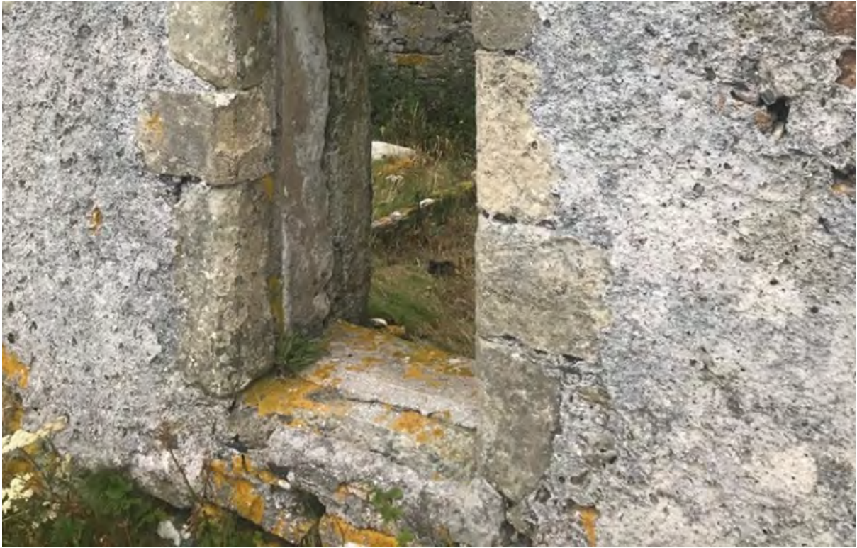
Figure 28.2. Old Vallay House - detail of surviving harl and its relationship to the window opening.
