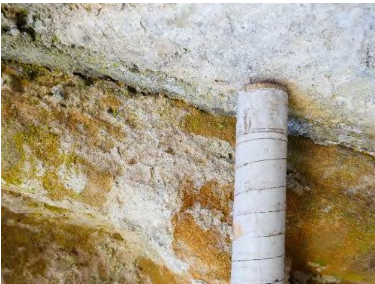
Figure 27.4. Detail of the remaining limewash or fine plaster on the arch.
