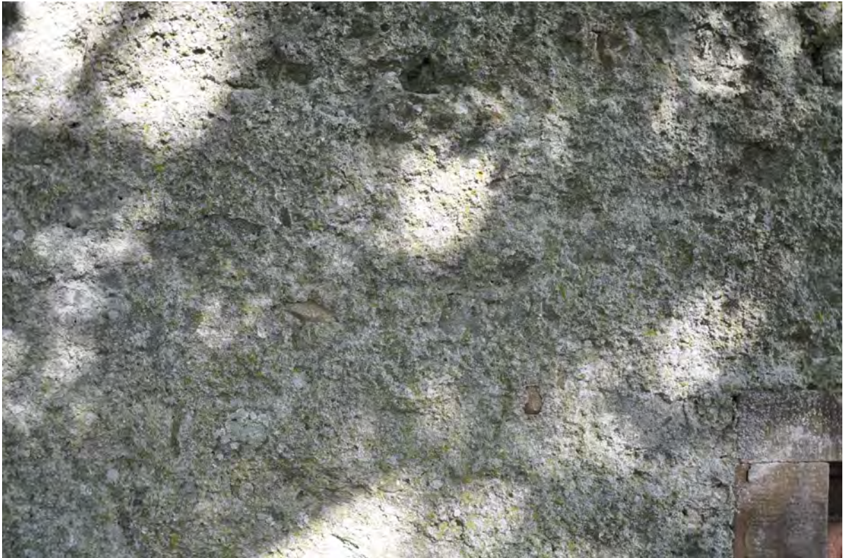
Figure 19.3. A detail of the harl on the west gable, showing a tight junction with the window margin.
