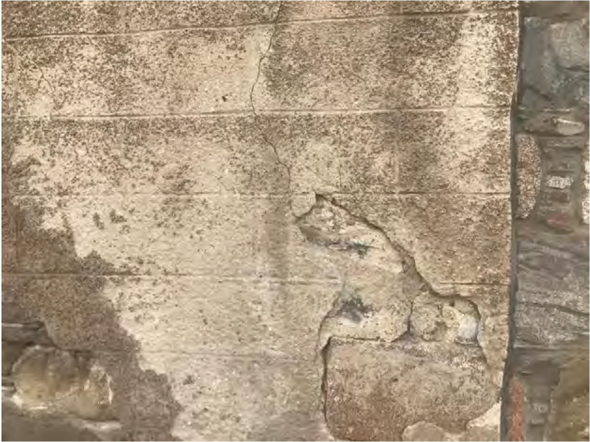
Figure 73.2. Detail of a well preserved area of the ruled-out dashed plaster. Note the junction with the next door property where the render has been removed.
