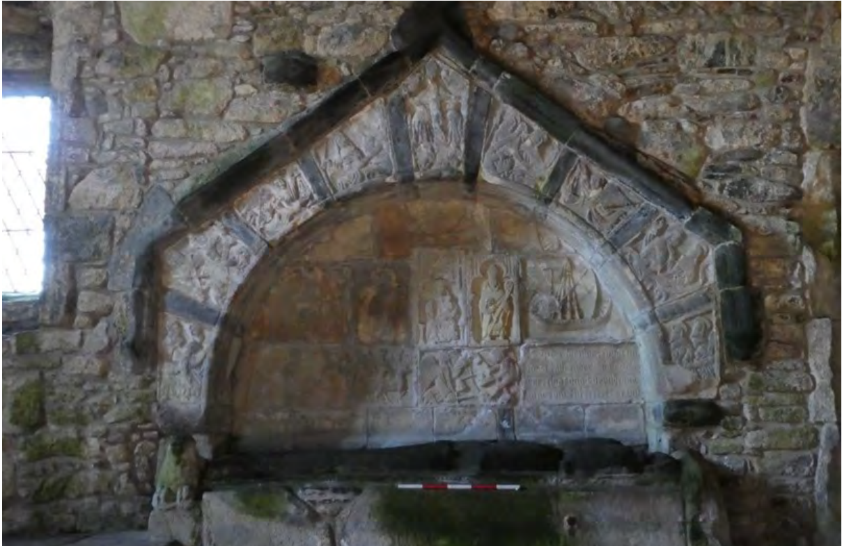
Figure 12.3. The building's interior which has problems with damp exacerbated by the incompatible cement pointing.
