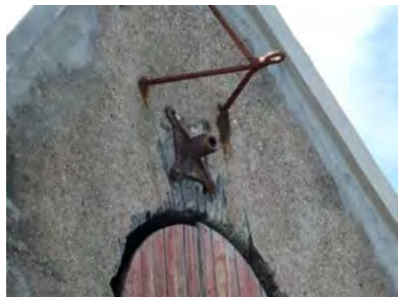
Figure 68.3. Area of harl decay.
