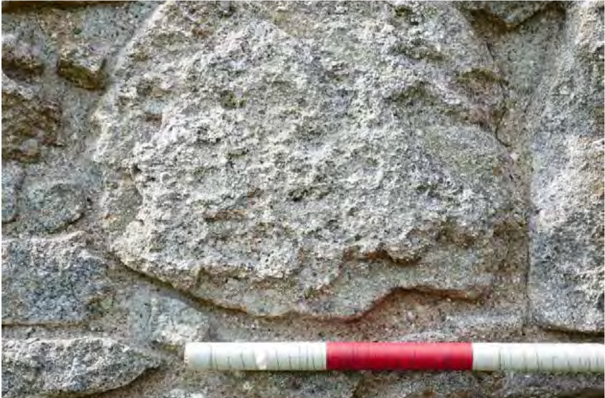
Figure 12.2. Detail of remaining harl, showing its coarse nature and tenacity.
