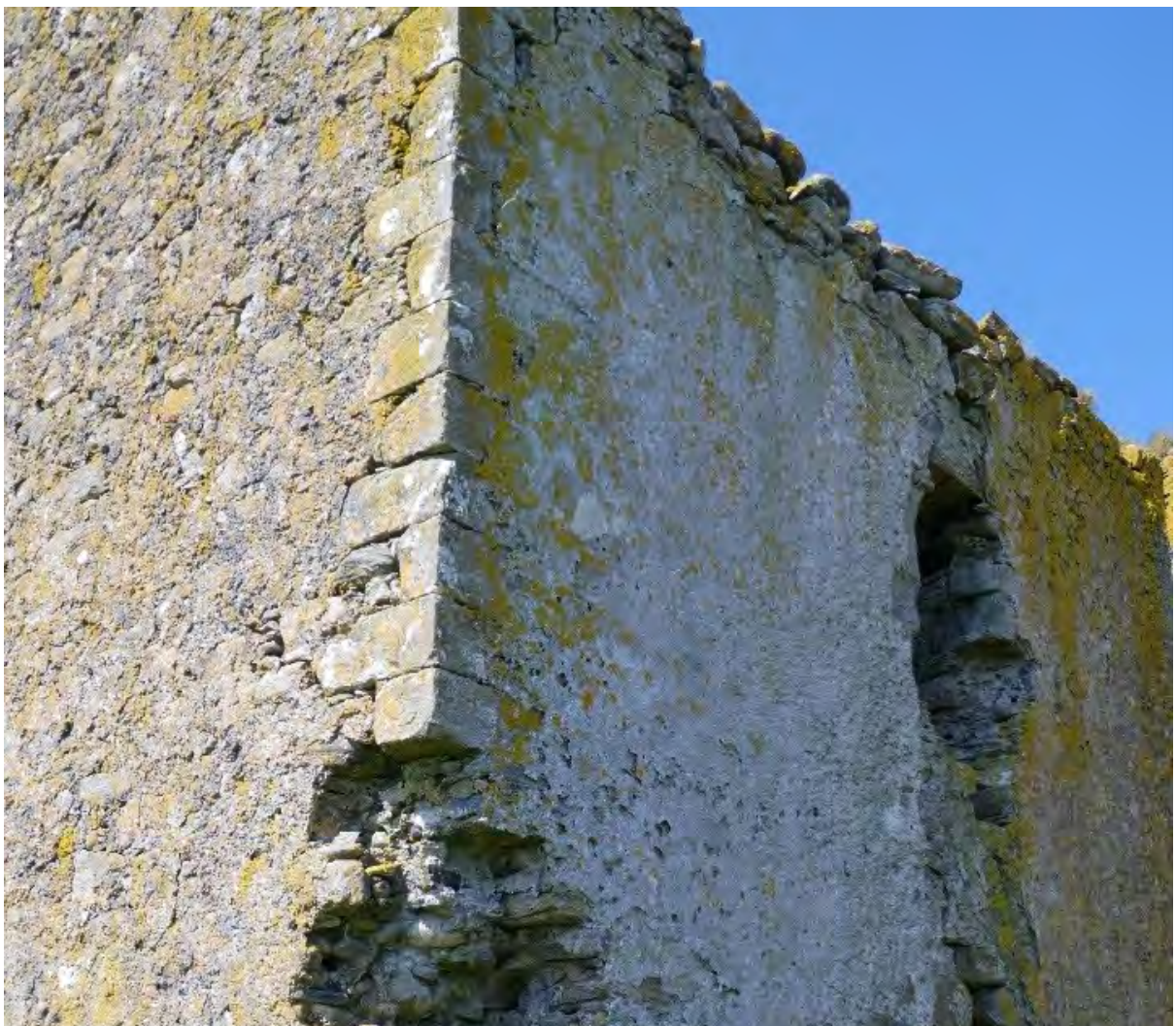
Figure 21.3. Detail of one section of quoining, where the harl is greatly degraded.
