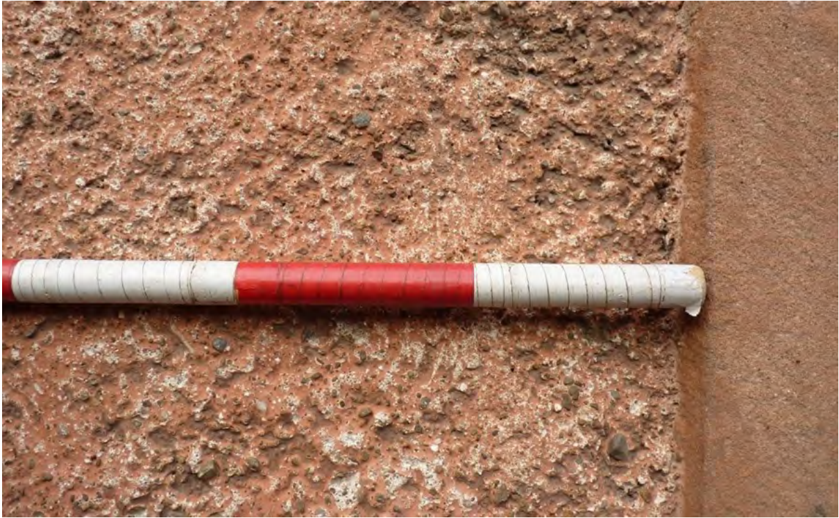
Figure 64.2. Limewashed harl on the principal elevation at the edge of the margin.
