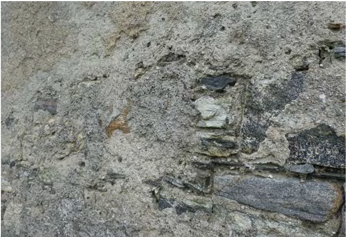
Figure 57.3. Detail of the original application with remains of overlying secondary applications.
