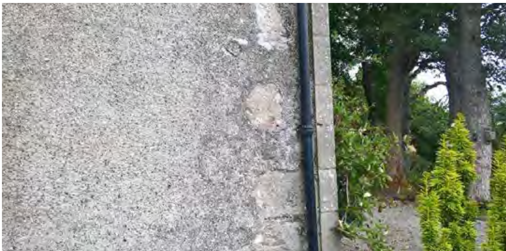
Figure 36.2. The harl covering the quoin on the north east corner, showing some flaking.
