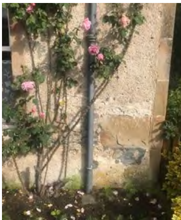
Figure 72.2. Detail of the lower part of the front elevation showing some spalling of the harl due to damp and frost.
