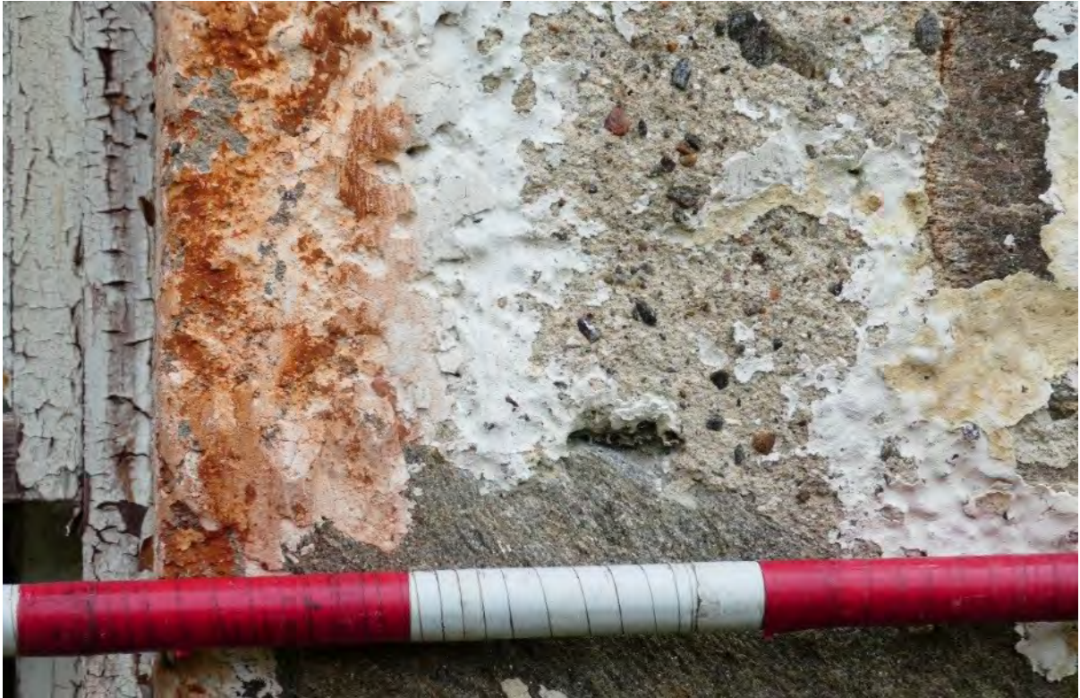
Figure 62.2. Evidence of the different coats of limewash which have been applied to the building.
