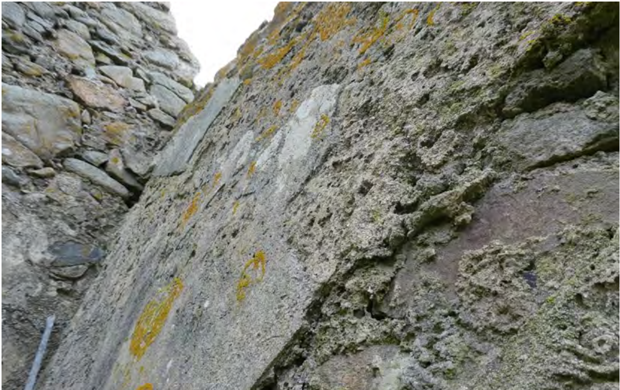
Figure 39.3. Remains of integral interior plastered finish.
