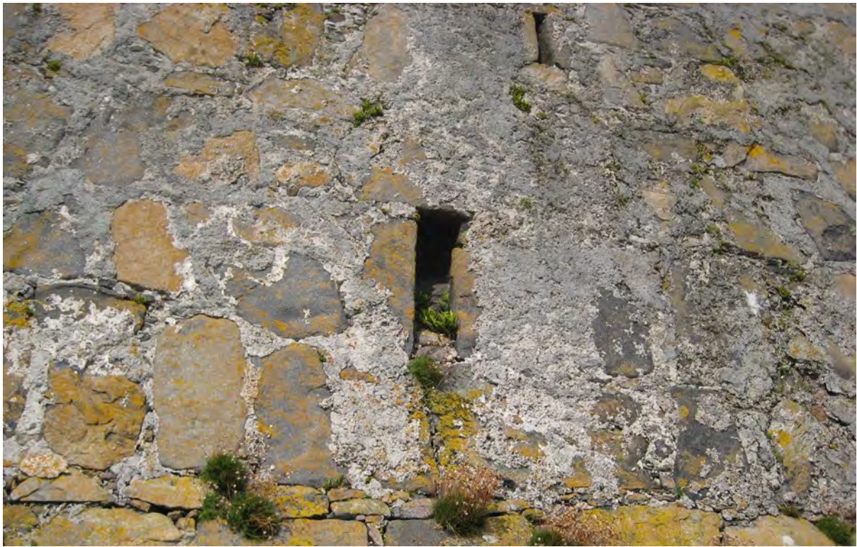
Figure 07.4. Even on the more exposed south elevation of the castle, the historic harl is still visible adhering well to the hard rubble and dressings.
