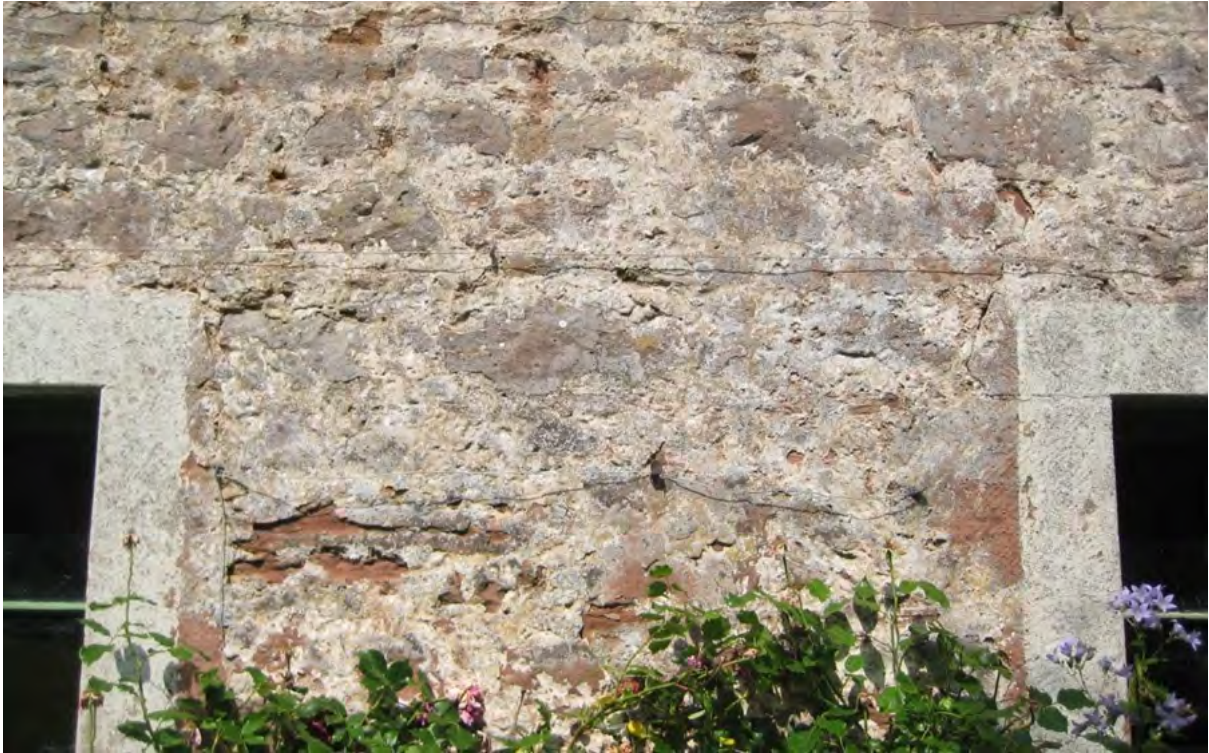
Figure 35.2. Detail of the south wall of the north range. The coursed rubble has been flushed out and lime washed; while most lime wash has weathered away, traces are easily identifiable.
