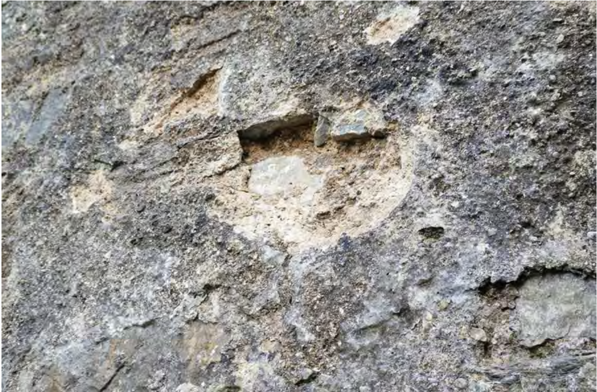
Figure 55.2. The single coat of lime harling, with the earth mortar showing through where the harl has detached.
