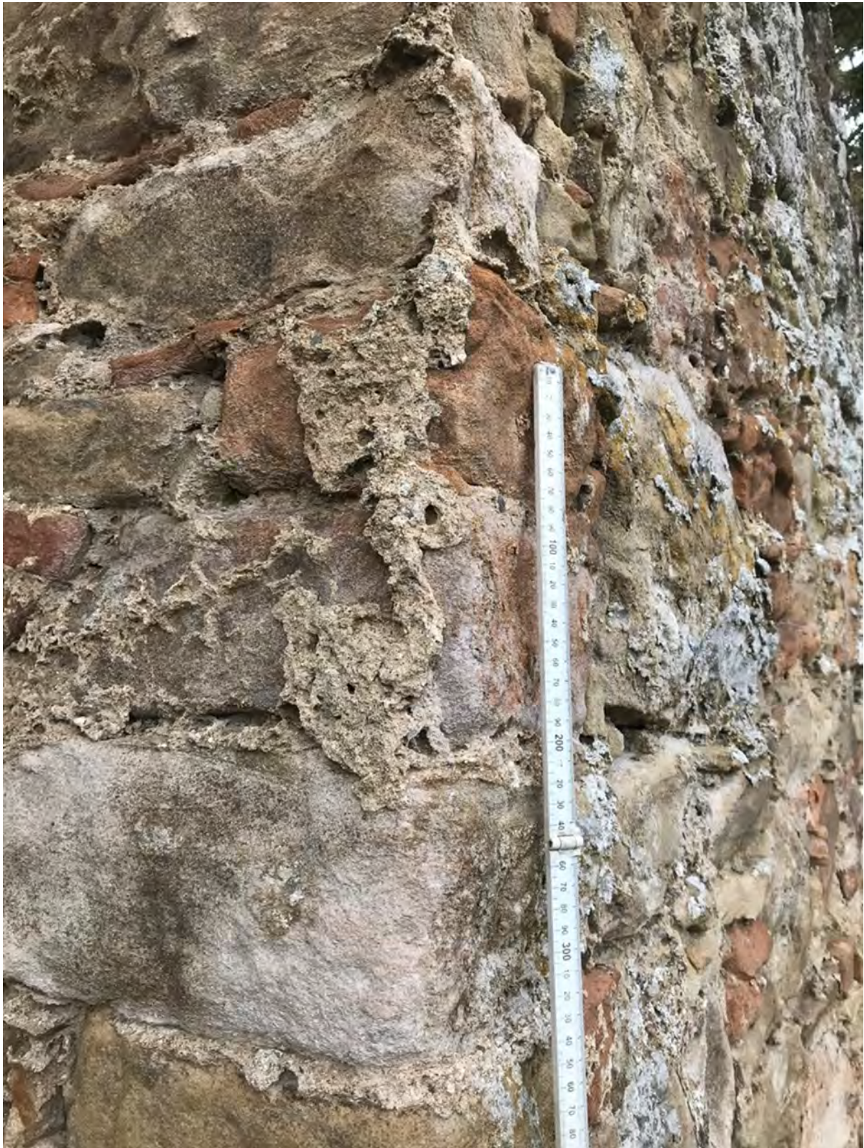
Figure 45.2. Detail showing harl remnants, some harl visible on the quoins.
