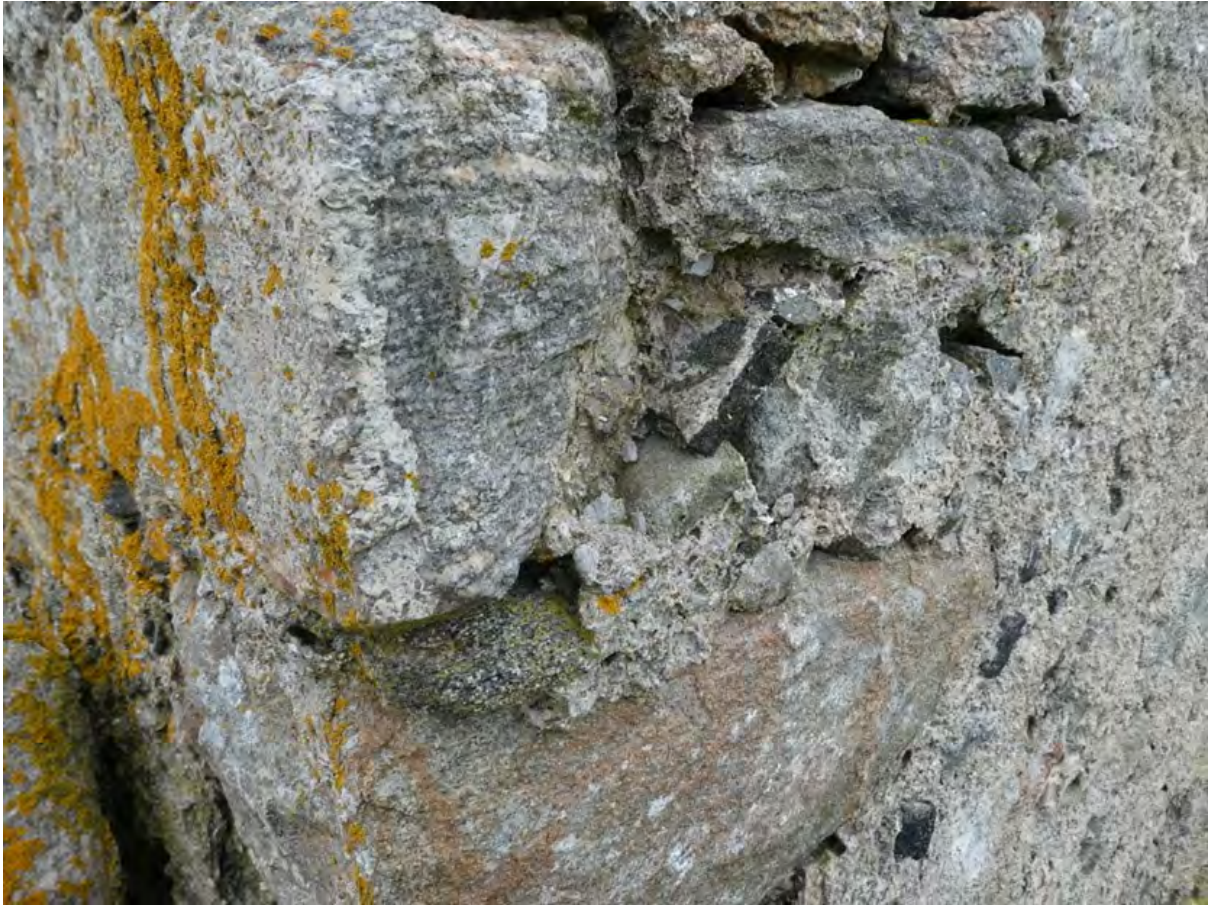
Figure 39.2. Remains of integral exterior harl.
