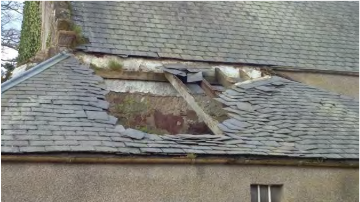
Figure 6. The collapsing roof of a later lean-to revealing earlier exterior harl applied to the rear of a 17th century building in Angus.
