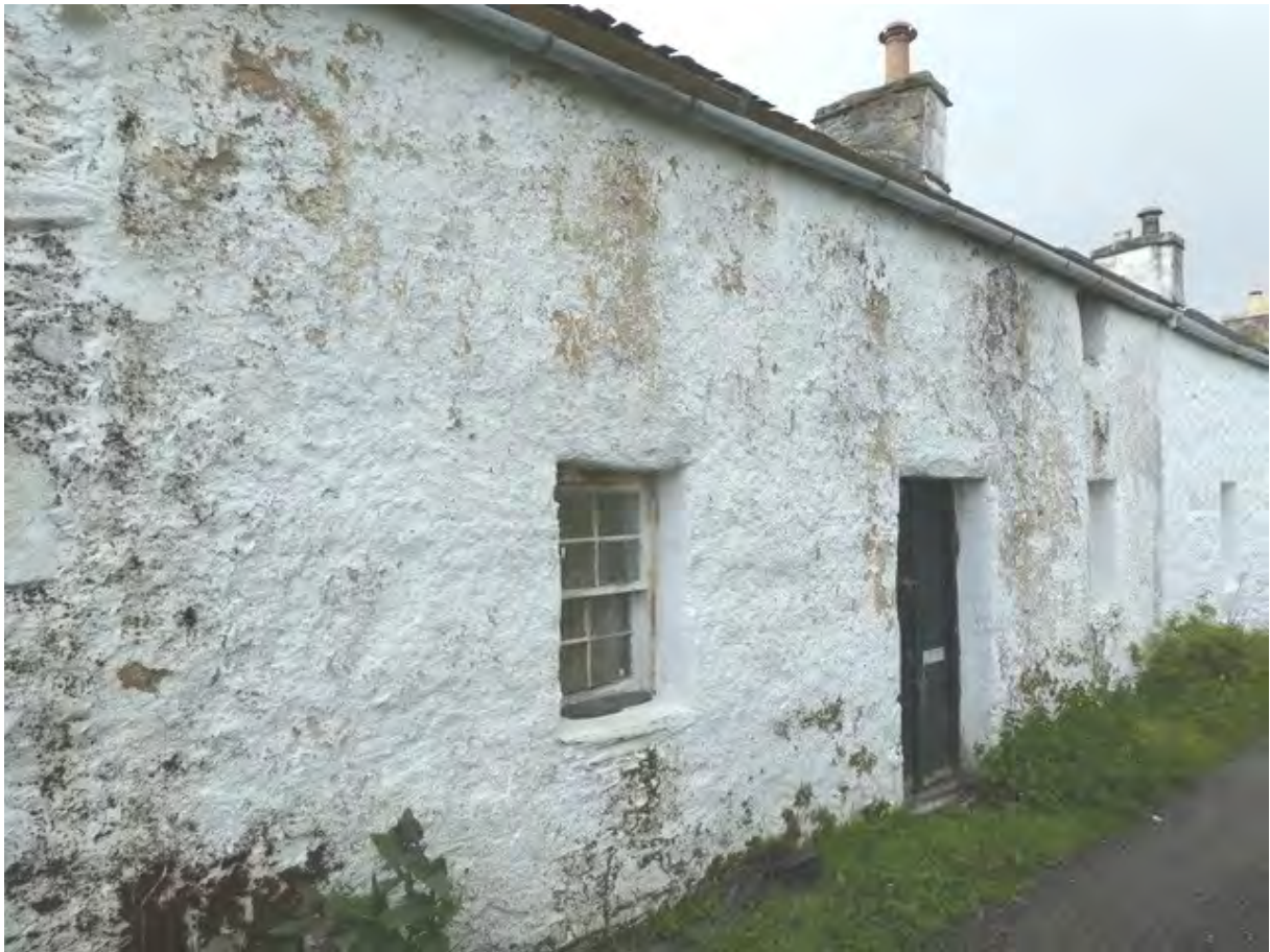
Figure 60.1. The West elevation of the cottage showing the nearly intact lime harl.
