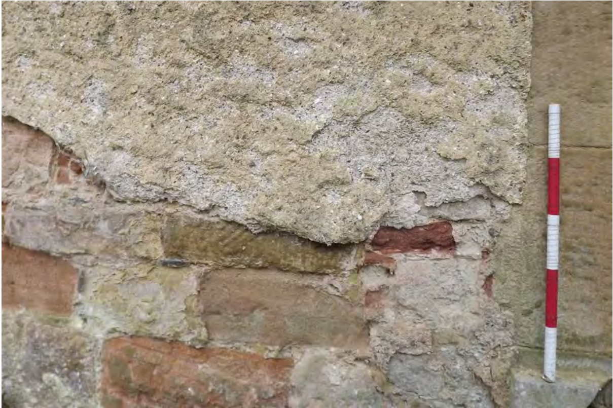
Figure 46.3. Area of remaining harl over rubble masonry.
