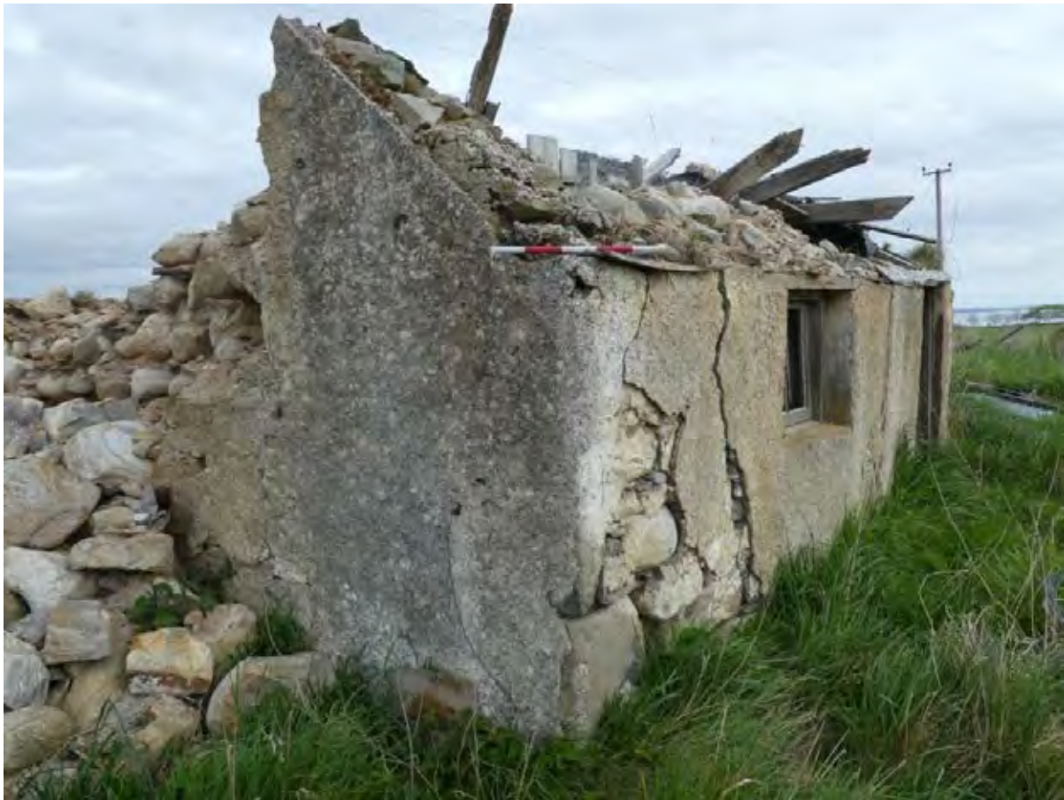
Figure 63.1. General view of the collapsed structure.
