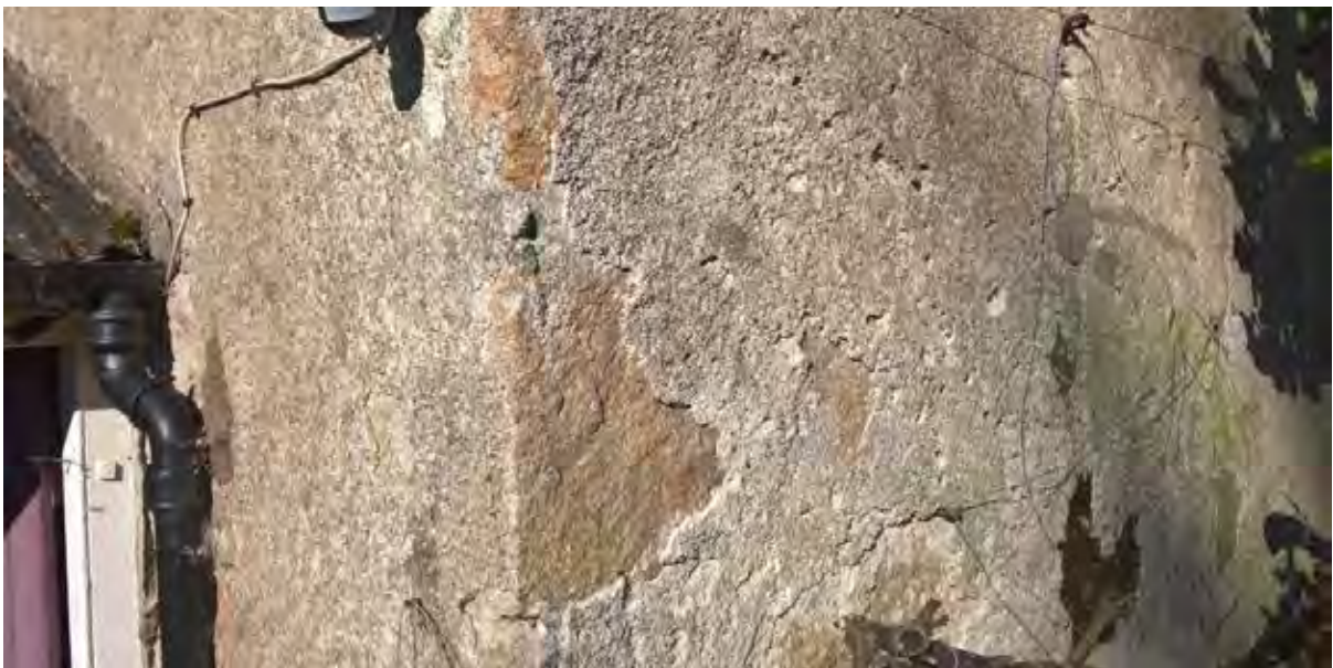
Figure 36.4. The harl is adhering relatively well to the quins, but some spalling.
