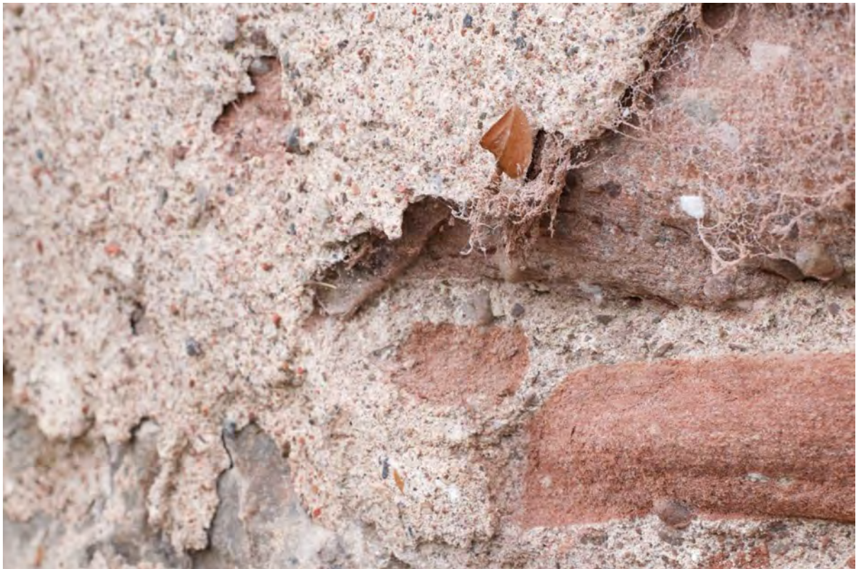
Figure 67.3. Detail of integrated finish seen at a damaged area on the gable; note the bedding mortar and harl are the same mix.
