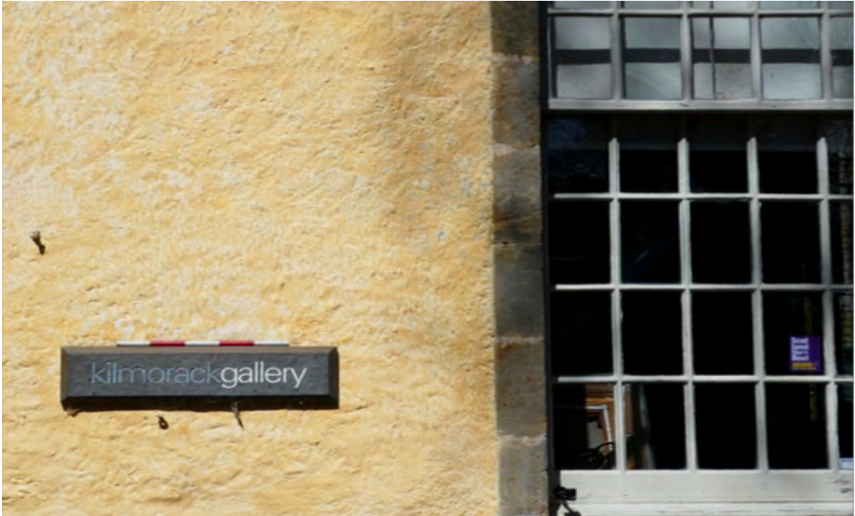
Figure 2. Kilmorack Old Kirk, Beaulieu, Inverness. Fading harl and limewash against the raised margins of the window.
