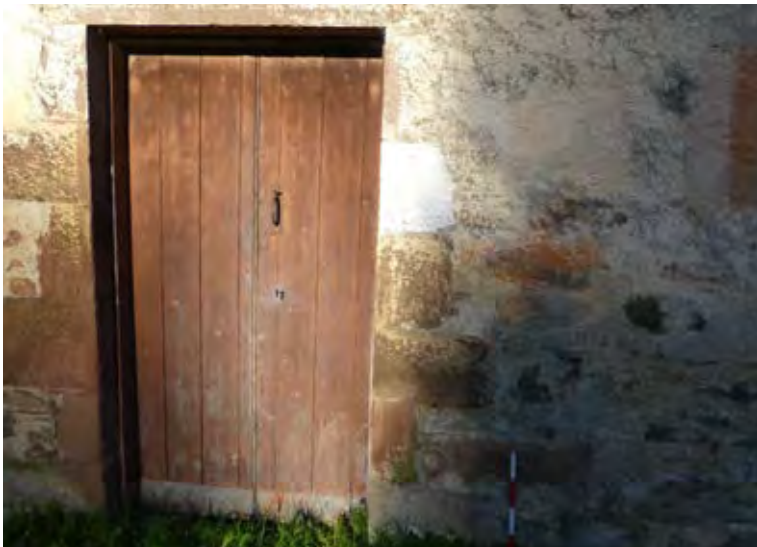
Figure 47.3. Degrading of the harl close to ground level.
