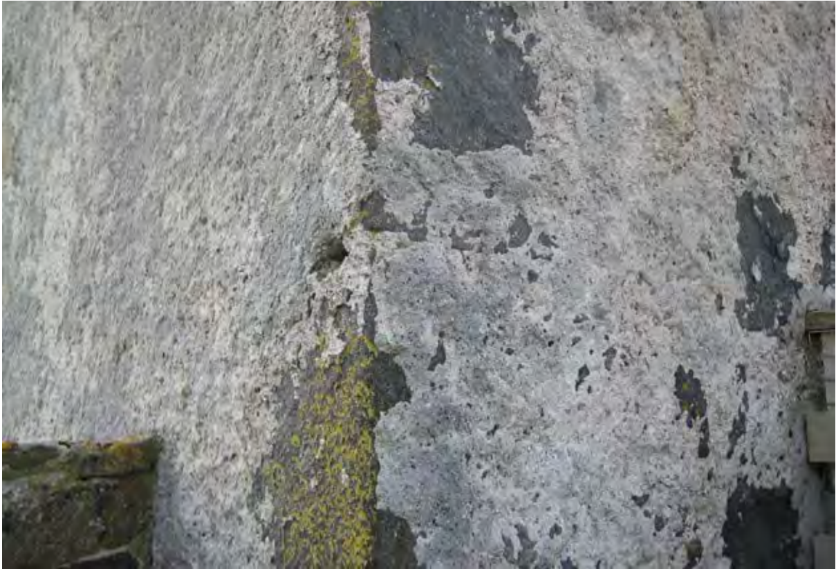
Figure 07.3. The historic harl covering the quoins at the south east corner of the tower.
