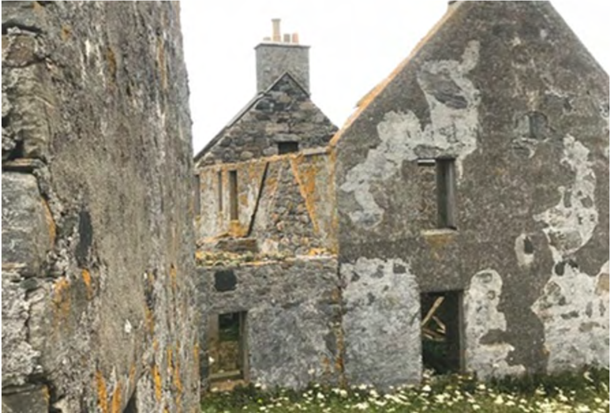
Figure 43.2. Integral harl on the gable wall of Old Vallay House (left). In contrast to the delaminating harl on the gable wall of Vallay Farm House (right).
