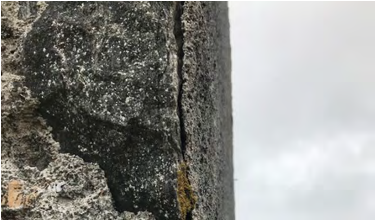
Figure 43.3. Vallay Farm House, the newer separately applied harl coming away from the wall.
