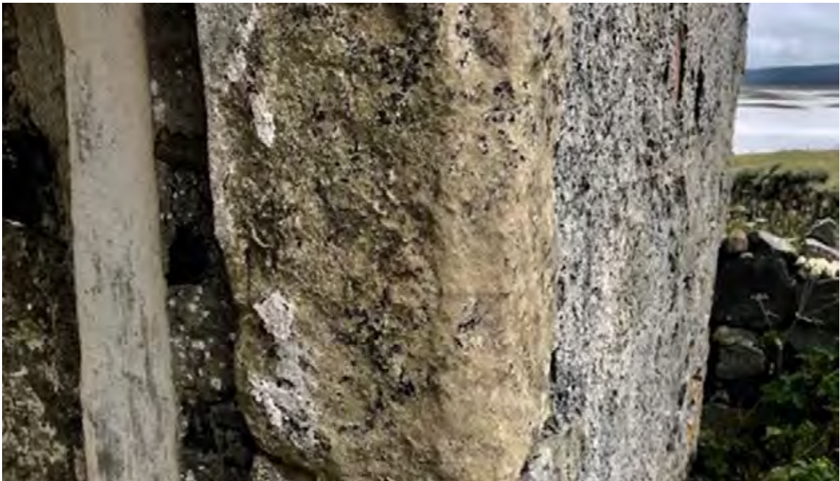
Figure 28.3. Detail of the harl dying out at the chamfer and terminating at the window frame.
