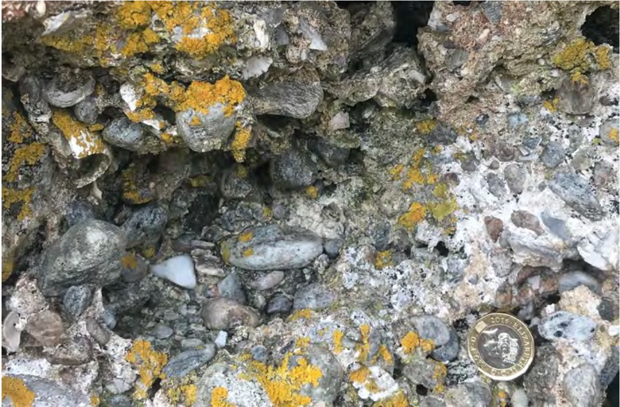
Figure 05.2. Detail illustrating the coarse nature of the mortar as it approaches the wall face.
