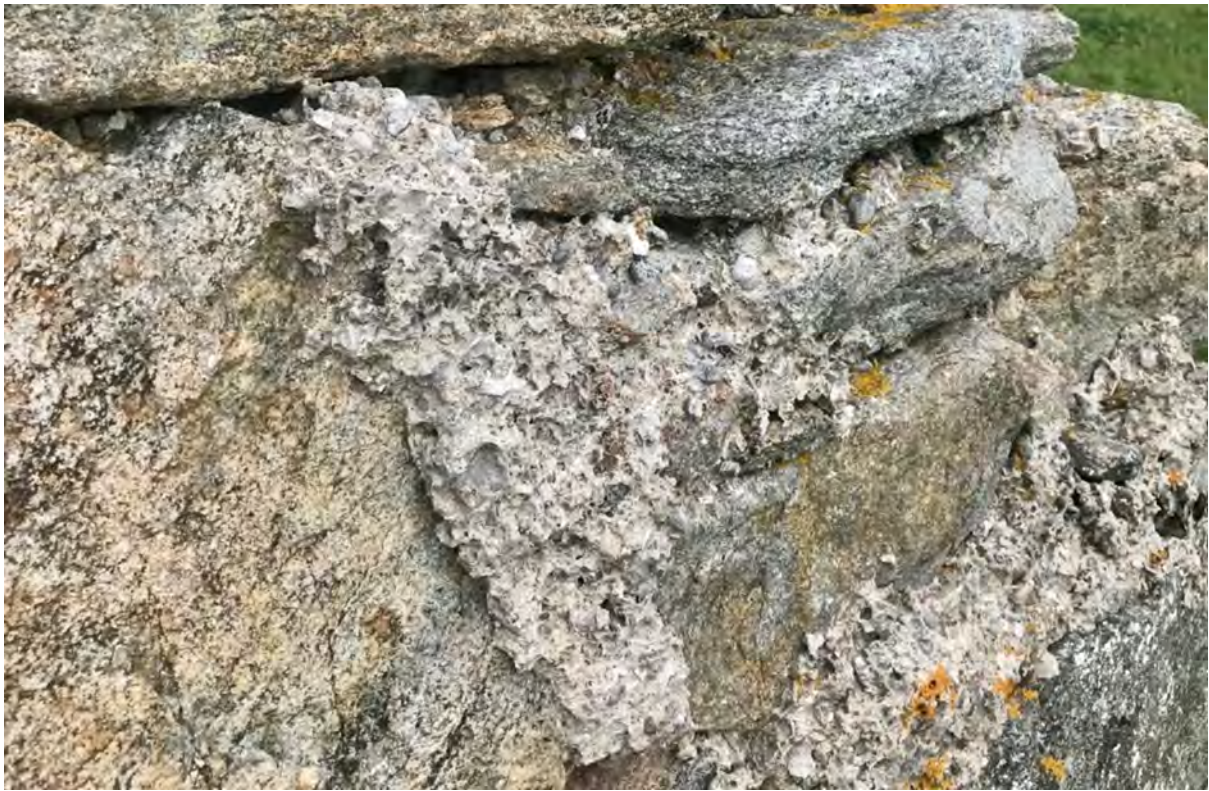
Figure 05.3. Localised survival of areas of surface harl finish, with evidence of integration of the finish with the joint. Note also the marine inclusions.
