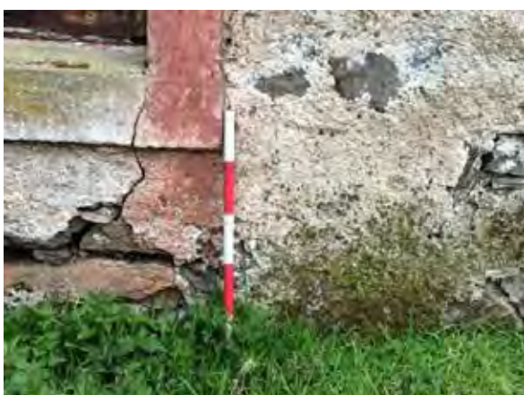
Figure 48.2. The harl exhibits no evidence of complete limewash, but does resemble the neighbouring barrack blocks in terms of texture and robustness.
