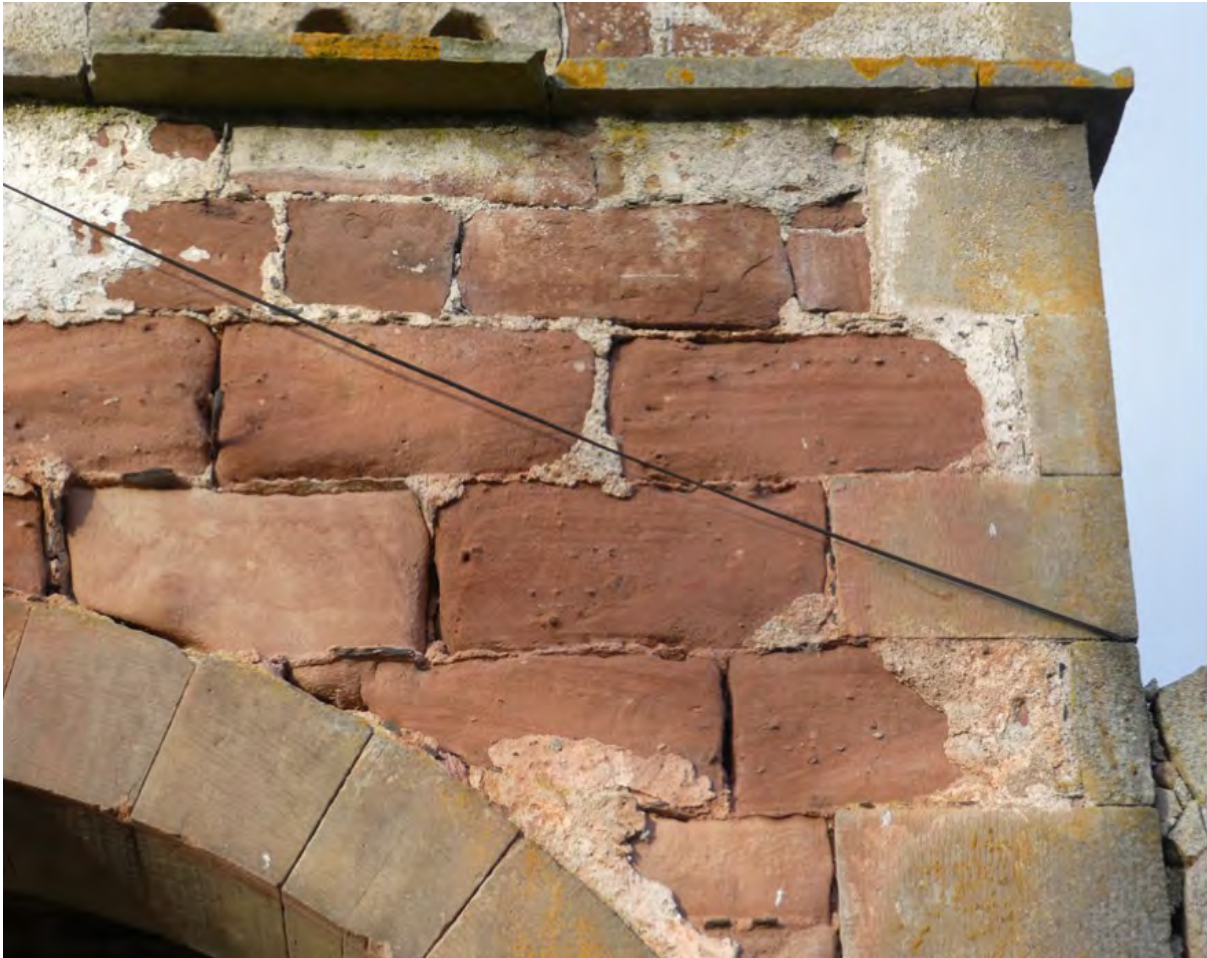
Figure 24. Harl clings to some areas protected by the string course of this mid-18th century steading. In other areas, where there is less protection, the surface of the sandstone has completely eroded away, taking with it any trace of finish.
