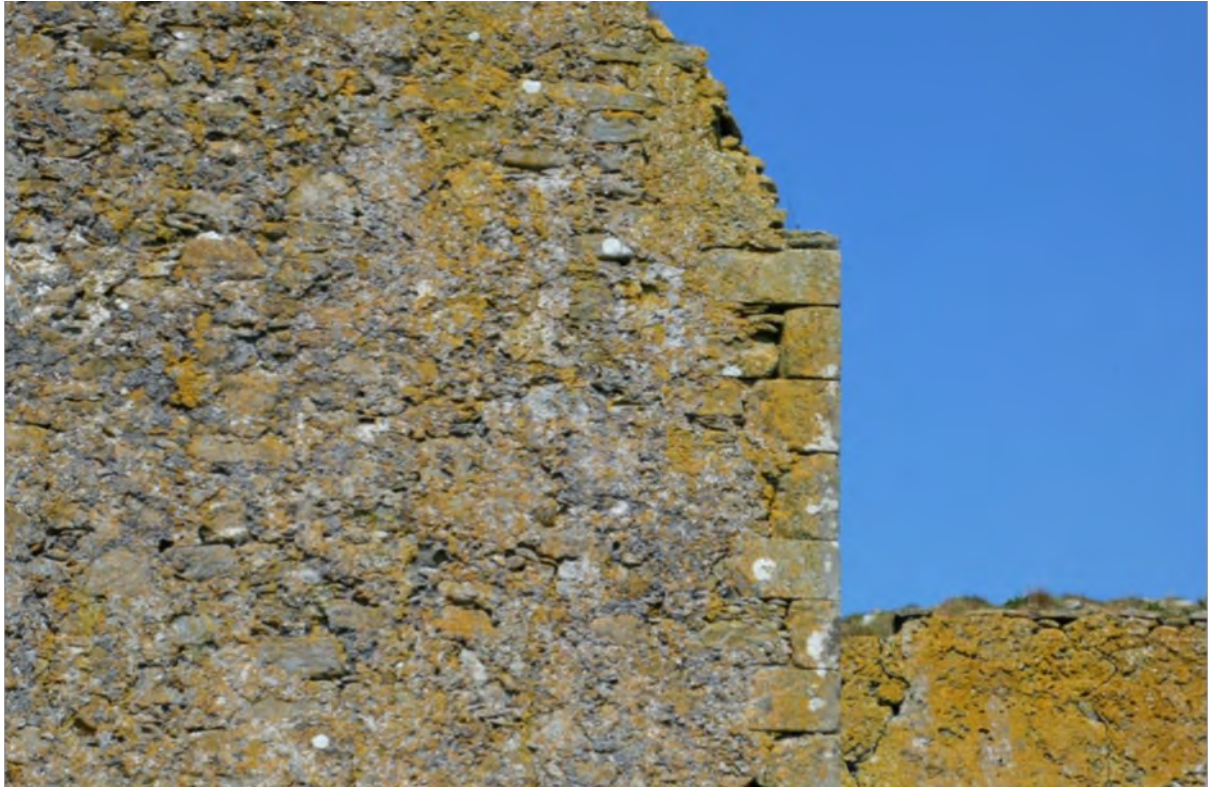
Figure 1. Ormacleit House, South Uist. Decayed harl surviving on the south-west gable.
