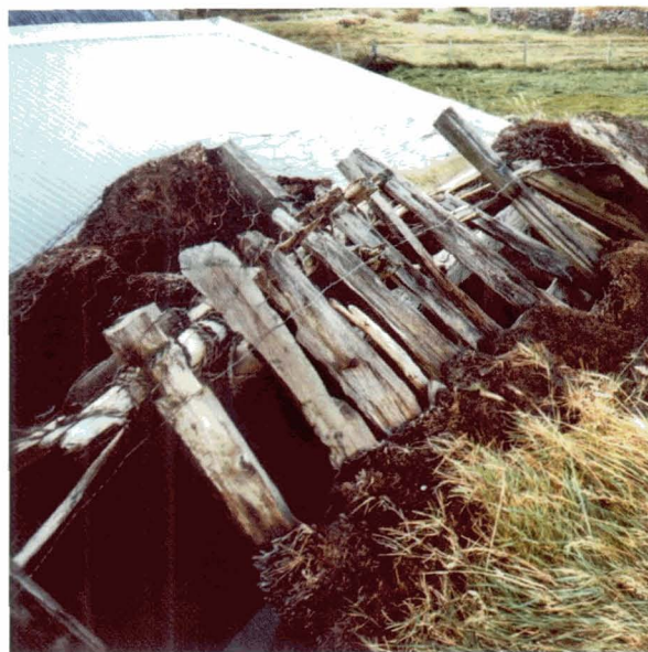
Illus 48 No. 9 Collapsed thatch roof (photograph by Headland Archaeology Ltd).
