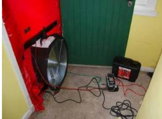
Fig. 3. Blower door testing to measure the air tightness of the unimproved building
