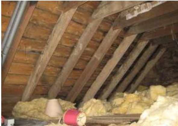
Fig. 4. Attic filled with variable depths of mineral wool and other discarded items, prior to the improvement works
