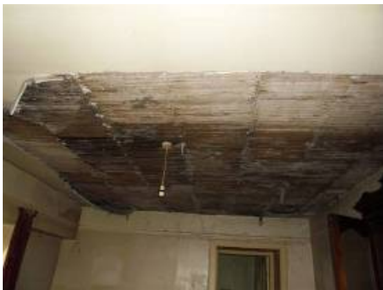
Fig. 6. Lath and plaster ceiling damaged by water leak
