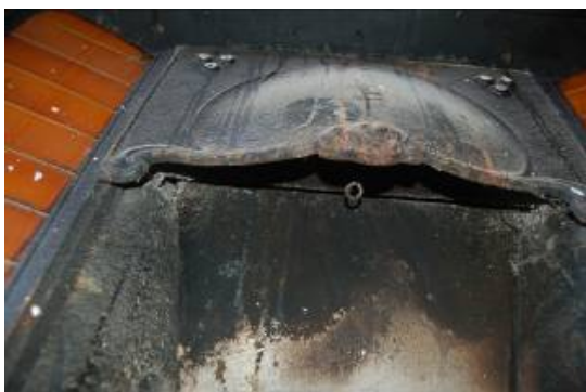
Fig. 17. The adjustable baffle allowing chimney ventilation to be controlled
