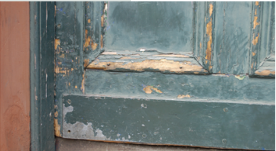
Fig. 1 External doors are subject to considerable wear and tear.
