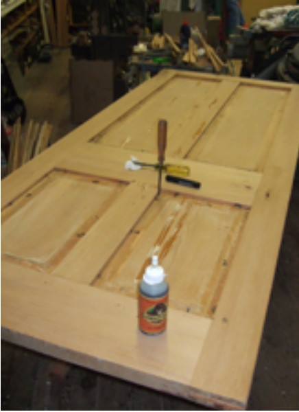
Fig. 6 Doors may need to be taken off for repairs.
