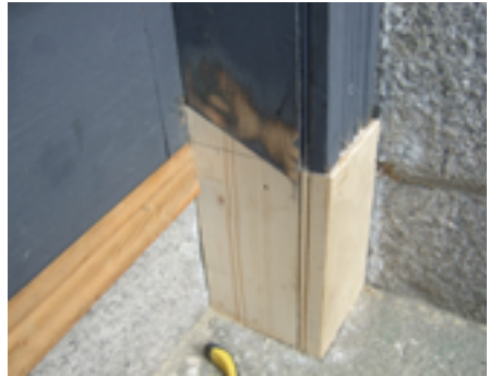
Fig. 5 A new piece of timber spliced in to replace a rotten section.
