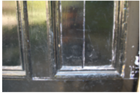
Fig. 4 Shrinkage or impact damage can cause door panels to split.
