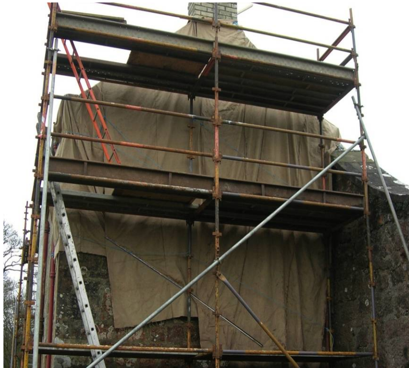
Fig. 3. Repointing masonry to prevent water ingress was a key part of the enabling works for the project which had to take place before any thermal improvement work could be undertaken
