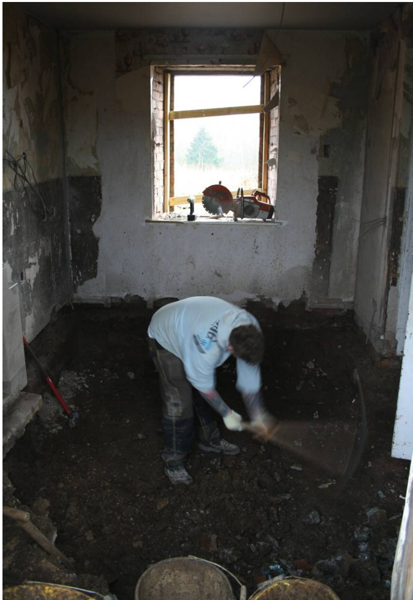
Fig. 7. Excavating the floor in preparation for the insulation layer being put down
