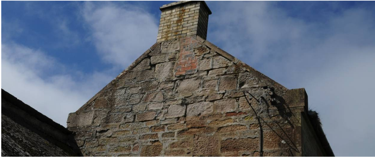
Fig. 2. The east gable end of the Garden Bothy, prior to enabling works
