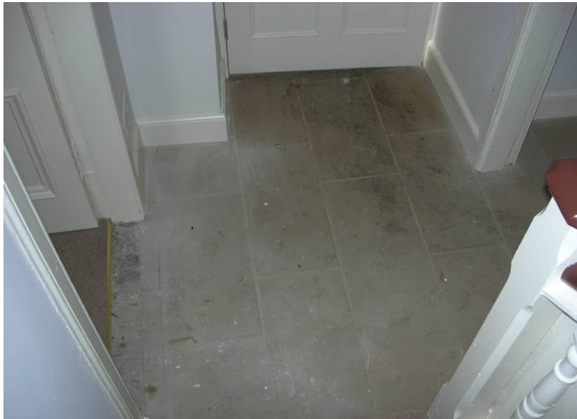
Fig. 12. British sandstone flagstones laid as a finish to the lime concrete floor
