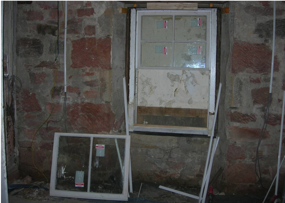
Fig. 13. Original sashes with new double glazed units being installed in repaired cases
