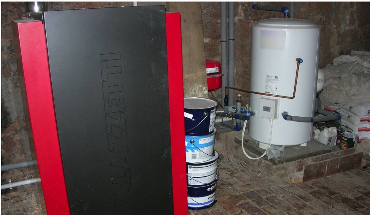
Fig. 16. The pellet fuelled biomass boiler and hot water tank
