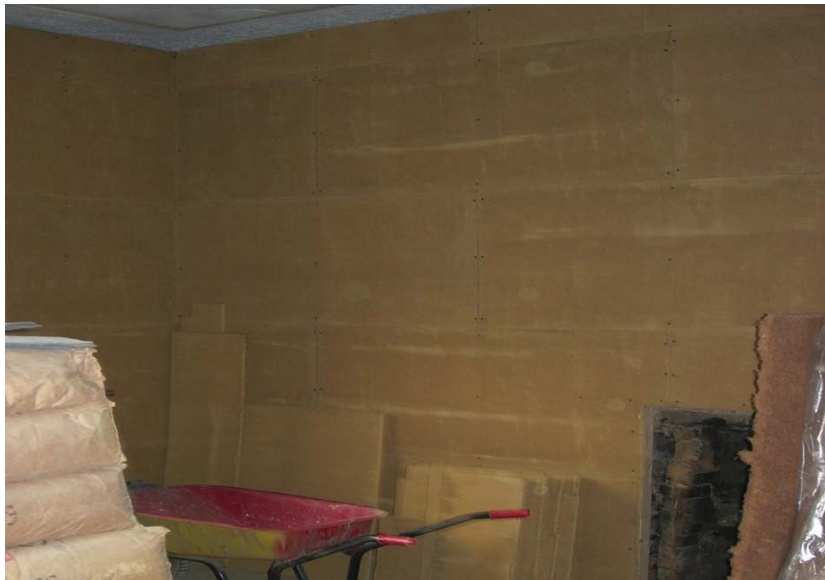
Fig. 4. Clay board in place over hemp board insulation ready to take clay plaster skim coat finish
