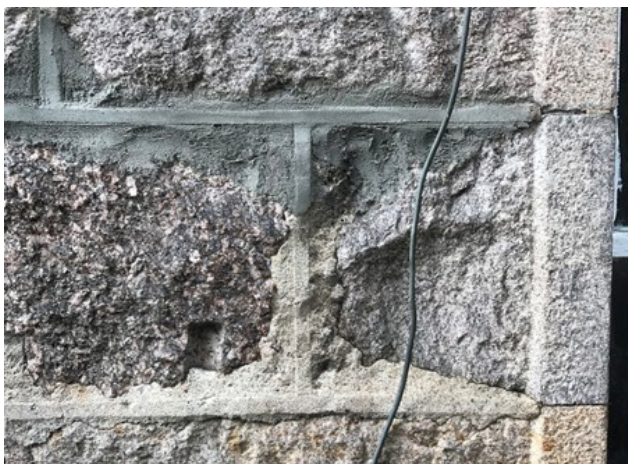
Figure 17: Strap or ribbon pointing in lime mortar, with later cement repairs above.
