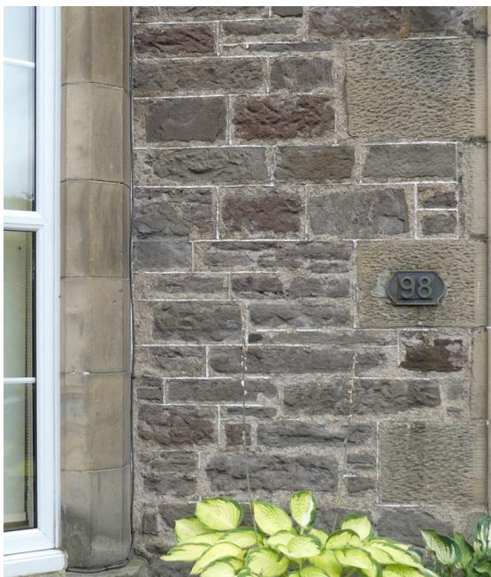
Figure 15 - Bridge of Allan. Front elevation is flush finished, ruled out and white lined.
