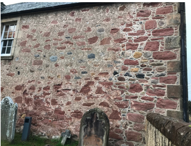
Figure 22 - This recently repaired building, using a lime mortar, illustrates well the change in the appearance of an elevation when a certain pointing style on the right is used in preference to what was clearly surviving on the left.
