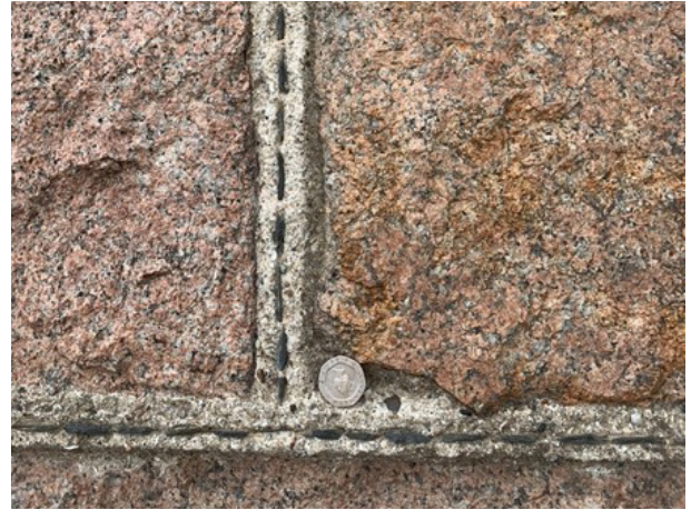
Figure 12 - Cullen, Moray. An early version of strap pointing with slate pinnings and a raised band of lime to form the joint (1810).
