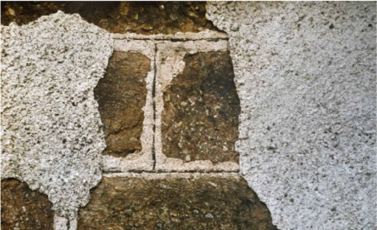
Figure 9 - An ancillary building at Craigston constructed with poor quality agglomerate sandstone with decorative slate 'cherry-cocking'. This has been retrospectively harled, which is assumed to be in response to decaying sandstone.
