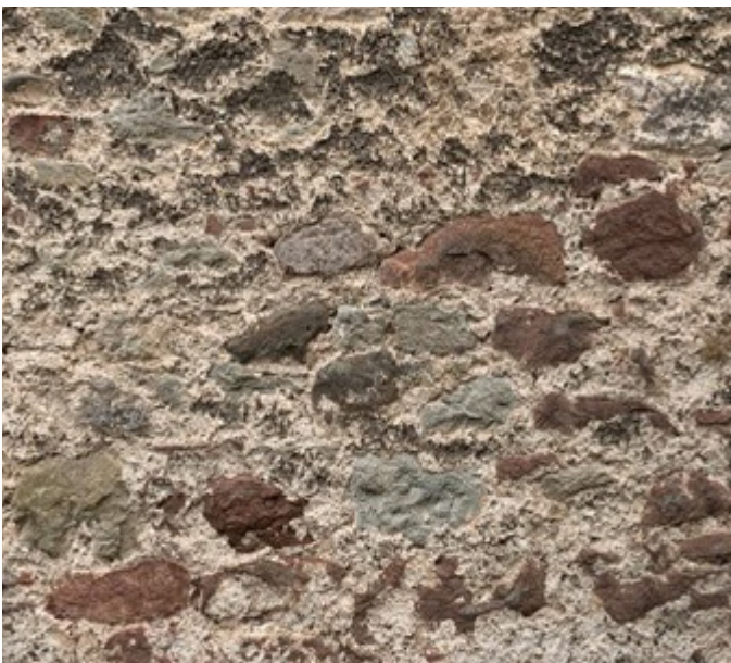
Figure 5 - Oven Wynd, Kelso. The decayed surface of what was once the typical finish for rubble. The full harl has graded away and it is difficult to differentiate this from an intentional 'sneck harl'.
