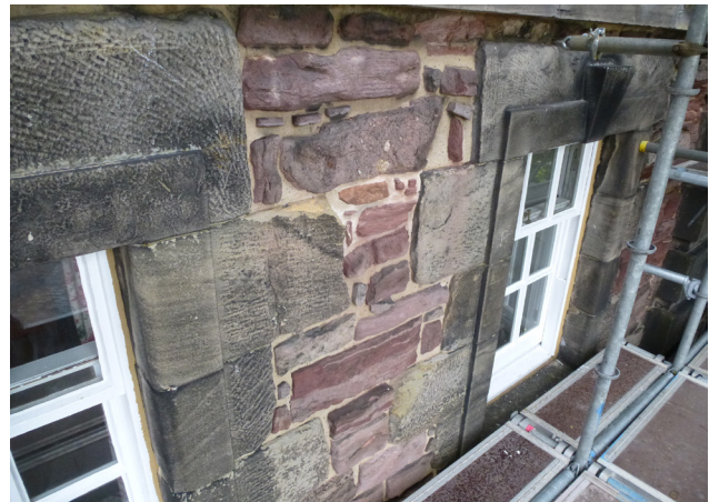
Figure 21 - The Governors house at Edinburgh Castle. Recessed pointing.
