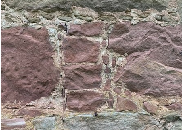
Figure 11 - Ladder pinning and cherry cocking showing on a building in Cromarty, where the covering harl has been lost.
