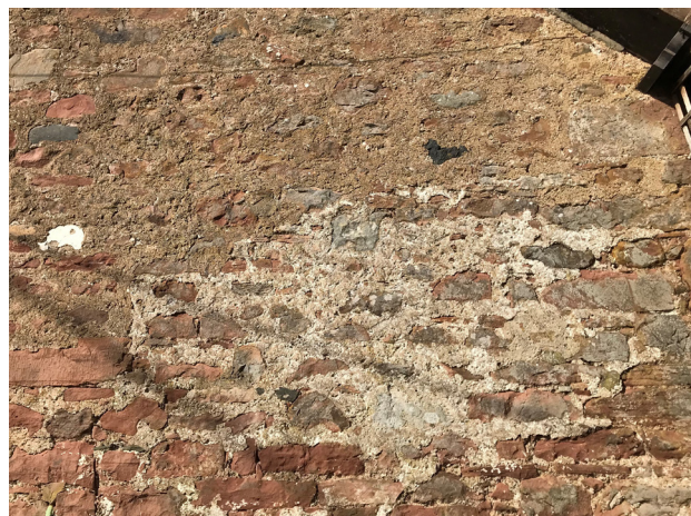
Figure 18: Weens Stables, Hawick. Above, un-limewashed flush point from 1905 (brown coloured mortar) with earlier 18th century work and limewashed flush pointing surviving below.
