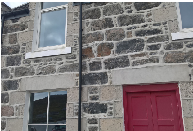
Figure 24 - New strap type pointing on a traditional building in the Hebrides. A significant change in the appearance of the building and in a style not previously found.
