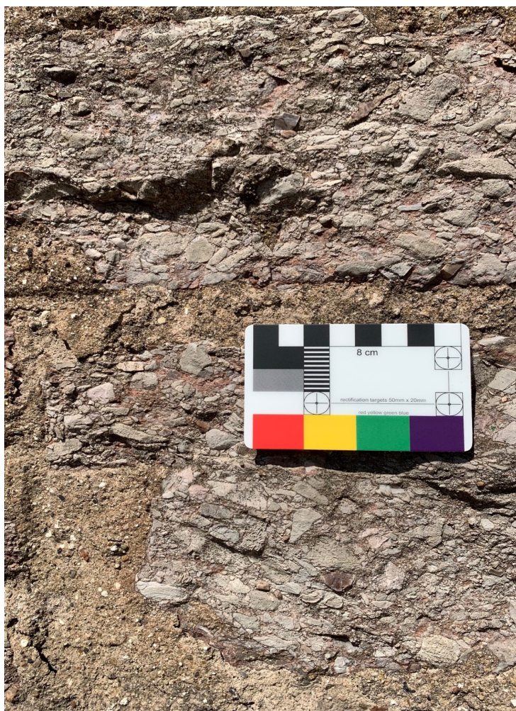
Figure 25 - A 19th century terrace in Kirkby Stephen. Flush pointing with traces of lining out.
