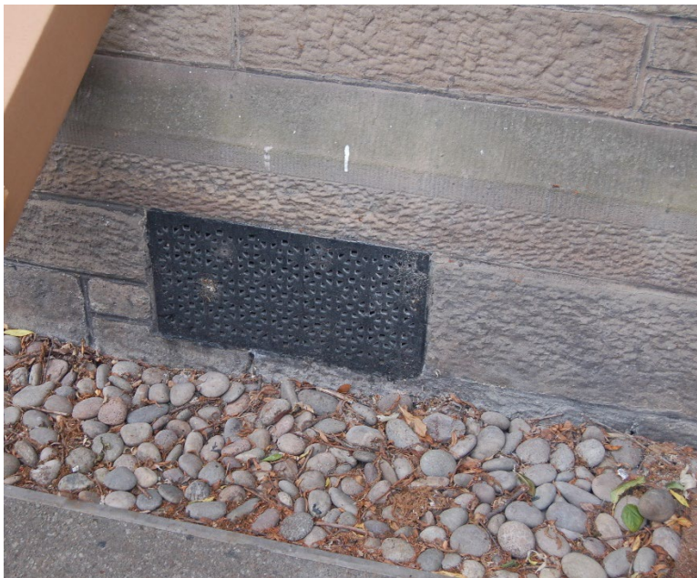
Figure 14. The external ventilation grilles to the floor void. These were cleaned to ensure full air movement.
