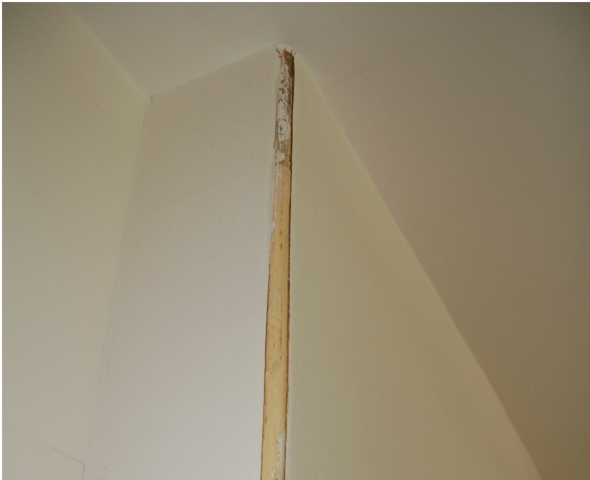
Figure 30. During the redecoration, the configuration of the timber corner detail, called a 'quirk', was re-instated.
