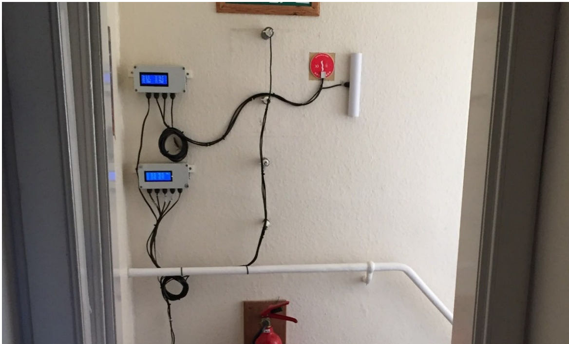
Figure 9. The in-situ U-value and humidity measuring equipment in place at the top of the stairwell. Note the four probes measuring humidity within the wall.
