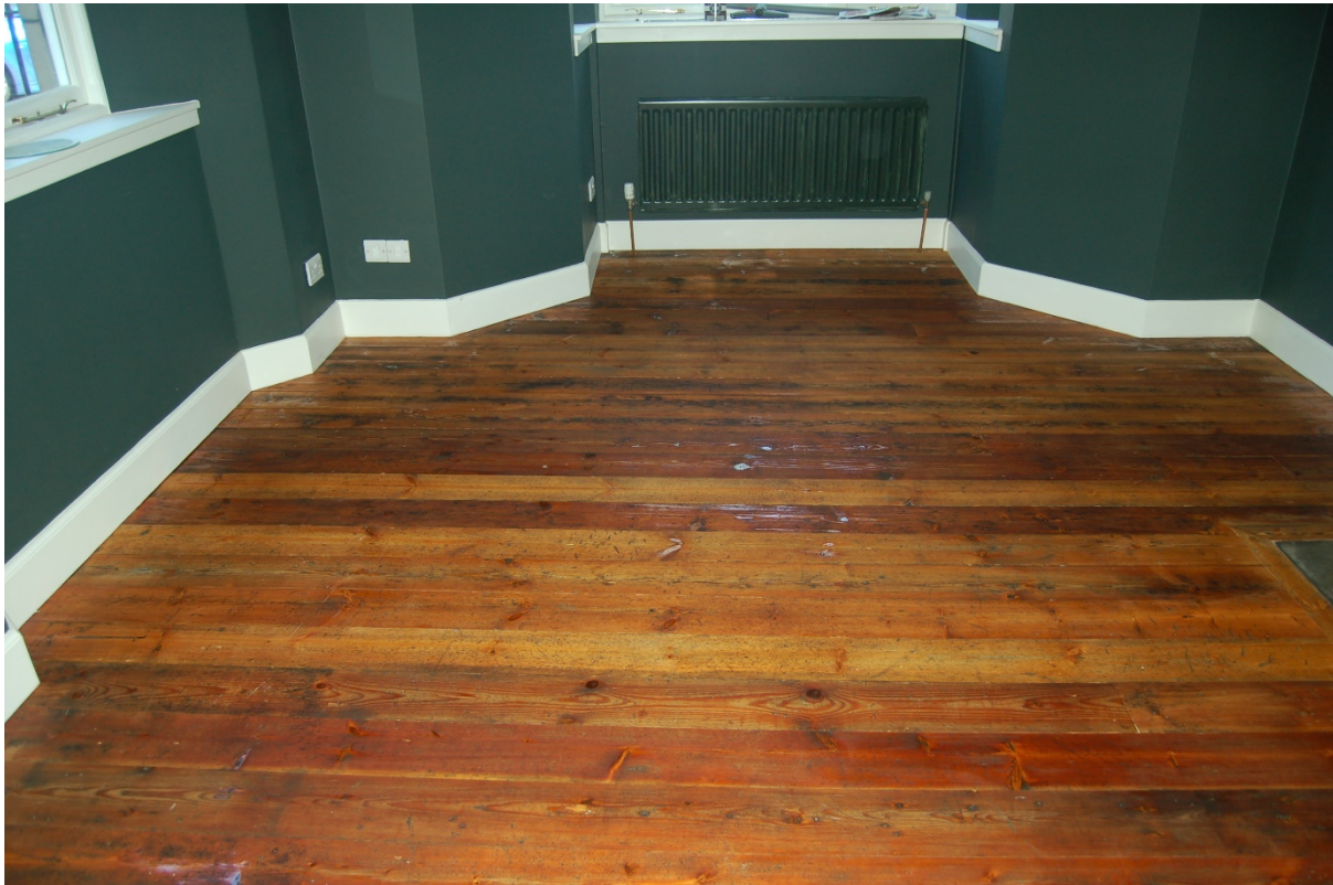
Figure 18. The re-laid floor in the exhibition room, note the rich colour of the historic timber and the mitred edging around the hearthstone on the right of the image.
