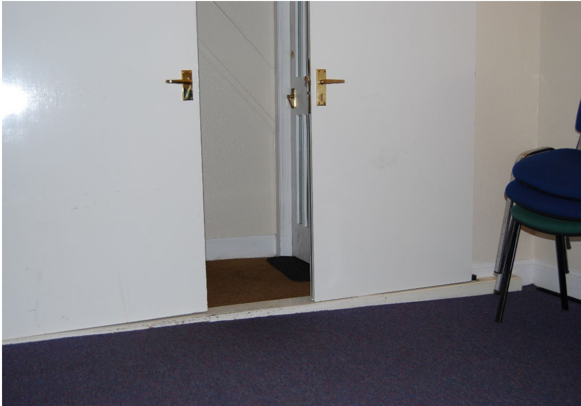
Figure 4. The downstairs meeting room showing the modern finishes and the settlement of the timber floor.
