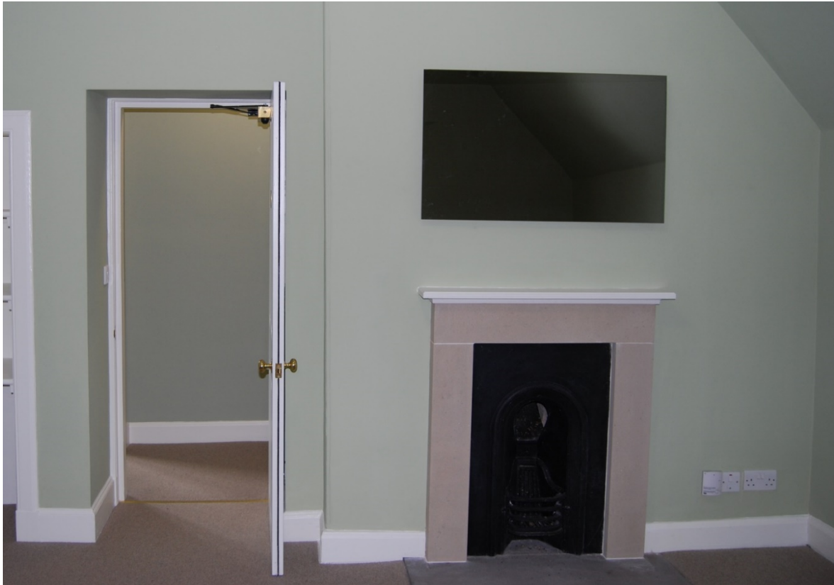
Figure 31. The infrared heating panel over the chimneypiece in the meeting room.
