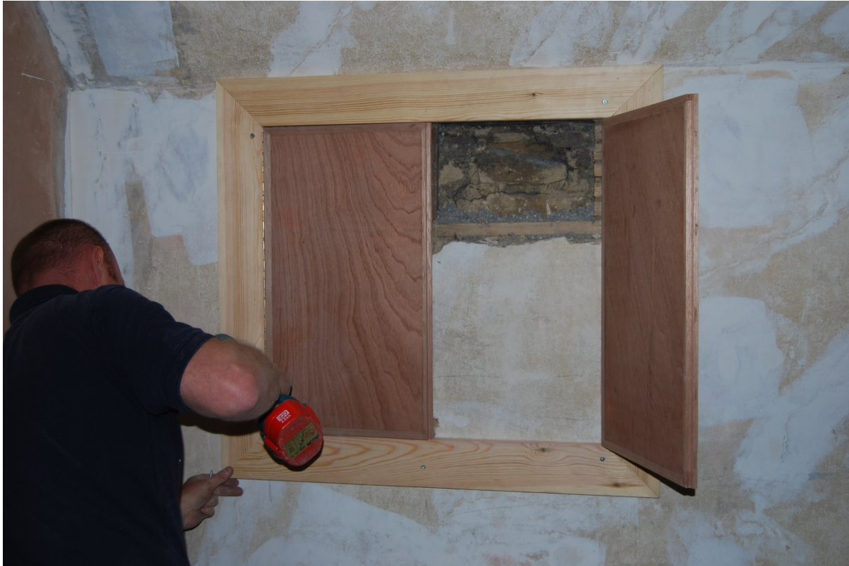
Figure 19. Fitting the interpretation panel to show the blown cellulose fibre behind the lath and plaster.
