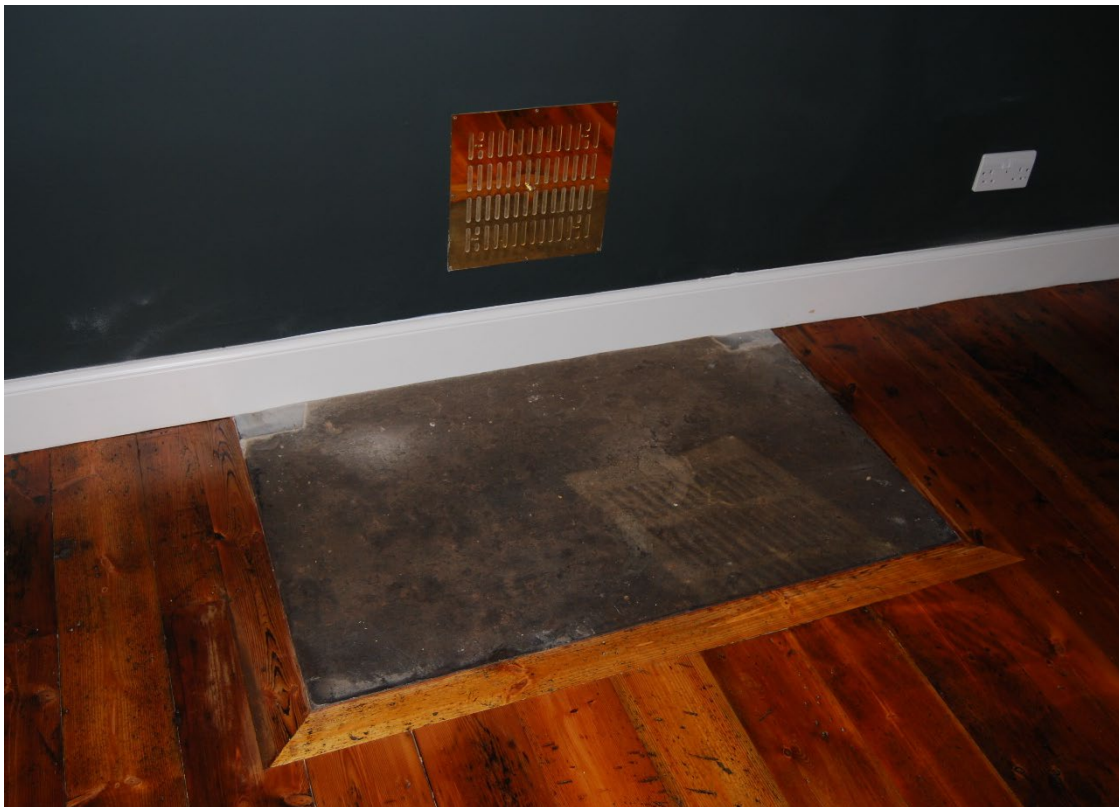
Figure 27. The new ventilation grille in the former hearth in the interpretation room.
