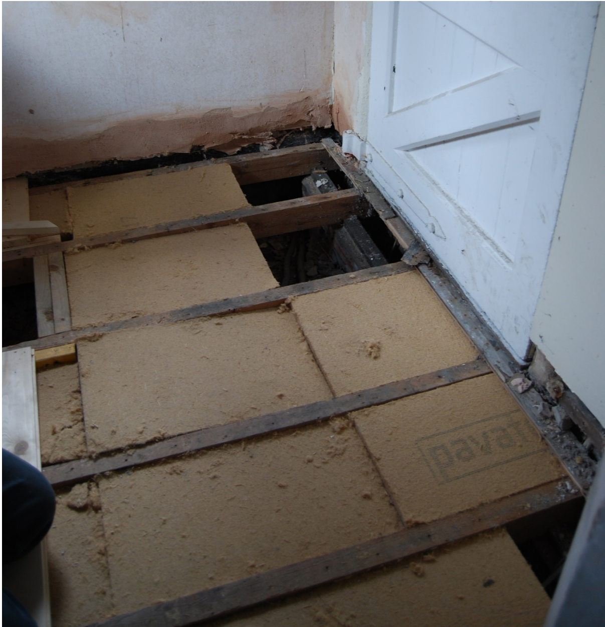
Figure 17. The floor insulation in place between the joists in the hall prior to the boards being laid.
