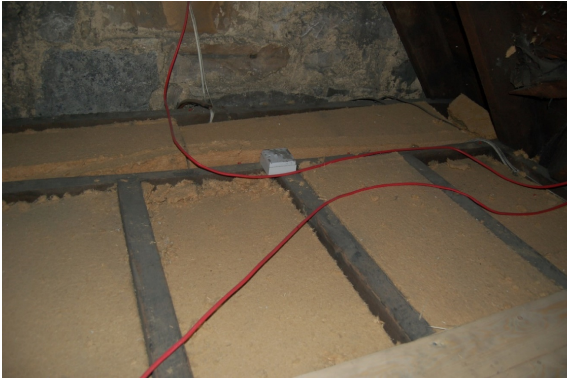
Figure 24. The wood-fibre insulation batts laid flat between the ceiling joists to give a 'cold roof'.
