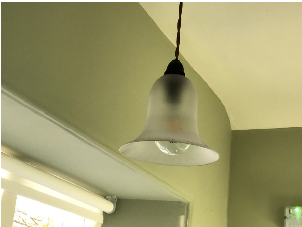
Figure 29. New light fittings of traditional pattern contributed to the improvement in amenity at the Lodge.
