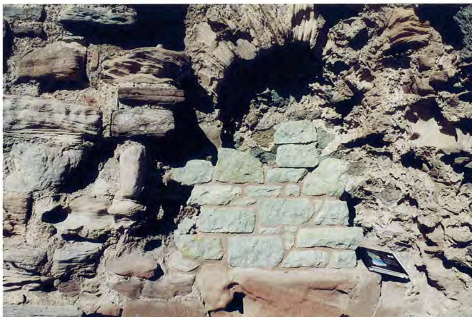
Figure 3.3: Small trial panels for mortar and masonry built on site help to assess the appearance of a replacement mortar and also its longer term durability, and compatibility with the associated materials.
