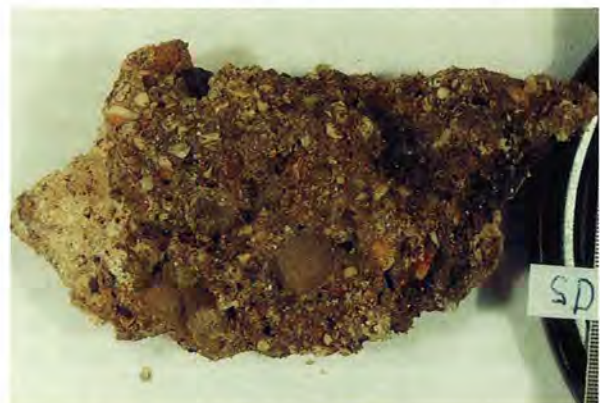
Figure 5.6 Historic mortar sample from St Andrews Cathedral precinct wall (early 16th Century). This image shows an external weathered surface of the mortar, which is darkened compared to a fresh unweathered surface. The weathering can accentuate features like the aggregate, especially if the lime binder is preferentially weathered away.
