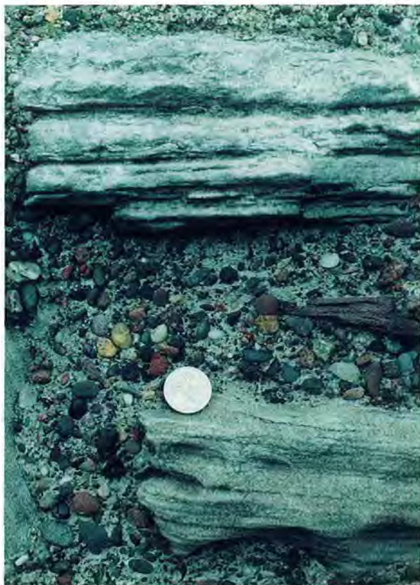
Figure 3.2: Sandstone masonry has been repointed with cement gauged mortar where a technique called 'Stirling grit wash' was applied to make the repointing look more weathered by exposing the aggregate. Although the pointing is done to resemble historic, weathered surface masonry, repointing in this or some other modern technique can be easily distinguished by any careful observer. However, when a traditional technique and materials are used, the distinction after some time and when it weathers, is much more difficult to make, without more detailed analytical techniques. Tantallon Castle, pound coin for scale.
