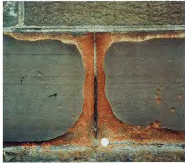
Figure 5.2: Is this mortar compatible with the masonry? Red sandstone ashlar masonry in Paisley. Cement based pointing mortar together with moisture and salt transport is often thought to cause such typical decay round the joints. The adjoining white sandstone is not suffering such extensive damage, suggesting the mortar is more compatible with that stone regardless of its composition.
