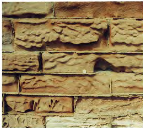
Figure 5.3: Is this mortar compatible with masonry? Red sandstone masonry has weathered due to wind exposure in combination with moisture evaporation. However, the hard pointing mortar has determined the weathering pattern and helped the weathering rather than protecting the masonry. It could also be said that the combination on a masonry surface of such materials with contrasting durability (related to the bond between components and overall hardness) has resulted over time in this aesthetically problematical weathering pattern, as the sandstone weathers away more readily than the cement-based mortar.
