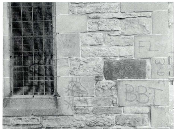
Illustration 32: City centre church. Graffiti on sandstone. Note spray paint on mesh window screen.
