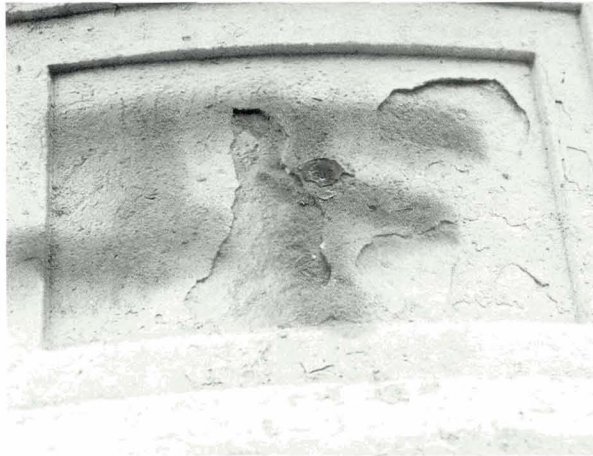
Illustration 12. Graffiti on decayed limestone surface.
