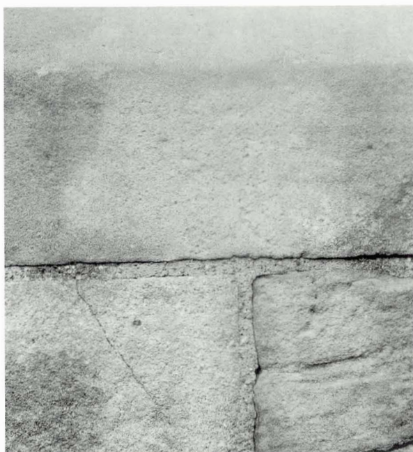
Illustration 5. Loss of sandstone surface by over aggressive graffiti removal.
