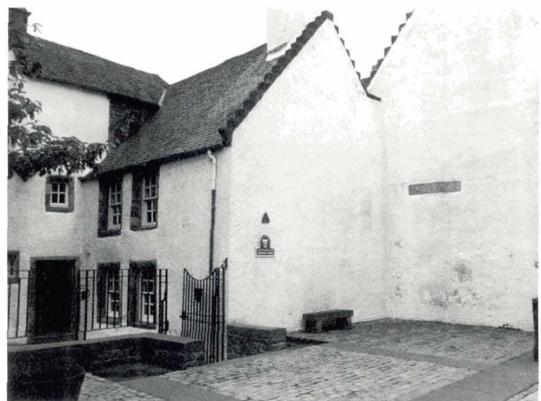
Illustration 34: Historic house. The harled recess is vulnerable to graffiti attack.
