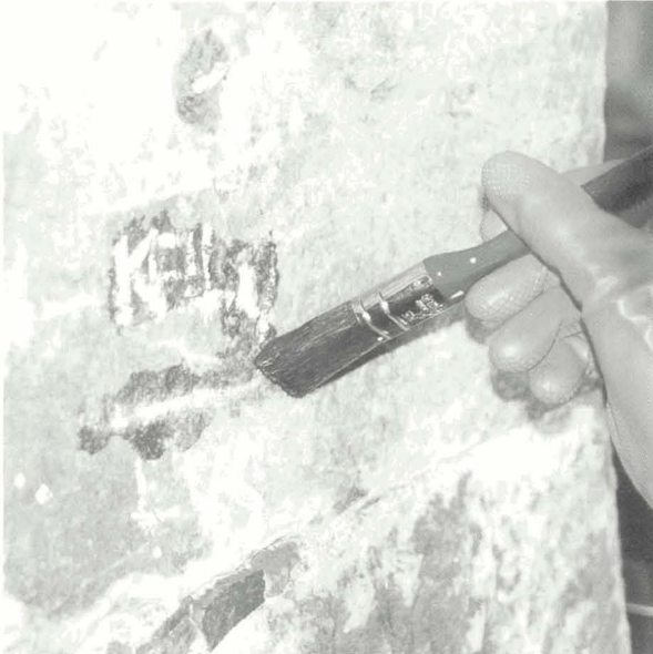
Illustration 28. The first application of paint stripper gel to the graffiti. Note the weathered surface of the sandstone.
