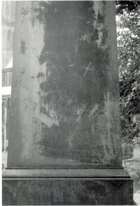
Illustration 24. Graffiti scratches on soiling on a sandstone headstone in a historic graveyard.
