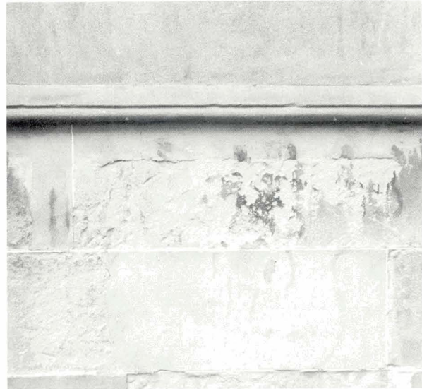
Illustration 9. Decayed sandstone showing increased damage because of attempts to remove graffiti paint. The undamaged surface is an area of plastic repair.
