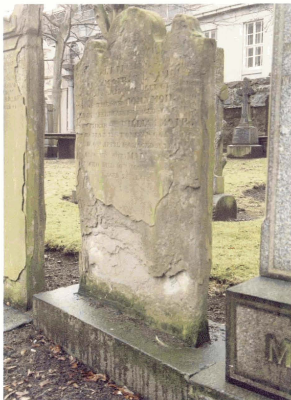
37. A typical example of the sandstone decay mechanisms shown in Illus 36
