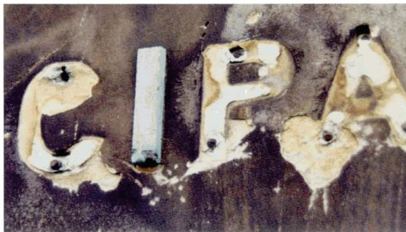
31. Applied metal lettering has been forcibly removed with resulting damage to the stone surface
