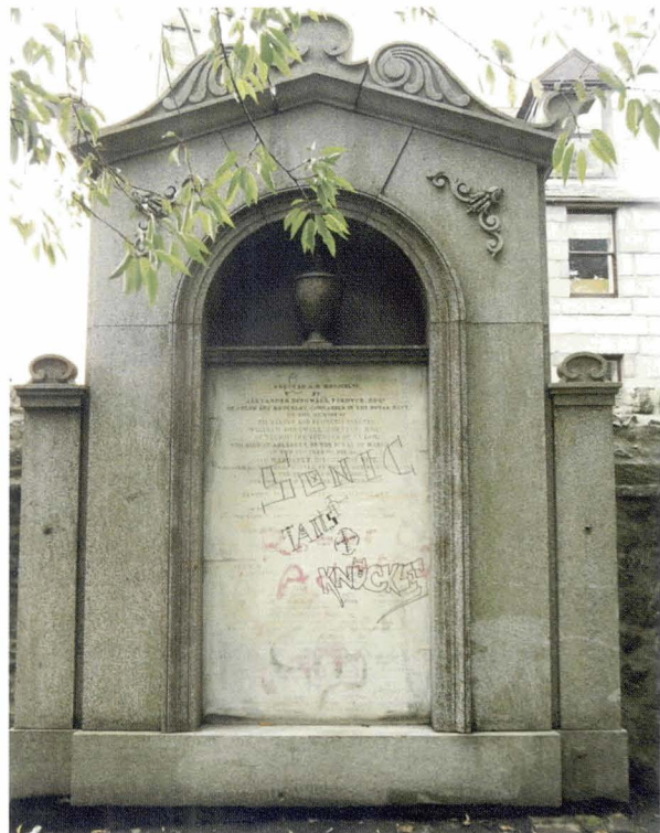
120. Loss of surface on a marble slab as a result of repeated graffiti removal
