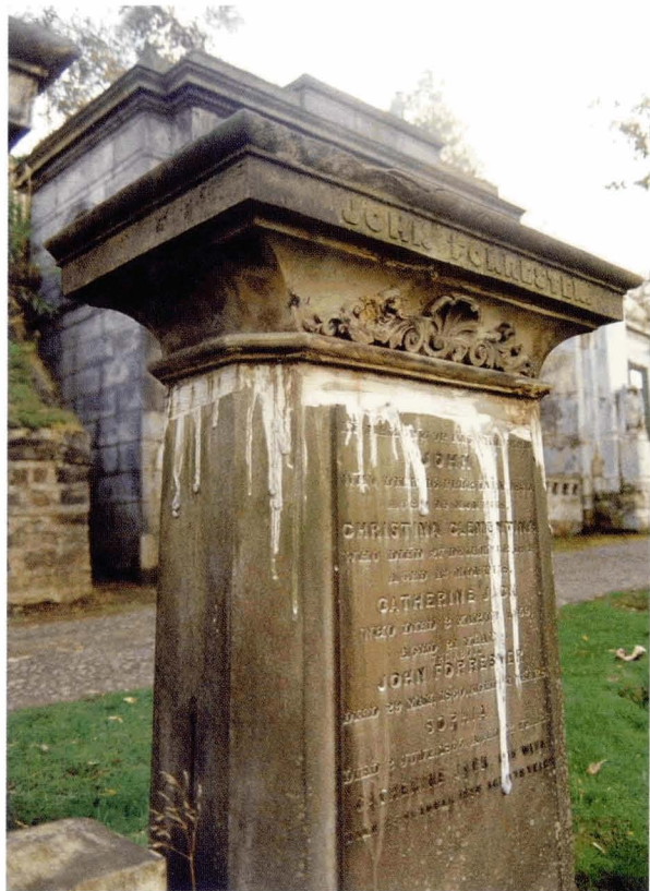
69. Example of a poorly executed mortar repair
