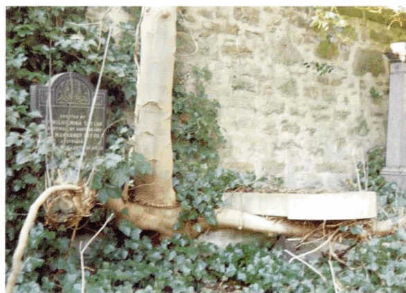
100. An example of damage due to uncontrolled tree growth
