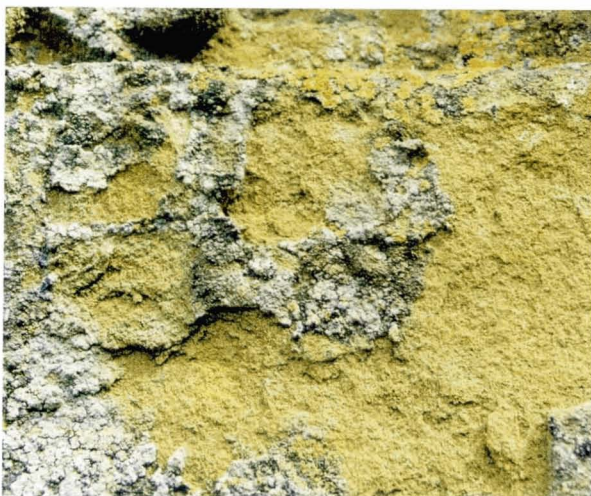
40. Typical example of long-term surface loss from sandstone
