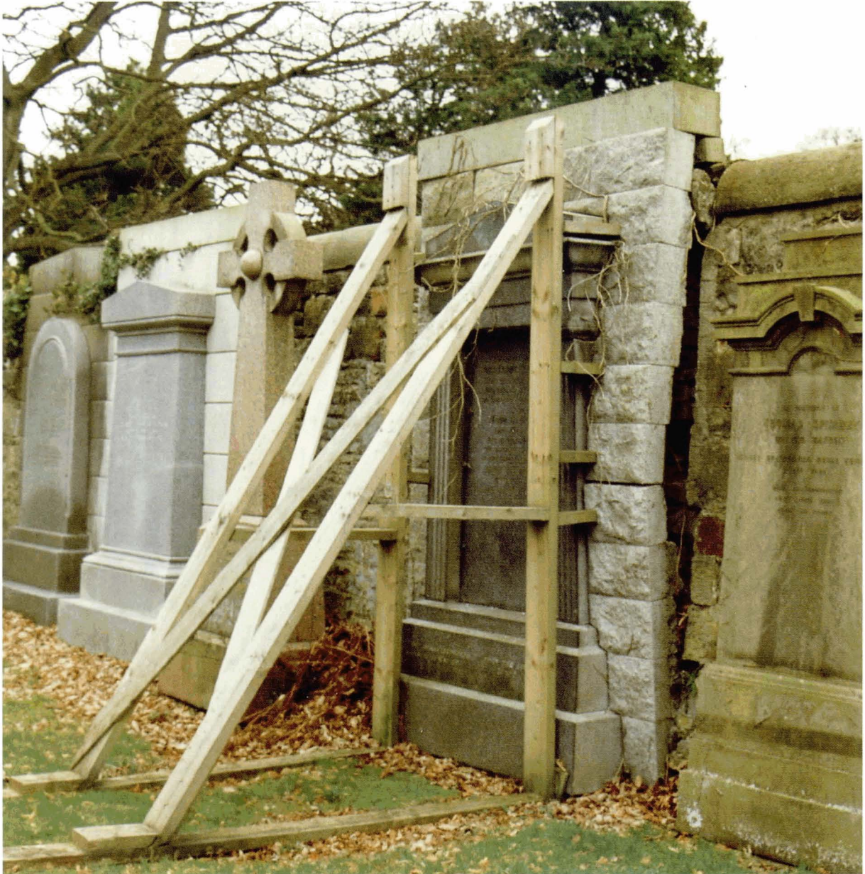
63. Temporary timber shoring to support a badly constructed backing wall which has separated from the adjacent boundary
