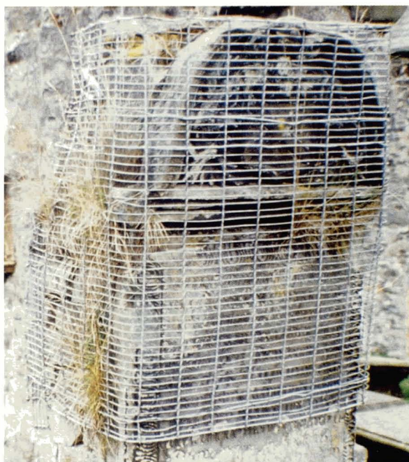
64. Galvanised steel retaining cage
