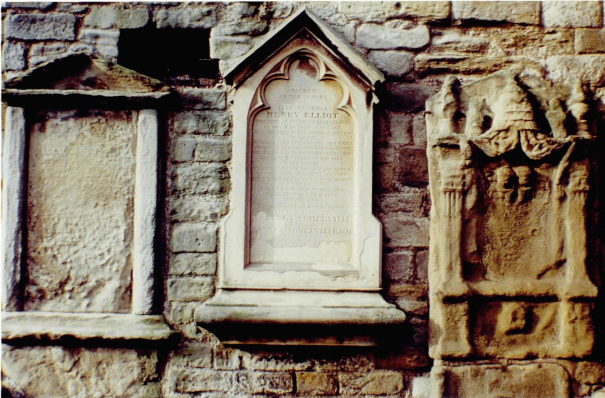
34. Weathering effects on a range of different sandstone wall monuments
