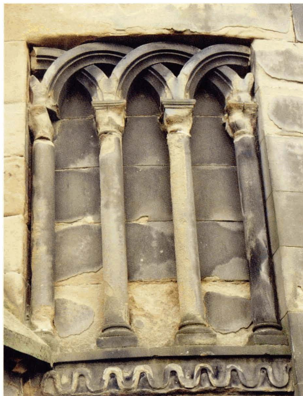
138. Carved detail on sandstone showing significant stone decay
