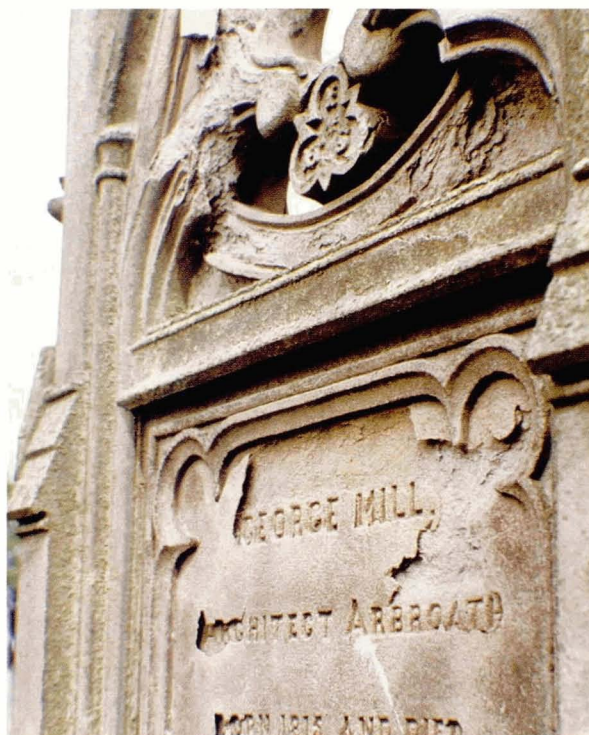
39. Blistering and resultant surface detachment
