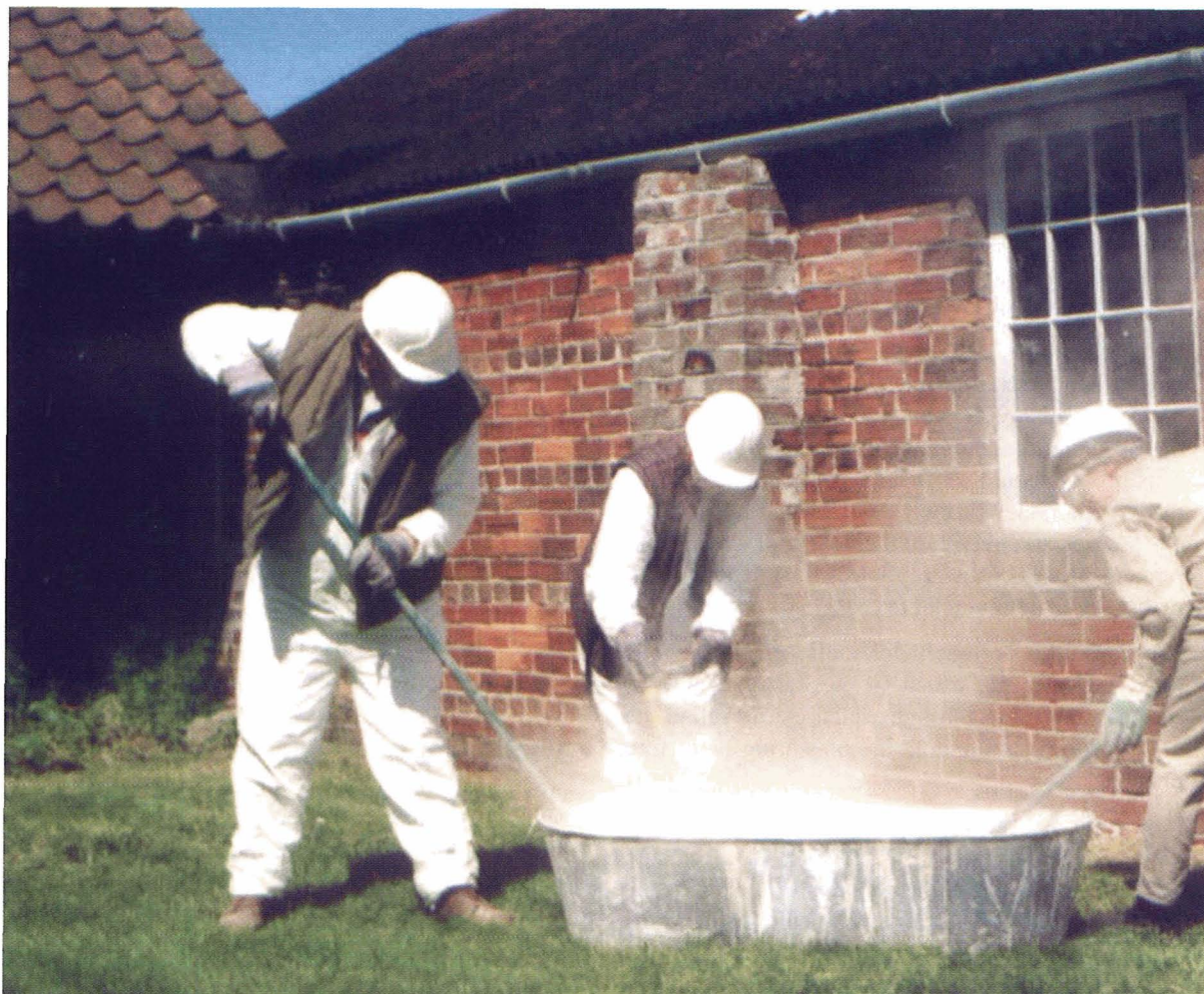
9. Slaking quicklime on site requires at least two people. Appropriate health and safety equipment should always be available. (refer to Appendix D)
