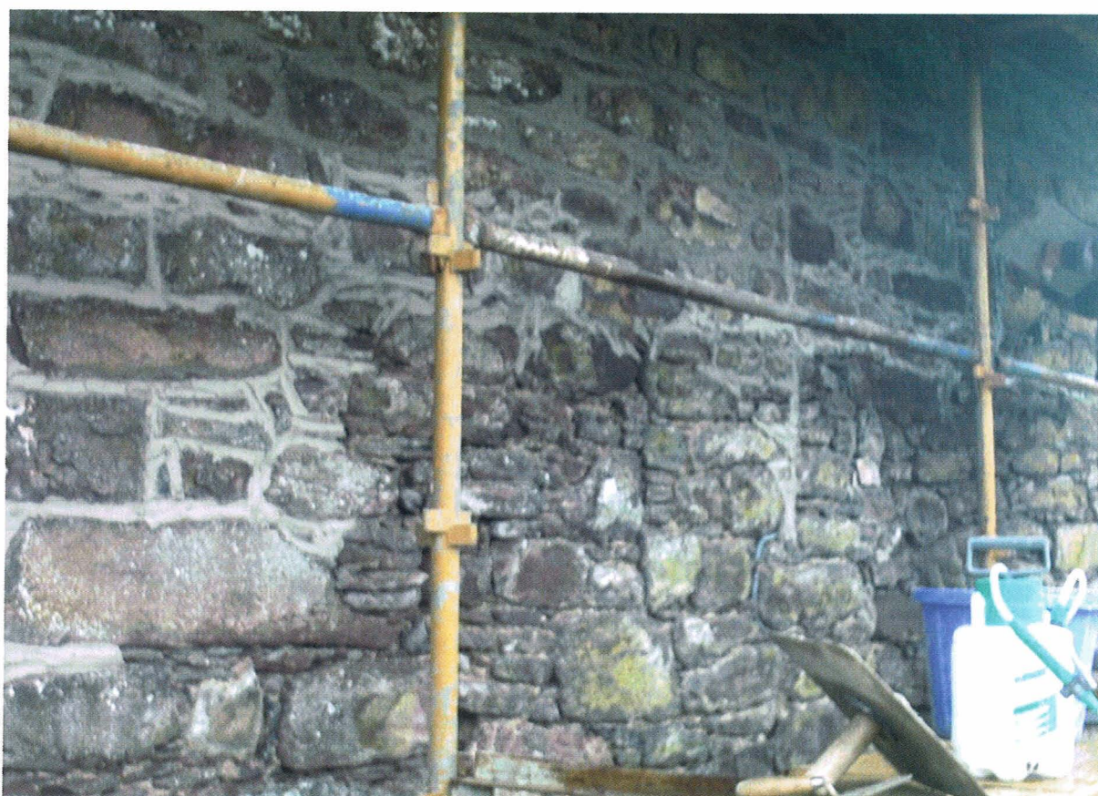
22. Section of rubble wall during repointing. (Lower right) wall prepared to receive lime mortar; (lower left) mortar inserted into joints and compacted and (top) repointing completed - in this example "faired out" to match the local tradition.
