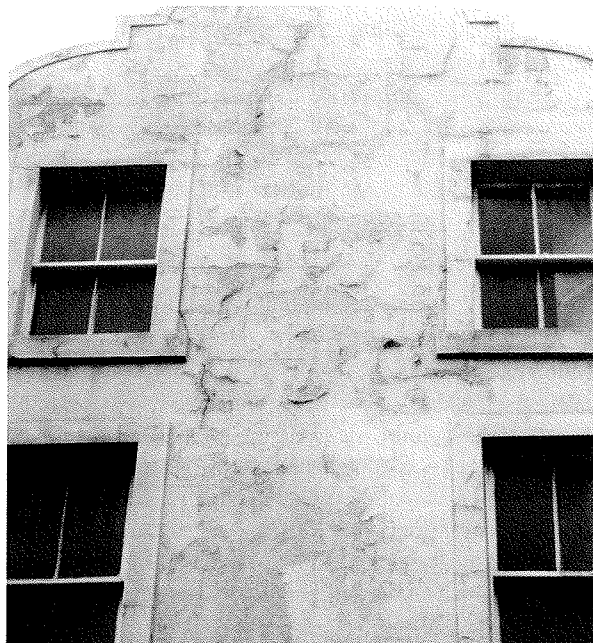
3. Cracking of cement-based render on sandstone masonry.
