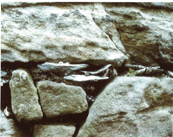
18. Oyster shell pinnings used to level up courses in a sandstone rubble wall.
